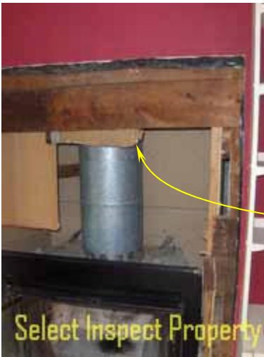
↑ family room fireplace
