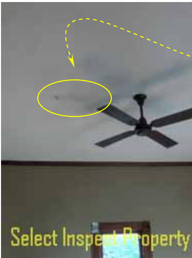
↑ moisture damage at family room; in proximity below upstairs water heater & roof leakage location; may be related
