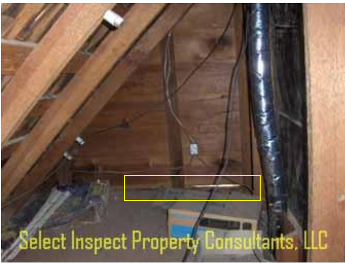
↑ inadequate seal from attic to south bedroom
