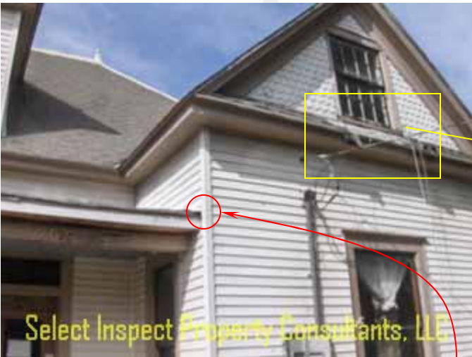
↑ deficient roof, deficient window, deficient flashing
