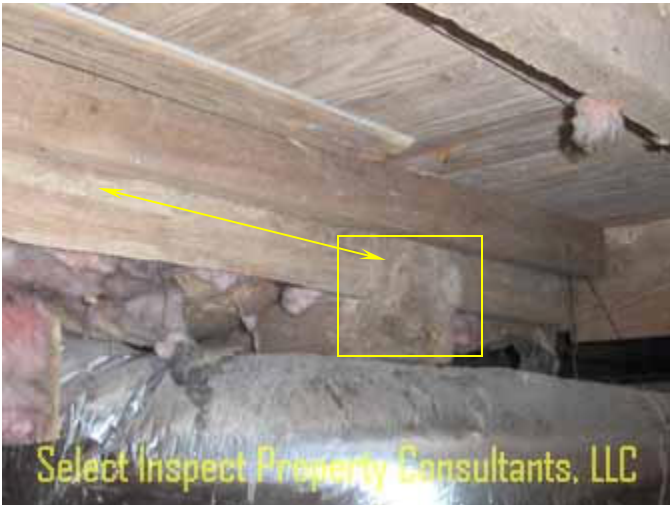
↑ insect damage; crawl space central
