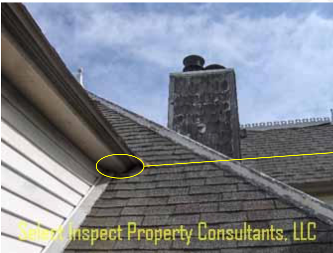
↑ expansive foam, west-southwest dormer
