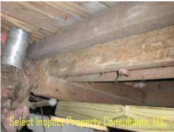
↑ insect damage, newer treated (small 2x4) bracing on wood shims
