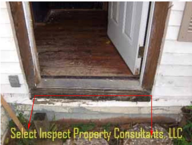
↑ step from door/interior too high; landing not present
