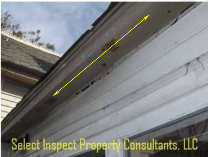
↑ deficient siding & moisture damage at eave; rear
