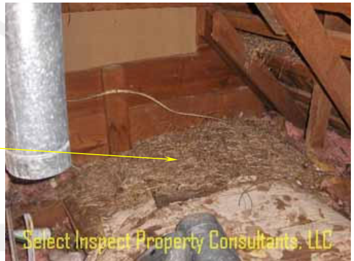
↑ rodent/bird nesting; rodent feces discovered at multiple attic locations.
