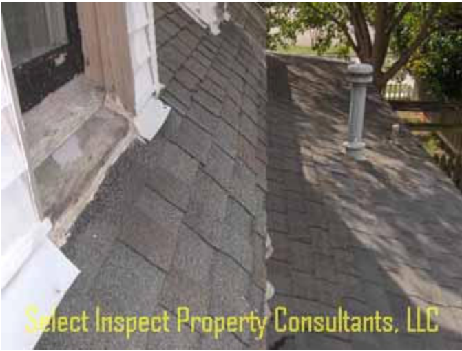
↑ deficient flashing at rear upstairs windows; undetermined flue; variant shingles imply patch/repair history
