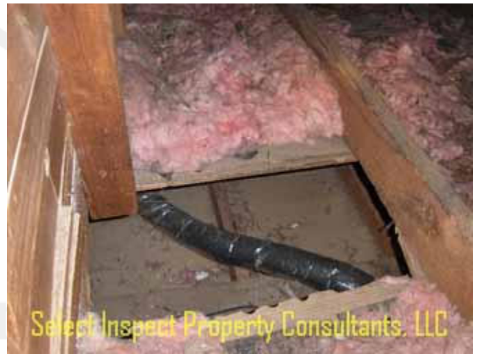
↑ missing insulation; rodent damaged refrigerant pipe insulation; southwest attic
