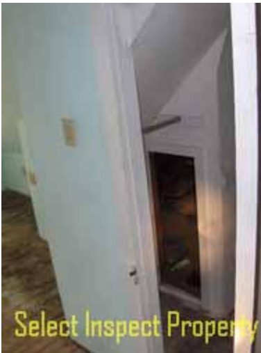
↑ attic access too small; east-northeast
