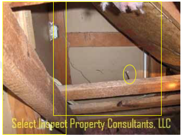
↑ inadequate seal attic to northeast bedroom & deficient insulation
