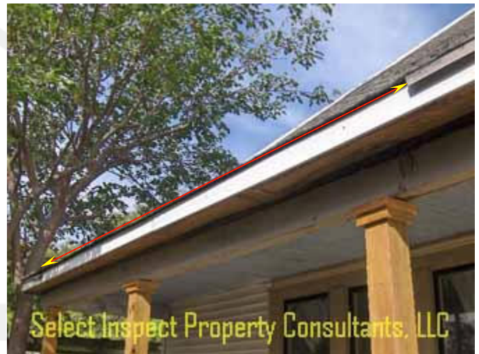
↑ incomplete drip edge flashing; side porch
