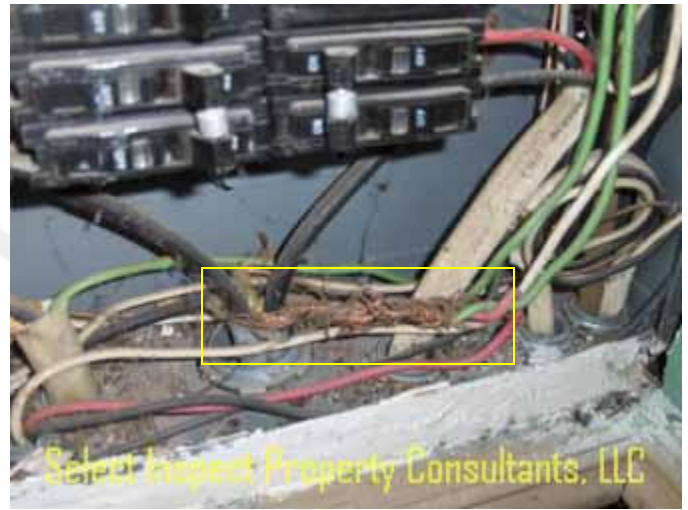
↑ unworkmanlike ground wires; small braided, disheveled; poor connections
