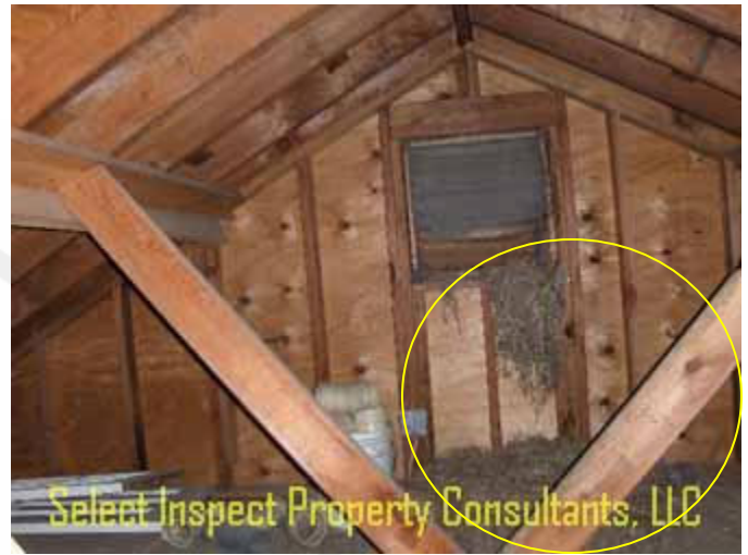
↑ nesting; detached garage attic
