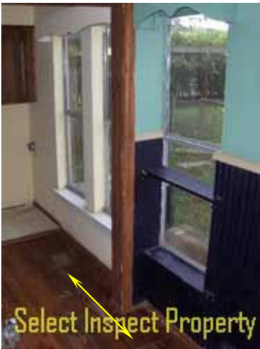
↑ insect damage; laundry room & kitchen hall
