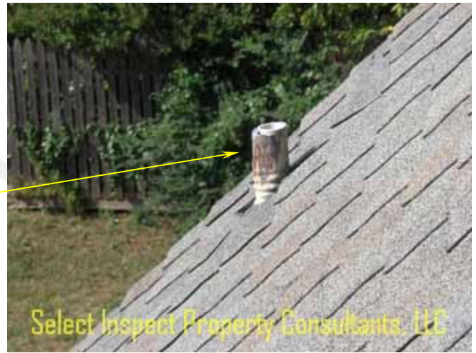
↑ close view of image at left; should be minimum 6" above roof, & lead wrap damaged (rodent)
