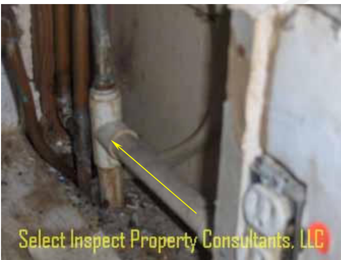
↑ Possible air conditioning primary condensate drain termination? These pipes were too small if they are drains, though may be supply piping (unusual copper / pvc mix); upstairs bathroom south
