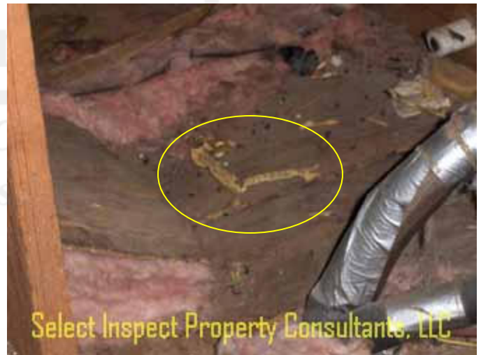
↑ rodent evidence & reversed insulation; upper attic
