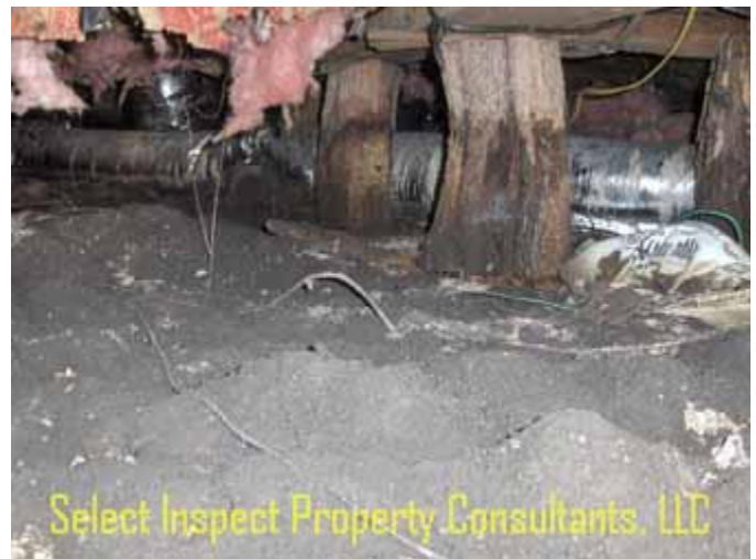
↑ deficient insulation & ducting; crawl space
