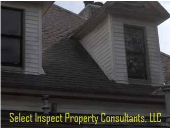
↑ short water heater flue below & in proximity to opening window
