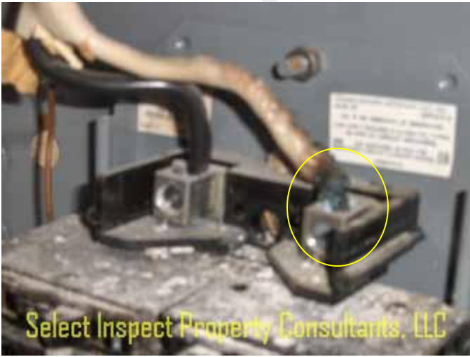
↑ overheating evidence; unsafe; upstairs panel
