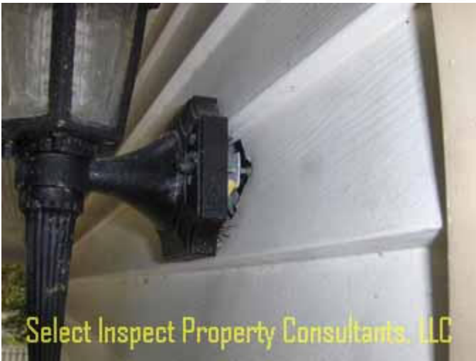
↑ caulking/sealant needed atop exterior lights; example; & Deficient excess reveal
