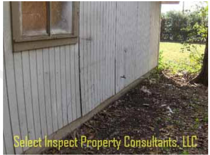
↑ detached garage siding; inadequately secured
