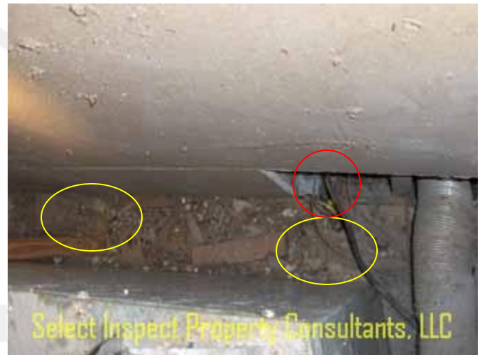
↑ incapacitated rodents & unworkmanlike electrical behind fireplace
