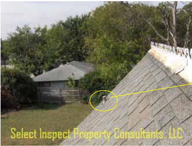
↑ plumbing vent too short
