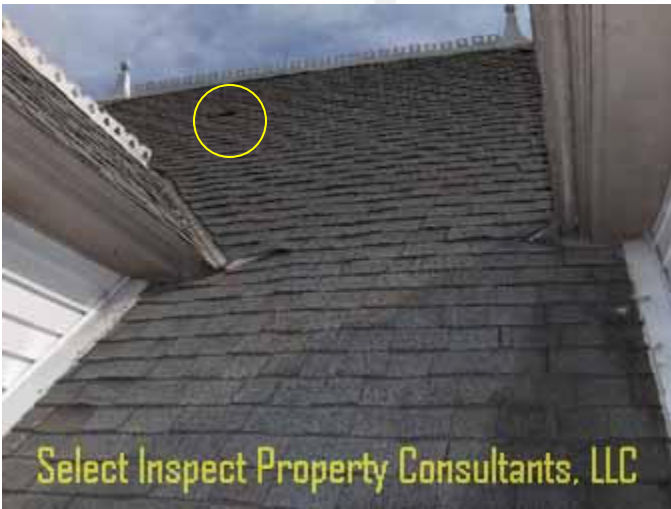
↑ popped nails, & worn shingles; example
