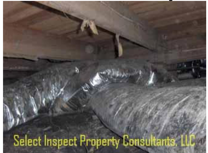
↑ crimped ducting on soil; crawl space
