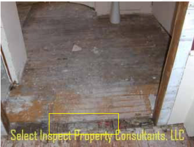
↑ example unstable floor; openings; trip hazards; debris & rodent feces discovered within
