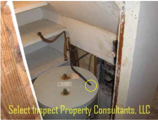
↑ upstairs electrical panel(s) did not have appropriate service clearance, & missing clamp at disconnected h2oh
