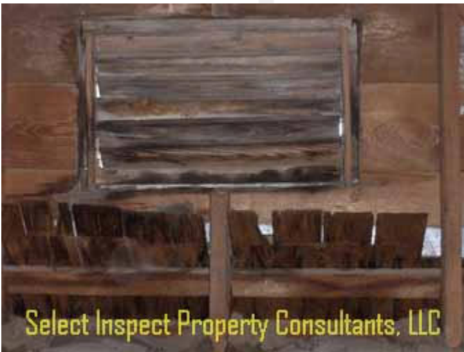
↑ moisture intrusion evidence at dormer/gable vents; example south east
