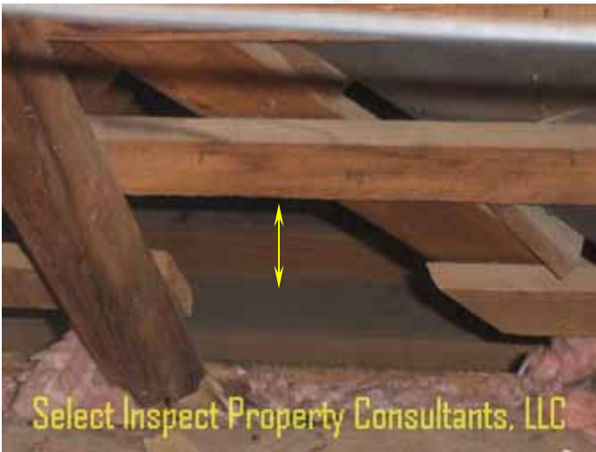
↑ missing insulation above upstairs west-southwest bathroom
