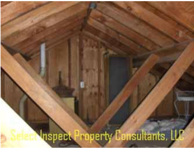
↑ detached garage attic
