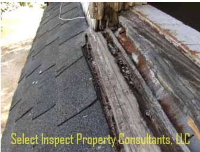
↑ moisture damage & amiss flashing; upstairs north
