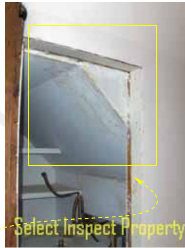
↑ moisture damage upstairs south adjacent the dormer
