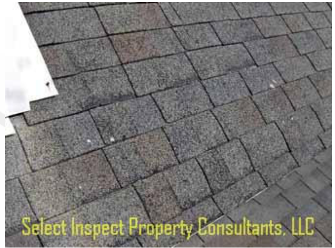
↑ example worn shingles
