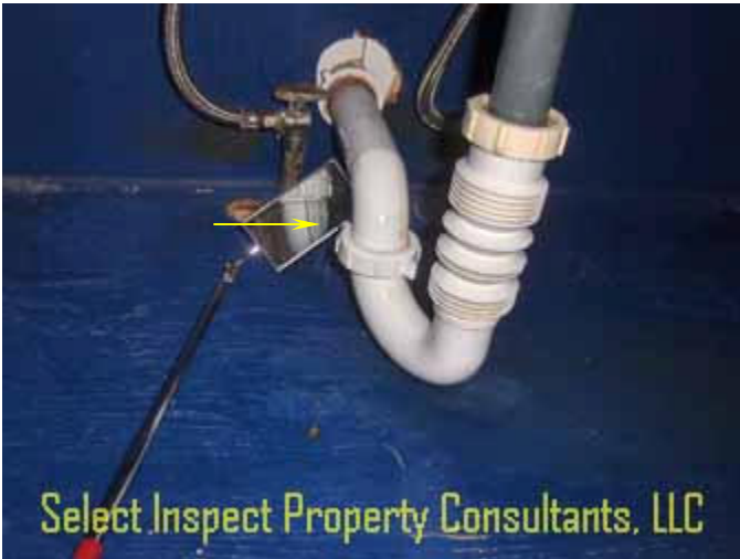
↑ leak at sink drain; flex drain tubing is not recommended; prone to congestion
