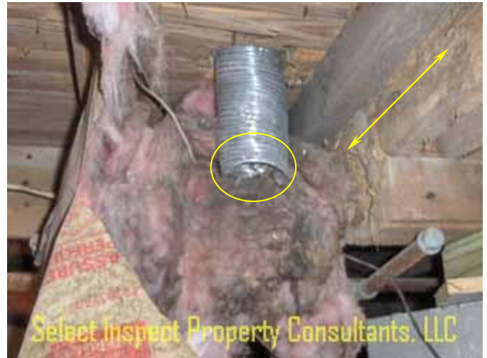
↑ insect damage, deficient insulation, & improper exhaust fan (suspected) termination; crawl space central
