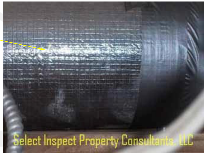
↑ some ducts were routed between ceiling/floor joists; example
