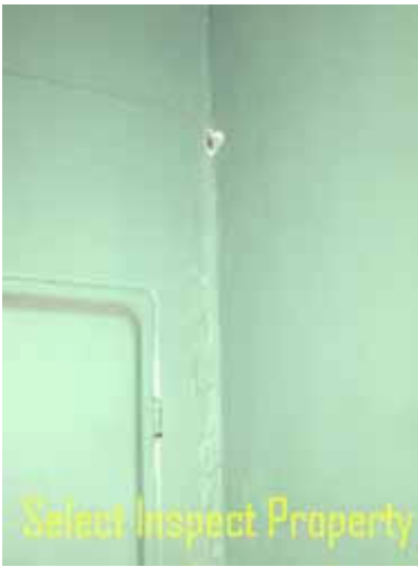
↑ downstairs electrical panel(s) did not have appropriate service clearance; painted panel cover;
