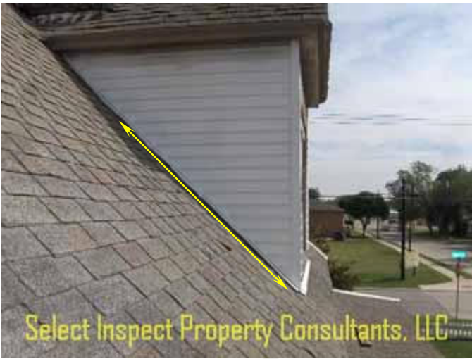
↑ raised flashing; example at south dormer
