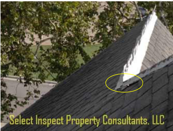
↑ deficient ridge cap north-northeast
