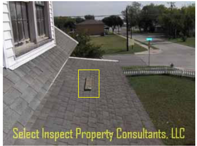
↑ toe board remains at side porch roof; remove & seal holes.
