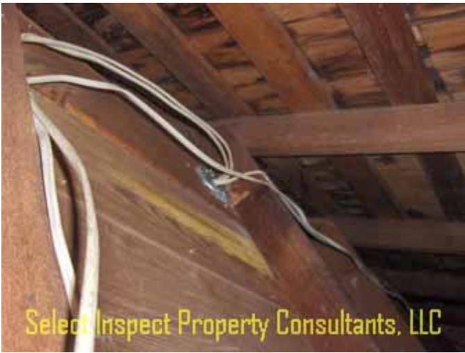
↑ Wires should be secured within 8 inches of junction boxes
