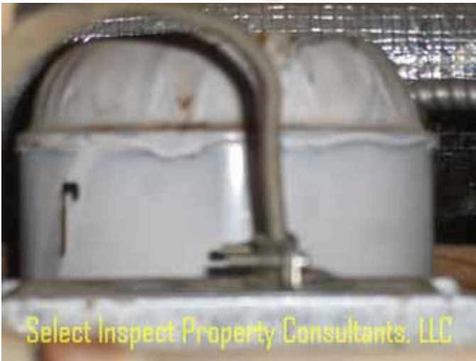
↑ some modern fixtures discovered; this above the downstairs bathroom shower; undetermined if it is rated for wet location.
