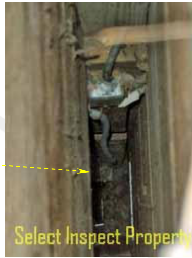
↑ looking down through chase; electrical here & missing continuous flue would make this unacceptable for venting
