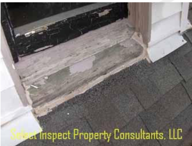
↑ close view of image above; missing flashing at window below sill; heavy sealant implies repair attempts.
