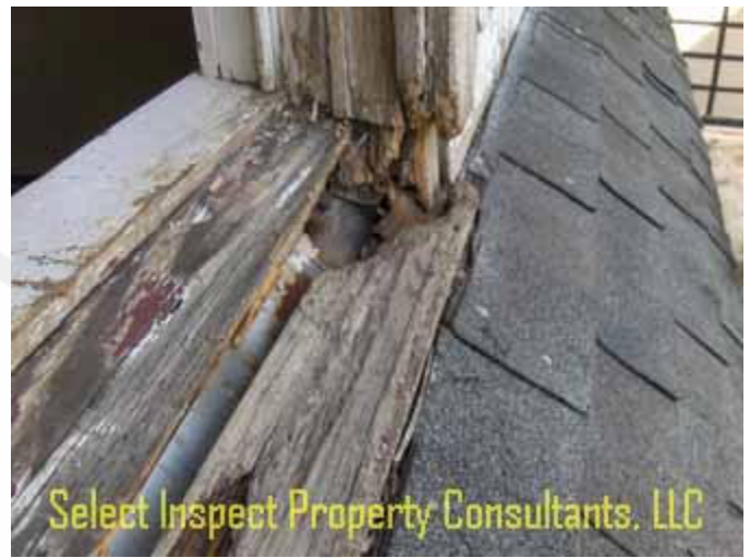
↑ moisture damage & amiss flashing; upstairs north
