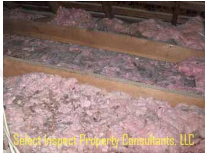
↑ rodent evidence & inadequate insulation; southwest attic
