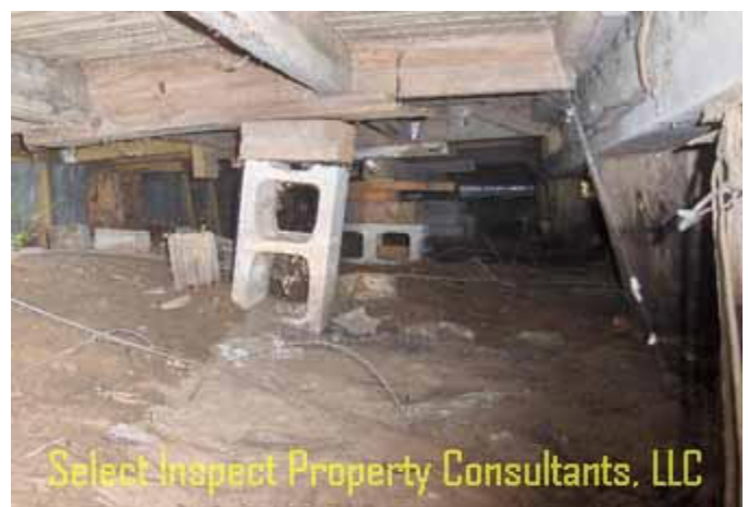
↑ leaning cinder block, should have holes vertical
