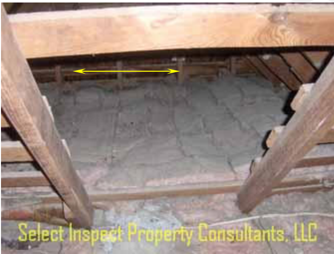
↑ insulation appeared reversed (unless backing is both-sides); & moisture staining at gable
