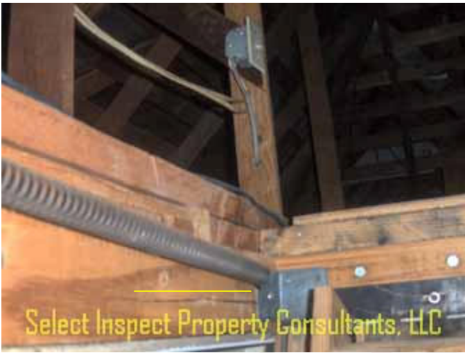
↑ cracked frame of attic stair at home
