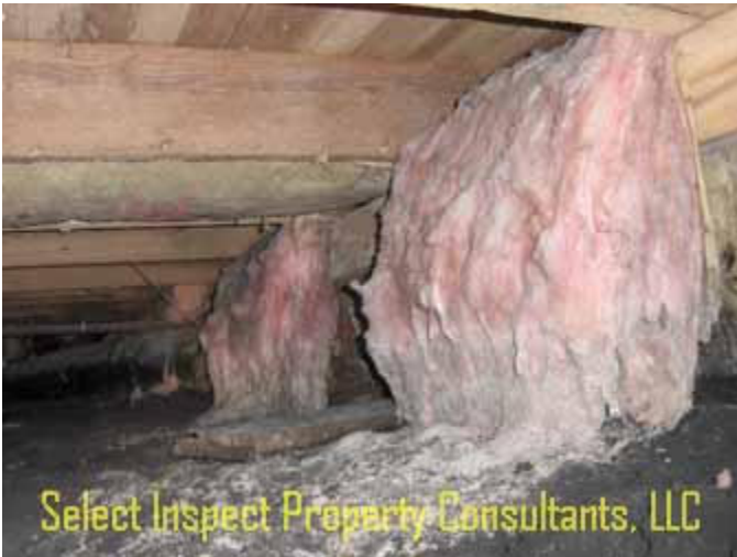
↑ deficient insulation; crawl space
