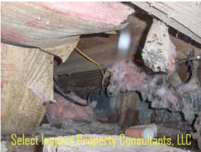
↑ low clearance & crawl space debris; under living room
