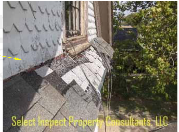
↑ 3 layers of composition/asphalt-type shingles seen here; extremely unworkmanlike cable work
