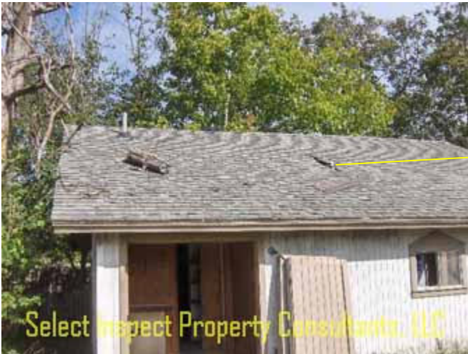
↑ tree damage at detached garage
