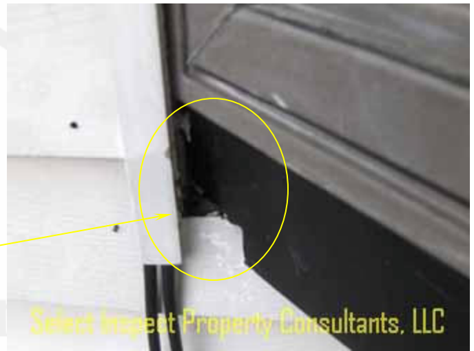
↑ close view of image at left
