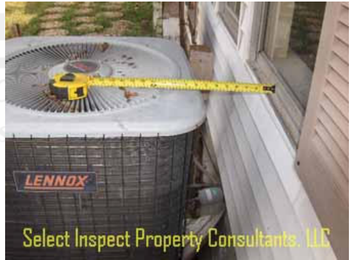
↑ air conditioning condenser(s) did not have adequate clearance; minimum 12" all sides
