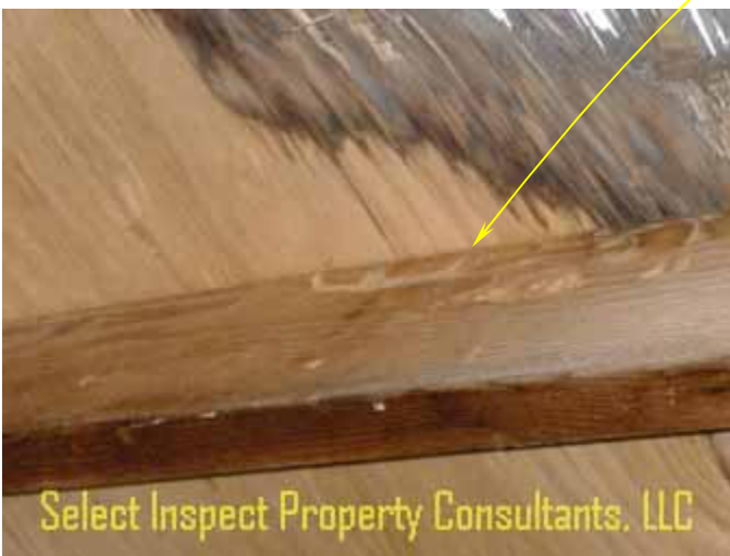
↑ damage from an undetermined wood-boring-insect
