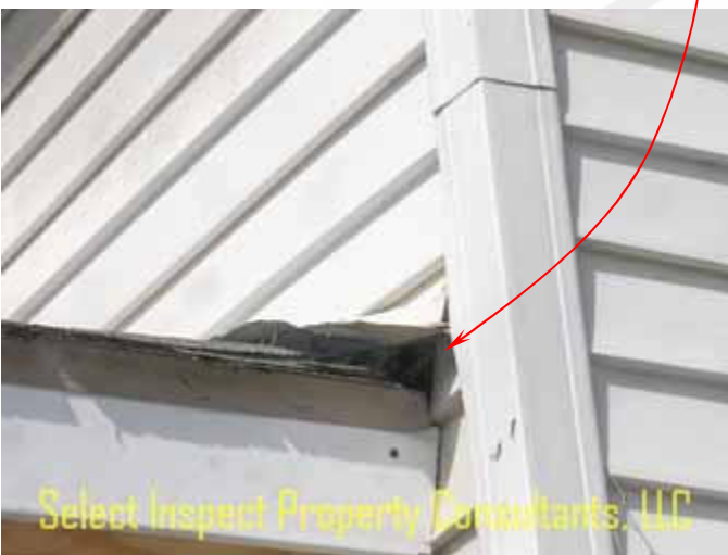
↑ opening may allow moisture intrusion in driving rains; daylight seen from attic
