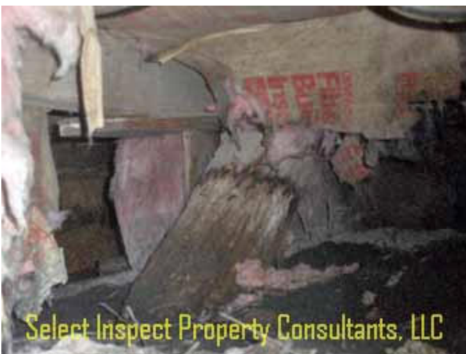
↑ deficient insulation in crawl space
