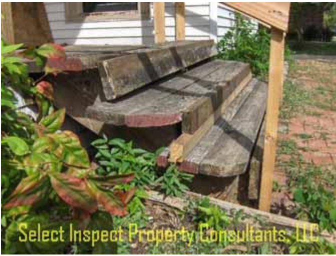
↑ unworkmanlike steps; trip/injury hazard
