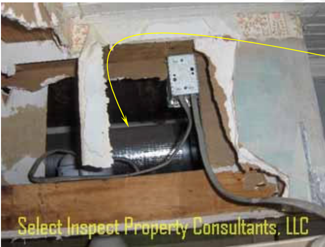
↑ Wires should be secured within 8 inches of junction boxes; above downstairs bathroom shower
