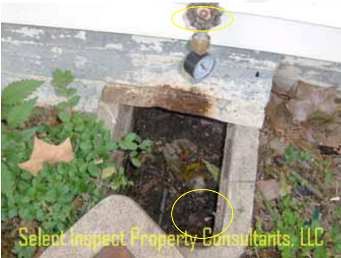
↑ deficient water shut-off-valve
