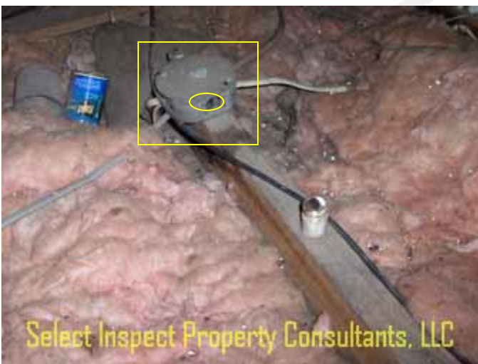
↑ deficient clamping; upper attic electrical
