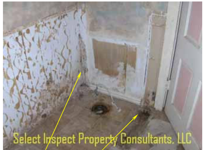
↑ insect damage & moisture damage & fungus downstairs bathroom
