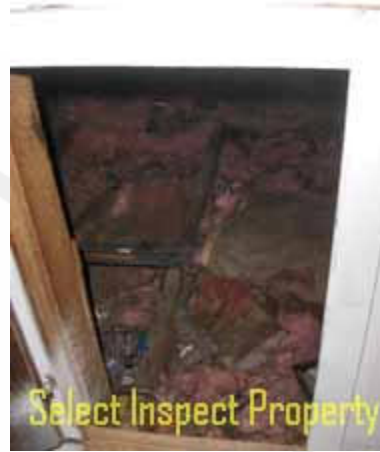
↑ attic access too small; southwest
