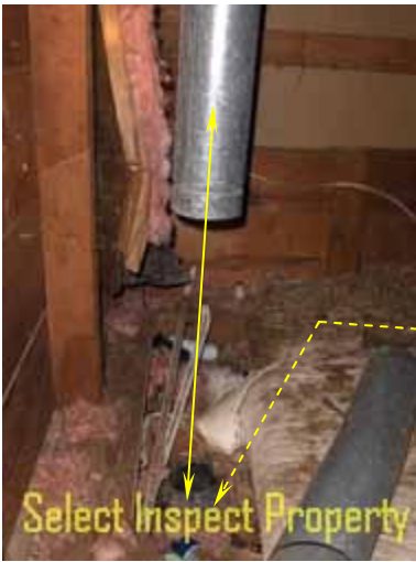
↑ undetermined flue; attic north-northeast
