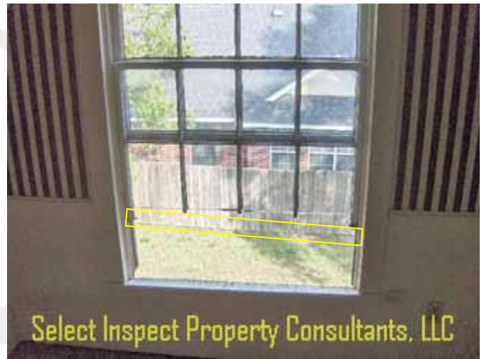
↑ missing window component(s); upstairs north
