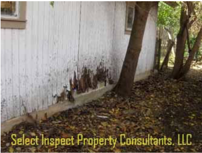
↑ detached garage siding; disrepair
