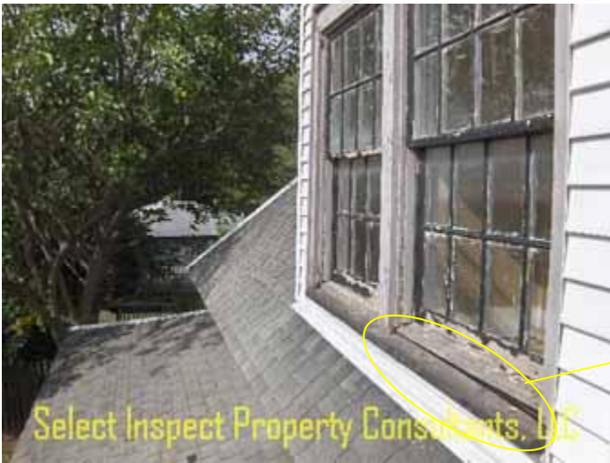
↑ moisture damage & openings; upstairs south
