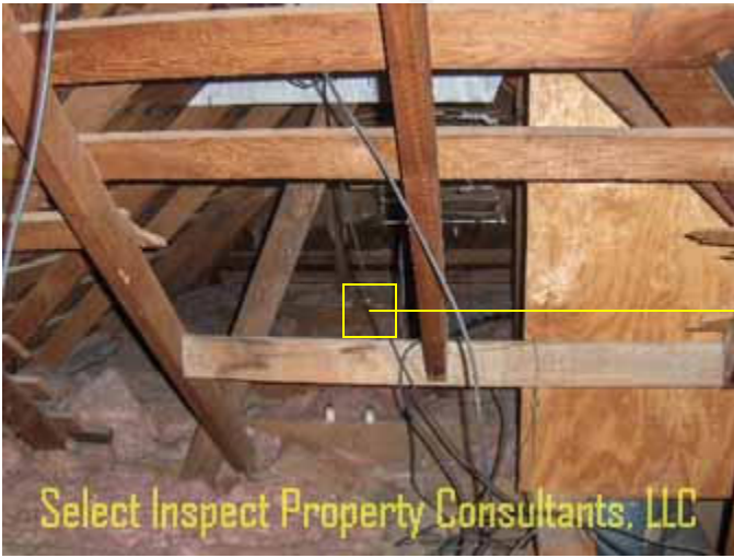
↑ unworkmanlike electrical upper attic south
