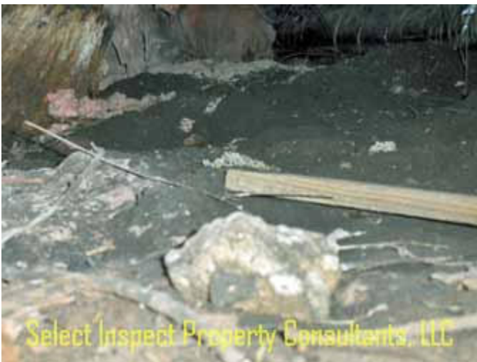
↑ crawl space debris & ducting on soil
