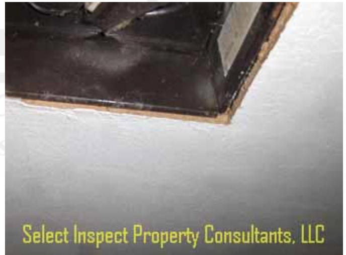
↑ close view of image at left; friable edges at exhaust fan(s) & perimeter may be prone to inhalation
