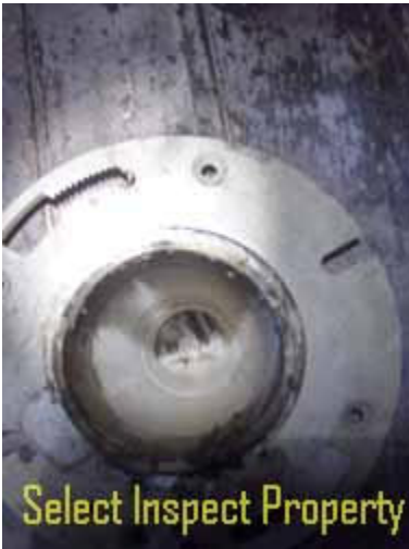
↑ debris present in various plumbing traps; example at toilet trap downstairs
