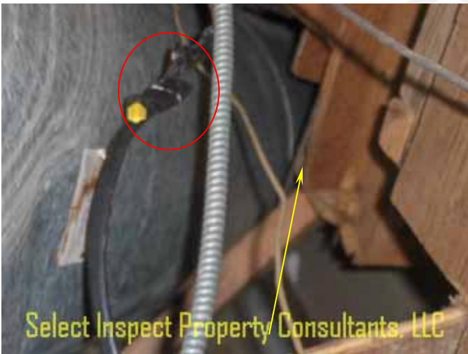
↑ fireplace flue did not meet clearance requirements to combustibles & unworkmanlike unsafe electrical
