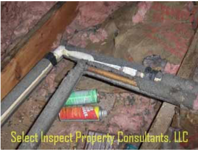
↑ rodent damaged plumbing pipe insulation; southwest attic
