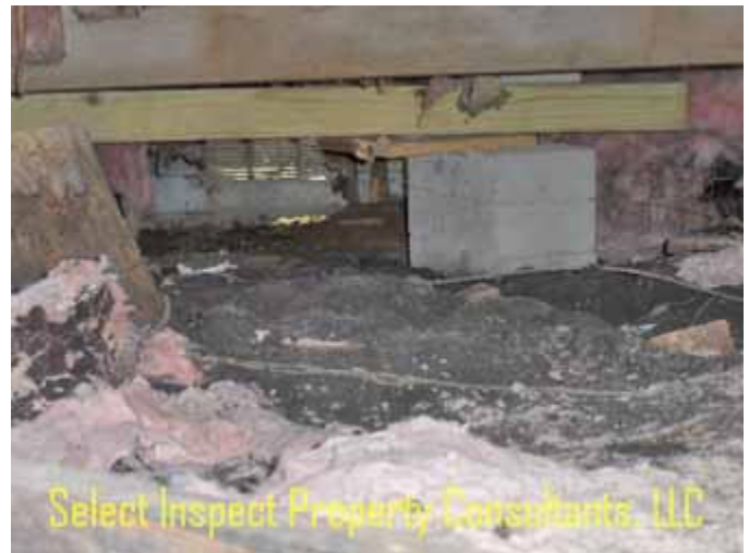
↑ low clearance at south crawl space; wood shims on stack block
