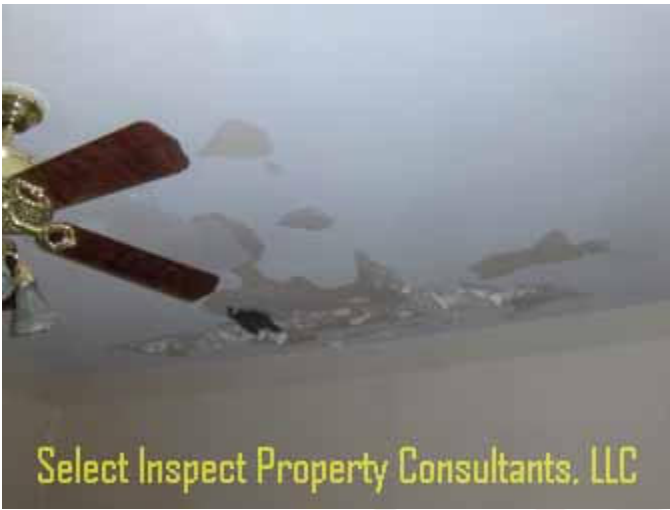
↑ moisture damage at downstairs bedroom
