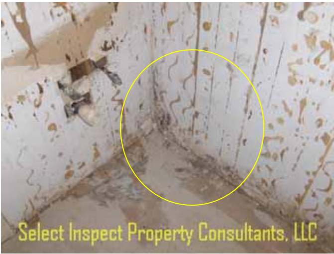
↑ moisture damage & fungus; downstairs bathroom
