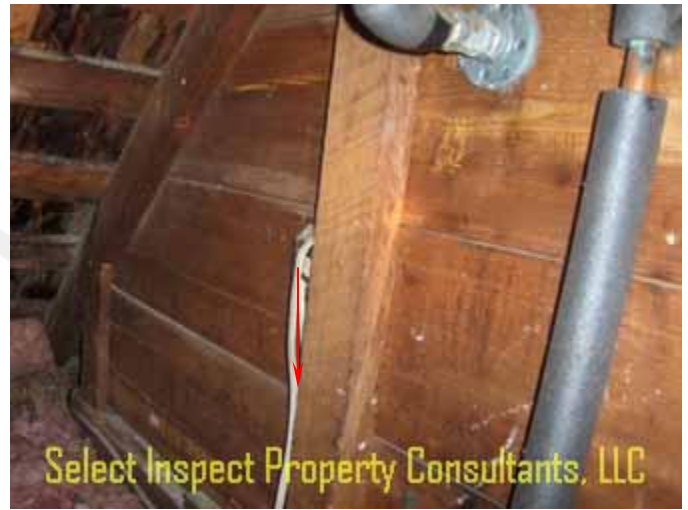
↑ unworkmanlike electrical Wires should be secured within 8 inches of junction boxes; southwest attic
