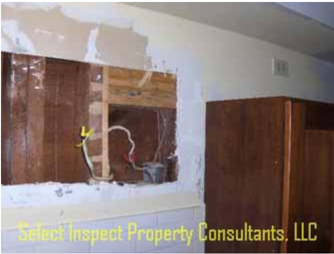
↑ unworkmanlike electrical; kitchen
