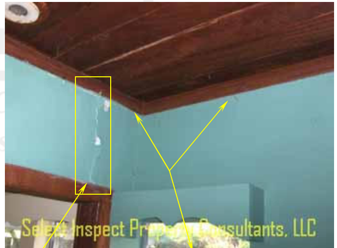
↑ stress cracks/compression, insect damage; laundry room & kitchen hall
