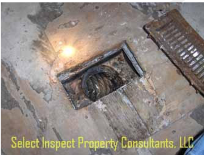
↑ corrosion, unsanitary ducting, damage, inadequately secured floor; example at downstairs bathroom
