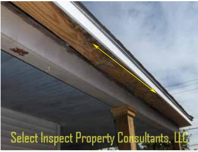
↑ moisture damage at side porch eave
