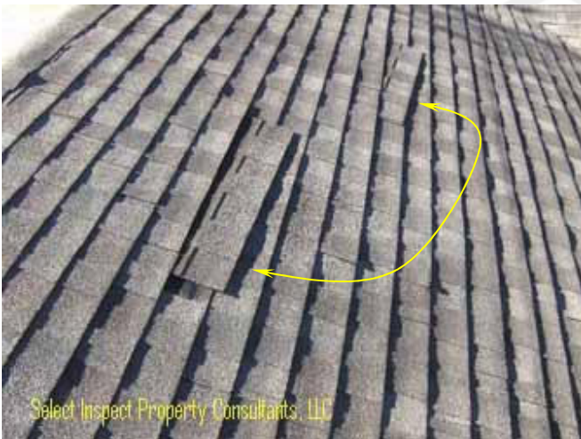
↑ slipped shingles; north exposure(s)
