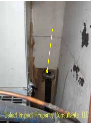
↑ undetermined plumbing pipe in HVAC closet
