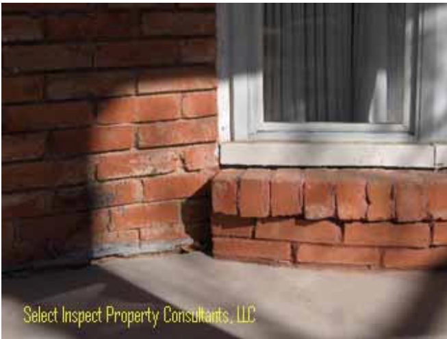
↑ uneven dining room bay window; openings exist
