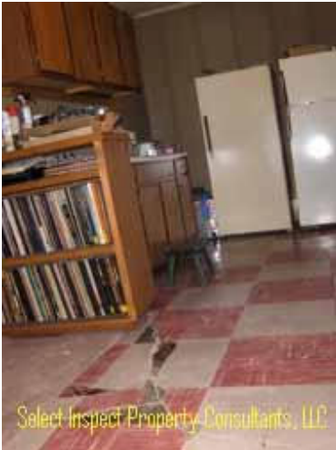
↑ upheaval cracks & other stress at garage conversion
