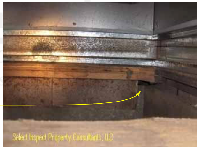
↑ inadequate seal of plenum below HVAC; pulls crawl space air
