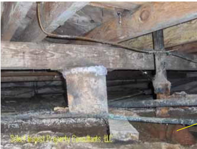
↑ leak below east bathroom & consistent moisture history (salt deposits at pier & muddy soils)
