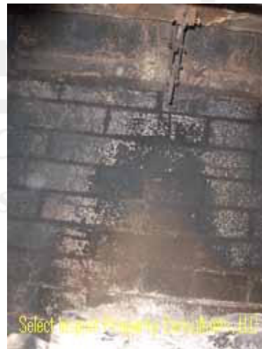
↑ moisture intrusion evidence & cracks at fireplace interior
