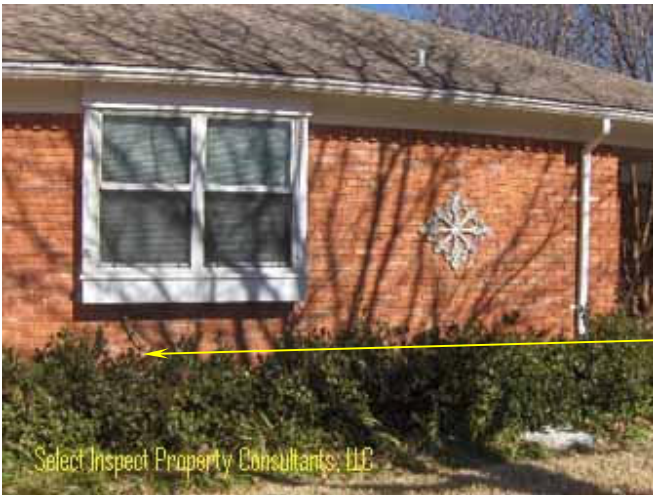
↑ opening & unworkmanlike electrical at front window
