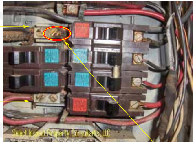
↑ double-tapped service terminals at sub panel; unworkmanlike; overheating evidence at black double tapped terminal; potential fire hazard
