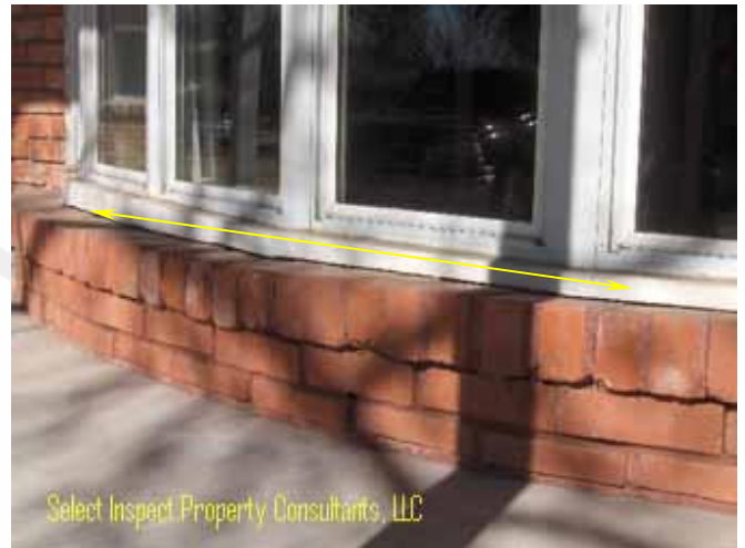
↑ window sill lower at west than east end
