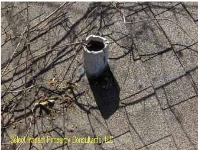
↑ unworkmanlike plumbing vent flashing below shingles; example
