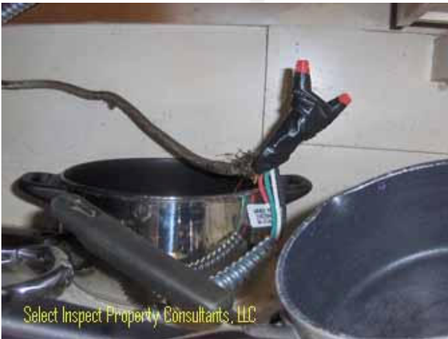
↑ unworkmanlike electrical under stove
