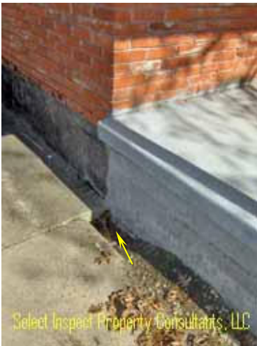
↑ rodent entry point at front porch
