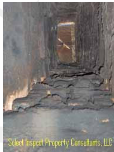
↑ fireplace flue needs professional cleaning & repair
