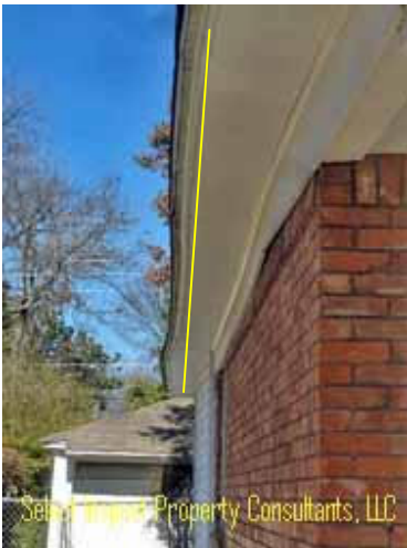
↑ wavy eave at west
