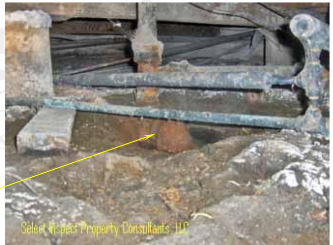
↑ close view of image at left; pooling water
