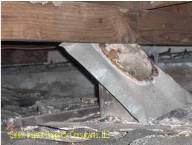
↑ corrosion & inadequate termite shield; example & worn pier; east crawl space
