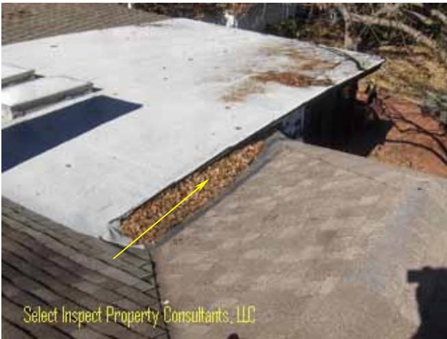
↑ converging valley; inadequate slope; excess tar & debris
