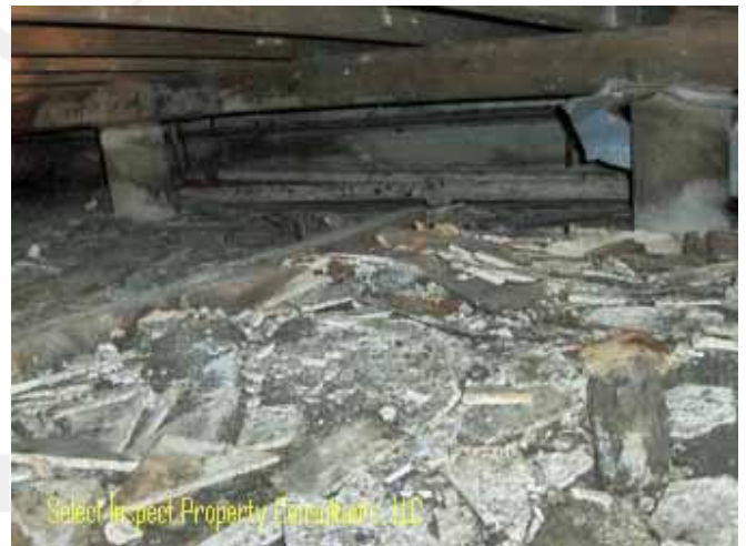
↑ wood debris; example at west side of fireplace foundation; conducive to wood destroying insects
