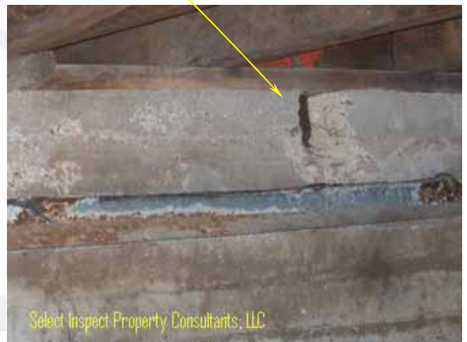
↑ spalling & unsecured anchor; crawl space southwest
