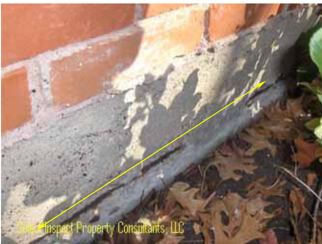
↑ spalling concrete & exposed reinforcement steel at south
