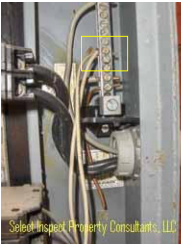
↑ conductors shall be terminated individually in lugs / breakers; main panel outside
