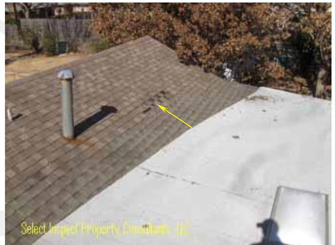
↑ slipped shingles; at east garage conversion exposure(s)
