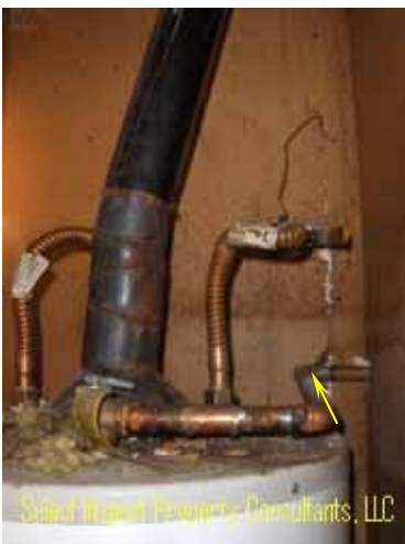
↑ temperature/pressure relief drain improperly routed uphill & moisture damage at flue; suspected moisture damage at interior of burn chamber as well
