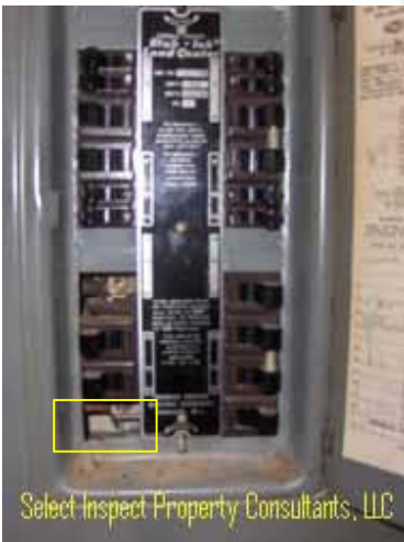
↑ missing knock-outs; example at closet panel
