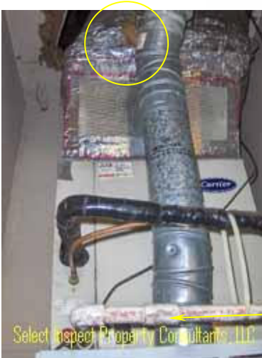
↑ inadequate seal at supply plenum above HVAC & fungus at primary condensate drain
