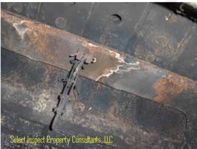
↑ corrosion at damper implies moisture intrusion history
