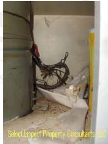
↑ unworkmanlike electrical at kitchen vent
