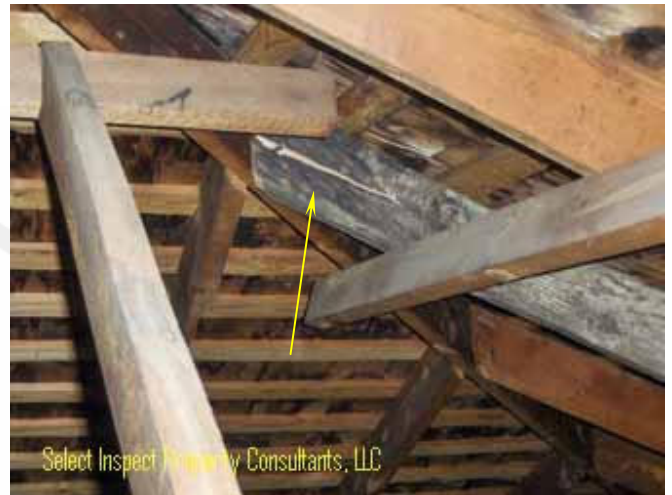
↑ example cracked framing in attic
