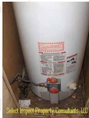
↑ moisture damage below water heater; auxiliary pan should have been installed with this device in 2000
