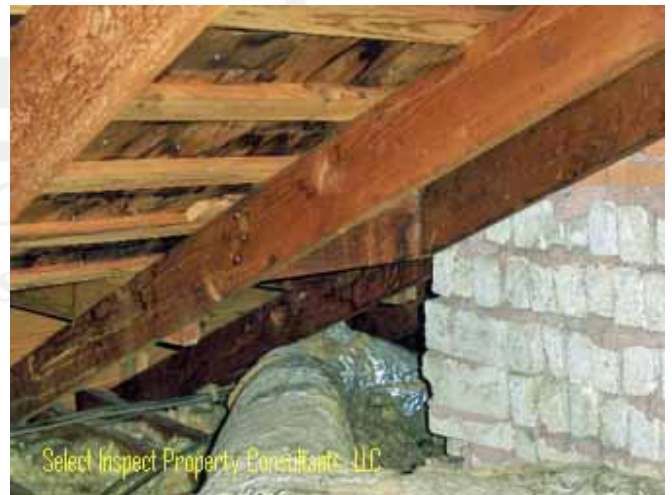
↑ moisture staining adjacent chimney in the attic
