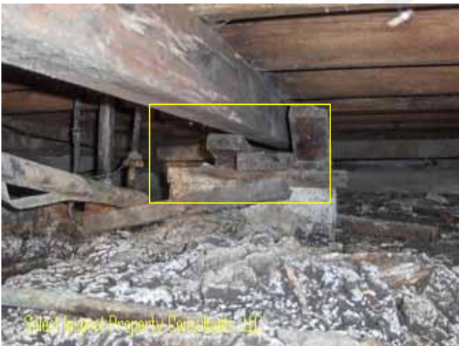
↑ inadequate wood shimming & calcium-like deposits on soil
