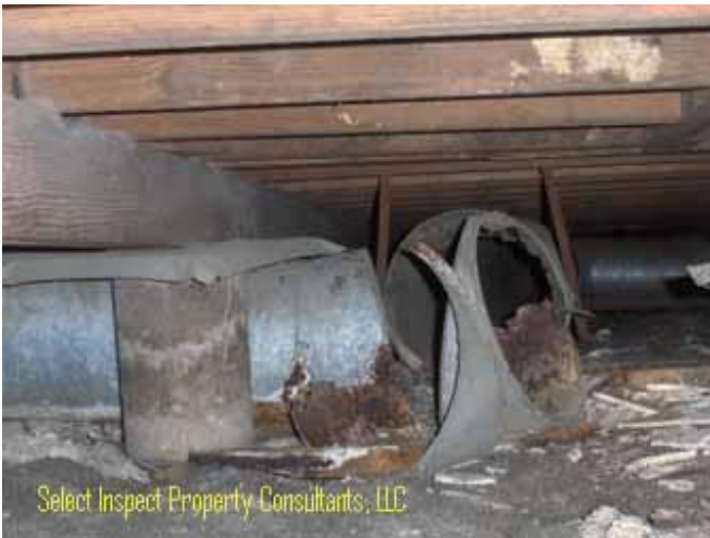
↑ unclean, corroded, disconnect return ducting in central crawl space; disrepair; very unhealthy
