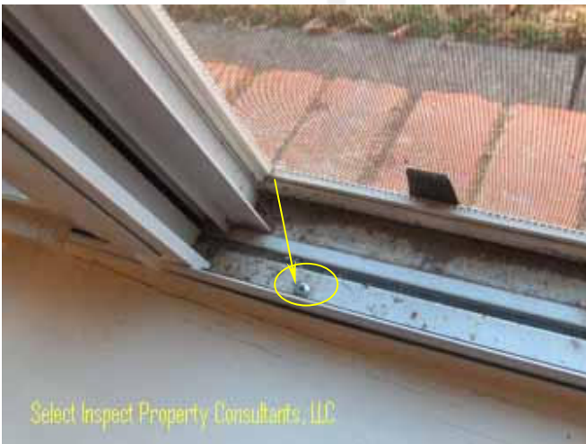
↑ screw at bottom of window is prone to moisture intrusion; unworkmanlike installation; example
