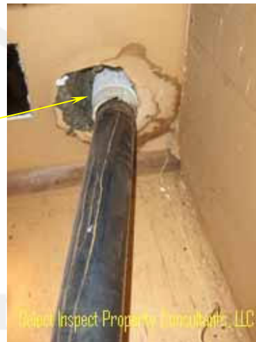
↑ moisture intrusion & corrosion evidence at water heater closet (white section is "transite" pipe)
