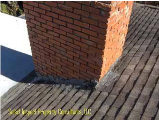
↑ excess tar repair attempt example at chimney
