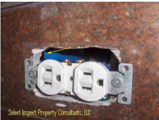
↑ unworkmanlike reveal; example at kitchen receptacle; space between box & back face of backsplash
