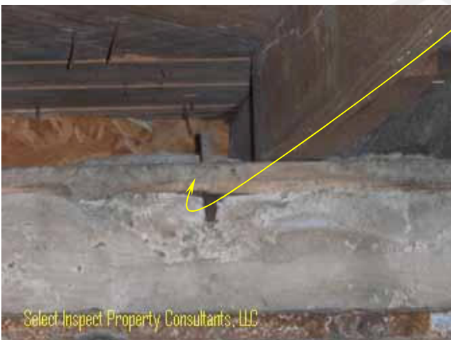
↑ spalling & unsecured anchor; crawl space southwest
