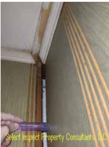
↑ wall stress greater than 1" garage conversion- southwest & western ceiling/wall
