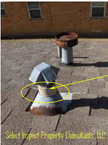
↑ missing rain shield at water heater flue
