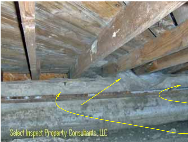
↑ plastic & moisture intrusion evidence below dining room window
