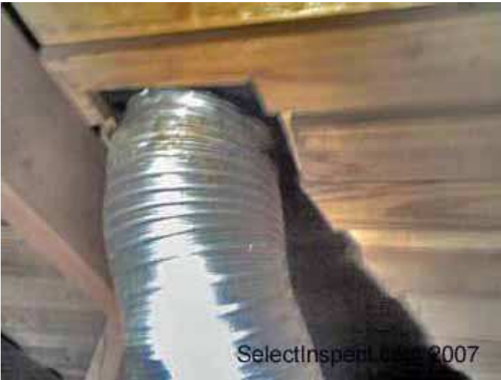
↑ recommend more thorough sealing of kitchen vent at roof penetration- metal tape and or mastic
