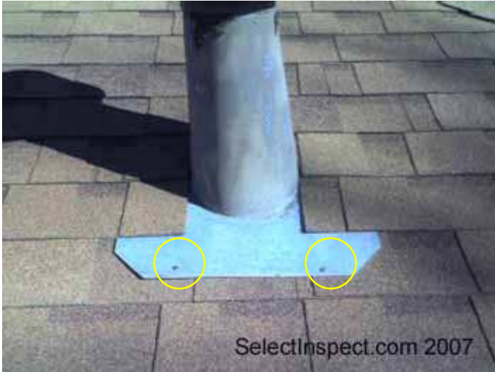
↑ uncaulked fasteners at roof- example
