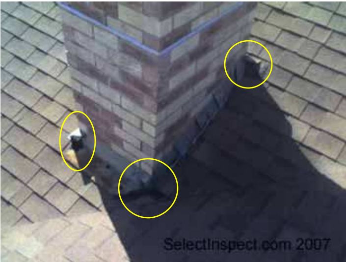
↑ tar repair at chimney flashing
