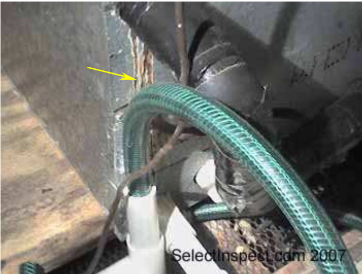
↑ close view of corrosion and leakage history at air-conditioner evaporator
