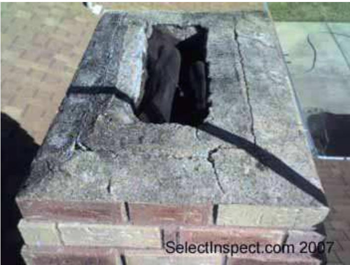
↑ chimney cap needs mortar repair and appropriate ember screen
