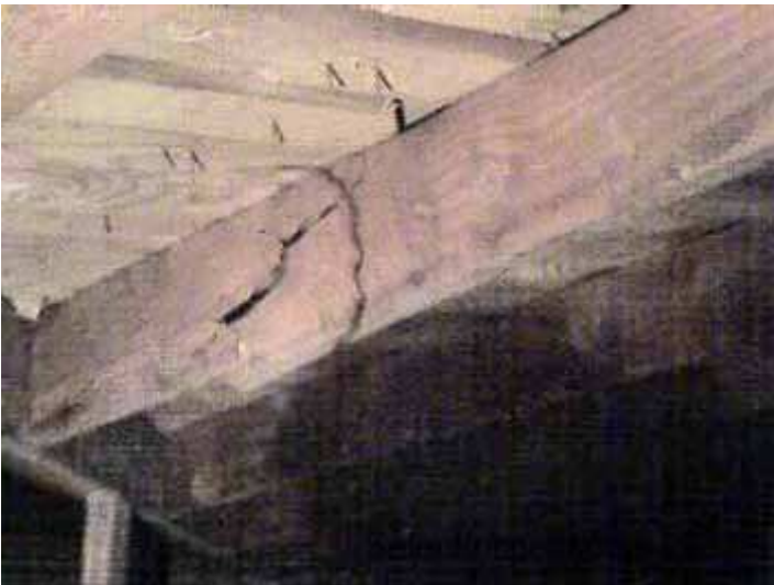
↑ failed rafter at northeast attic –left
