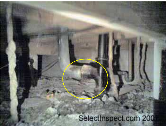
↑ leakage and moisture discovered below hall bathroom toilet
