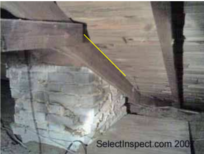
↑ moisture staining/evidence at chimney – attic
