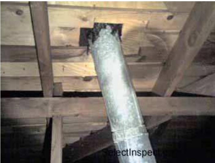
↑ furnace- flue does not meet listed clearance ratings from combustible materials; tar repair history and current leakage
