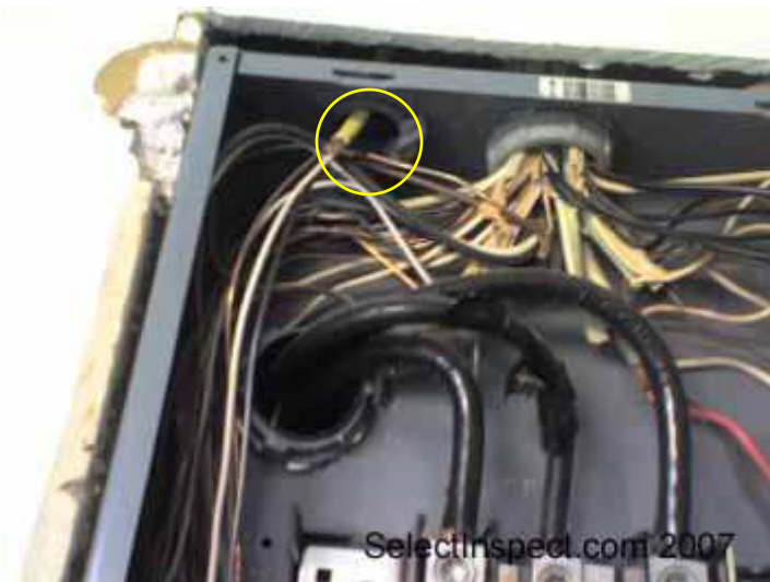
↑ unsealed opening at electrical panel
