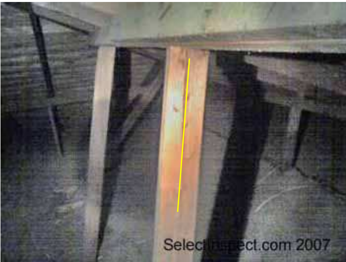
↑ cracked strut at south-southeast attic
