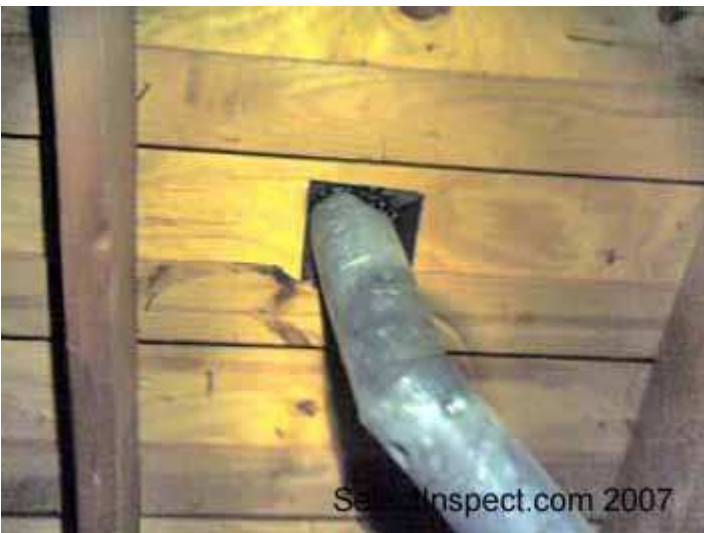
↑ water heater- flue not meeting wood clearance requirements
