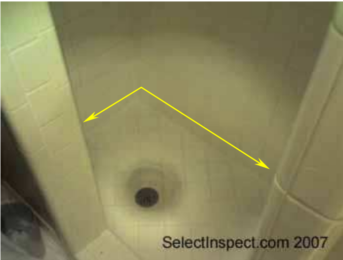
↑ cracked perimeter at master shower tiles
