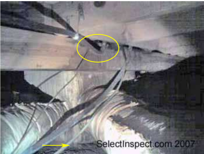
↑ crimped primary condensate line and plenum/duct components not raised 4 inches above soil- below HVAC (crawl space)
