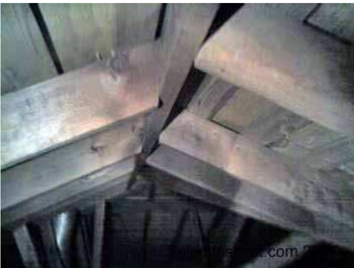
↑ offset rafters and undersized ridge example in attic
