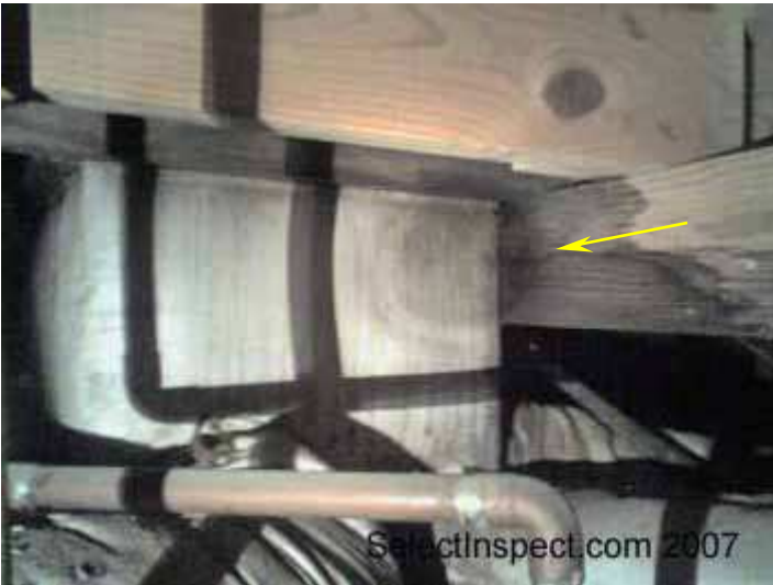
↑ moisture staining/evidence below HVAC (crawl space) and fungus on air plenum components
