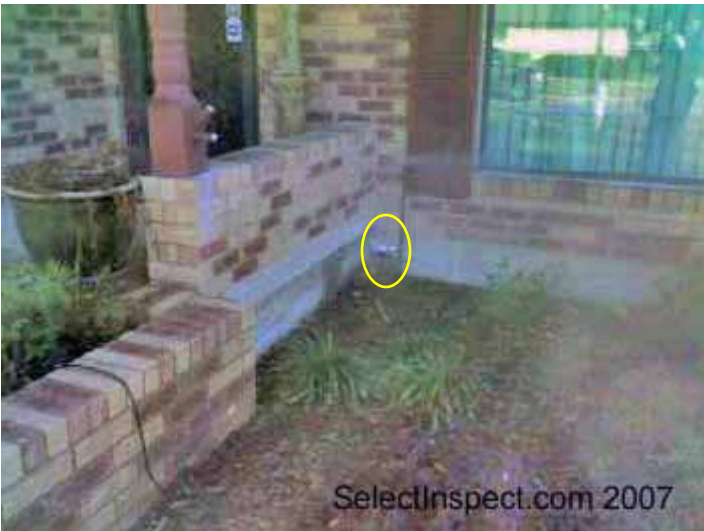
↑ small leak discovered at irrigation connector, adjacent front porch- zone 4
