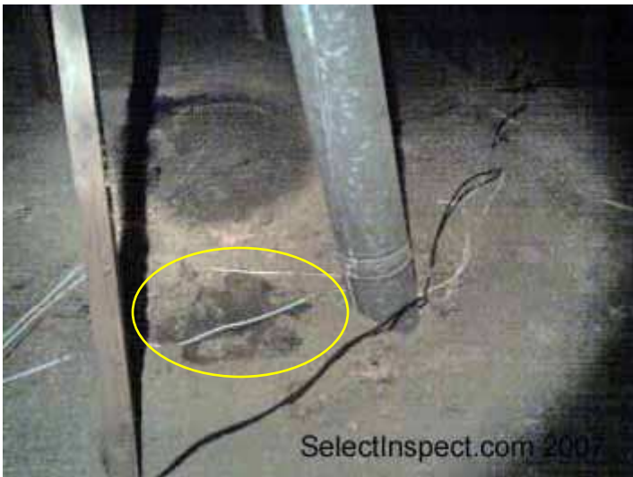
↑ wet, moisture damaged insulation adjacent furnace flue
