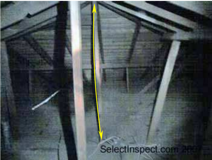
↑ "T backs" not present and deflected struts in central east attic
