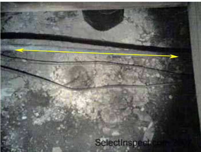
↑ air-conditioner refrigerant line not insulated at crawl space
