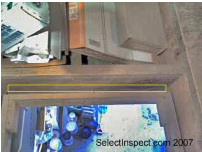
↑ unworkmanlike connection of attic ladder to footer
