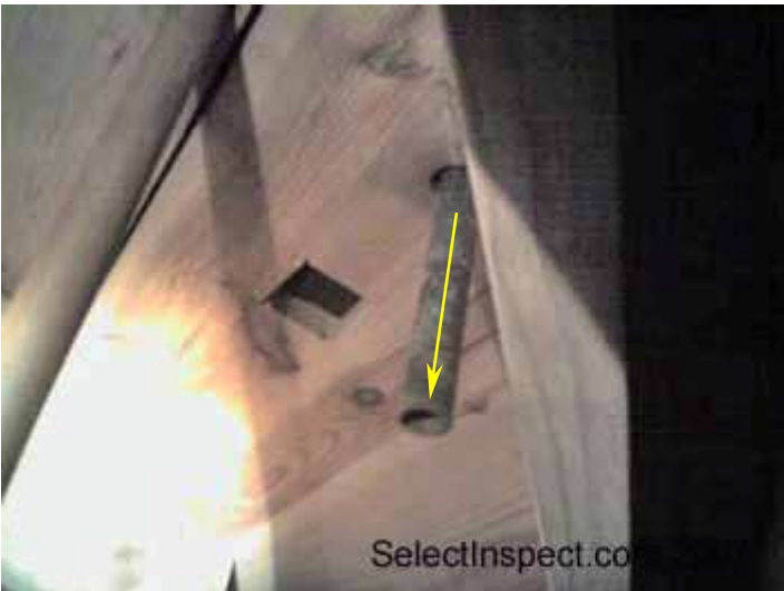
↑ water heater temperature-pressure-relief improperly terminates in the crawl space
