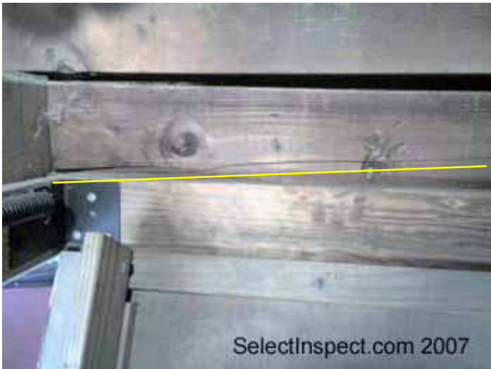
↑ failed and poorly secured header at attic ladder
