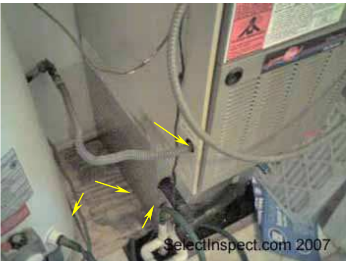
↑ flexible gas pipe unprotected at furnace cabinet penetration; no pan under water heater; HVAC resting on deflected plywood; leakage (corrosion) evidence at air-conditioner evaporator
