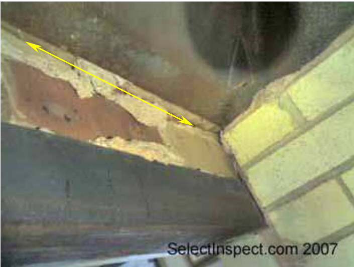
↑ poor mortar seal at smoke shelf- fireplace
