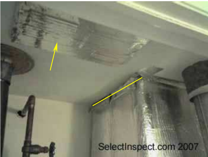
↑ sealed mechanical closet fresh air port and amiss / deficient tape joints at HVAC
