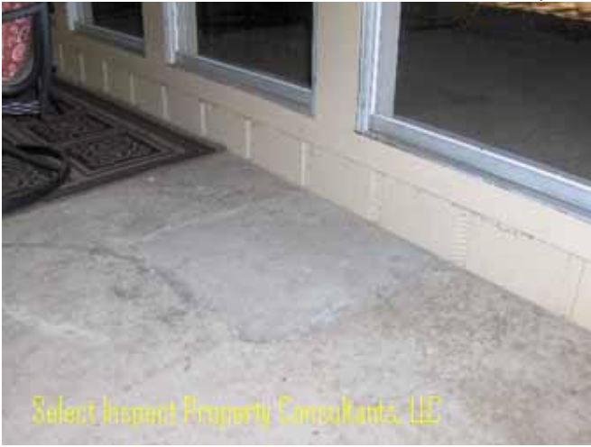
↑ low siding obstruction & pier location; example at rear porch
