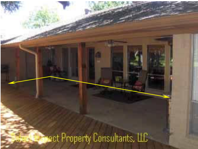
↑ rear porch roof is on separate foundation from the home
