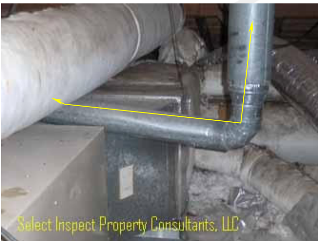
↑ unworkmanlike negative slope; inadequately secured furnace flue
