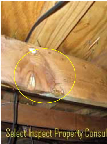
↑ cracked rafter at knot; example
