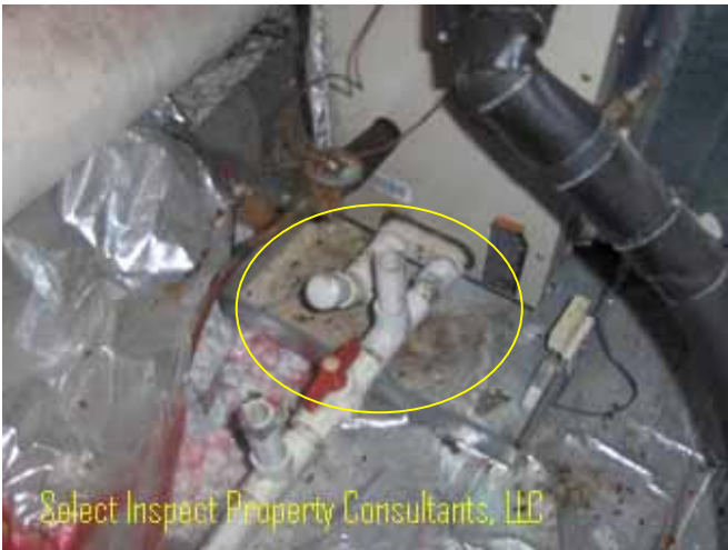
↑ leakage history at evaporator(s) auxiliary pan; monitor
