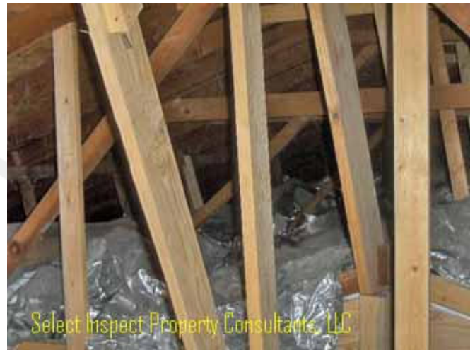
↑ east & southeast attic not readily accessible; "newer" framing seen above the family room
