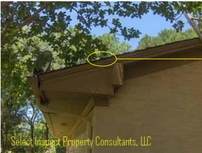
↑ inadequate lap at drip edge flashing; southeast
