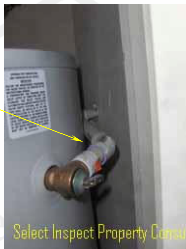
↑ improper piping, routed uphill, & improper termination
