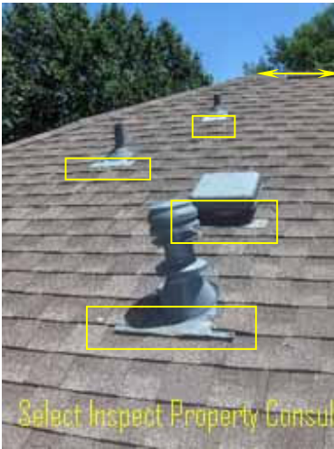
↑ lifted flashing and uncaulked, exposed fasteners locations
