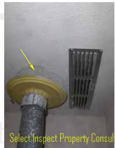
↑ moisture staining, incorrect flue material, & screened vent
