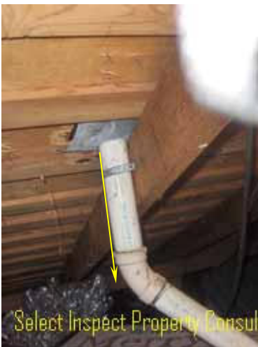
↑ leakage history at laundry room plumbing vent
