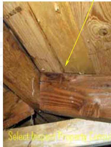
↑ close view & undersized ridge example & moisture staining
