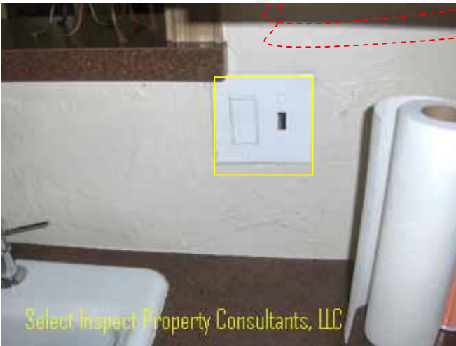
↑ Deficient excess electrical reveal at kitchen; incorrect cover plate
