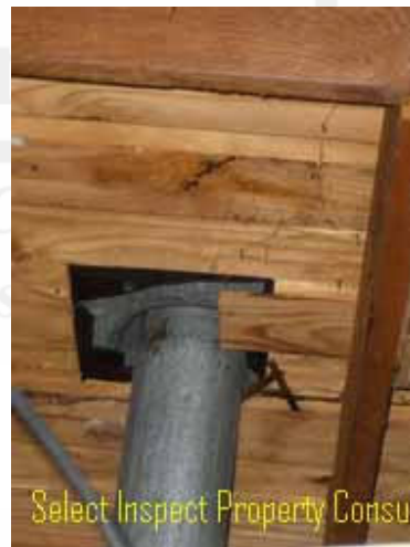
↑ HVAC flue did not meet clearance requirements to combustibles
