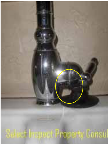
↑ kitchen sink leaks when operated
