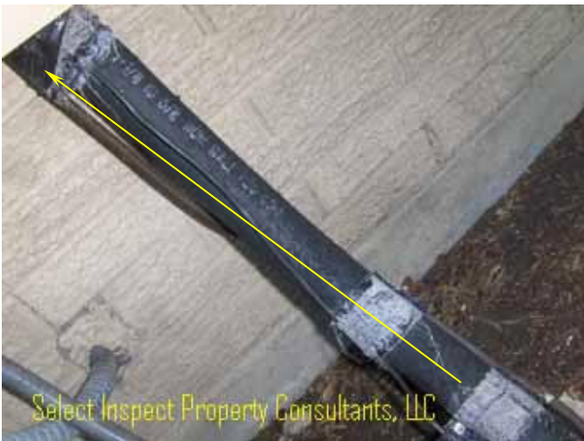
↑ damaged refrigerant insulation; rodent entry point to attic-exterior north
