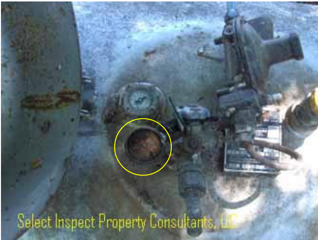
↑ damaged gauge at propane tank
