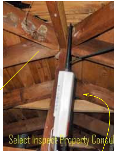
↑ cracked rafters example
