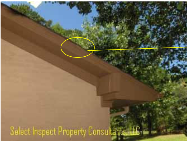
↑ inadequate lap at drip edge flashing; northeast
