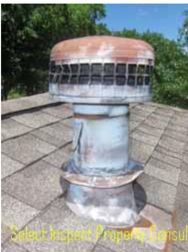
↑ damaged HVAC flue
