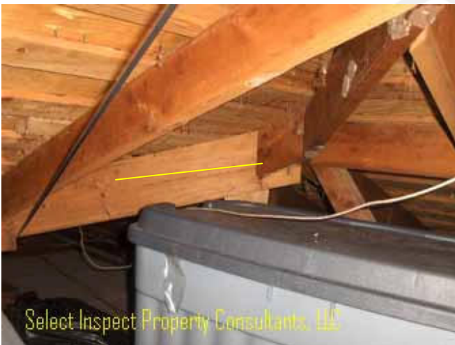
↑ cracked rafter example
