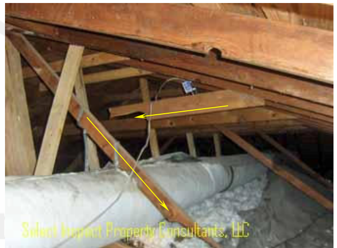
↑ cut/broken strut & collar tie over family room
