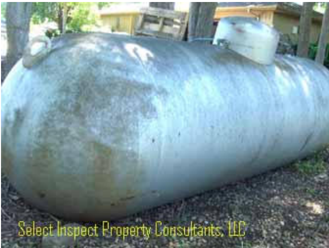
↑ some surface rust seen at visible areas; recommend rust inhibitive paint & consider raising off soil to extend service life of the tank.
