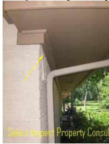
↑ frieze-board separation at the northeast
