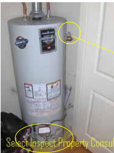
↑ multiple deficiencies at both water heaters; example at hall unit
