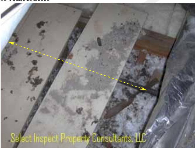
↑ attic floor partially supported on gas piping- northwest of family room
