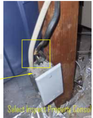
↑ unworkmanlike, missing sheathing
