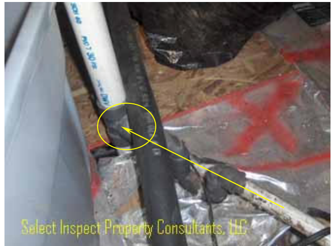
↑ primary condensate drain terminates at plumbing vent
