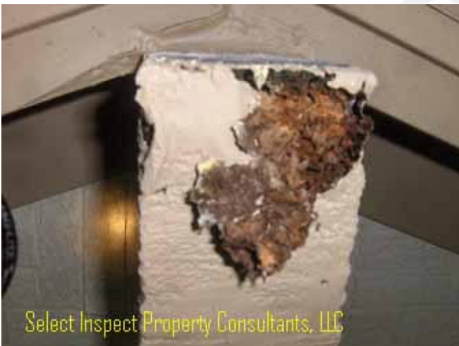
↑ moisture damage & fire ants at southeast beams
