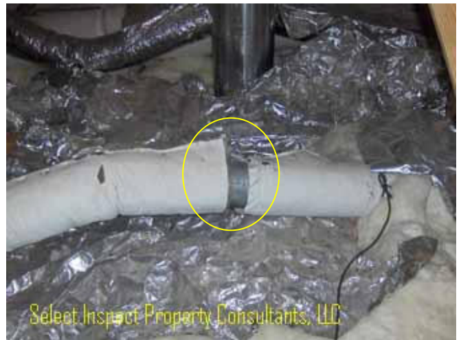
↑ energy loss at air ducting; inadequate insulation & seals
