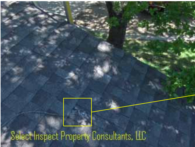
↑ delaminated shingle; southeast
