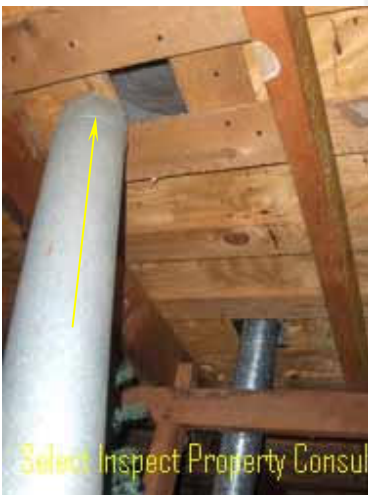
↑ deficient exhaust fan termination (& unclean screen) & garage water heater flue did not meet clearance requirements to combustibles
