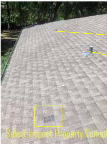
↑ delaminated shingle & plumbing vent(s) was shorter than required
