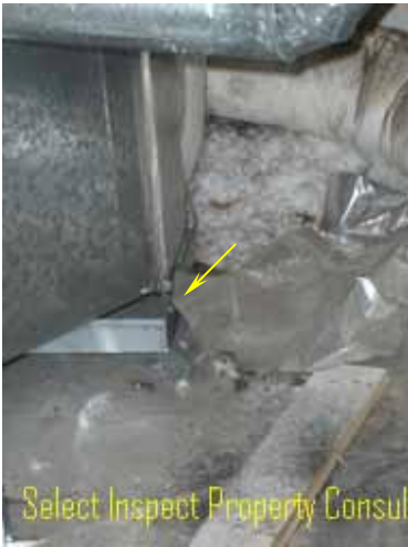
↑ improper alignment of evaporator(s) auxiliary pan
