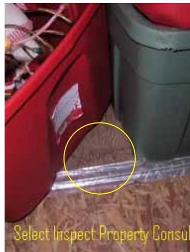
↑ moisture staining below vent penetration
