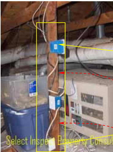
↑ multiple deficiencies at attic electrical
