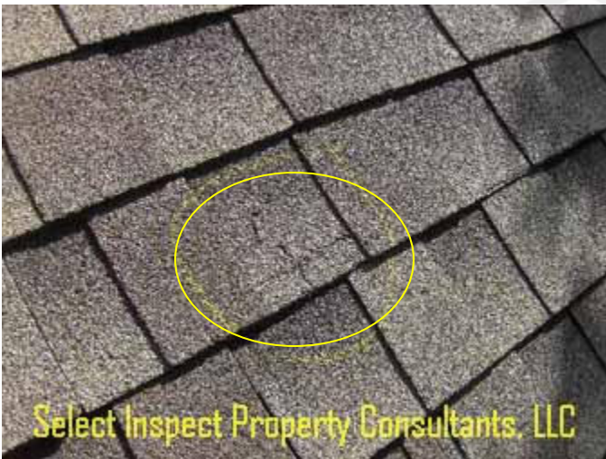
↑ undetermined damage/cracking; example
