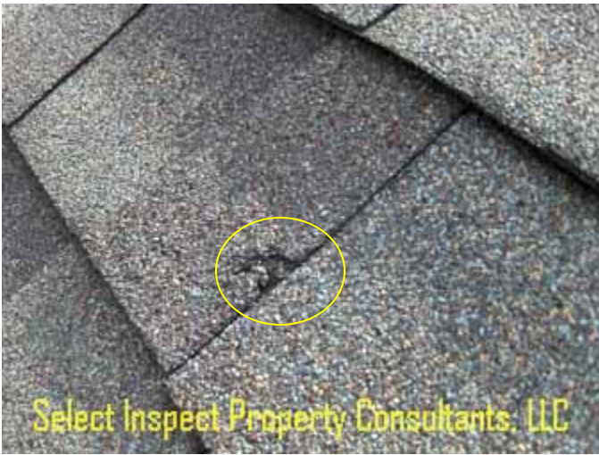
↑ impact or popped nail damage; example
