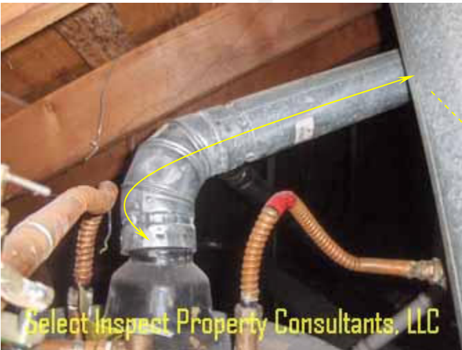
↑ inadequately supported & partially disconnected water heater flue; north
