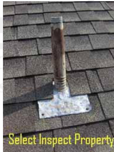
↑ deficient vent lead & uncaulked, exposed fasteners
