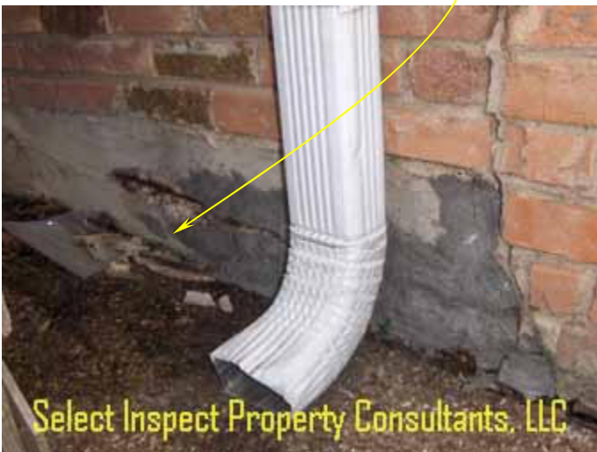
↑ deficient concrete & exposed reinforcement steel; northwest master
