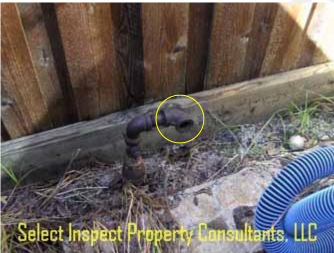
↑ abandoned gas pipe should be plugged
