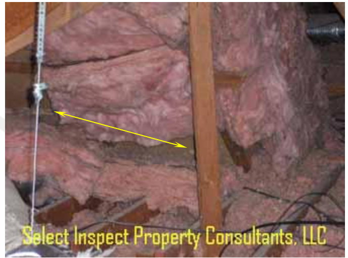
↑ deficient insulation; skylight
