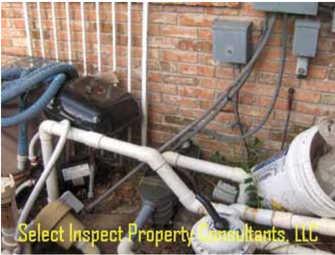
↑ multiple deficiencies, unworkmanlike, & unsafe conditions at pool equipment.
