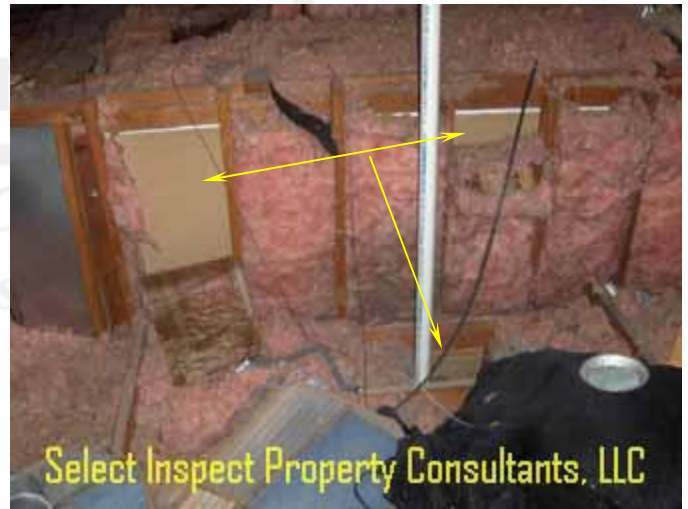
↑ deficient insulation; raised wall
