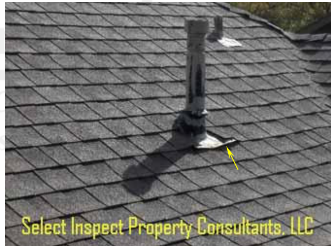
↑ lifted flashing; inadequately secured flue
