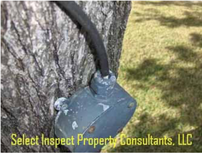
↑ deficient electrical; inadequate weather seal; example
