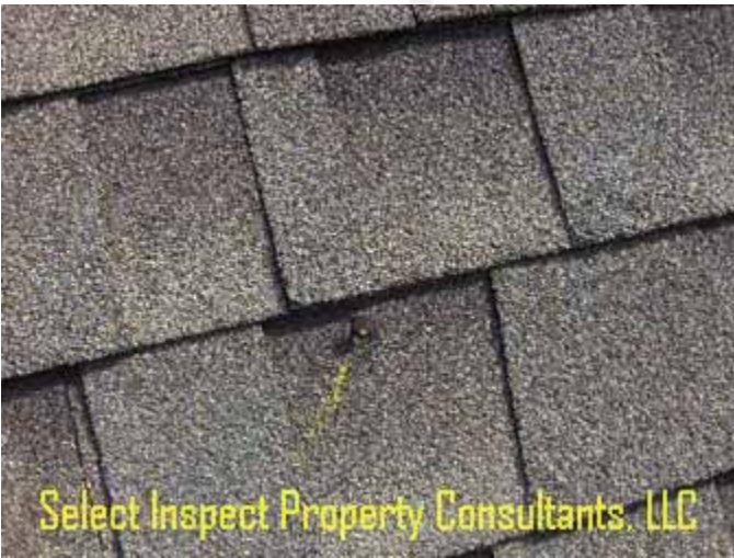
↑ popped roof nail; example
