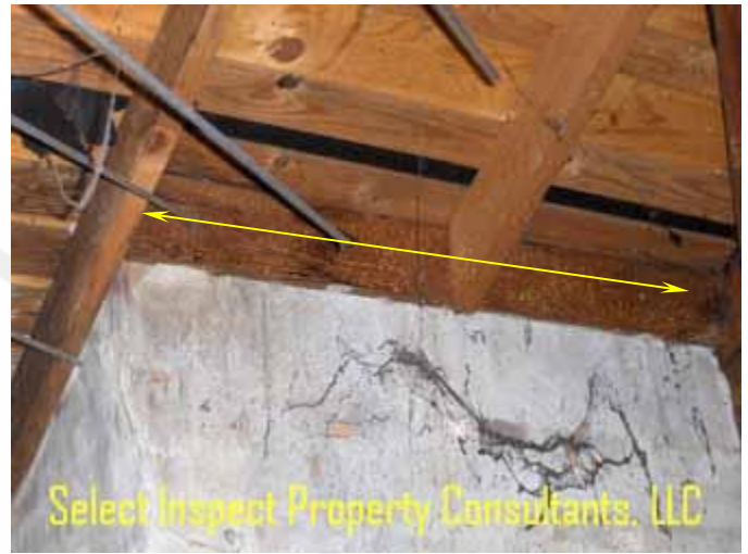
↑ moisture staining at fireplace framing
