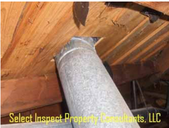
↑ furnace flue did not meet clearance requirements to combustibles
