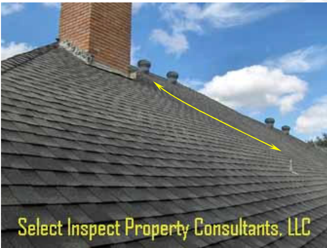
↑ deflection seen at rear roof structure
