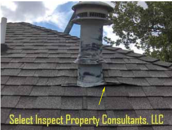
↑ lifted flue flashing example
