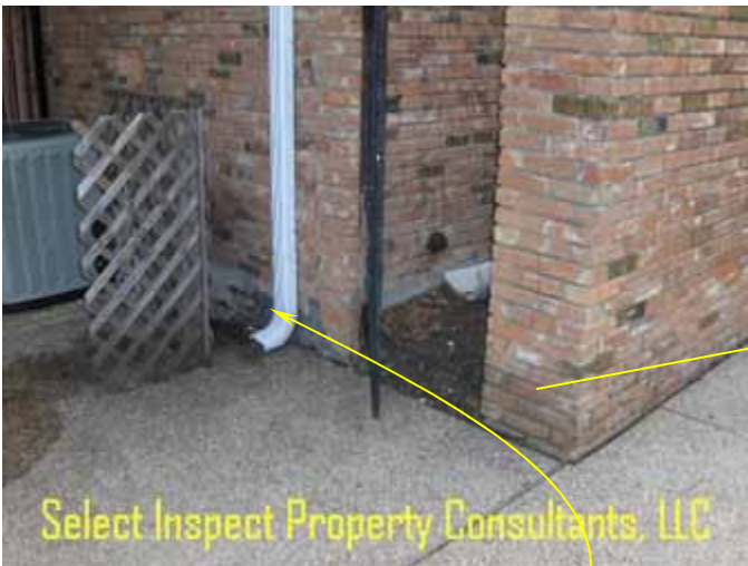
↑ deficient concrete, reinforcement steel, stress
