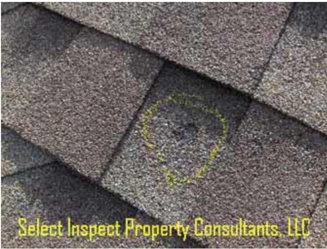
↑ impact damage example
