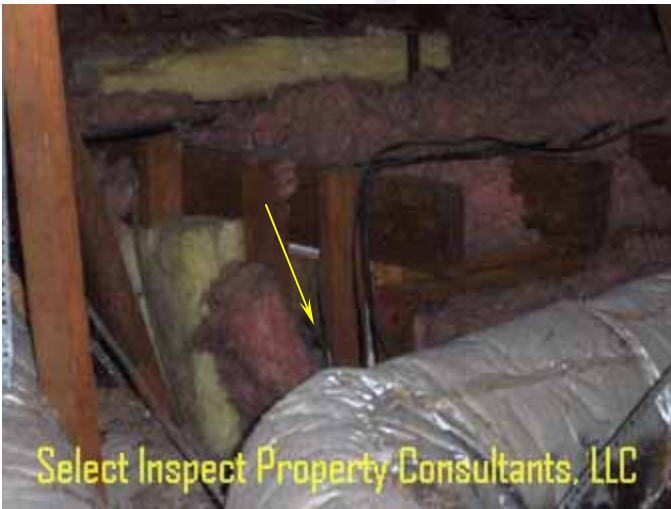
↑ deficient insulation; raised wall
