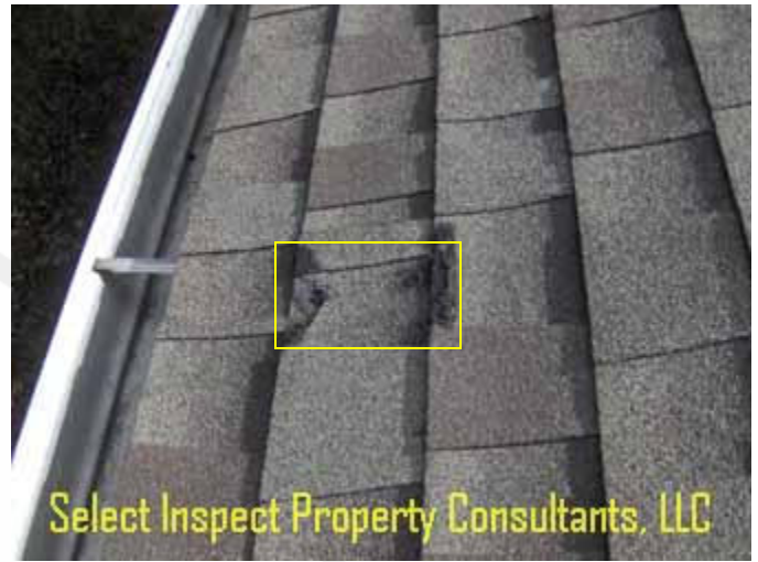
↑ missing shingle tab example
