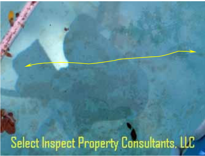
↑ close view of suspected crack
