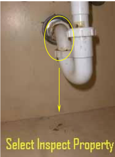
↑ leakage evidence & moisture damage under north bathroom sink
