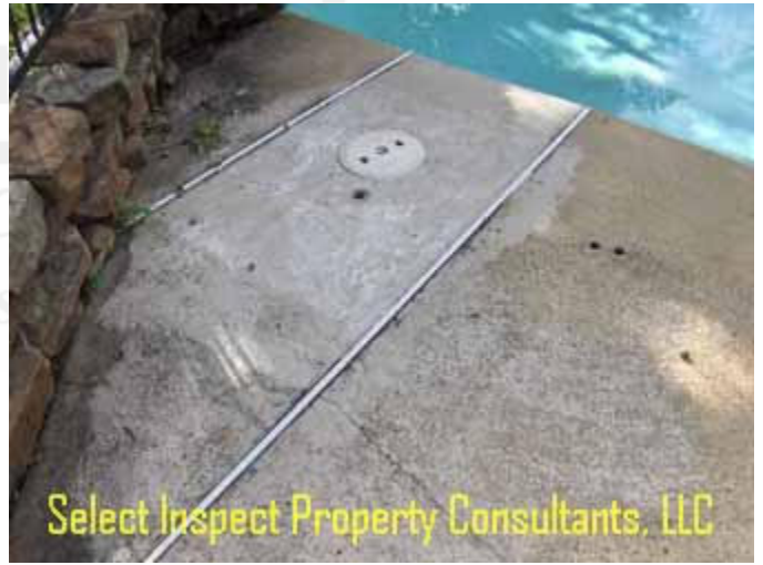
↑ repair evidence at north skimmer
