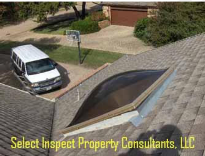
↑ deficient skylight; rot & moisture intrusion
