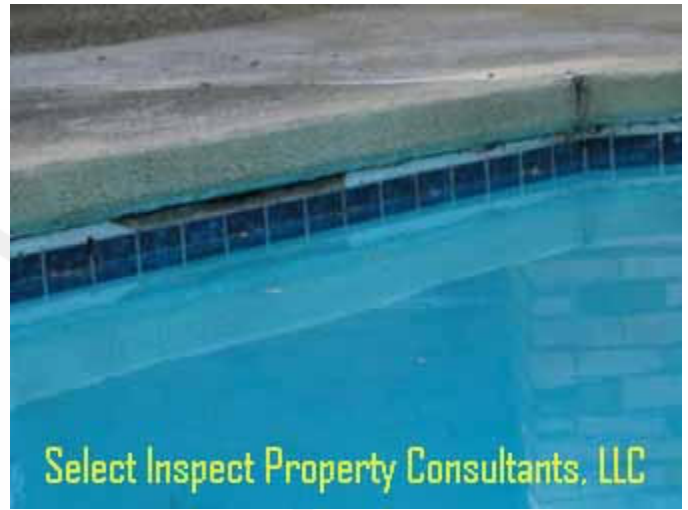
↑ deficient mortar at deck overhang; example
