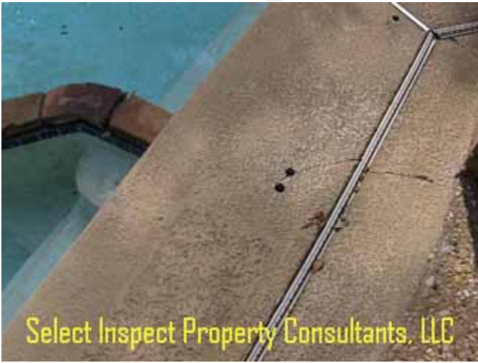
↑ stress & cracks at pool deck
