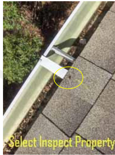
↑ uncaulked, exposed fasteners at multiple gutter locations; example
