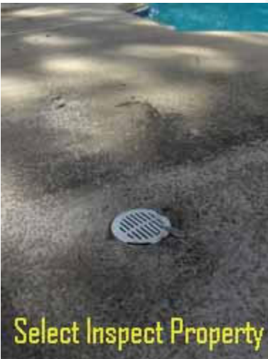
↑ sharp drain edges may be a cut hazard; example
