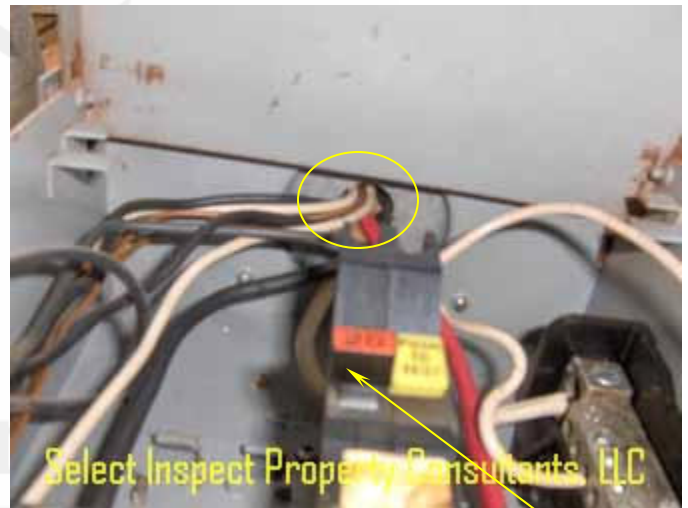
↑ missing grommet & not functioning as intended ground-fault circuit interrupt (GFCI) overcurrent-protection-device; sub panel
