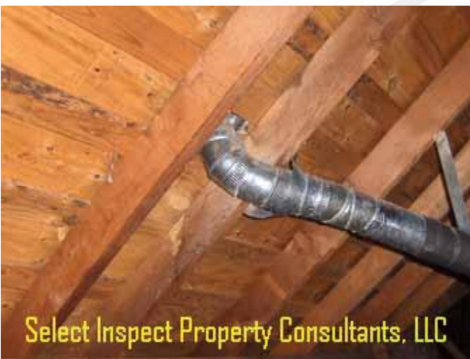
↑ dryer vent amiss/deficient & lint spillage into attic; fire hazard
