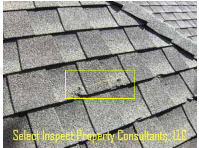
↑ undetermined damage; example
