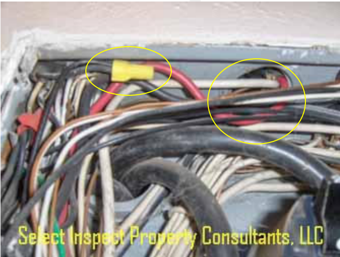
↑ splices & missing grommet; main panel
