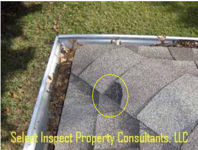
↑ damaged ridge shingle
