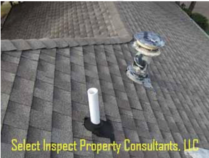
↑ unpainted plumbing vent; uncaulked, exposed fasteners
