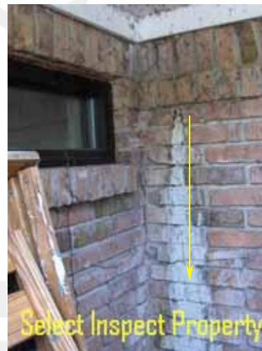
↑ stains from prior auxiliary condensate drainage
