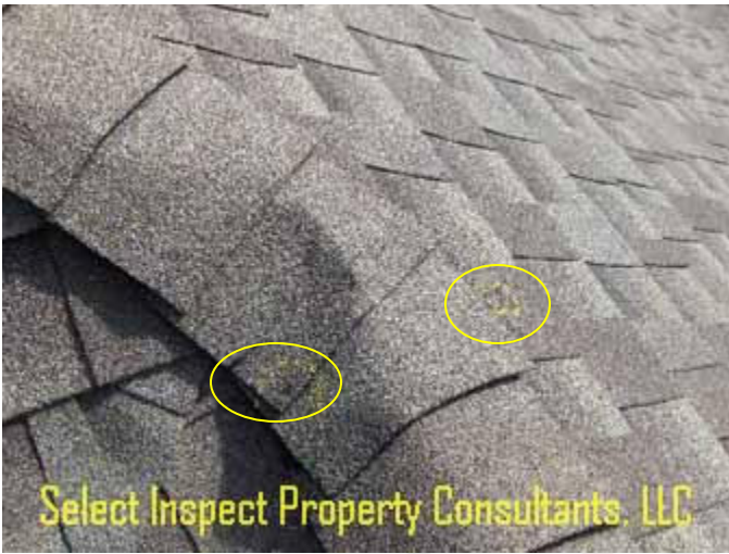
↑ uncaulked, exposed fasteners
