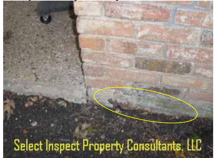
↑ deficient concrete & exposed reinforcement steel; northeast
