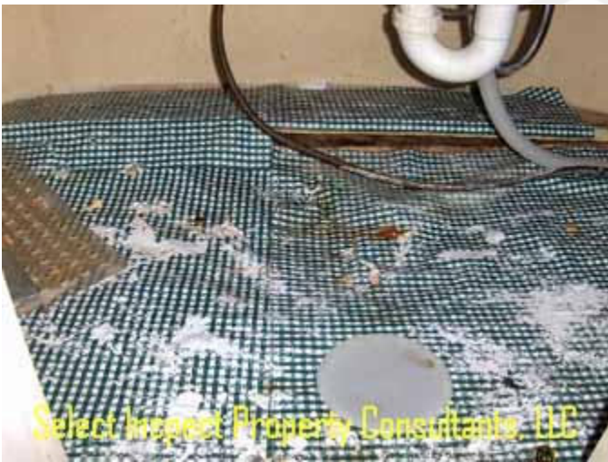
↑ moisture damage & fungus below sinks; example at kitchen
