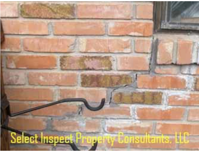
↑ stress crack; south example
