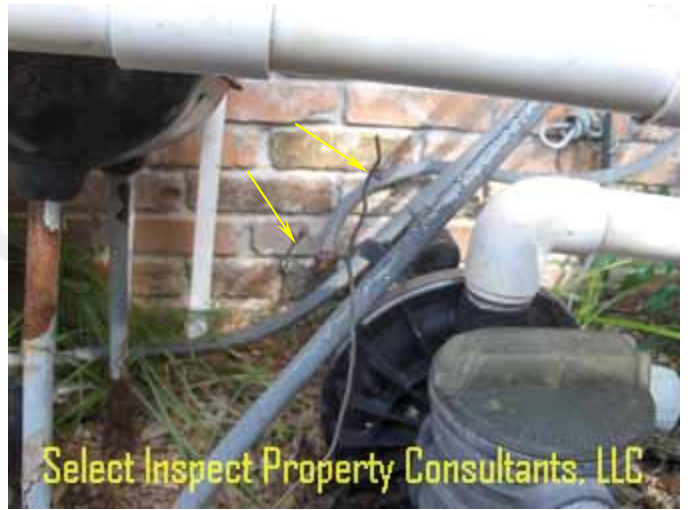
↑ unbonded pool equipment & damaged/stressed conduit
