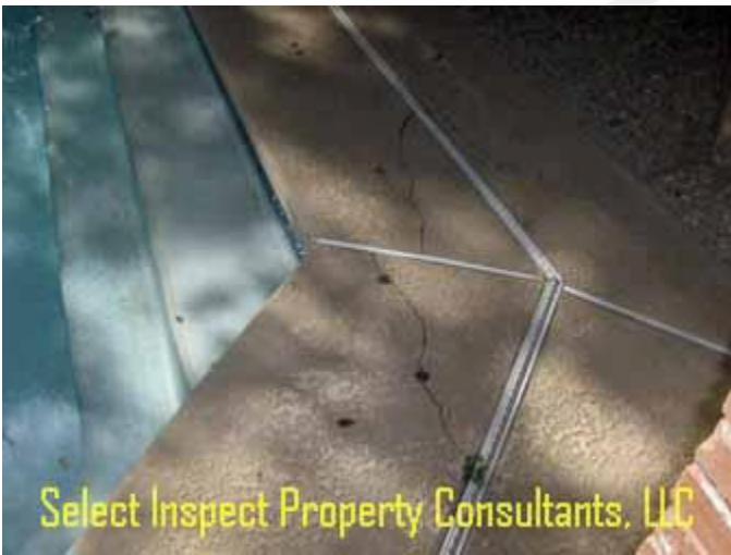
↑ stress & cracks at pool deck & channel drains
