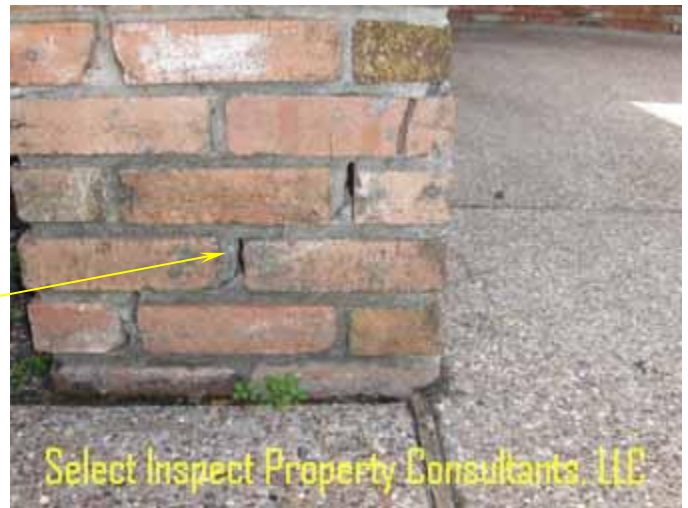
↑ differential movement at north wingwall
