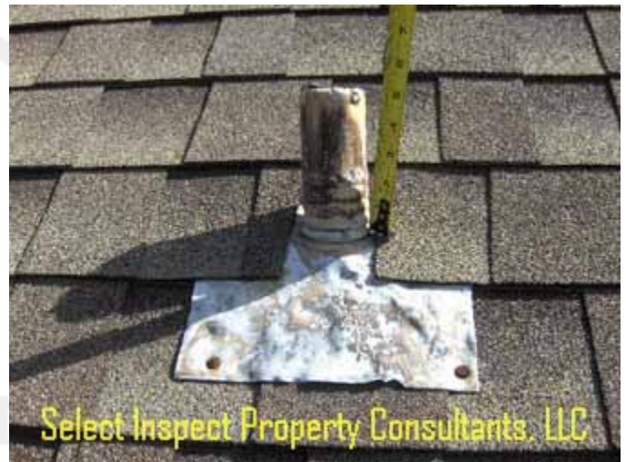
↑ plumbing vent(s) was shorter than required & uncaulked, exposed fasteners
