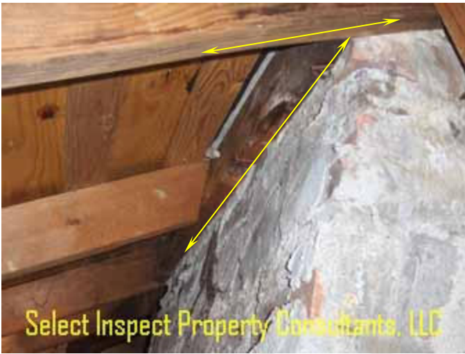
↑ moisture damage & fungus at fireplace framing
