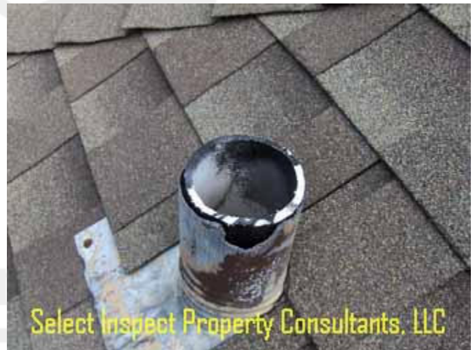
↑ rodent damage example at plumbing vent; moisture intrusion concern & uncaulked, exposed fasteners
