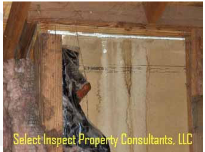
↑ deficient insulation & moisture intrusion/damage at front skylight
