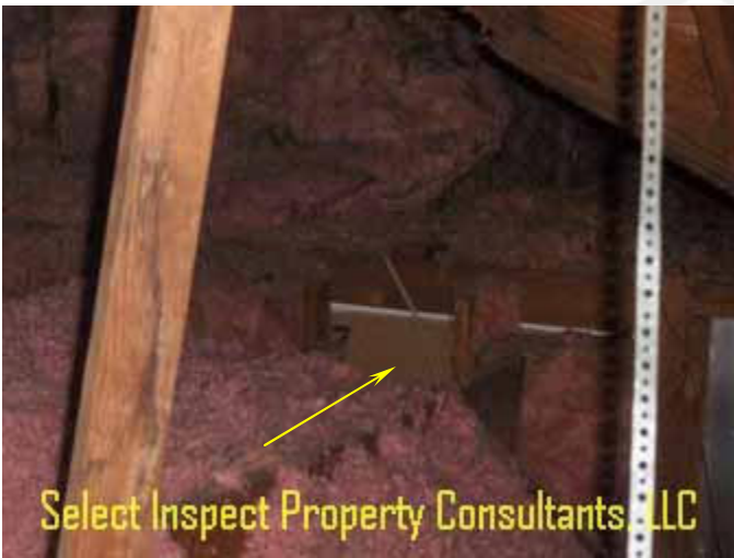
↑ deficient insulation; raised wall
