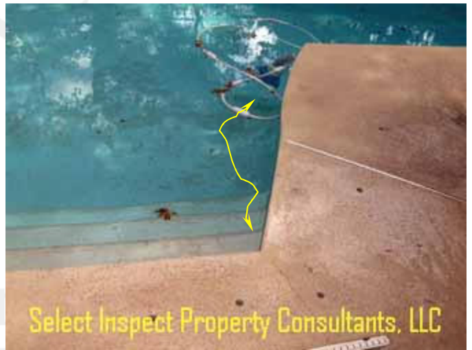
↑ suspected crack at pool
