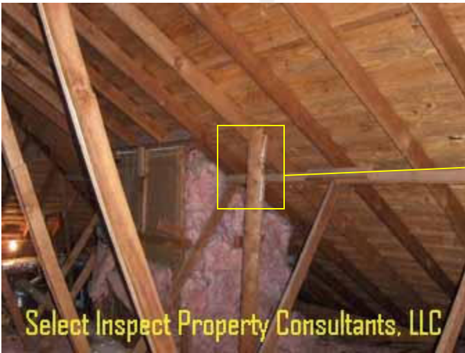
↑ failed framing adjacent front skylight
