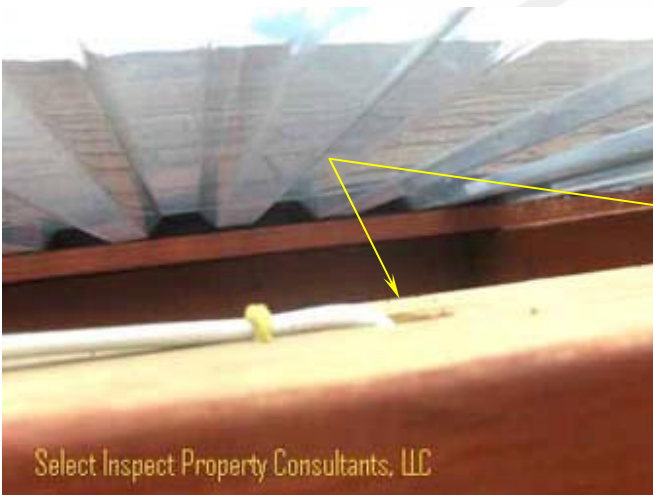
↑ Deficient excess reveal (opening) at patio fan electrical/mounting
