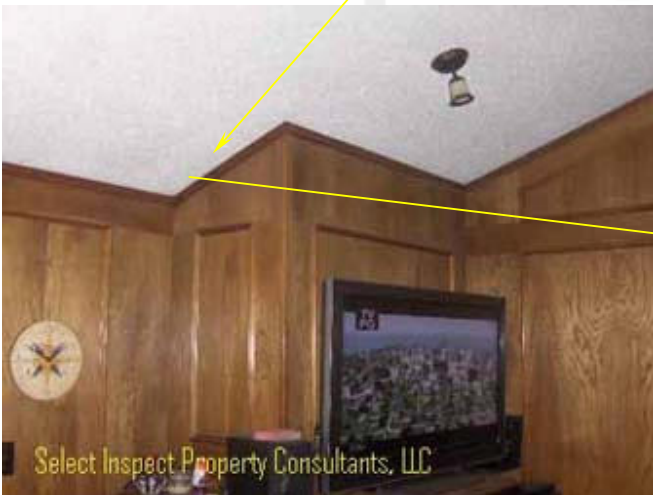
↑ moisture damage & fungus at family room interior below the deficient chimney flashing- inaccessible from the attic
