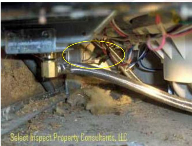
↑ unworkmanlike electrical below/behind dishwasher
