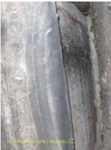
↑ unclean evaporator(s) coils & cabinet
