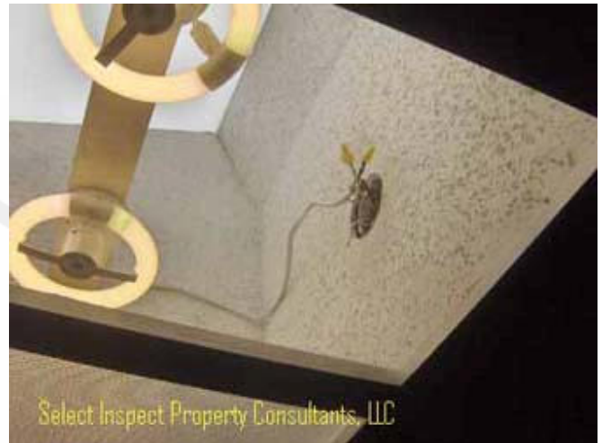
↑ unworkmanlike/unsafe electrical at skylight; splices, open conductors, Wires should be secured within 12 inches of junction boxes, switches, receptacles, fixtures
