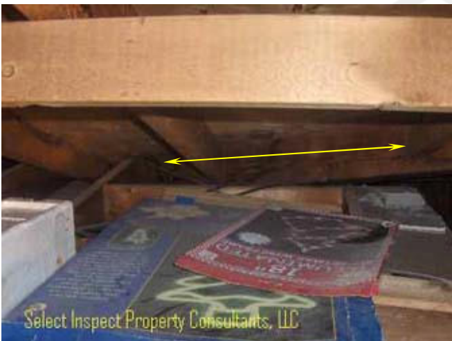
↑ moisture staining at valley rafters; garage attic west
