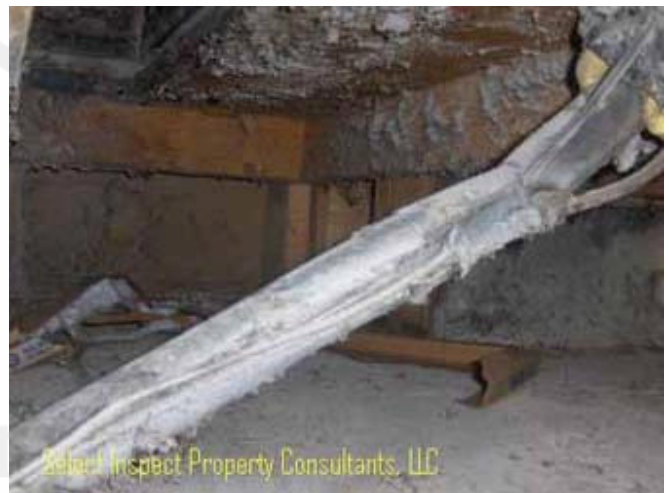
↑ unclean plenum & debris; below HVAC
