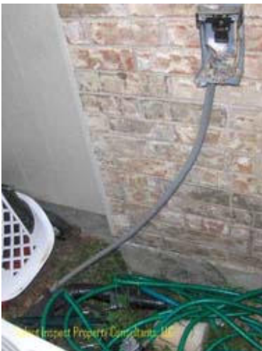
↑ inadequately secured conduit at air conditioning condenser
