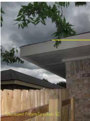
↑ inadequate drip edge flashing overlap at all sides; example at north-northeast
