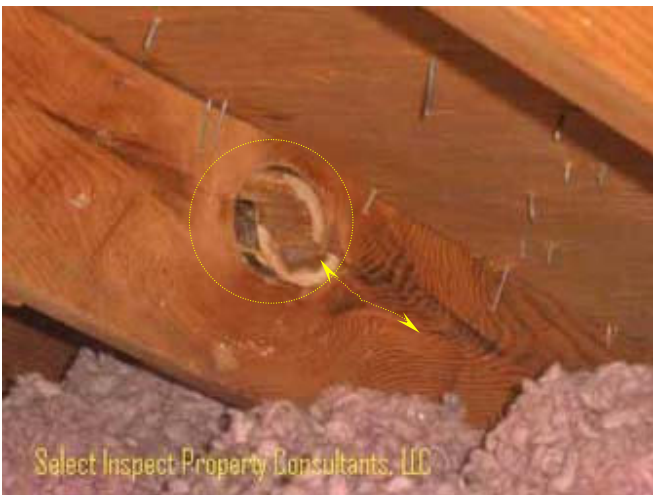
↑ close view of image above
