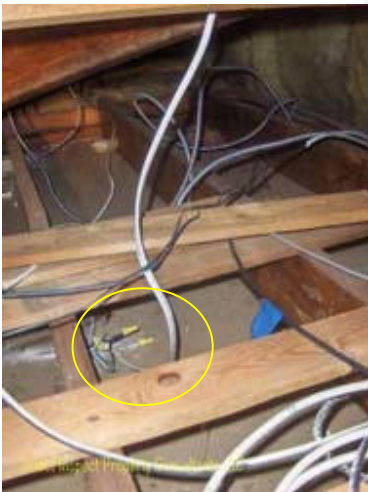
↑ unworkmanlike electrical in attic
