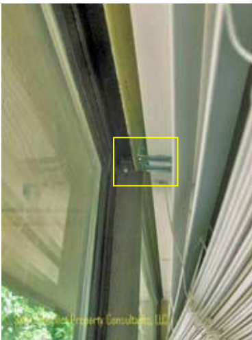
↑ unworkmanlike blind install- master- obstructed window; emergency escape concern
