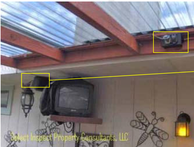
↑ multiple unworkmanlike/unsafe conditions at patio electrical
