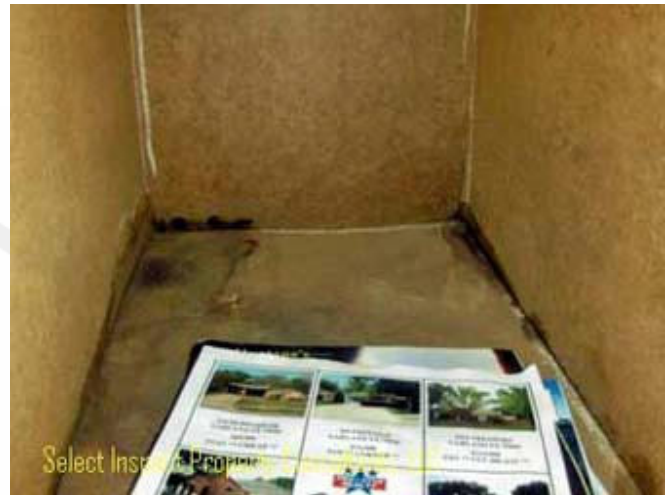
↑ moisture damage & fungus right kitchen cabinet-east
