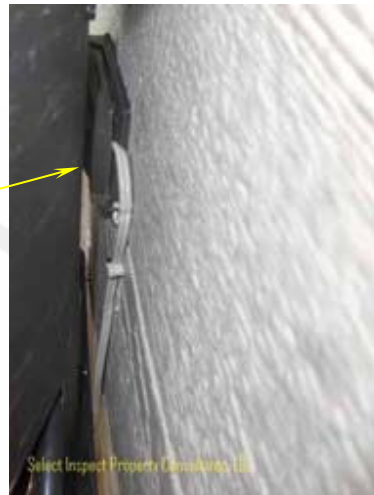
↑ crimped cord & improper permanent use cover
