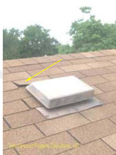
↑ example deficient shingle at roof vent
