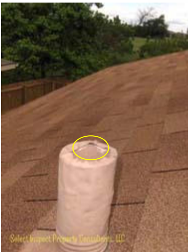
↑ inadequate wrap at plumbing vent; opening may allow moisture intrusion; not readily accessible from attic-west bathroom
