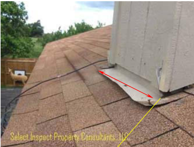
↑ deficient chimney flashing
