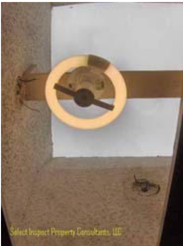
↑ unworkmanlike/unsafe electrical at skylight; open conductors
