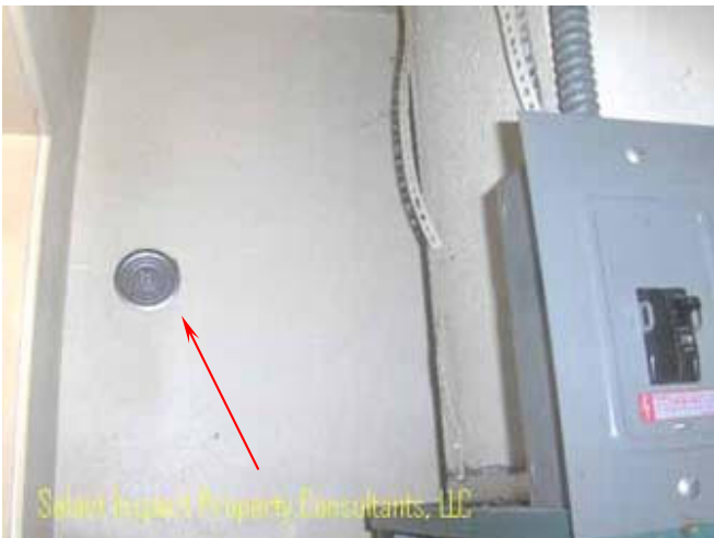
↑ tin can lid at mechanical closet wall- undetermined reason- not removed
