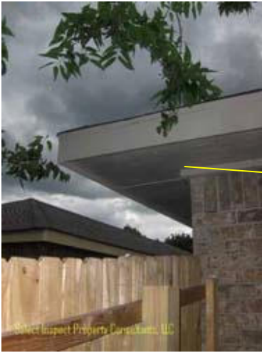
↑ frieze-board separation at the northeast
