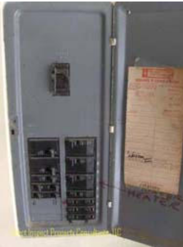
↑ black label square D overcurrent-protection-devices
