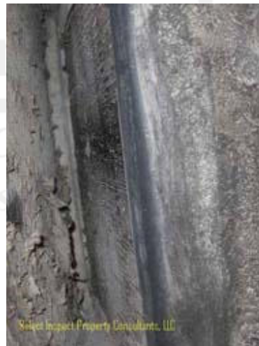
↑ unclean evaporator(s) coils & cabinet
