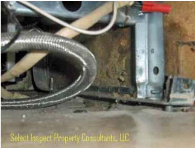
↑ moisture damage & fungus under dishwasher
