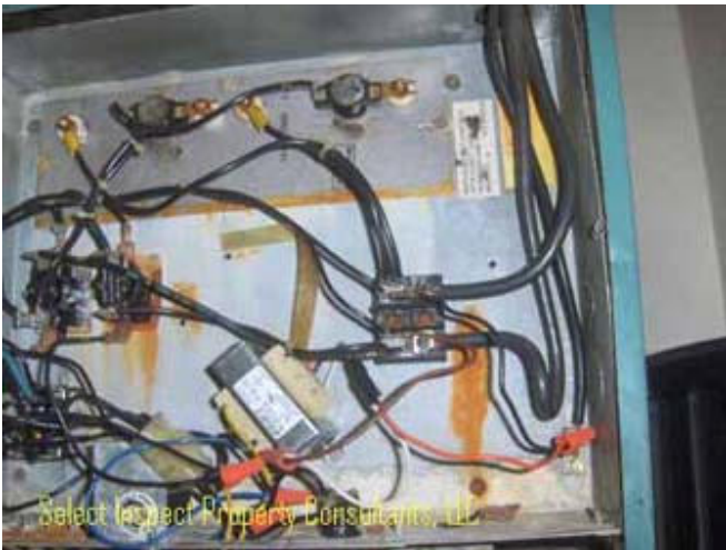
↑ corrosion at heat components; HVAC
