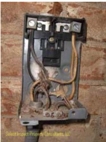
↑ missing overcurrent-protection-device at air conditioning disconnect (lack of disconnect) ; hardwired; unworkmanlike & unsafe
