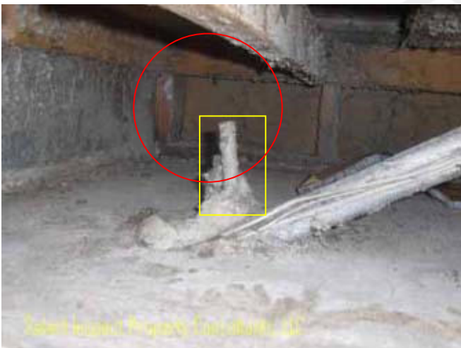
↑ unclean plenum; hollow stake (yellow), moisture staining (red); below the HVAC
