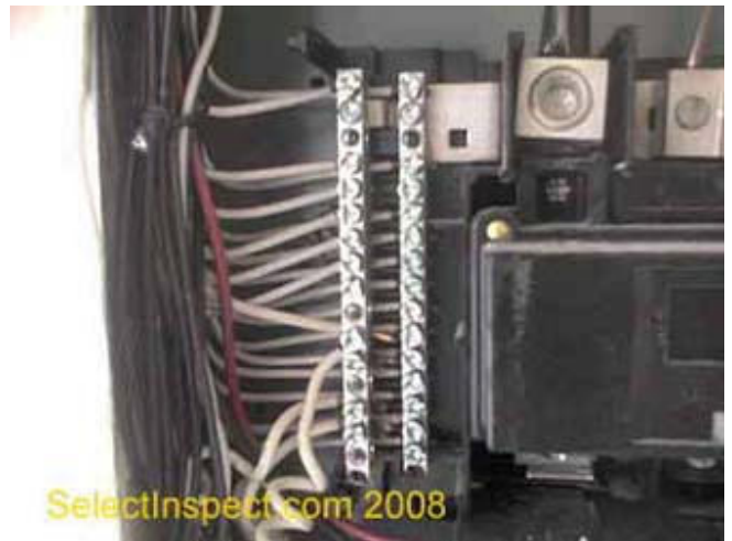
example at another property of correct neutral wiring
