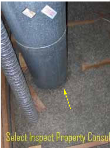
↑ fireplace flue did not meet clearance requirements to insulation
