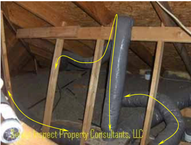
↑ inadequate support of air ducting; example; crimped air ducting; example
