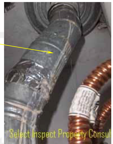
↑ moisture intrusion & rust/corrosion at water heater flue
