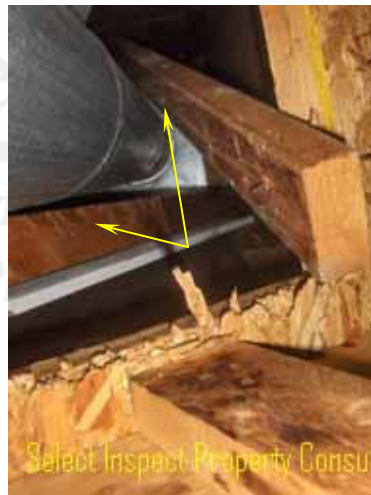
↑ inadequately secured framing & fireplace flue did not meet clearance requirements to combustibles
