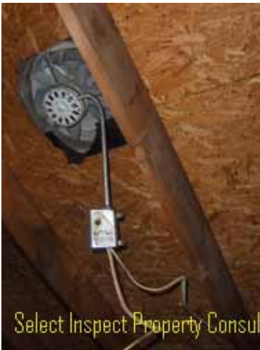
↑ unworkmanlike electrical & inoperable attic fan- 1 of 2 fans
