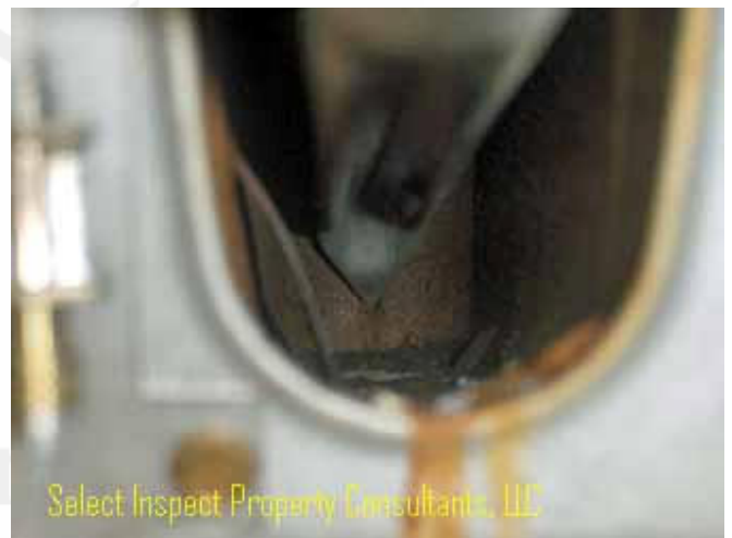
↑ rust & scale in burn chambers; example
