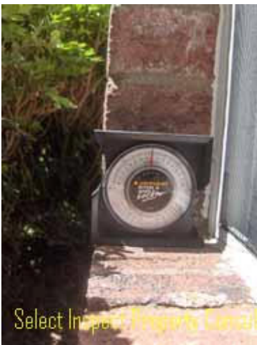
↑ brick ledge(s) had inadequate slope
