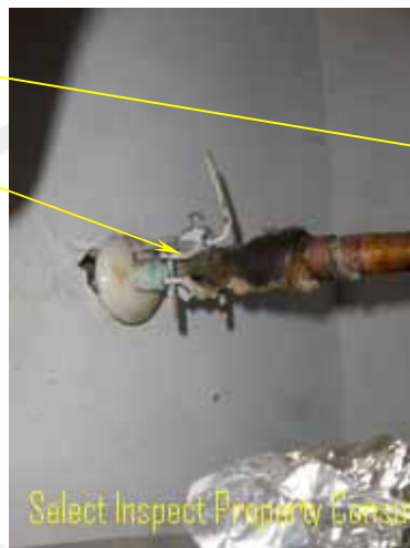
↑ seepage at shut-off-valve
