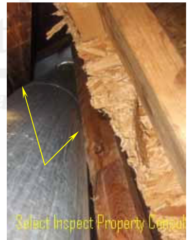
↑ fireplace flue did not meet clearance requirements to combustibles
