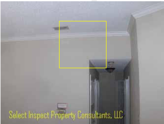
↑ Thermal imaging implies energy loss at family room adjacent the HVAC chase
