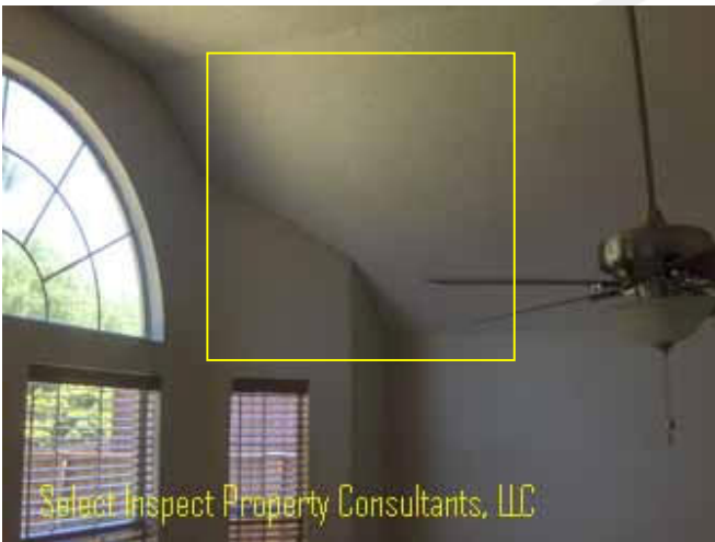
↑ Thermal imaging implies energy loss at master
