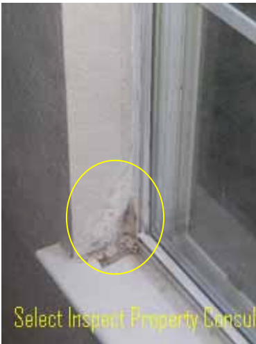
↑ leakage, moisture damage & fungus at master window
