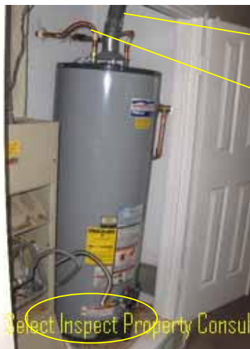
↑ out of level; missing auxiliary pan; moisture damage at deck
