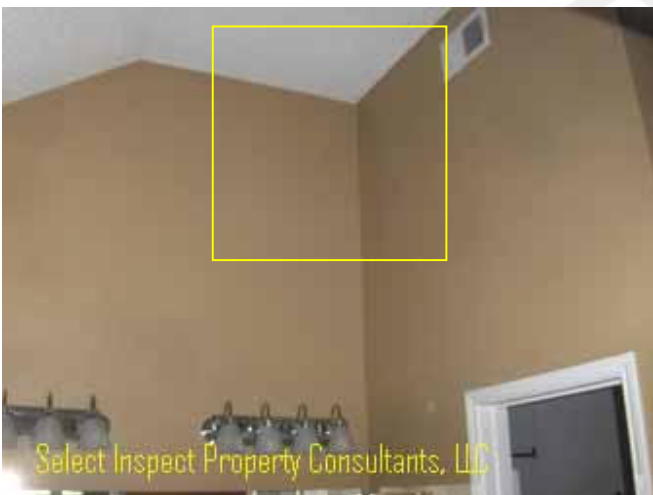
↑ Thermal imaging implies energy loss at master bathroom
