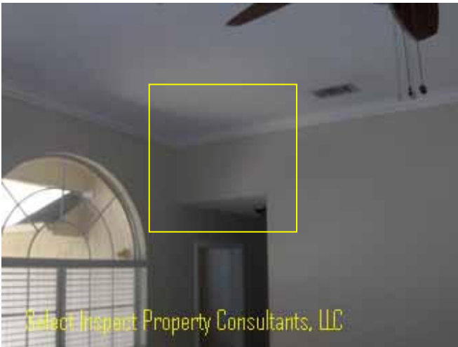
↑ Thermal imaging implies energy loss at family room
