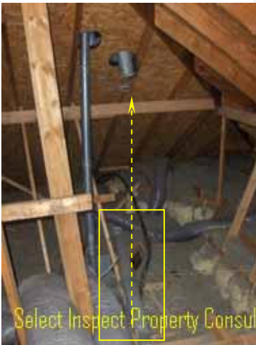
↑ deficient furnace flue & HVAC & water heater flues did not meet clearance requirements to combustibles
