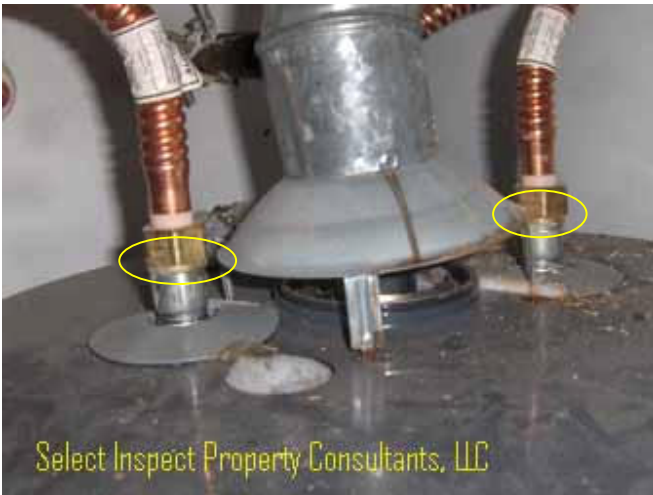
↑ water heater- monitor the compression fittings & copper/galvanized pipe connections for potential electrolysis
