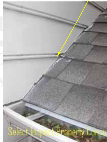
↑ low siding; missing kick-out-flashing; rotting siding below eave
