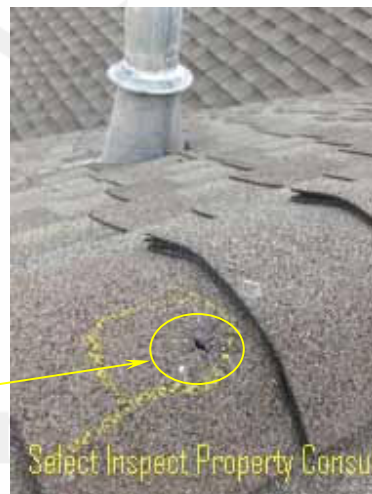
↑ opening at shingle; example
