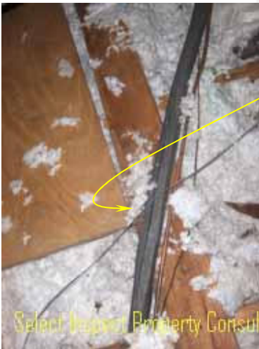
↑ close view of image above right; moisture staining at attic insulation
