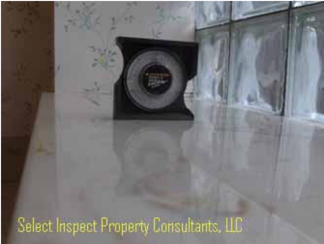
↑ master bathroom window has shifted outward & the bathtub(s) ledge has negative slope.
