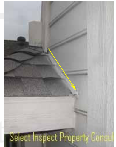
↑ missing kick-out-flashing; chimney south
