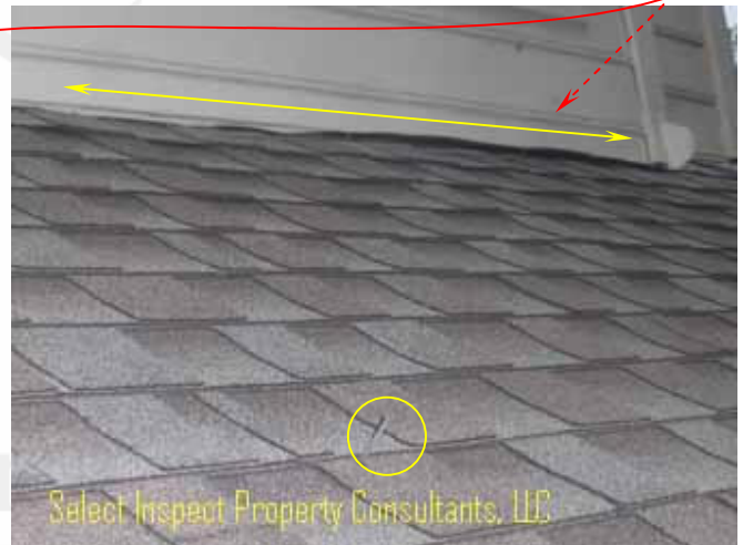
↑ inadequately secured flashing & nail
