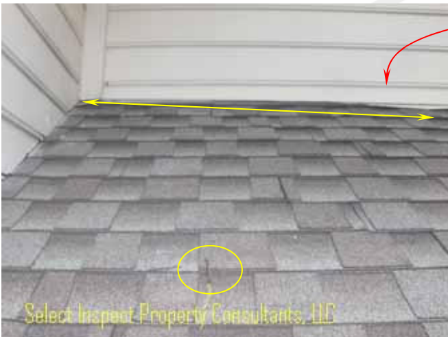
↑ inadequately secured flashing & nail
