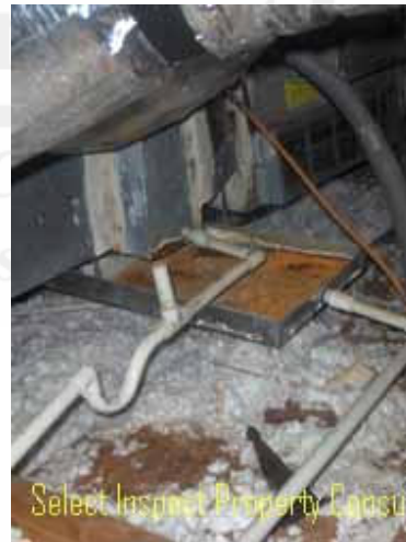
↑ air conditioning primary condensate drain should be insulated; moisture staining at floor & attic insulation; corroded evaporator(s) & auxiliary pan; inadequately sealed joints- downstairs HVAC
