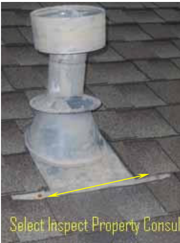
↑ uncaulked, exposed fasteners; example at water heater flue
