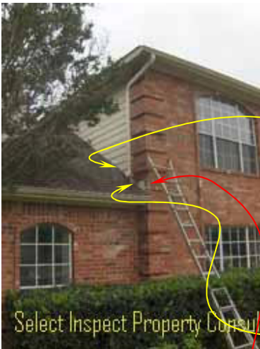
↑ low siding; deficient flashing; openings
