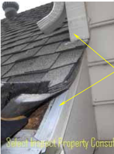
↑ missing kick-out-flashing; rotting deck
