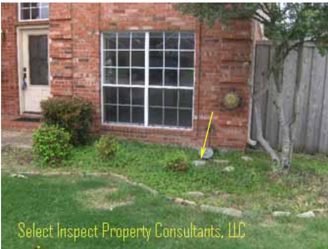
↑ high water pressure at home & buried components at front garden
