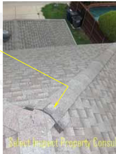
↑ unusual full shingle tab at ridge; upper southwest
