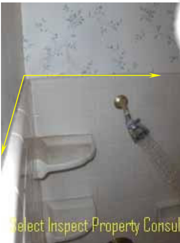
↑ caulking/sealant needed atop shower tile/panels; example
