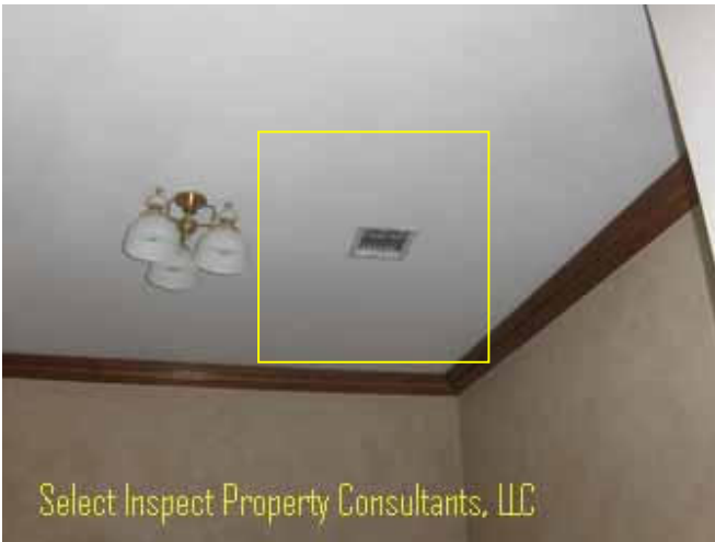
↑ suspect inadequate seal at HVAC register/boot/duct- study
