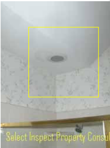
↑ Thermal imaging implies energy loss & or moisture at master bathroom (staining present during the inspection); deficient plumbing vent discovered above at roof
