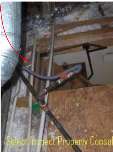
↑ unprotected gas components & HVAC drain piping & flue impeding attic access; unworkmanlike & unsafe
