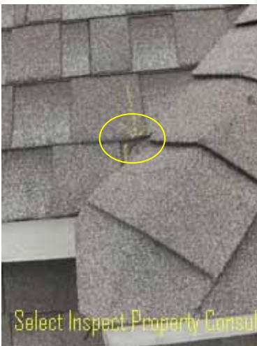
↑ damaged shingles at valley over image pictured above
