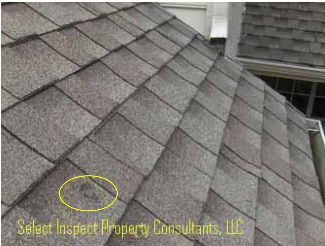
↑ impact damage at garage east
