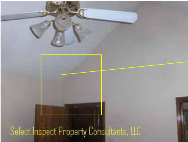
↑ Thermal imaging implies energy loss at vaults; example at master
