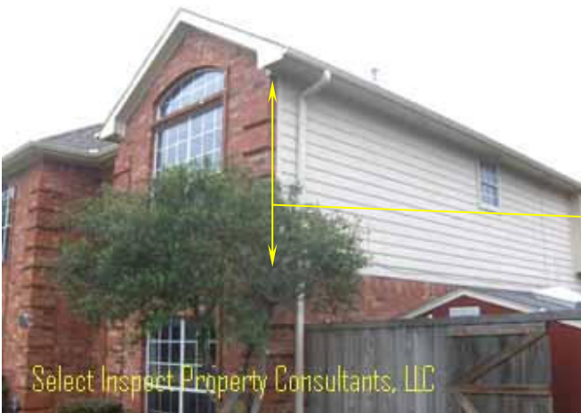
↑ veneer separation at the northwest
