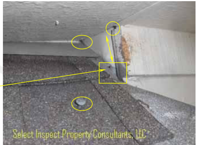
↑ uncaulked, exposed fasteners & unworkmanlike flashing; openings; & rodent gnawing evidence
