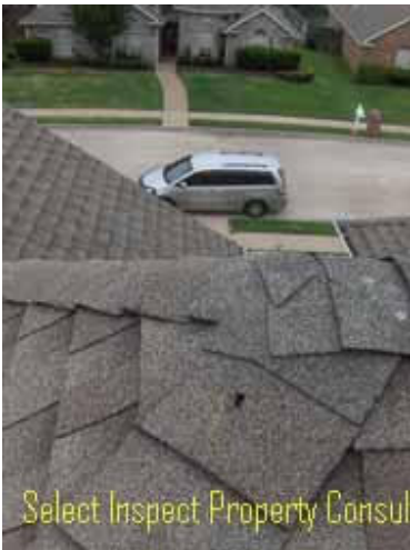
↑ openings at shingles & uncaulked, exposed fasteners
