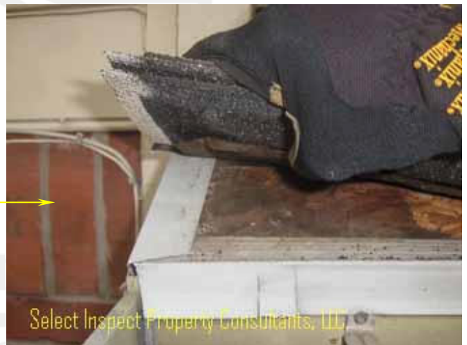
↑ close view of image at left; rotting roof deck
