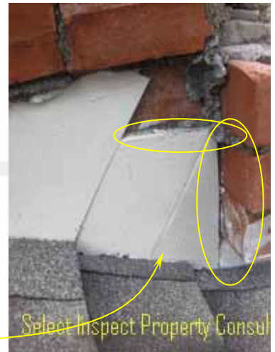
↑ unworkmanlike flashing; openings
