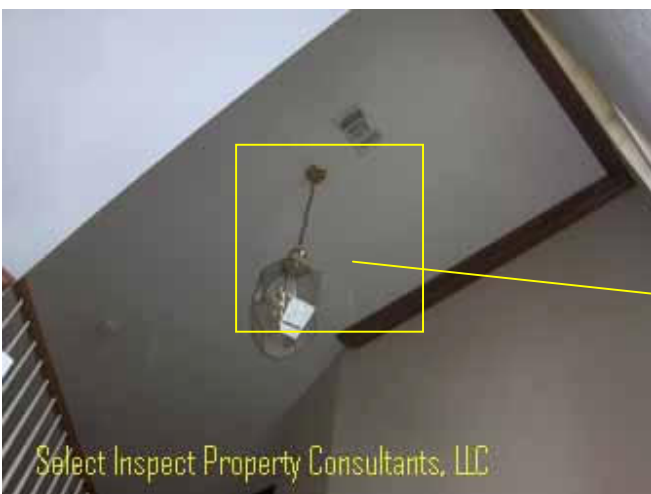
↑ Thermal imaging shows energy loss & or moisture evidence above the foyer
