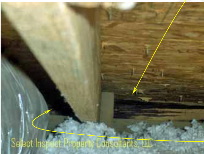
↑ moisture damage/rot in attic; adjacent the image above right
