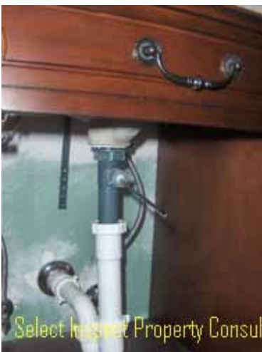
↑ unworkmanlike inoperable drain stop; upstairs bathroom
