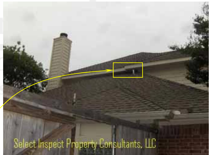
↑ moisture intrusion; moisture damage
