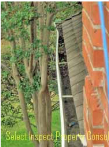
↑ example deficient guttering
