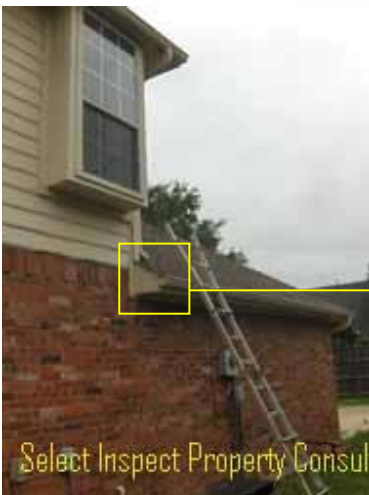
↑ moisture damage at roof deck; missing kick-out-flashing
