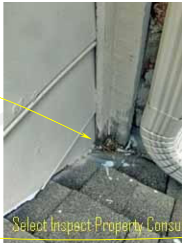
↑ close view of image at left; moisture damage, inadequate converging valley slope
