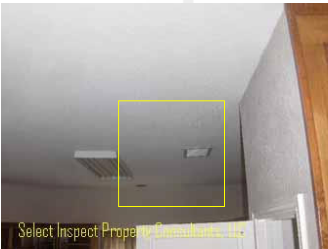
↑ suspect inadequate seal at HVAC register/boot/duct-kitchen
