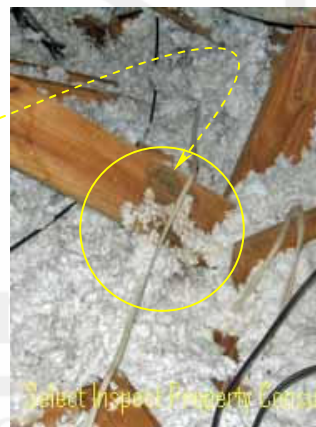
↑ moisture staining at insulation & framing; moisture staining at east bedroom ceiling below this location
