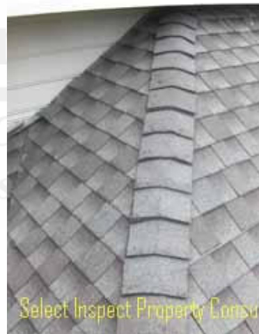
↑ damaged roof ridge near chimney
