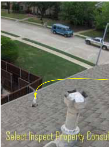
↑ example deficient plumbing vent collar; moisture intrusion point
