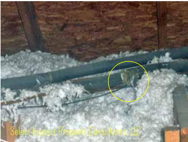
↑ deficient refrigerant insulation joint & leakage evidence above moisture staining at southwest bedroom
