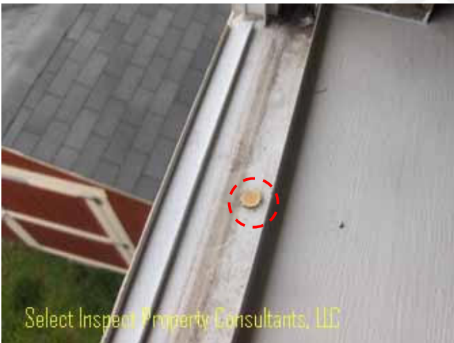
↑ Alarm holes at the lower portion of the window may allow moisture intrusion; caulk and monitor
