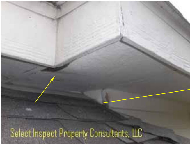
↑ moisture damage; east eave
