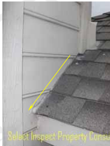
↑ missing kick-out-flashing; chimney north
