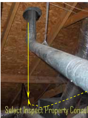
↑ both flues did not meet clearance requirements to combustibles & moisture intrusion from roof
