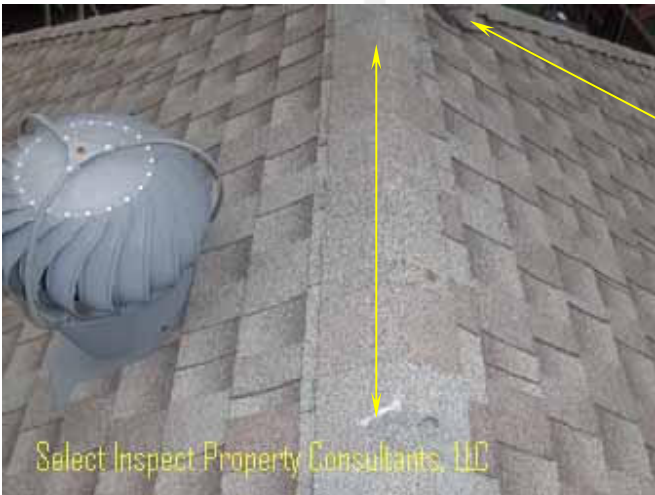
↑ impact damage example
