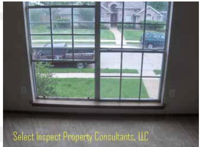
↑ window(s) lower than 24" interior & higher than 72" exterior; example
