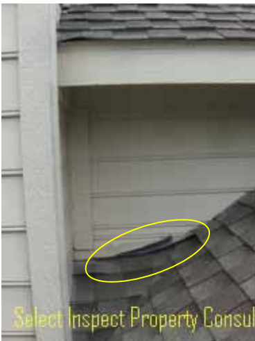
↑ deficient flashing behind chimney
