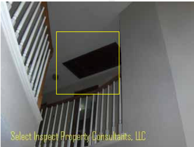
↑ energy loss at attic accesses; example at ladder
