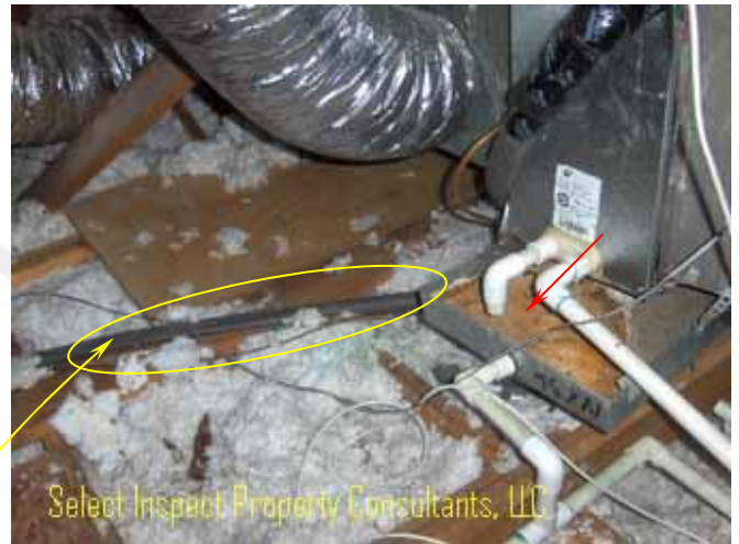
↑ corrosion at auxiliary pan & deficient refrigerant insulation; air conditioning primary condensate drain should be insulated; upstairs HVAC
