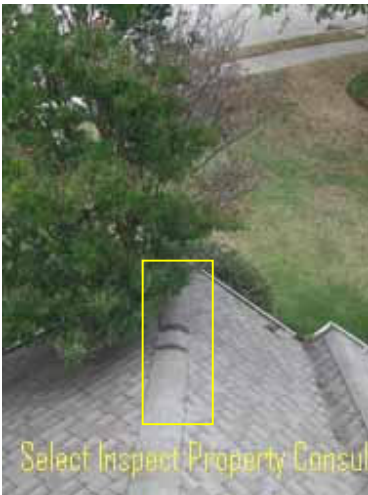
↑ deficient ridge shingles; northeast
