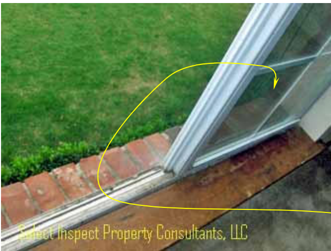
↑ moisture staining & worn mortar example at upstairs window
