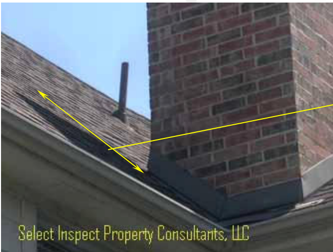
↑ deflection of roof noted adjacent the chimney
