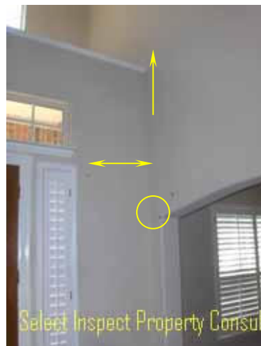
↑ cracks discovered at entry
