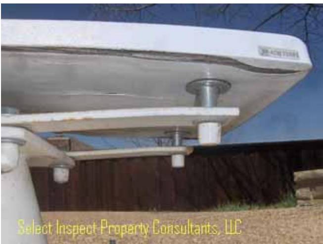
↑ corrosion & damage at diving board components
