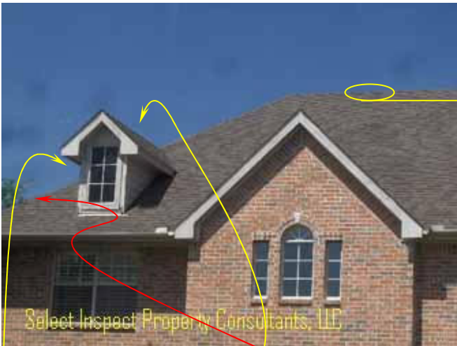
↑ damaged shingles discovered
