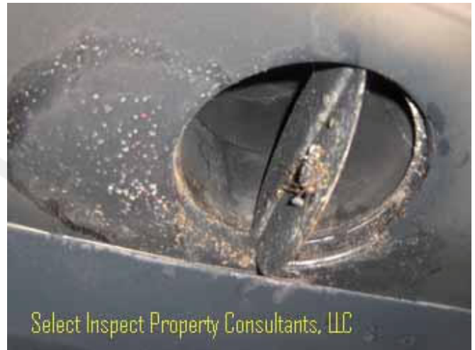
↑ moisture staining at flue & damper of fireplace
