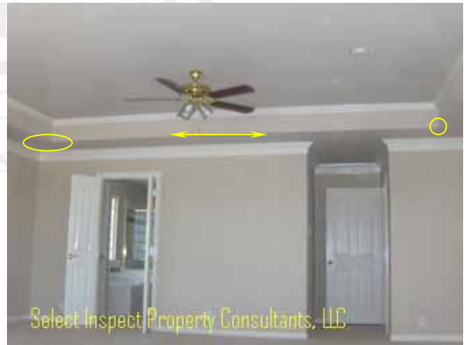
↑ cracks discovered at master
