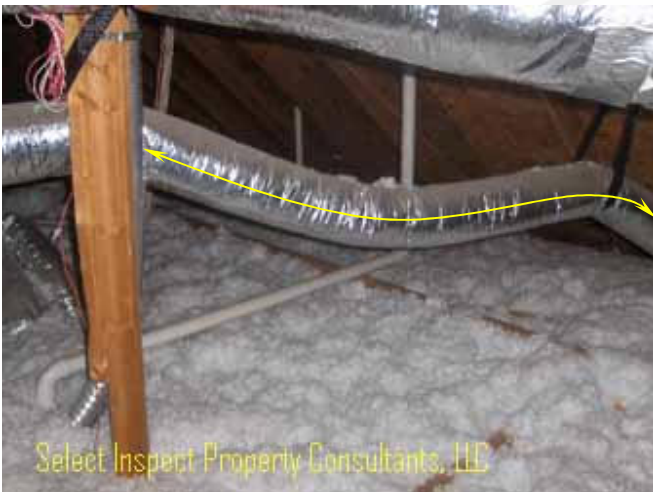
↑ inadequate support of air ducting; example
