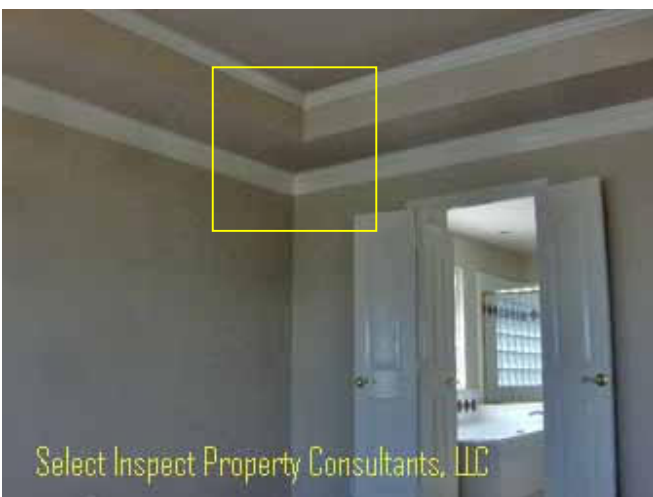
↑ Thermal imaging implies energy loss at master bedroom furr down- south corner
