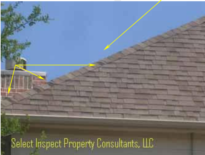
↑ close view of image above ridge damage
