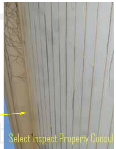
↑ bulging/warped siding- indicates stress; northwest
