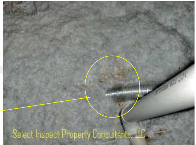
↑ moisture damage at insulation
