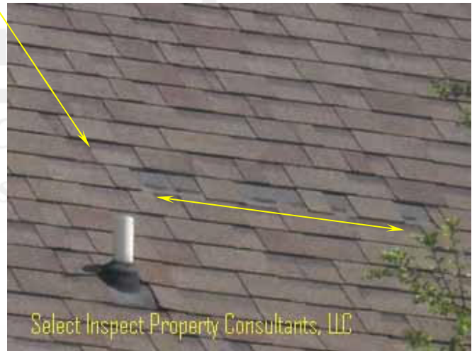
↑ close view of image above; damage & unpainted vent stack
