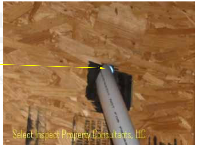
↑ close view of image at left; daylight visible from attic
