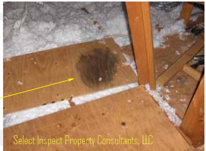
↑ moisture staining at attic floor –note, this plywood is NOT stable
