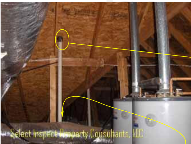
↑ moisture intrusion from deficient vent collars; example
