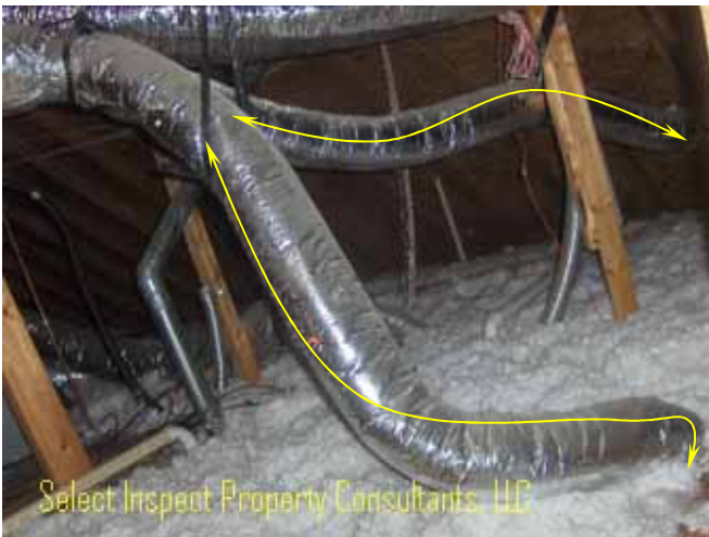
↑ inadequate support of air ducting; crimped air ducting; example
