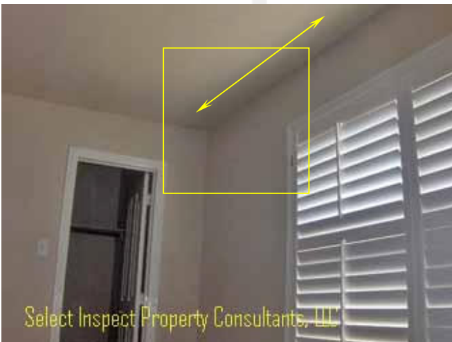
↑ Thermal imaging implies energy loss at south bedroom
