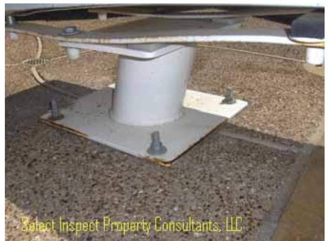
↑ corrosion & damage at diving board components
