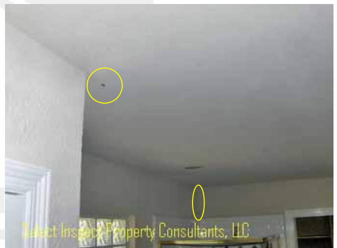
↑ cracks discovered at master bathroom
