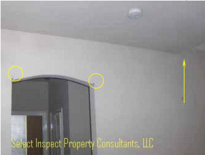
↑ cracks discovered at downstairs hall
