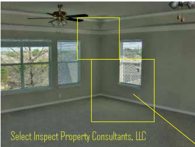
↑ Thermal imaging implies energy loss at master-east
