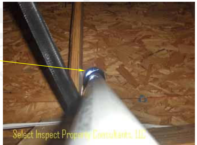
↑ close view of image at left; damaged collar- daylight visible from attic
