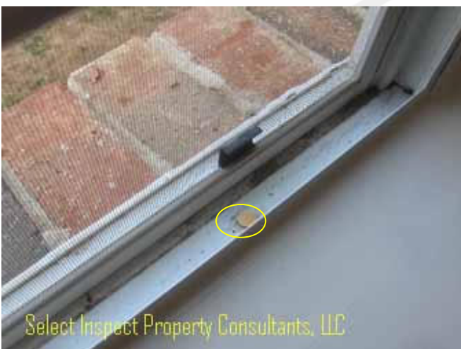
↑ Alarm holes at the lower portion of the window may allow moisture intrusion; caulk and monitor
