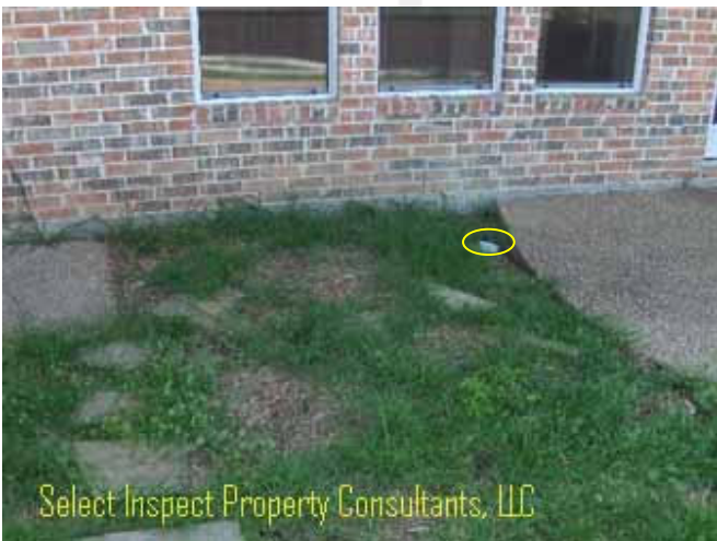
↑ area drain port not at low point & missing covers; negative grading adjacent the rear porch
