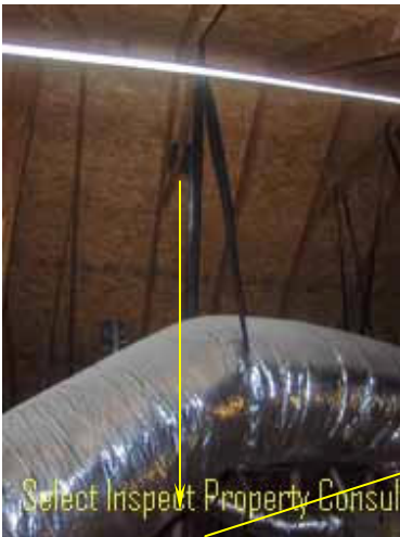
↑ moisture staining below roof vent implies moisture intrusion
