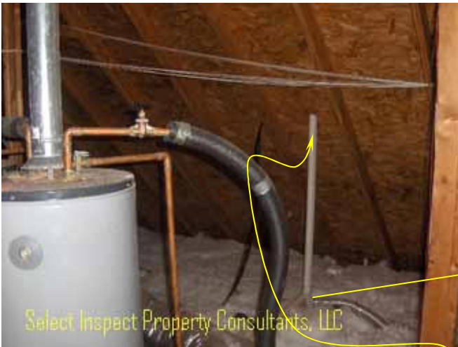
↑ moisture intrusion from deficient vent collars; example
