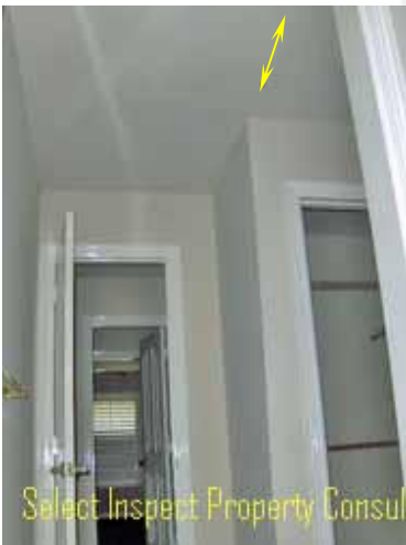
↑ cracks discovered at split bath
