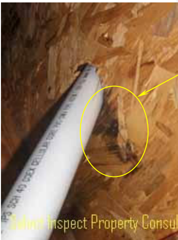
↑ moisture intrusion & decay at roof deck
