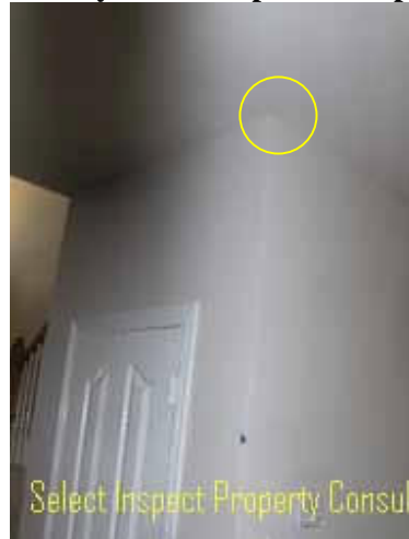
↑ cracks discovered at family room/loft
