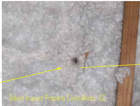
↑ moisture evidence at insulation
