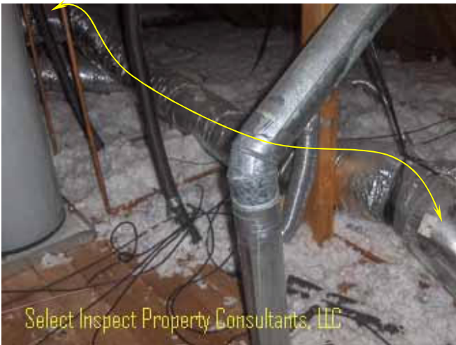
↑ inadequate support of air ducting; example
