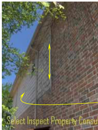
↑ exterior stress & openings; west-northwest
