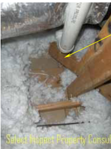
↑ moisture staining at framing & ceiling drywall
