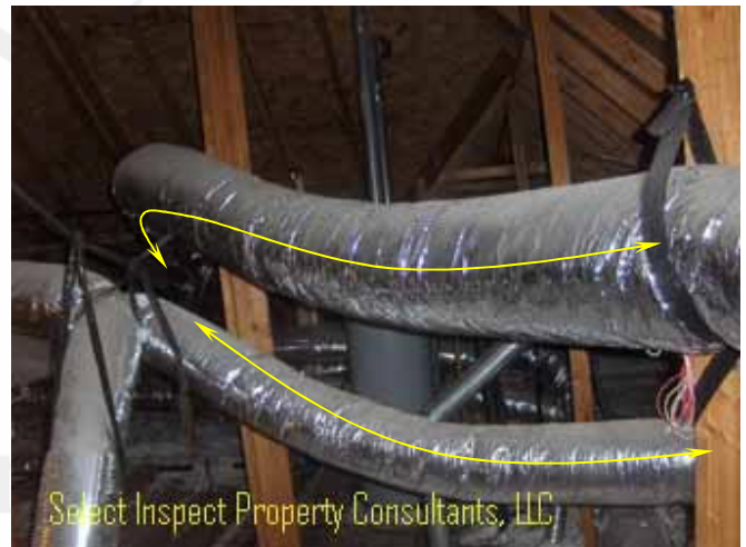
↑ inadequate support of air ducting; example
