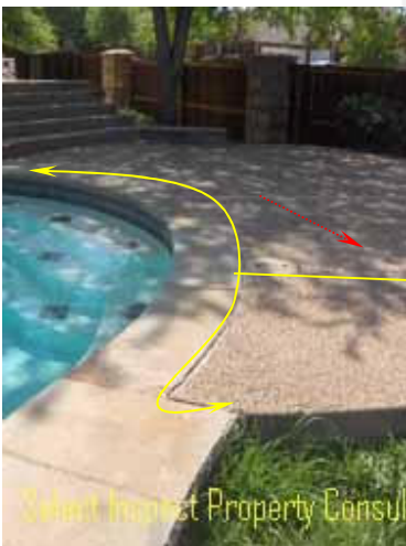
↑ deck has settled downhill
