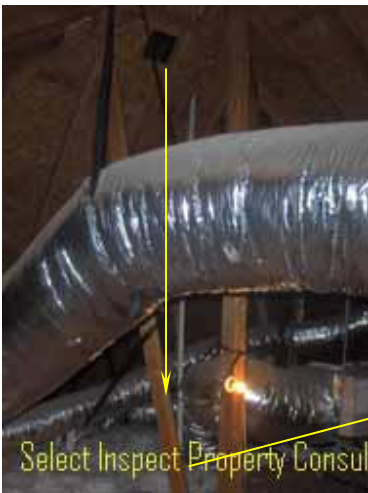
↑ moisture intrusion suspected from roof vent; example
