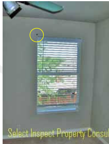
↑ cracks discovered at north bedroom
