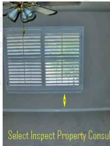
↑ cracks (crack repair evidence) discovered at west bedroom
