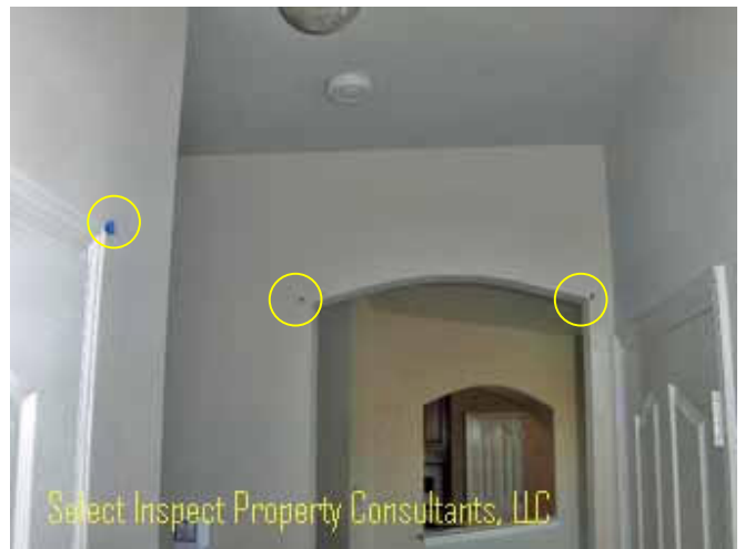
↑ cracks discovered at downstairs hall
