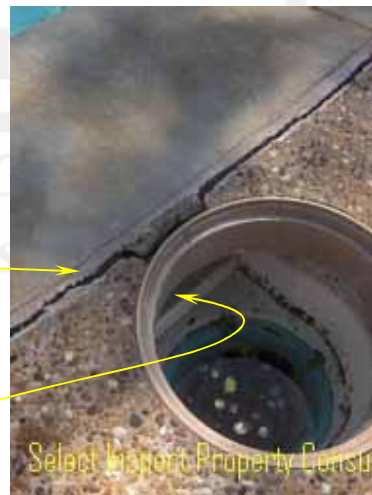
↑ separation of pool coping & deck/skimmer; close view of image at left
