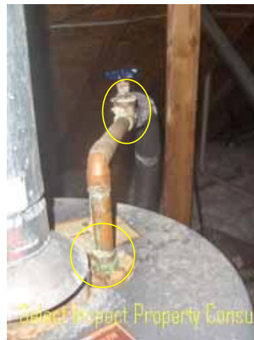
↑ seepage & corrosion at the water heater connections
