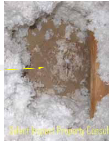
↑ moisture damage & fungus below insulation at ceiling drywall
