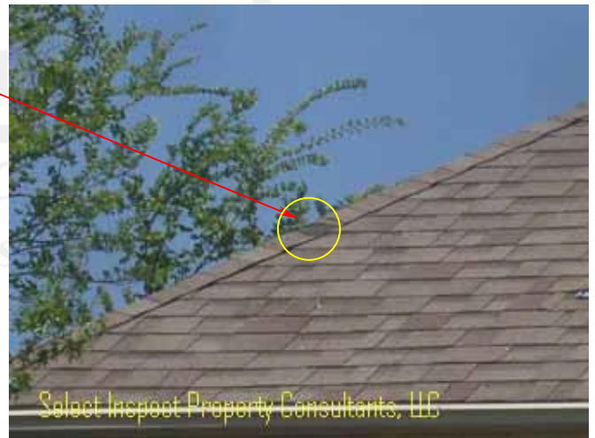
↑ close view of image above
