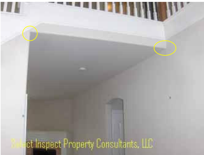
↑ cracks discovered at loft
