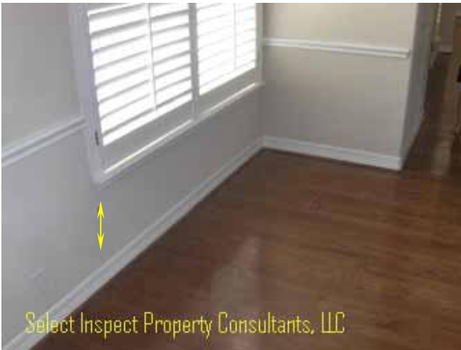
↑ cracks discovered at living room
