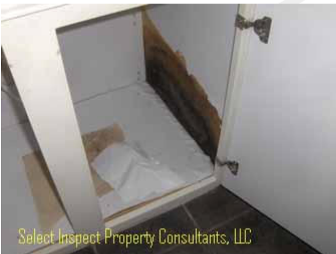
↑ moisture damage & fungus below downstairs bathroom cabinet
