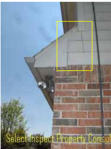
↑ exterior stress; garage east corner
