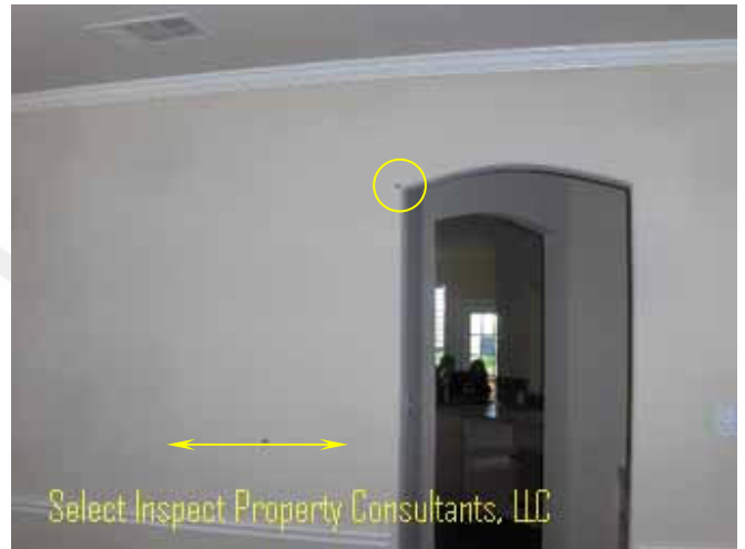
↑ cracks discovered at dining room
