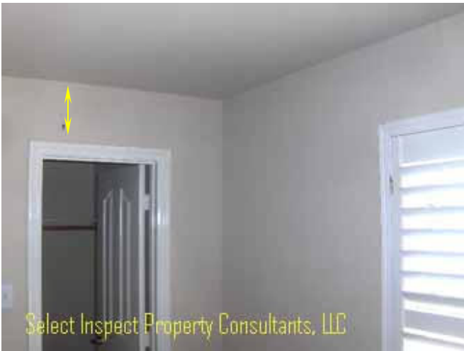
↑ cracks discovered at south bedroom
