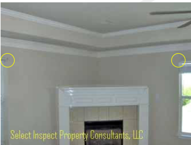
↑ cracks discovered at master
