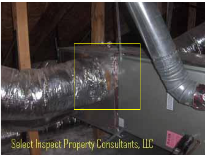
↑ energy loss at HVAC; example poor duct/plenum connections
