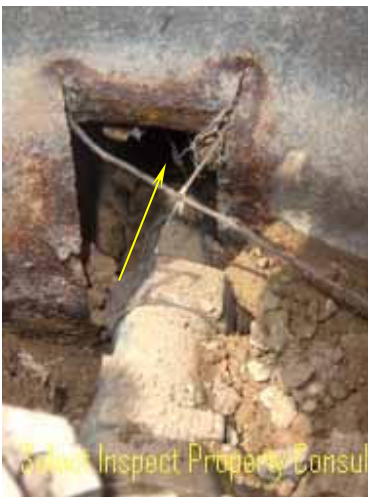
↑ water supply broken/disconnected adjacent the meter
