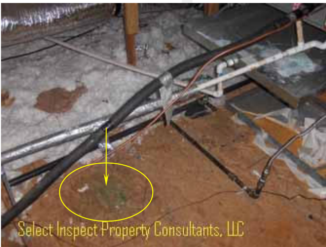
↑ green moisture staining implies copper, indicating refrigerant pipe insulation deficiency
