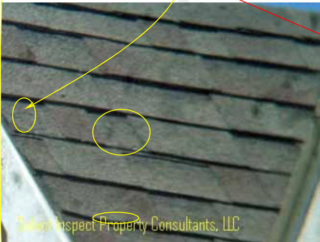
↑ close view of image above; weather damage
