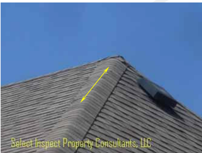
↑ damaged ridge at the south (front right when facing the house)
