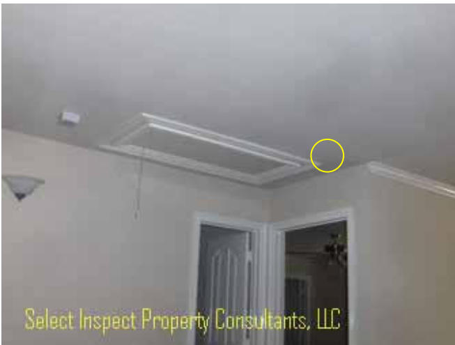
↑ recommend smoke detectors at halls directly adjacent the bedrooms; example at south bedroom hallway
