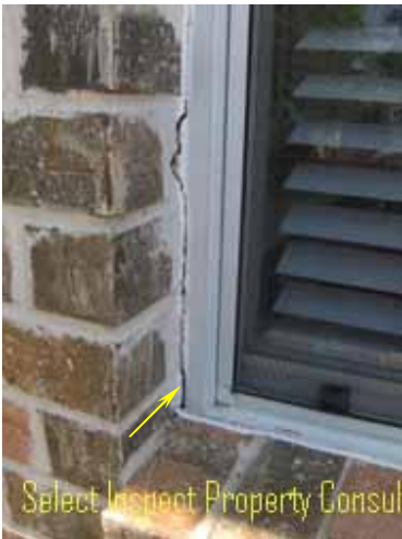
↑ window separation from brick veneer- indicates structural stress; example at breakfast nook
