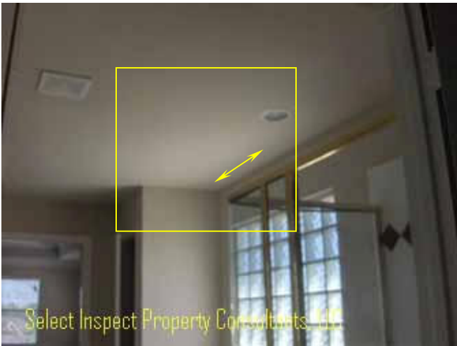
↑ Thermal imaging implies energy loss at the master bathroom
