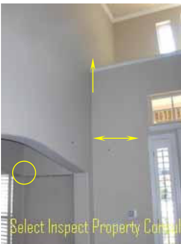
↑ cracks discovered at entry
