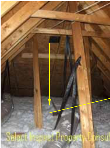
↑ moisture damage & fungus; attic above master
