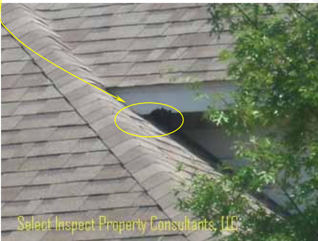
↑ close view of image above shingle damage & rodent damage
