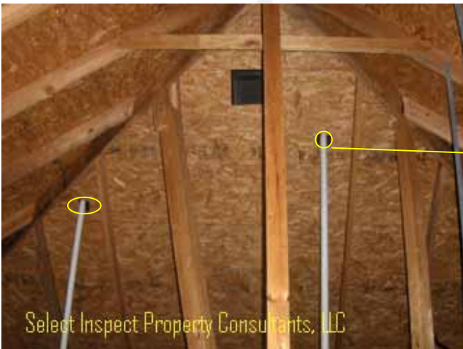
↑ moisture intrusion from deficient vent collars; example
