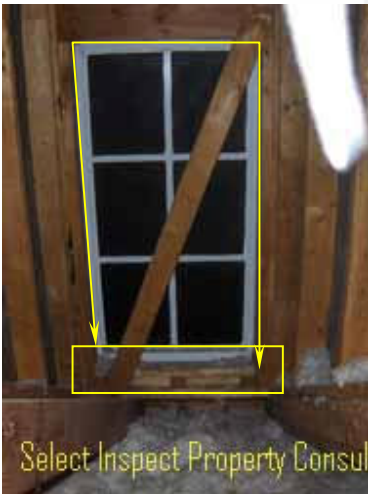
↑ missing master bathroom flashing at attic (dormer) windows; interior windows undetermined due to drywall
