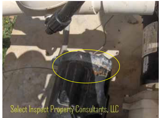
↑ corrosion at pool pump
