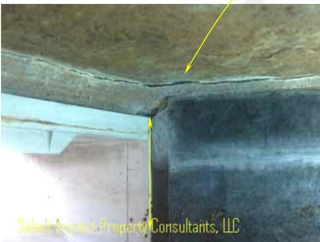
↑ cracks; holes at skimmer interior may allow leakage from the pool
