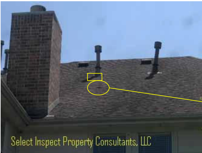
↑ raised flue flashing & deficient shingle
