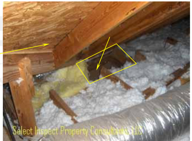
↑ cracks not discovered at framing in the attic; missing insulation was noted-not related to deflection
