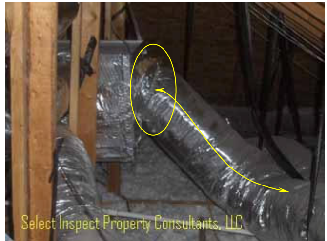
↑ inadequate support of air ducting; example-deficient connection to plenum; energy loss- upstairs HVAC
