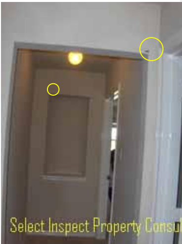
↑ cracks discovered at master hall
