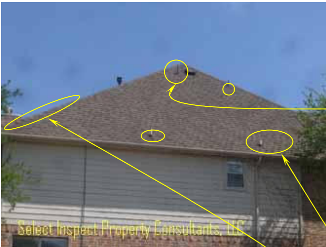
↑ damaged plumbing vent collars, damaged shingles, unpainted vent stacks
