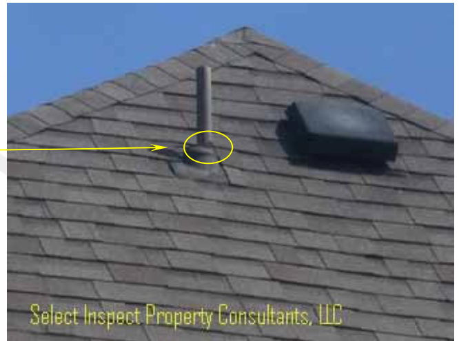
↑ damaged vent collar; example
