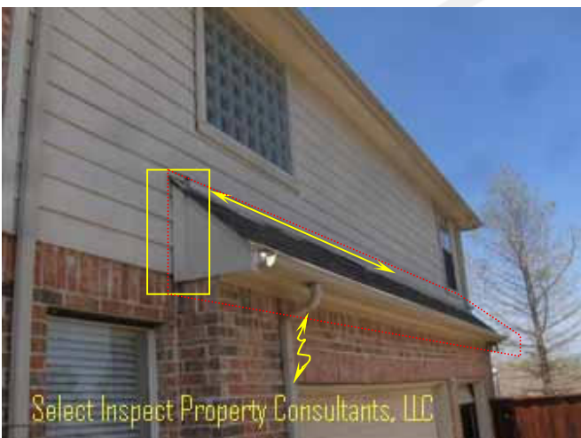
↑ openings (square); crack with differential movement & garage frame separation from adjacent brick; inadequately secured siding & raised flashing edge (upper arrow); unvented enclosed attic space (red)
