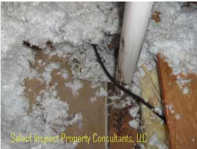
↑ moisture damage & fungus at framing & ceiling drywall- below image above also rodent feces discovered at this location
