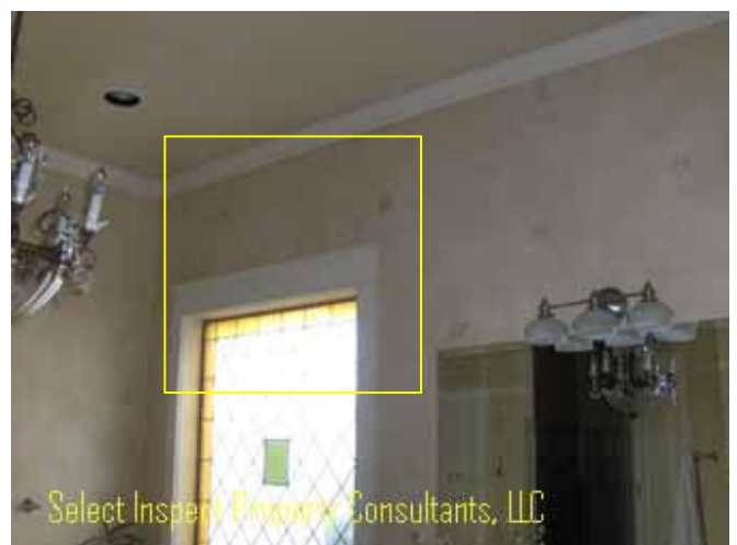
↑ Thermal imaging shows energy loss & or moisture at master bathroom window area
