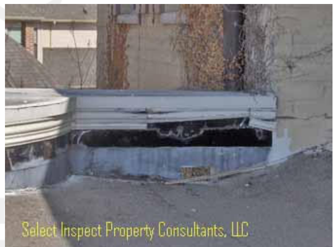
↑ moisture damage & aged roll roofing; front porch
