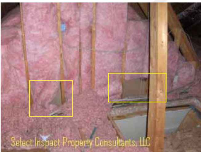
↑ example deficient insulation at upstairs bedroom south
