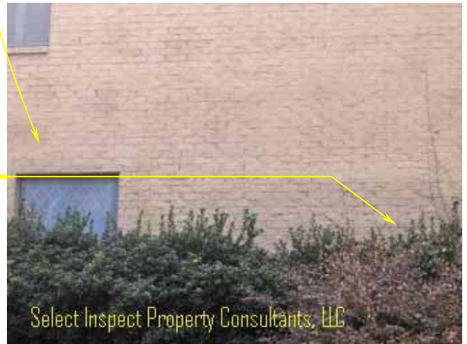
↑ diagonal/step cracks & horizontal crack(s)
