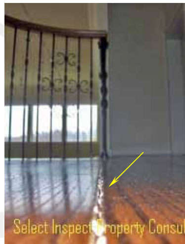
↑ close view of image at left; suspect moisture intrusion & swelling of subfloor framing
