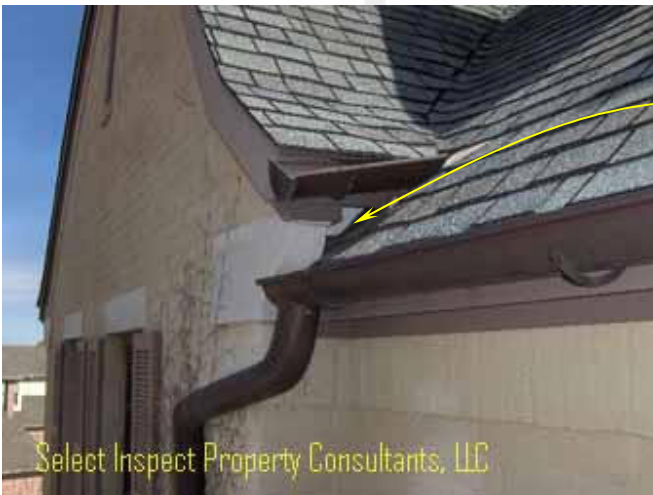
↑ deficient gutters & openings/unworkmanlike flashing; example at front porch left
