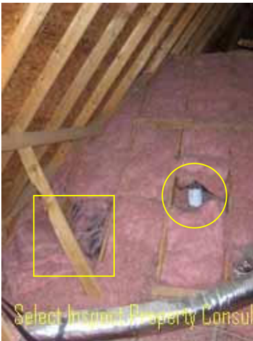
↑ example deficient insulation above family room east
