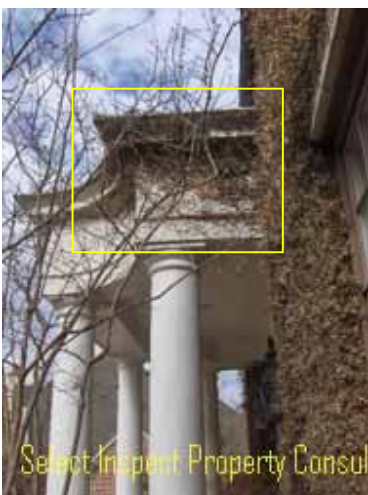
↑ moisture damage & fungus exists at the front porch components; example right side
