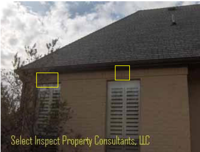
↑ stress cracks at the guest bedroom east
