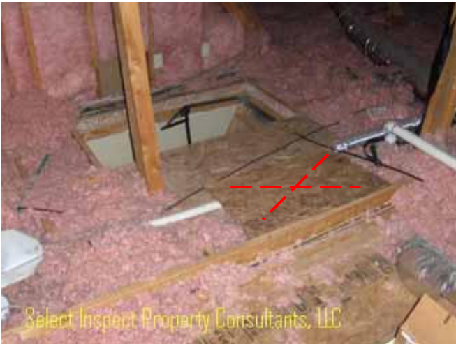
↑ there should be a minimum 24" pathway to the HVAC from the top of the access, with no gaps or obstructions; electrical wires/cables shall not be routed along walking surfaces or in any location prone to traffic damage; soft floor may be a trip risk (red "X")
