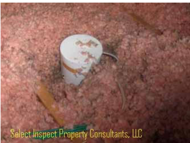
↑ recessed lights require minimum 3" clearance from insulation-per manufacturer label, to avoid overheating & fire hazard conditions; example one of many (all seen were amiss)
