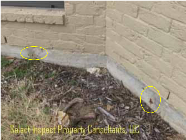
↑ discovered exposed post tension end(s) at the exterior master bedroom
