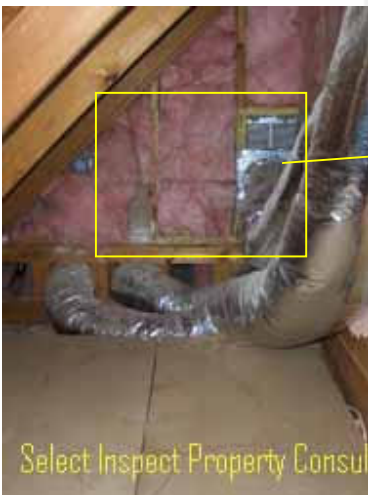
↑ example deficient insulation & unworkmanlike modification of return duct at exercise room south
