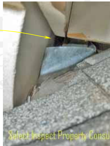
↑ close view of image above-behind cast stone; openings & moisture damage- suspect moisture intrusion exists
