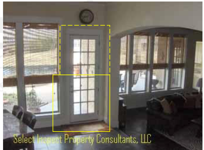
↑ Thermal imaging implies energy loss at receptacles & switches adjacent exterior walls & at exterior & attic doors; example at breakfast nook patio doorway
