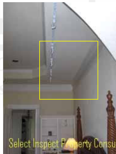
↑ Thermal imaging implies energy loss at master bedroom perimeter & furr down; example at north side of the room
