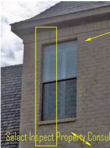
↑ 1/4" +- crack above window, thin cracks below window, & window separation from veneer/frame
