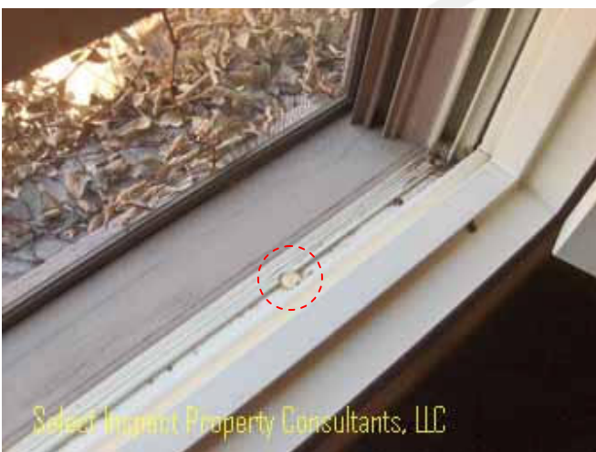
↑ Alarm holes at the lower portion of the window may allow moisture intrusion; caulk, maintain, and monitor
