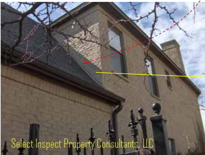
↑ flashing gap implies suspect deflection at roofline or wall stress
