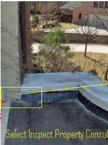
↑ deficiency flashing & openings; front porch right
