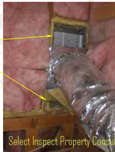
↑ close view of image at left; return is pulling air from the attic/unconditioned space
