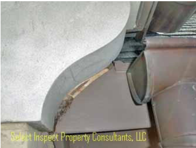
↑ stress, openings, & moisture damage above front porch; left
