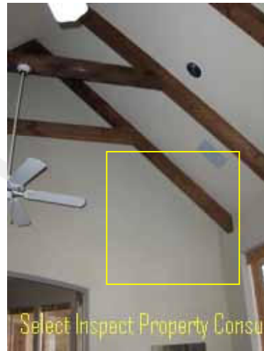
↑ Thermal imaging implies energy loss at family room
