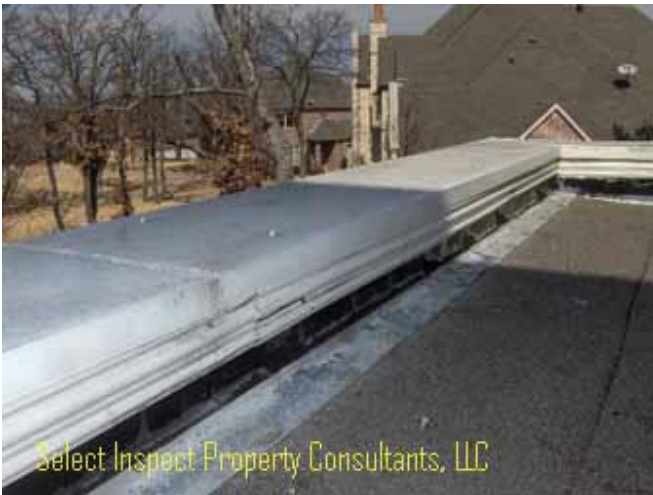
↑ moisture damage & aged roll roofing; front porch
