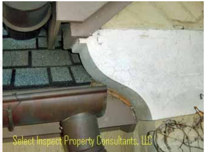
↑ stress, openings, & moisture damage above front porch; right
