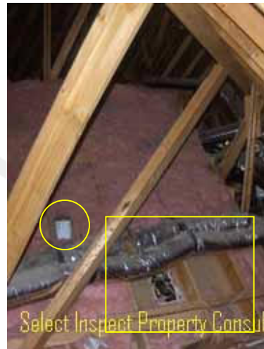
↑ example deficient insulation & location adjacent moisture staining above family room east
