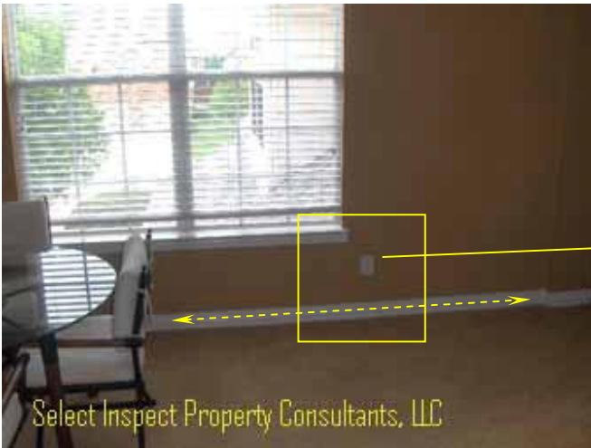
↑ example of slight energy loss at receptacle & sill plate
