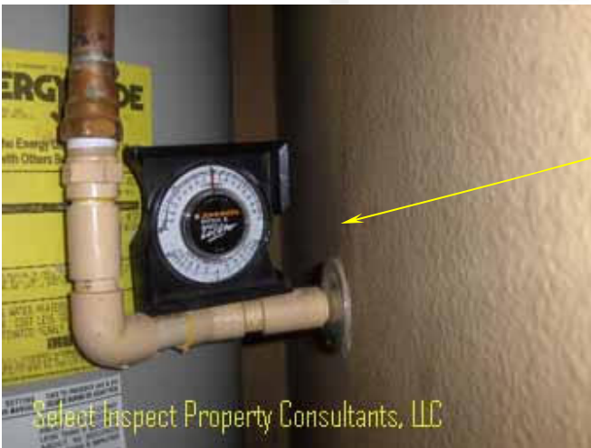
↑ temperature/pressure relief drain improperly routed uphill at this section
