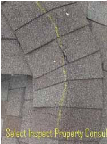
↑ example ridge/hip shingle cracks
