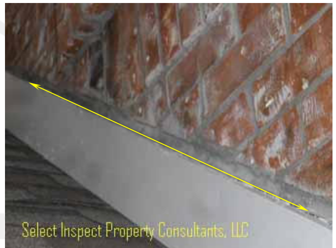
↑ deflection implied by mortar & flashing separation
