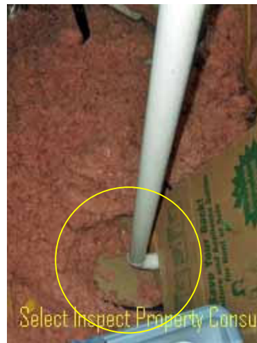
↑ moisture intrusion evidence above image at left
