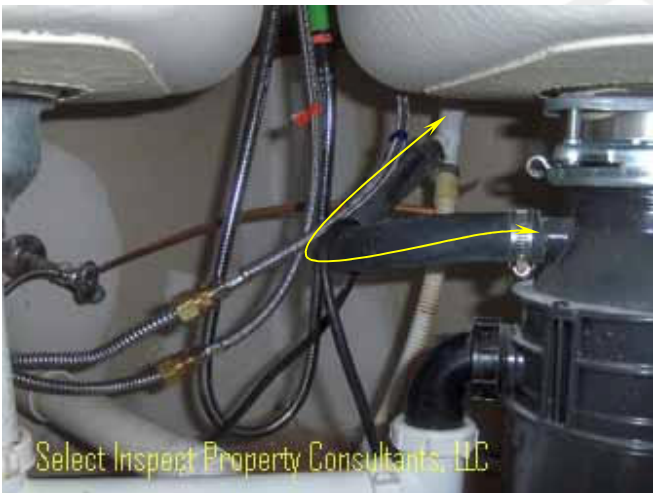
↑ dishwasher drain not appropriately routed for backflow protection
