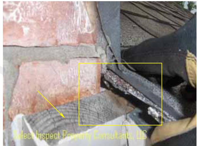
↑ openings; inadequate seal at master bedroom east-northeast
