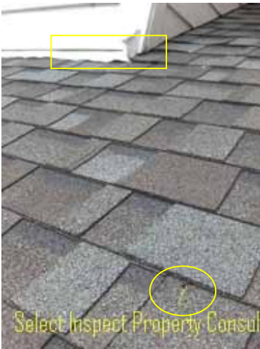
↑ deficient shingle fastener & raised flashing (moisture intrusion noted below in garage)
