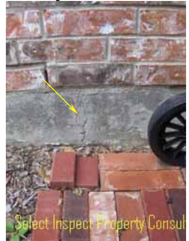
↑ slab crack discovered west
