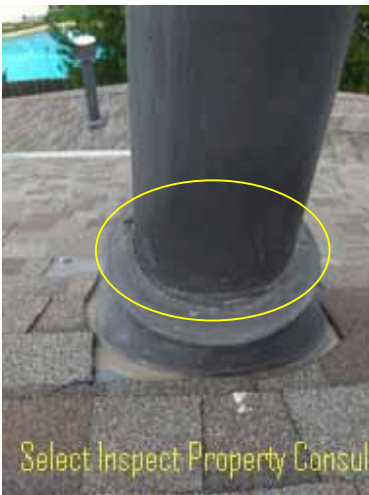
↑ openings at fireplace flue rain shield
