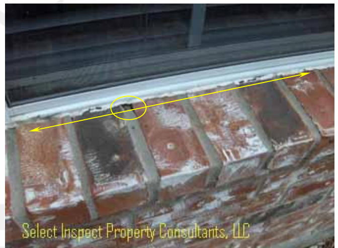
↑ openings & stress evidence at window sill
