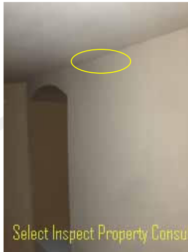
↑ moisture damage discovered at family room below image at left
