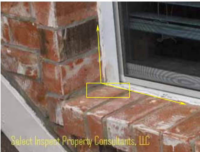
↑ cracked sill & window/veneer stress
