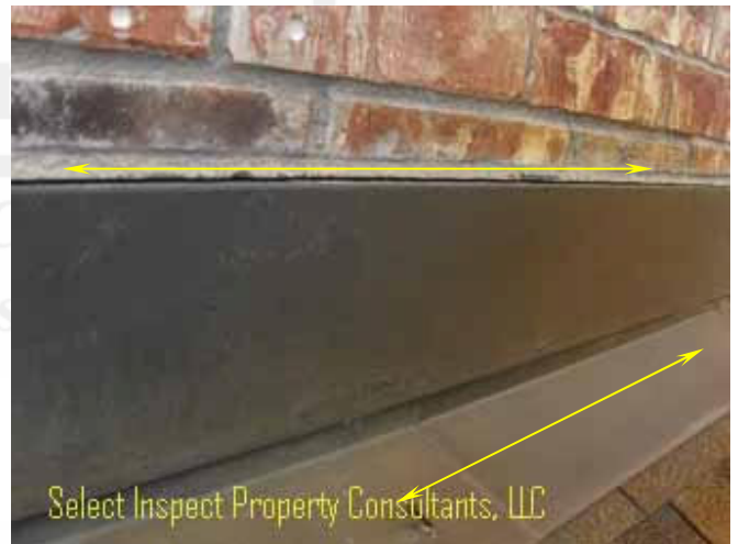
↑ unsealed counter flashing & uncaulked, exposed fasteners; example at master bathroom small roofs
