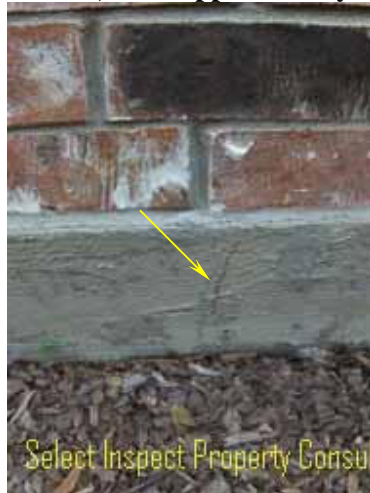
↑ slab crack discovered west
