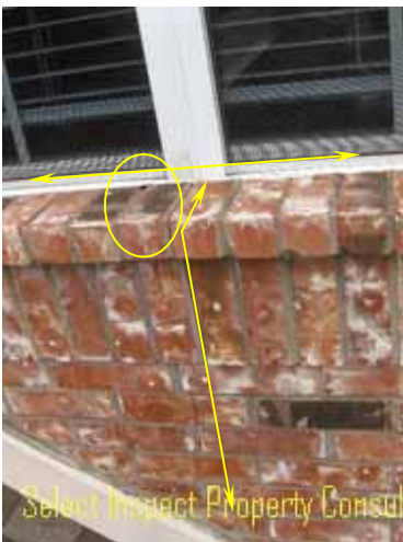
↑ cracked brick & or mortar & cracked sill & window/veneer stress & openings
