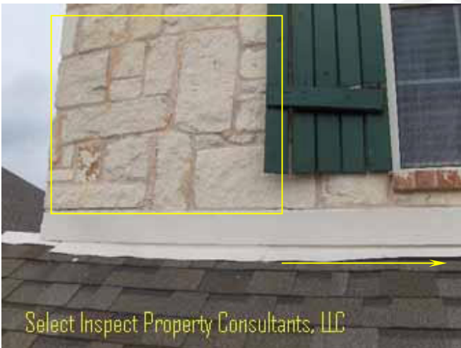
↑ stress cracks & mortar repair history with new cracks & lifted flashing
