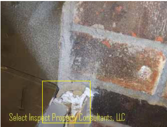
↑ inadequate seal at master bathroom small roof corners example
