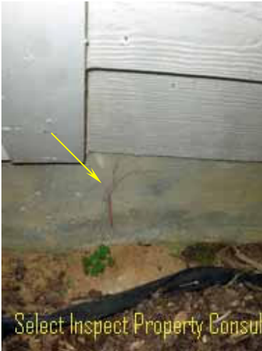
↑ slab crack discovered-east 1 of 2
