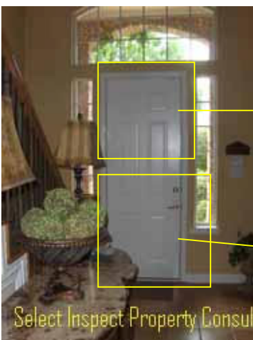
↑ Thermal imaging implies energy loss at front doorway
