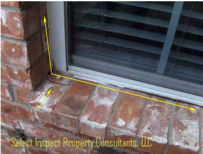
↑ cracked sill & window/veneer stress & deficient window moisture barrier/flashing
