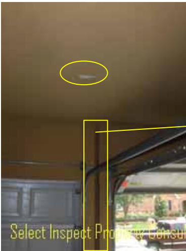
↑ moisture damage & garage drywall deficient; separation provisions compromised
