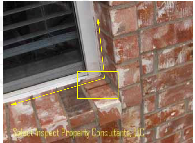
↑ cracked sill & window/veneer stress
