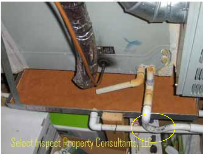
↑ rust at evaporator(s) auxiliary pan & air conditioning primary condensate drain should be insulated; fungus at condensate trap
