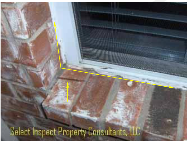
↑ cracked sill & window/veneer stress
