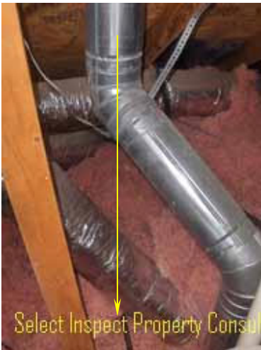
↑ moisture intrusion discovered around fireplace flue
