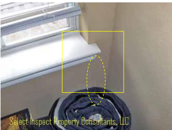
↑ moisture staining at northwest bedroom below window
