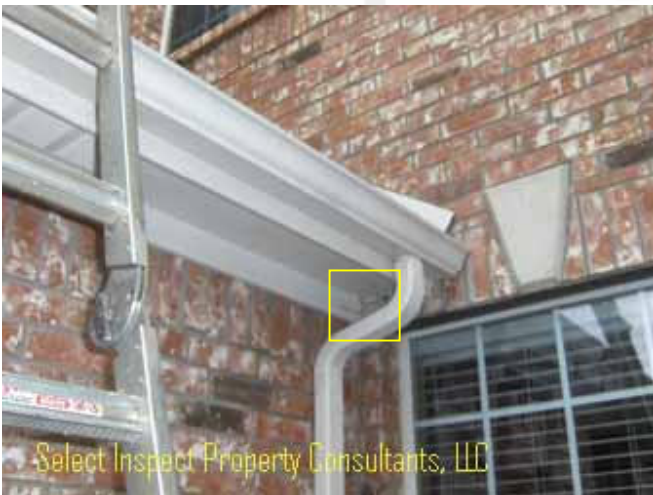
↑ moisture damage discovered at frieze-board left of front porch
