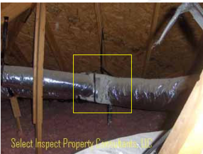
↑ significant energy loss not discovered at air ducting; some manifold joints lose some due to compression at connections
