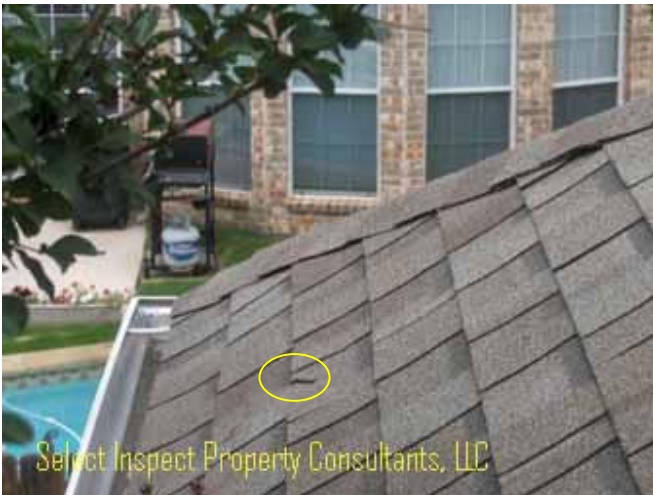
↑ damaged shingle at north
