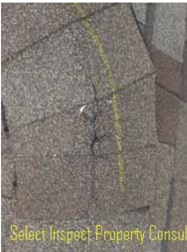
↑ example ridge/hip shingle cracks
