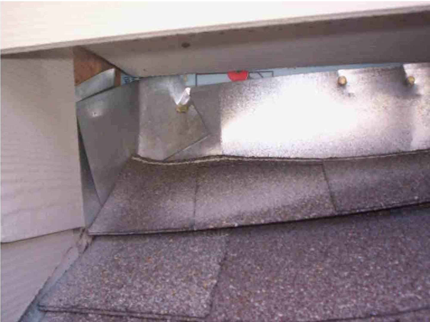
↑ eave under west side of chimney remains amiss / deficient.
