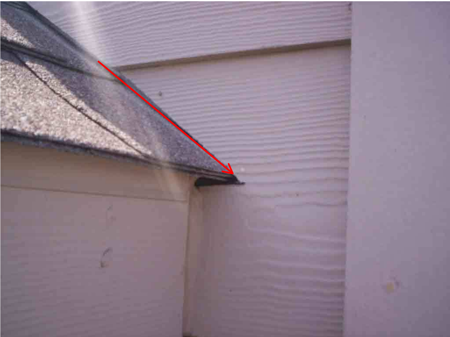
↑ incorrect flashing- eastern side of chimney. water (rain) can be directed behind the siding, into the structure interior.
