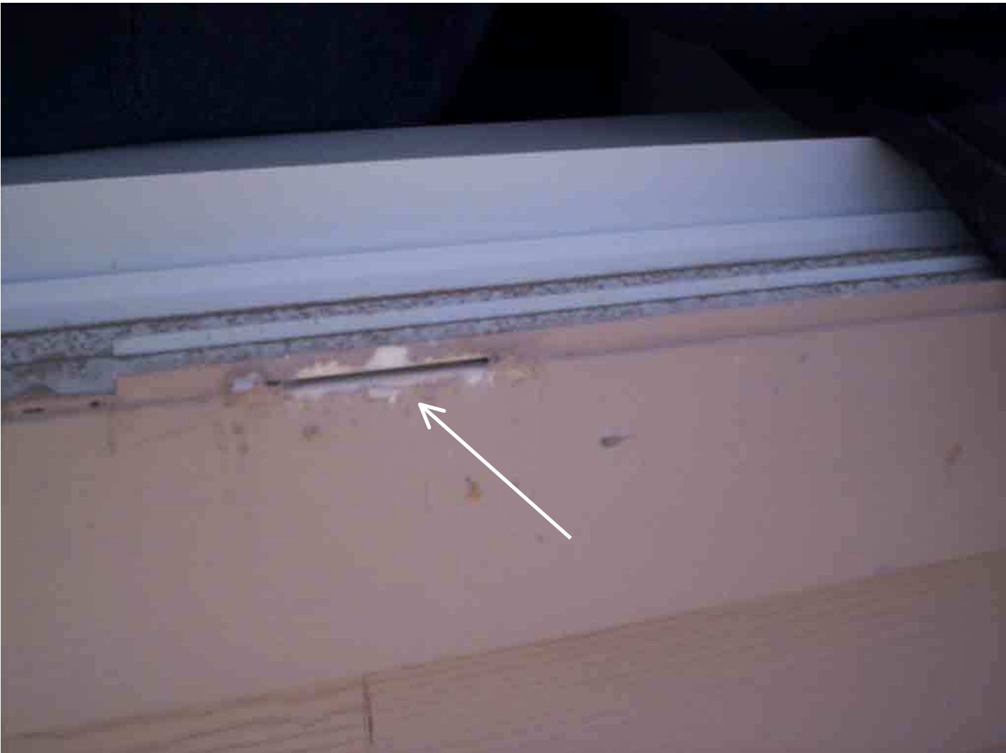
↑ caulk touch-up needed at window above rear patio door.
