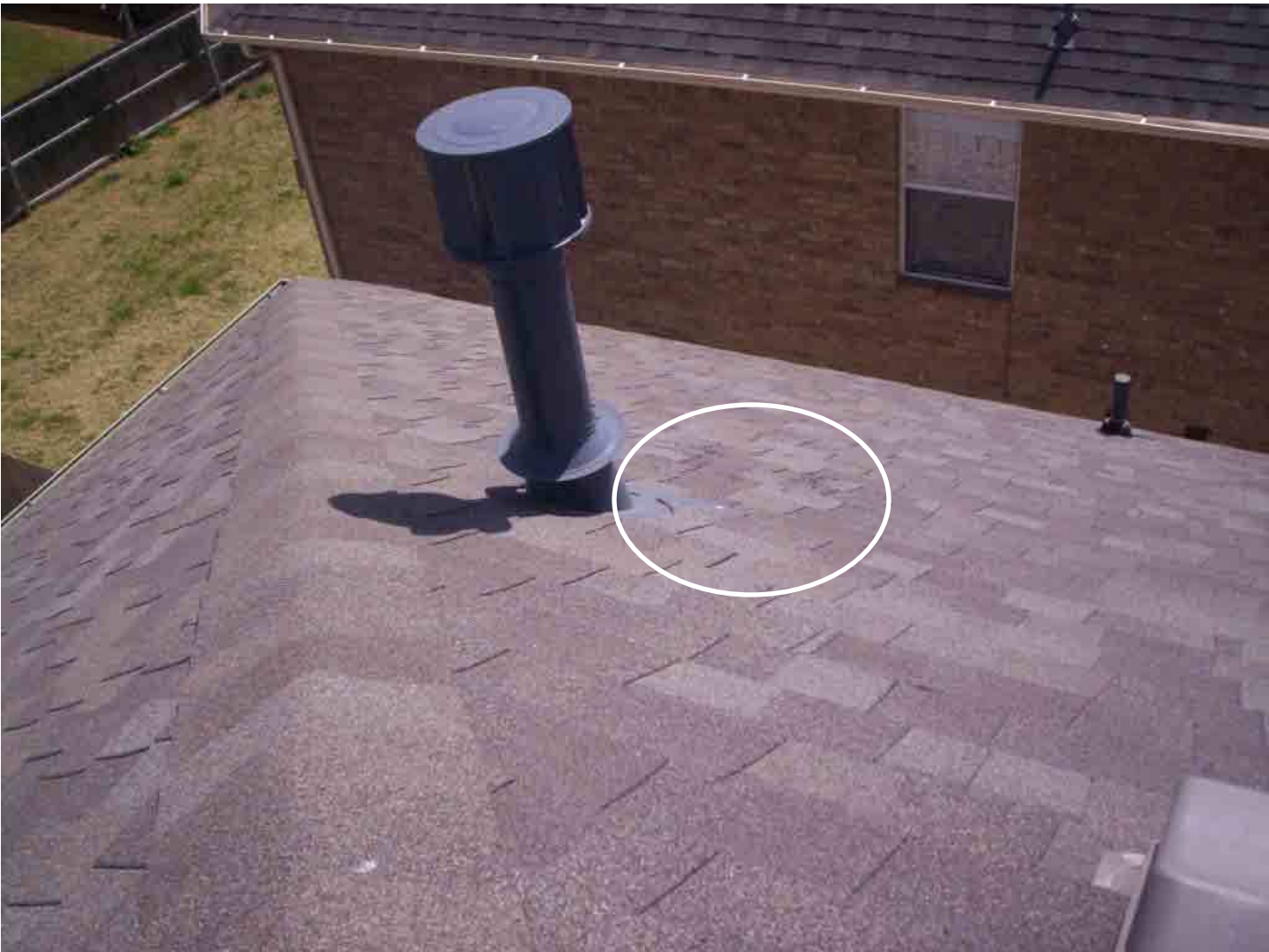
↑ slight worn area at southeast roof. Repair needs were not discovered at the time of inspection.
