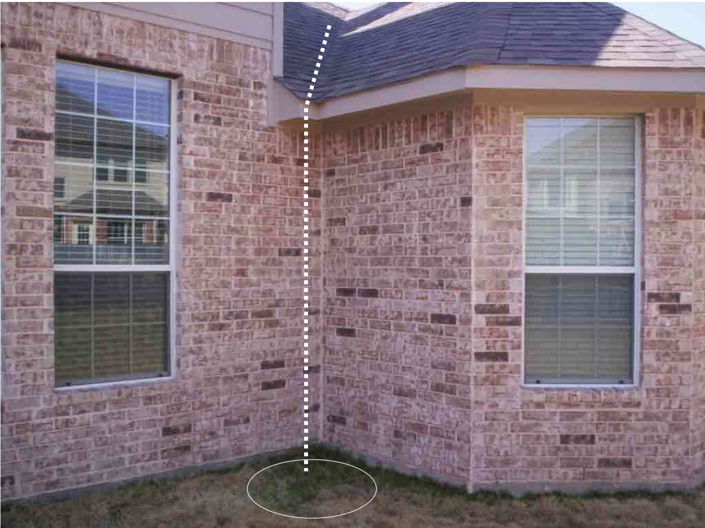
↑ area of erosion noted in the drainage section
