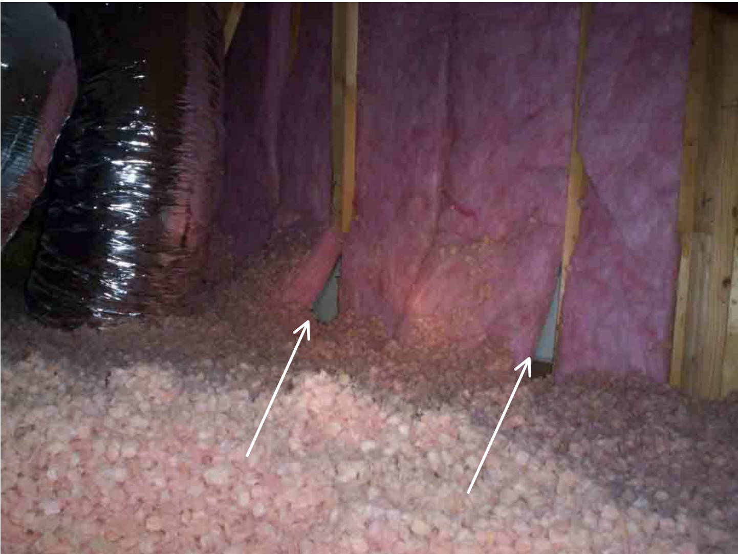
↑ amiss insulation at garage attic –example
