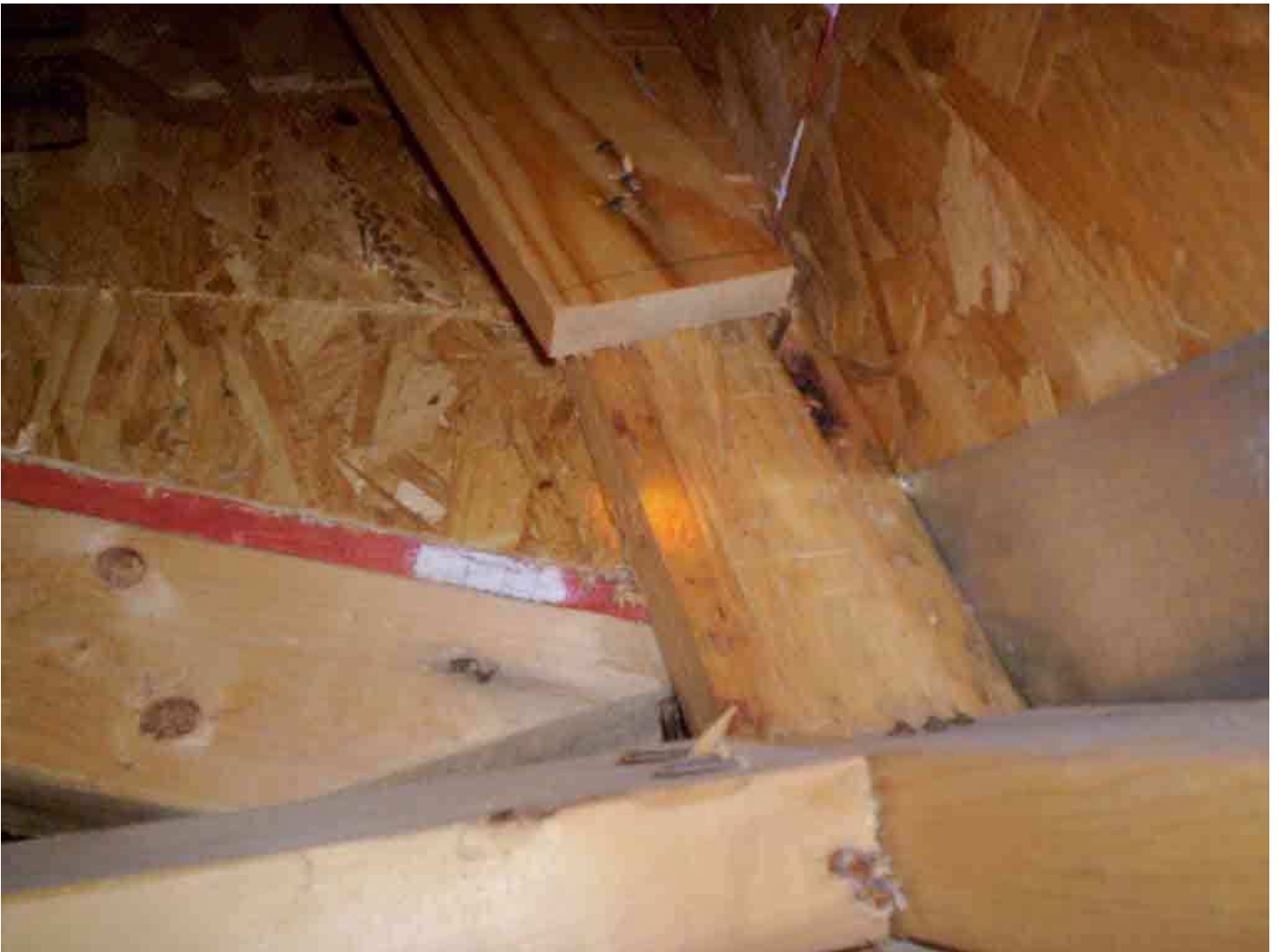
↑ interior view of chimney chase adjacent amiss eave location.
