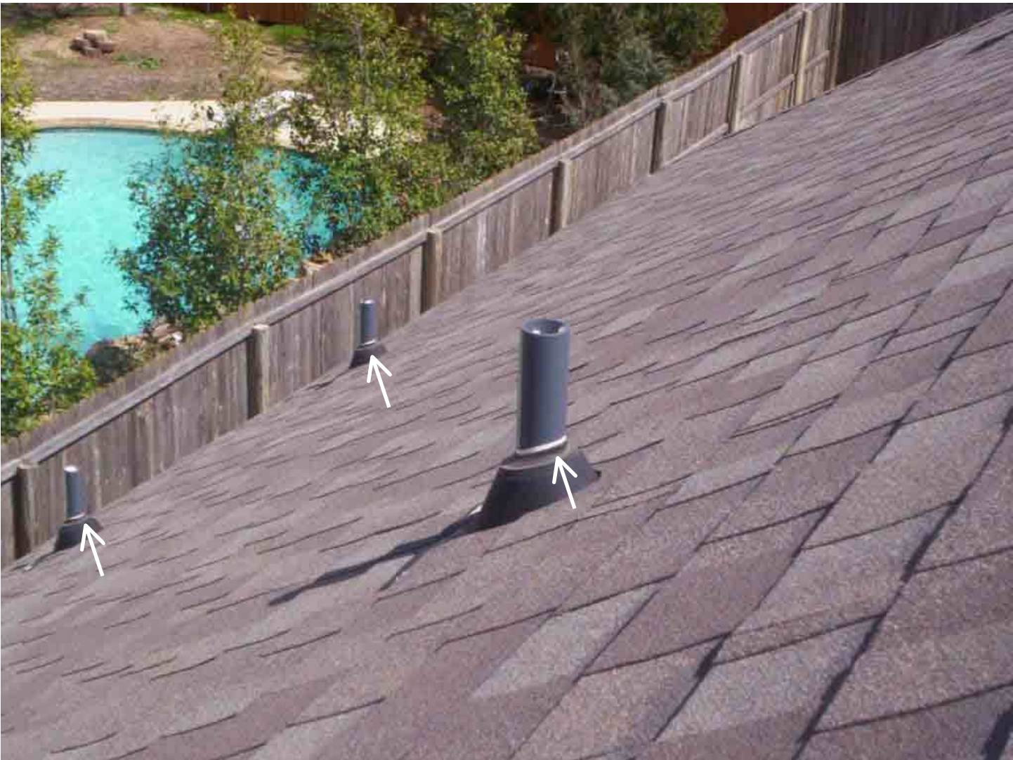
↑ vent separation examples at north
