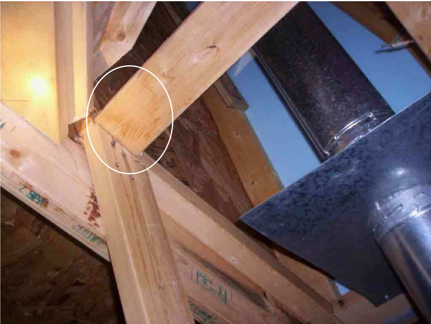
↑ slight staining at chimney framing in attic- when the condition occurred or if it is ongoing is undetermined.
