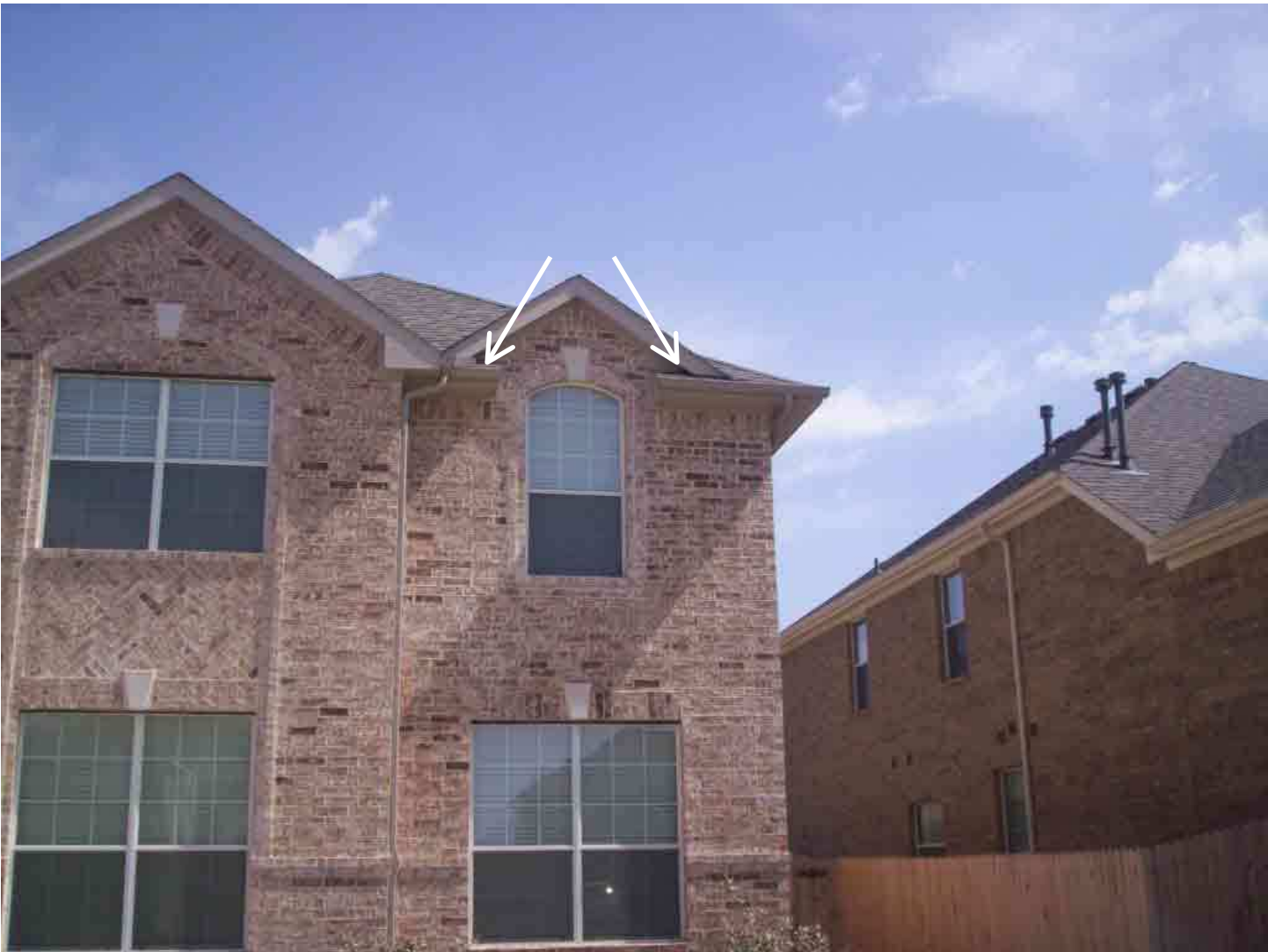
↑ location of uncaulked fasteners discovered.
