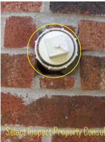
↑ opening should be sealed; northwest
