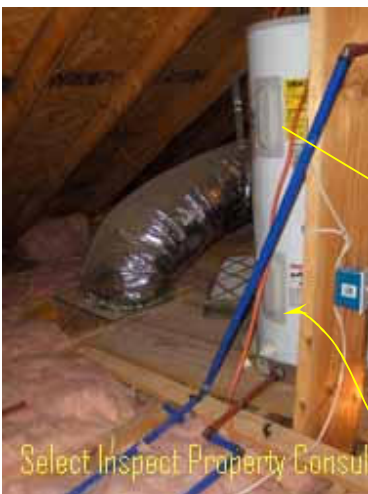
↑ inadequate clearance at service side of water heater
