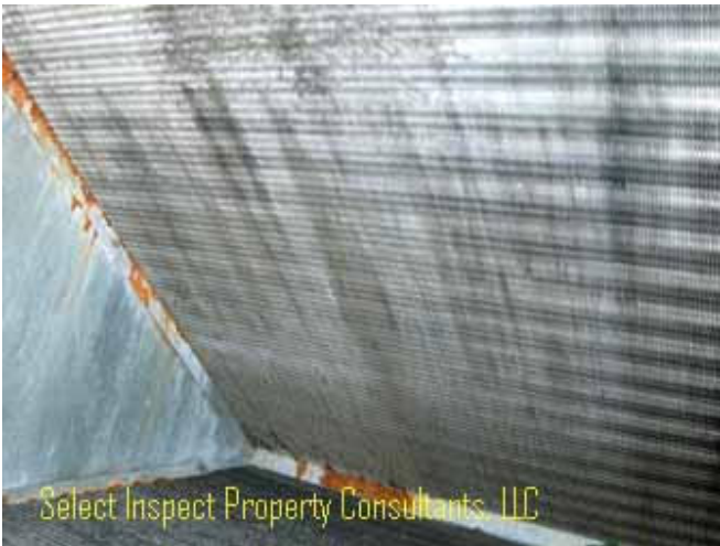
↑ air conditioning evaporator(s) coils should be serviced
