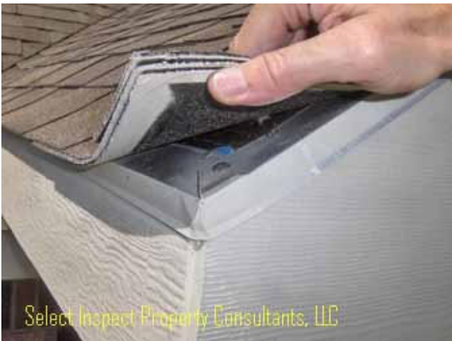
↑ close view of image above; roof underlayment incorrect
