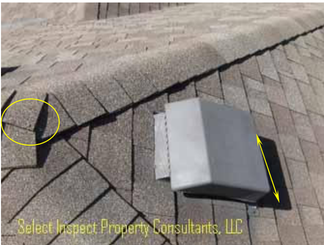
↑ uncaulked, exposed fasteners; example
