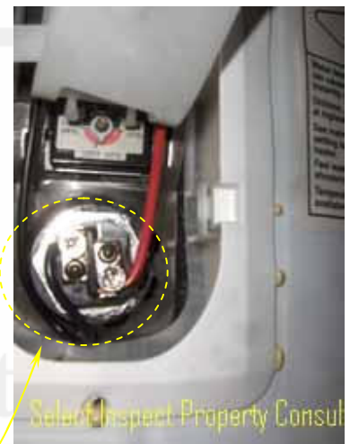
↑ seepage evidence at lower element
