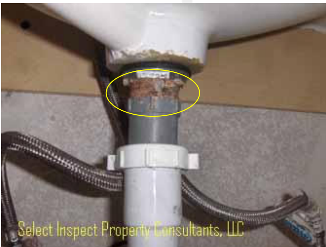
↑ leakage history under bathroom sink; drain stem
