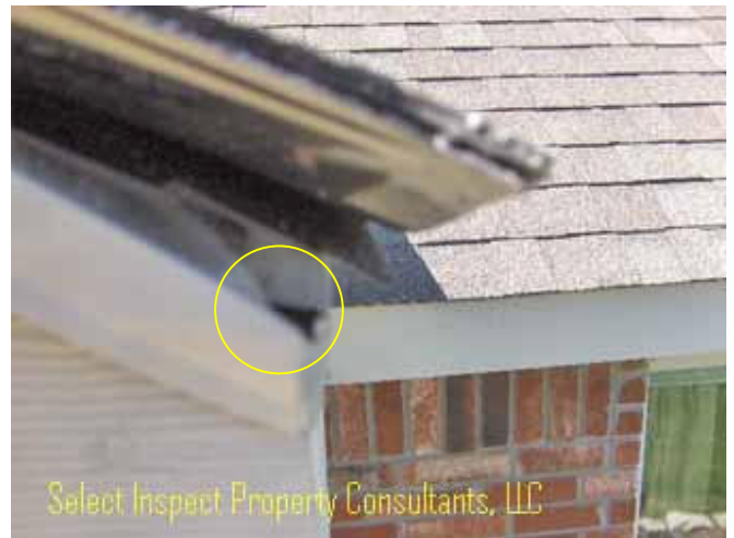
↑ close view of image above roof underlayment incorrect & gap/opening at incorrect drip edge flashing corner
