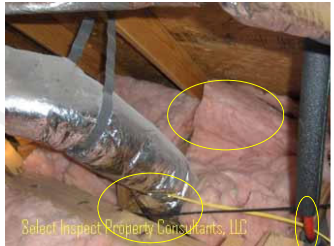
↑ unworkmanlike insulation & "same" deficient insulation at plumbing pipe
