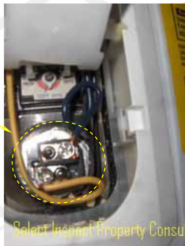
↑ seepage evidence at upper element
