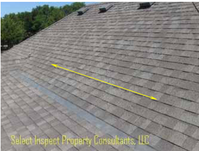
↑ minor damage discovered at rear roof Significant issues were not discovered regarding this specific condition; monitor & maintain
