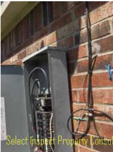
↑ inadequately secured electrical cabinet
