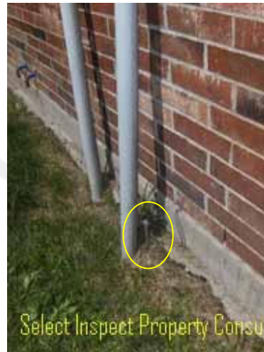
↑ grounding electrode protrudes grade; deficient
