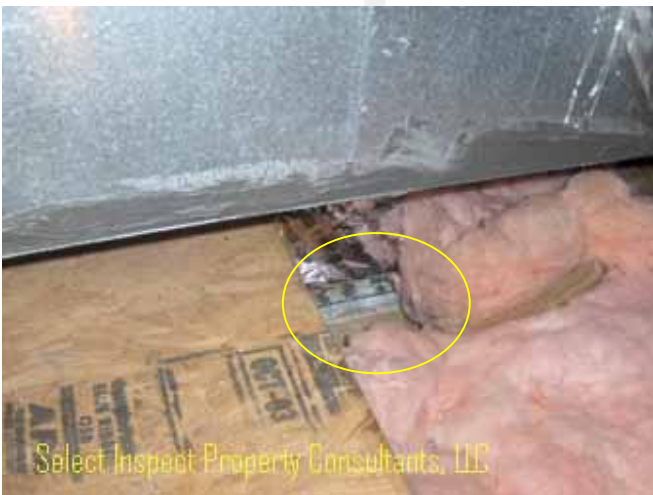
↑ unworkmanlike insulation under HVAC
