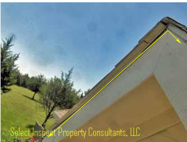
↑ close view of image above; gaps at drip edge flashing/fascia
