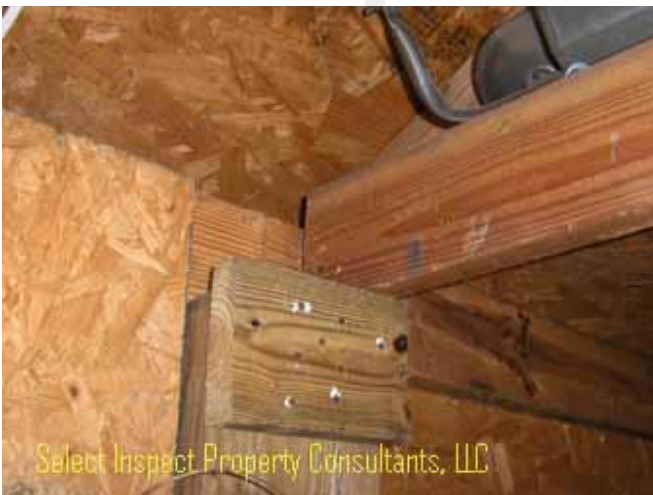
↑ undersized joist; inadequate connections; example
