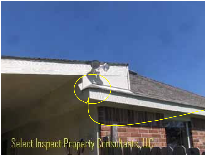
↑ missing/incomplete drip edge flashing
