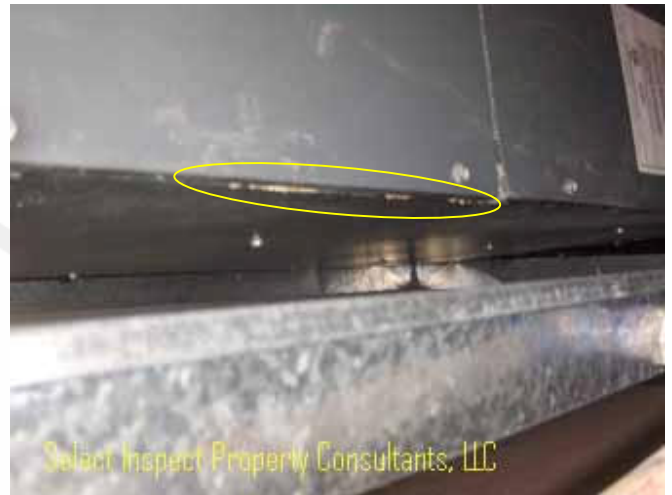
↑ sediment/leakage history at air conditioning evaporator(s) cabinet
