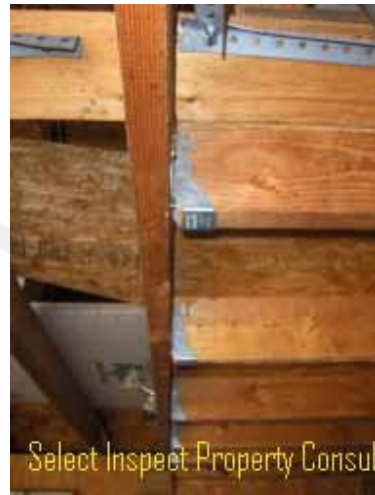
↑ unworkmanlike cut, connection & joist hangers; example
