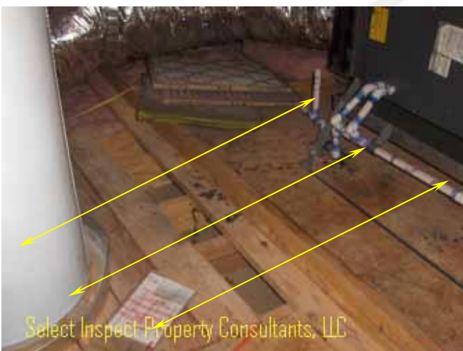
↑ missing insulation under mechanical decks
