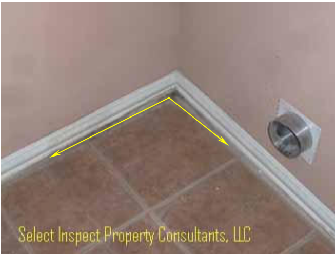
↑ moisture damage & fungus at laundry room baseboard trim
