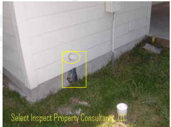
↑ opening should be sealed at plumbing clean-out & exposed piping is prone to freeze damage
