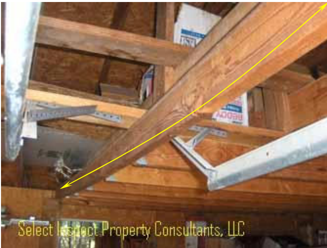
↑ cracks, deflection, undersized framing, & multiple unworkmanlike framing conditions discovered at the garage
