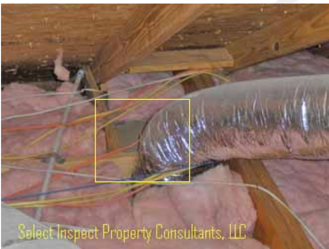
↑ unworkmanlike insulation at the southwest
