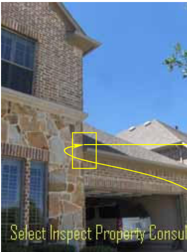
↑ unworkmanlike eave/wall; openings
