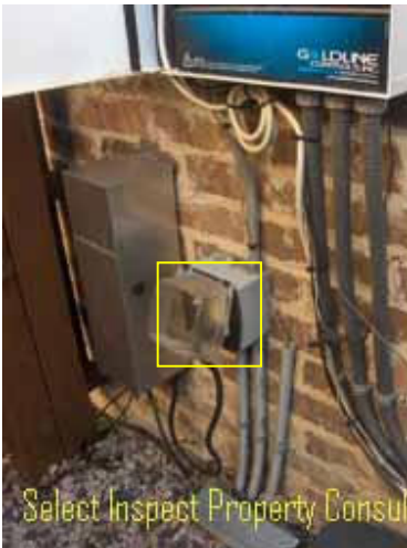
↑inadequate enclosure of electrical at exterior receptacle
