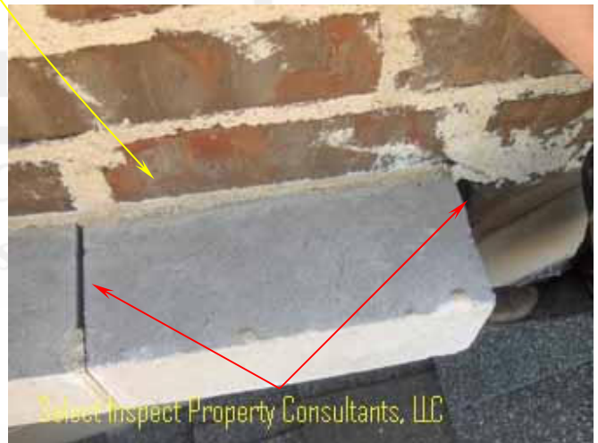
↑ deficient mortar; openings at cast stone ledge
