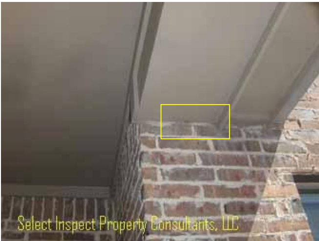
↑ unworkmanlike eave/wall; openings at rear porch; visible framing
