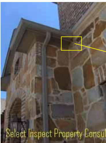
↑ unworkmanlike eave/wall; openings
