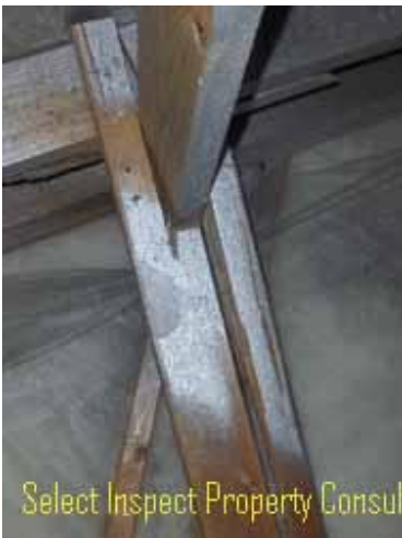
↑ marginal fastening/joints at northwest walk-in attic struts
