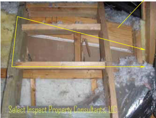
↑ attic view of images above- missing insulation
