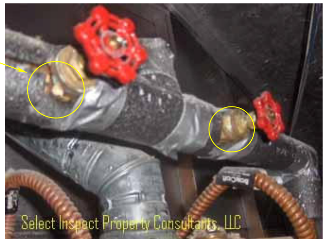
↑ seepage evidence discovered at shut-off-valves
