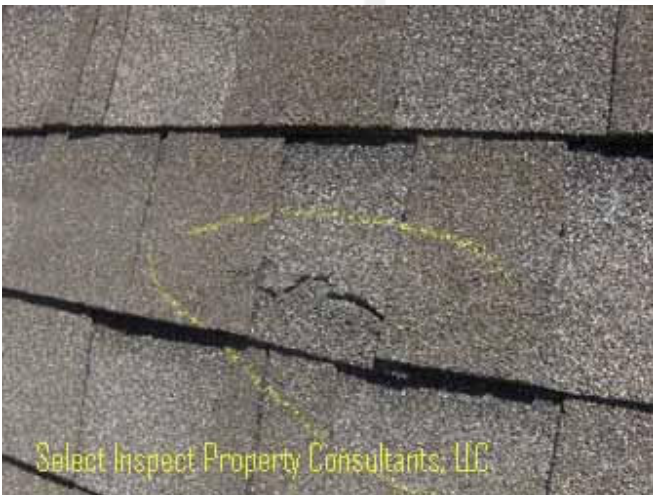
↑ damaged shingle; upper west-northwest
