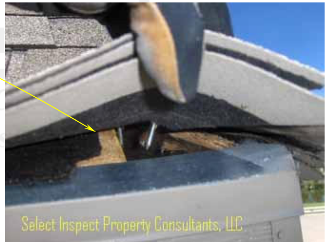
↑ unworkmanlike roof underlayment, openings, missing deck, unsecured roofing
