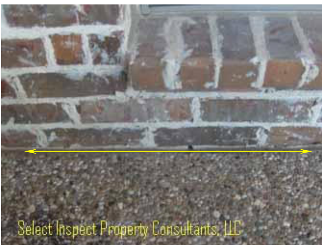
↑ obstructed weep openings at rear porch
