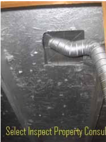
↑ exhaust fan termination at passive vent
