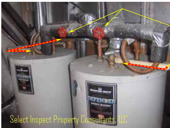
↑ temperature/pressure relief piping was smaller than required by the device manufacturer
