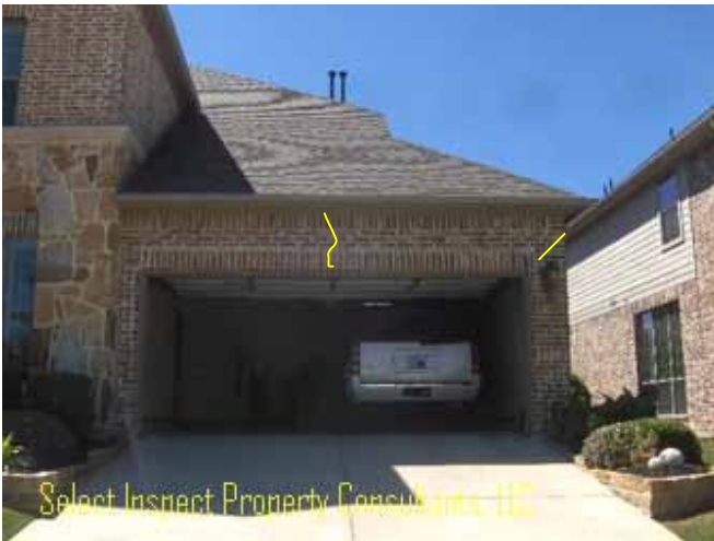
↑ deflection & 1/8" crack at overhead door
