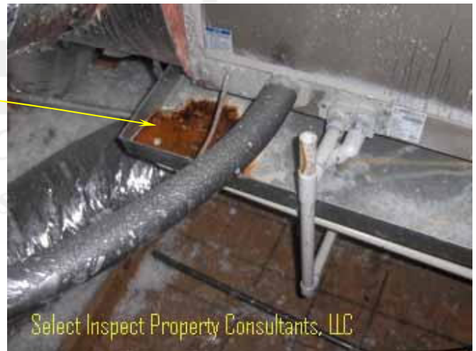
↑ active moisture/condensate in auxiliary pan & some corrosion seen at bottom of evaporator cabinet
