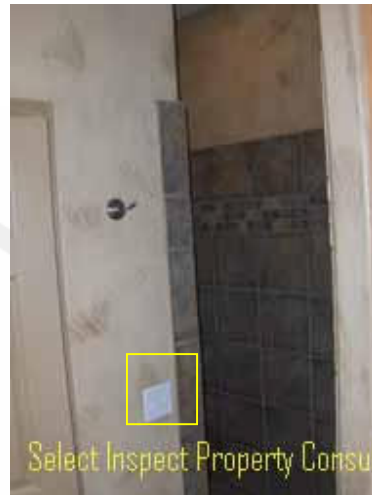
↑ electrical switch within 5' of shower
