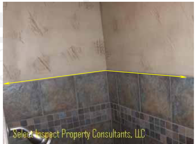
↑ caulking/sealant needed atop shower tile/panels; example
