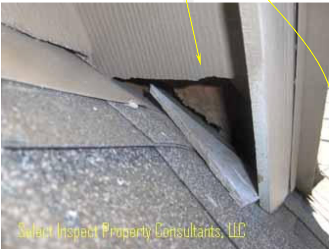
↑ damaged soffit; openings to attic/eave
