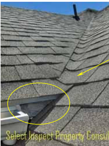
↑ deficient fascia; exposed framing
