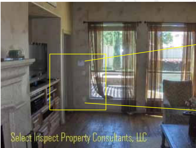
↑ Thermal imaging implies energy loss at pool control & receptacle
