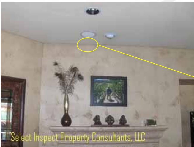
↑ stain ?? or paint variation at family room ceiling
