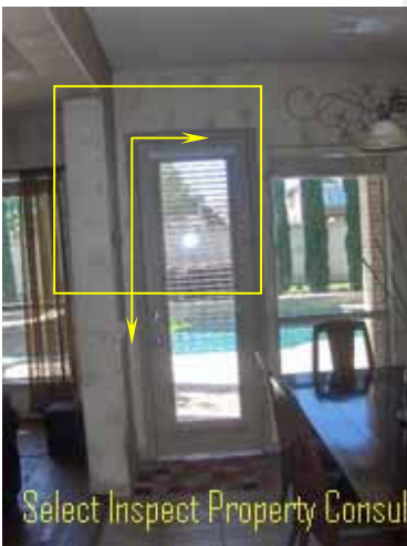
↑ Thermal imaging implies energy loss at framed area around the patio doorway
