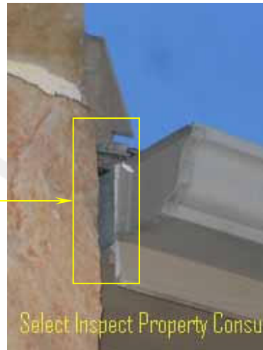
↑ close view of image at left; visible framing, missing fascia/trim, missing drip edge flashing
