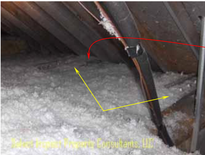
↑ deficient baffles lying on insulation; not secured in position; example in upper northwest attic
