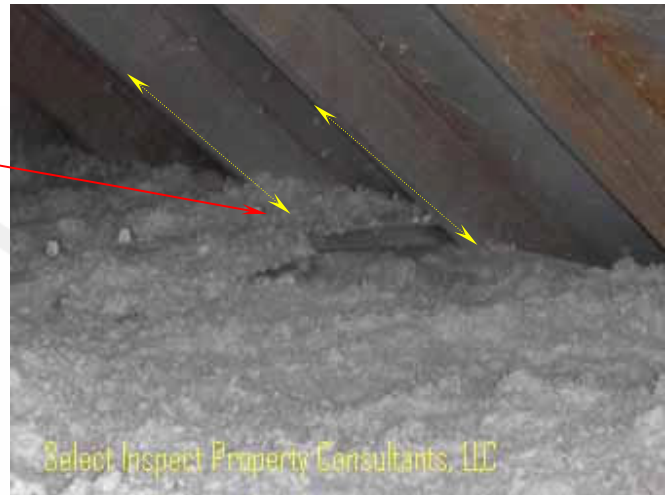
↑ close view of image at left; these should be parallel with the rafters/rafter bays to keep insulation from obstructing eave vents.
