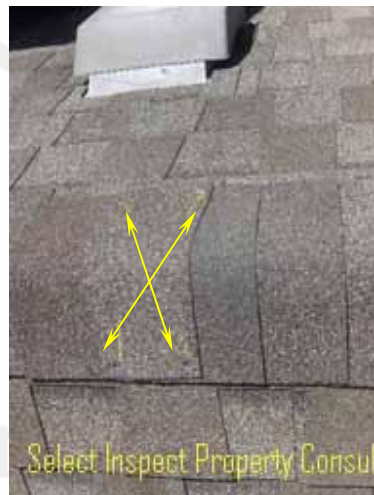
↑ uncaulked, exposed fasteners example at upper roof
