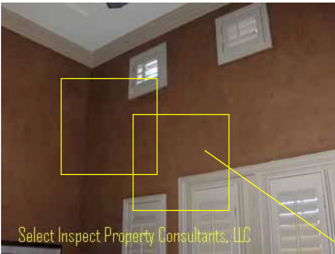
↑ Thermal imaging implies energy loss at the study
