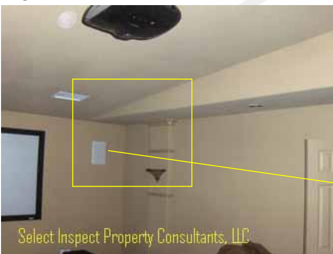
↑ Thermal imaging implies energy loss at media room speaker, & common vault, corner, framing areas; example
