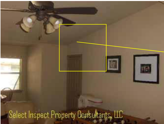
↑ deficient insulation discovered in attic; gameroom northwest
