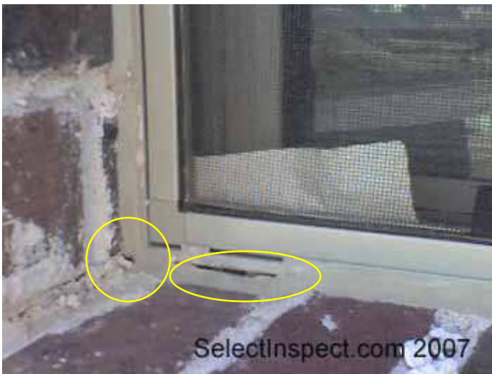
↑ example sealant repair location adjacent window
