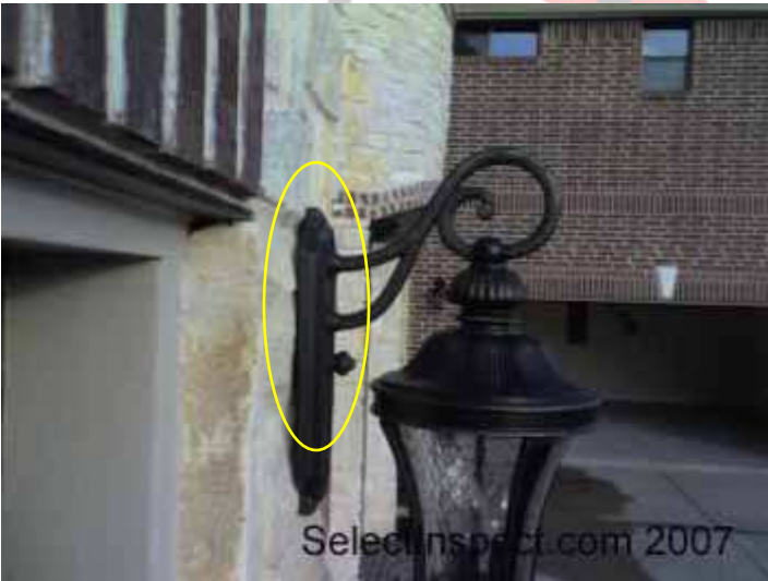
↑ Recommend caulking the top of exterior horizontally mounted lights to prevent moisture intrusion to the electrical conductors – example
