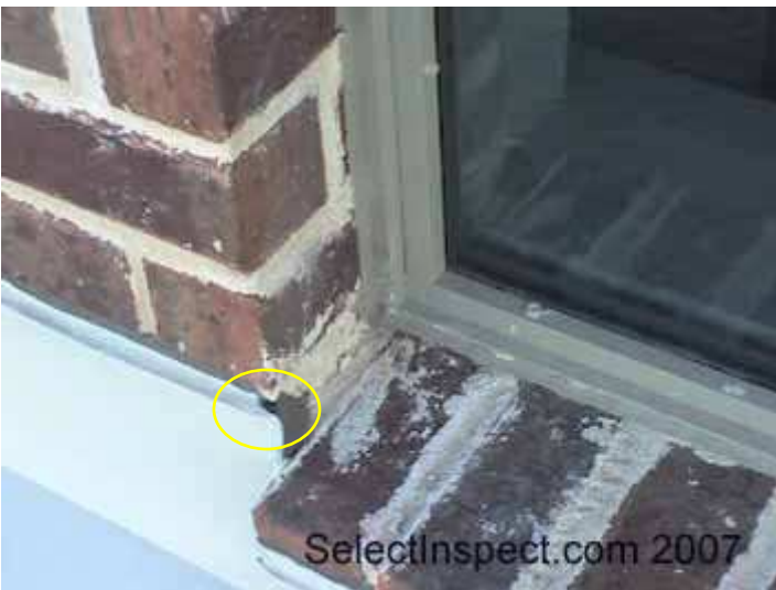
↑ sealant touch-up needed at flashing adjacent upper family room window
