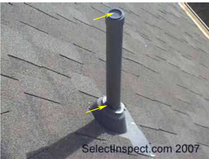
↑ close view of prior image and collapsed vent flange collar
