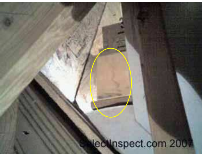
↑ close view- moisture staining/evidence; this may or may not be related to the opening- may be from earlier construction phase- prior to completion of roof.
