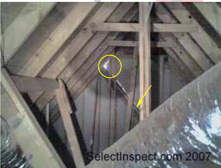
↑ left- daylight visible from attic and moisture staining/evidence; right- unsecured vertical framing
