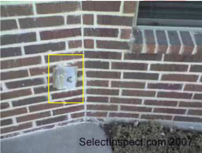
↑ damaged fireplace air intake cover at rear porch
