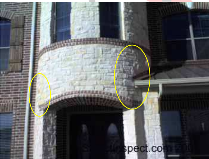
↑ exterior cracks discovered
