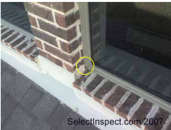
↑ close view of prior image- sealant needing touch-up at corner- upper family room
