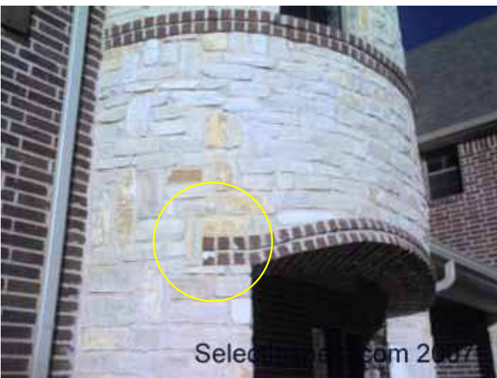
↑ variant tone of mortar implies prior repair
