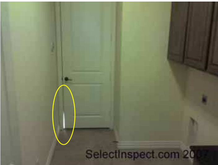
↑ door from laundry room to garage- poor seal and unsquare
