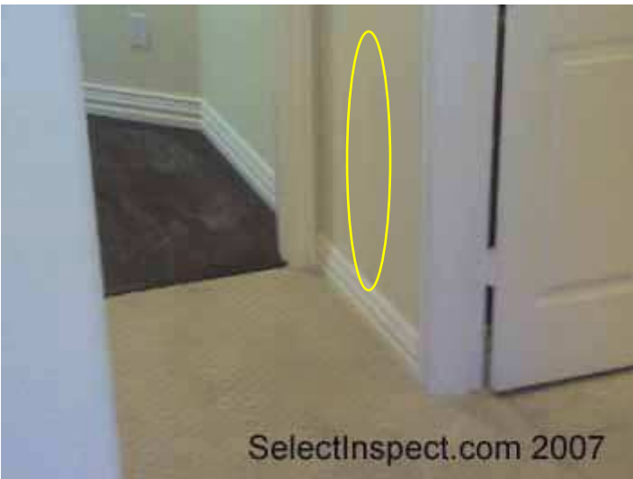
↑ moisture staining/evidence at master bedroom entry
