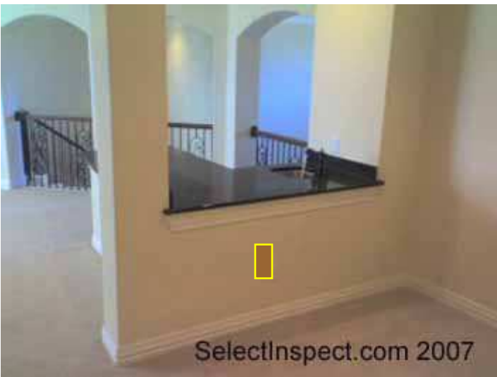
↑ non-GFCI receptacle(s) at bar
