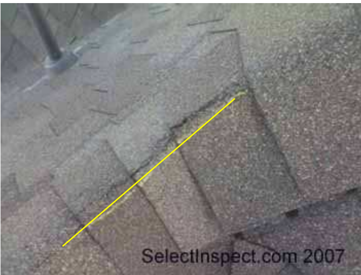
↑ split ridge shingles at roof
