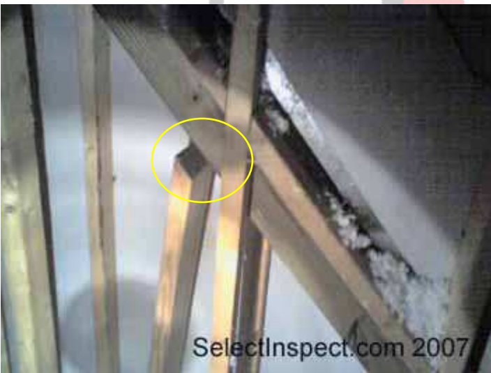
↑ close view- unsecured framing- vertical support
