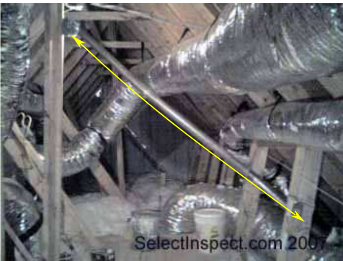
↑ poorly supported water heater flue- southeast attic
