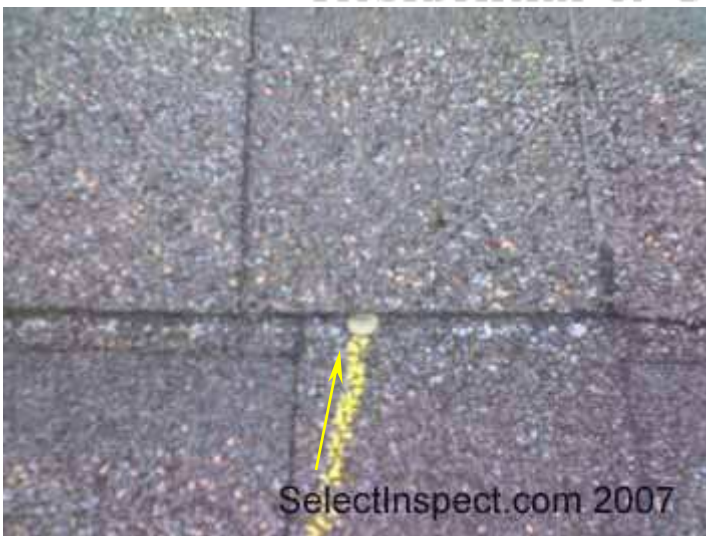
↑ example uncaulked fasteners at roof
