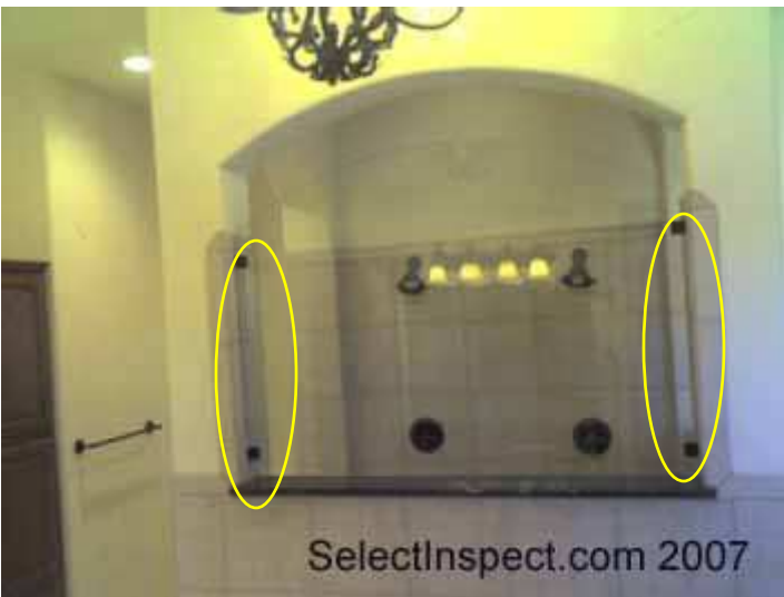
↑ unsealed sides at master shower glass
