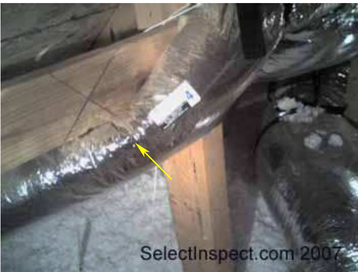
↑ example- crimped air duct in attic
