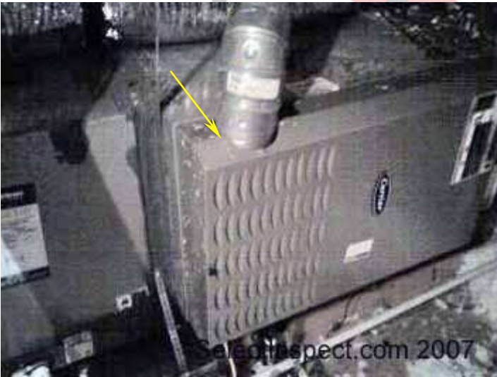
↑ flue obstructed HVAC service panel- attic
