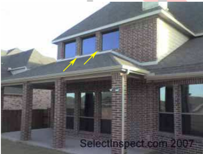
↑ flashing and window need sealant touch-up
