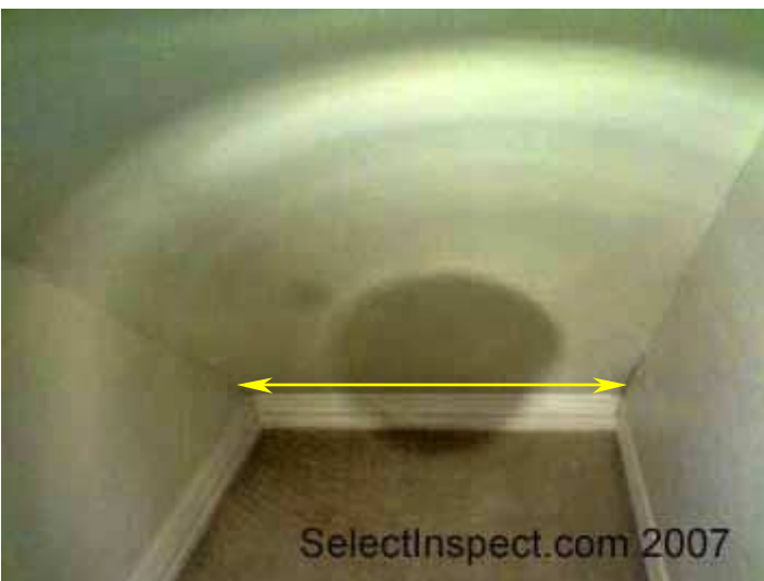
↑ unfinished wall joints below stairs
