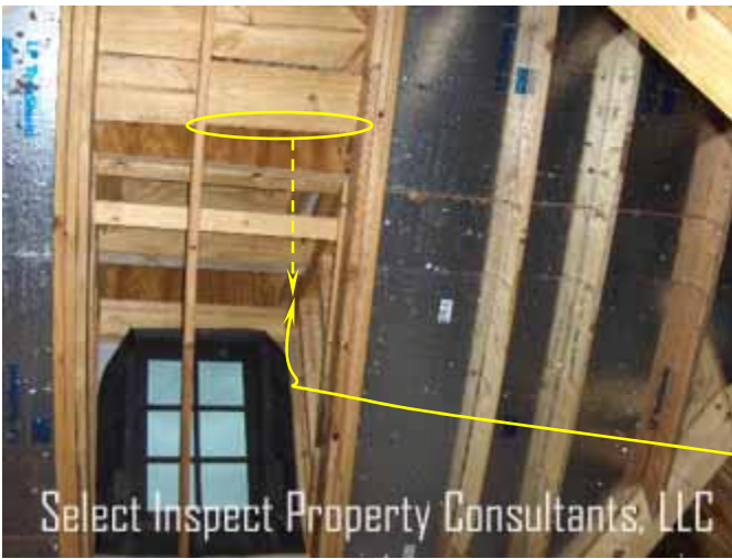
↑ wood at this location of the dormer appeared stained, when viewed from below.
