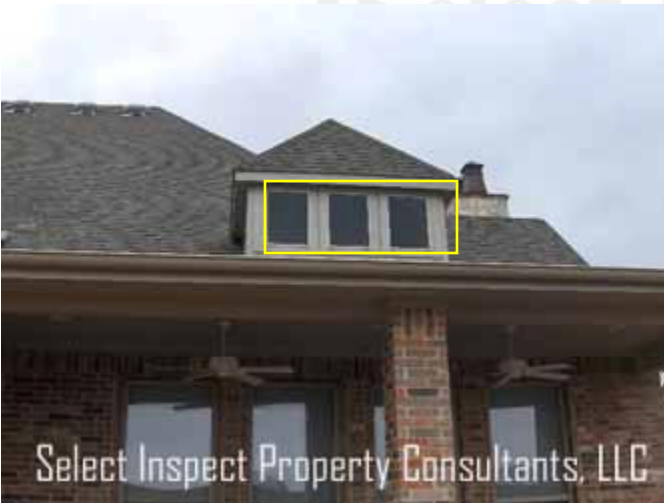
↑ sealant repair needed at upper family room window perimeters
