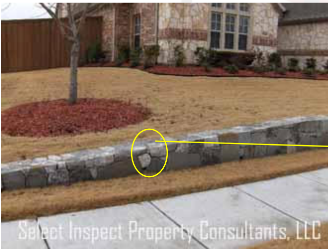
↑ crack discovered at retaining wall
