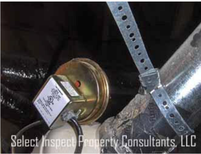
↑ http://www.fantech.net/dbf4xl_i.pdf ; other than electrical deficiencies; installation of the inline dryer boost fan appeared satisfactory.
