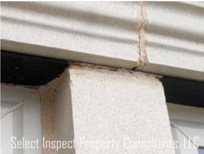
↑ mortar fallen from office/study window at lintel; satisfactory; the steel does not "hold" mortar well; this is common & not considered a deficiency
