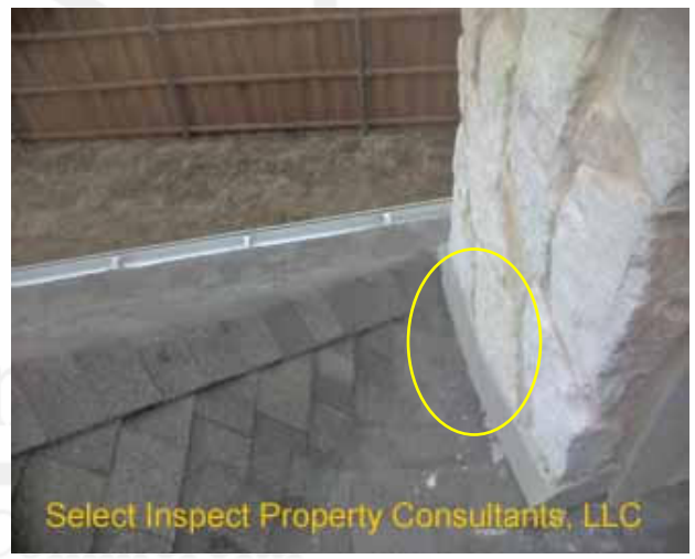
↑ marginal slope at the converging valley adjacent the chimney; prone to ice damming, debris accumulation, & moisture intrusion.
