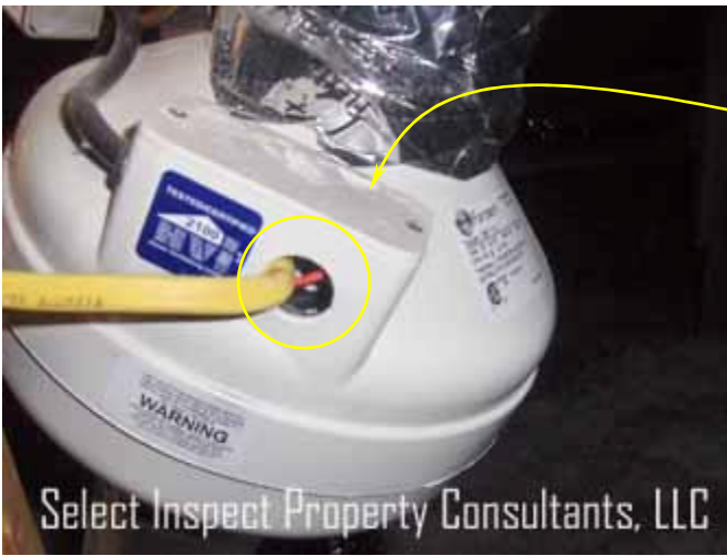
↑ missing clamp at dryer vent blower in attic
