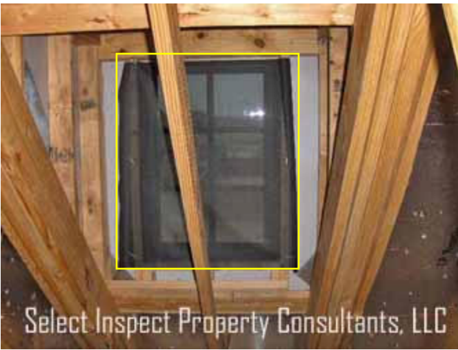
↑ flashing not visible at dormer windows.
