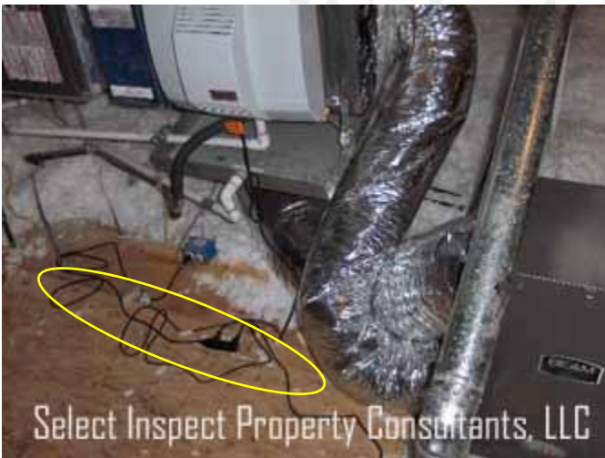
↑ extension cord for permanent use; example at northeast HVAC
