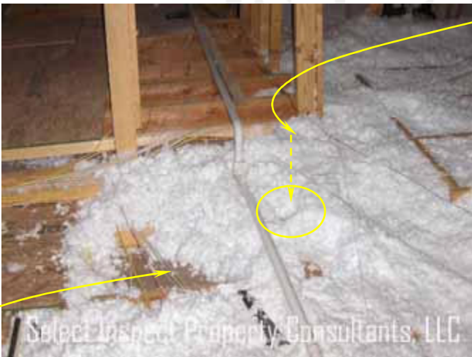
↑ moisture staining at insulation below location in image above; in proximity to moisture damage repaired at the mudroom ceiling.
