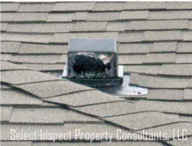
↑ dryer vent termination appeared congested; flapper appeared stuck open
