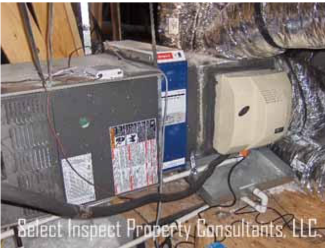
↑ multiple questionable conditions/deficiencies regarding humidifier model and installation
