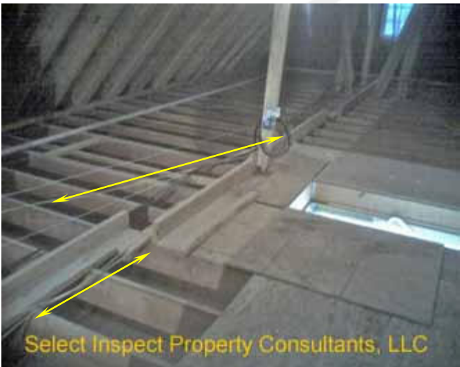
↑ Unprotected electrical wires within 6 feet of scuttle or 7 feet of attic stair
