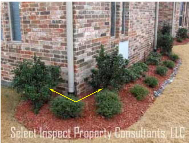
↑ bark is slightly higher than recommended at the north corner; Significant issues were not discovered; monitor and maintain
