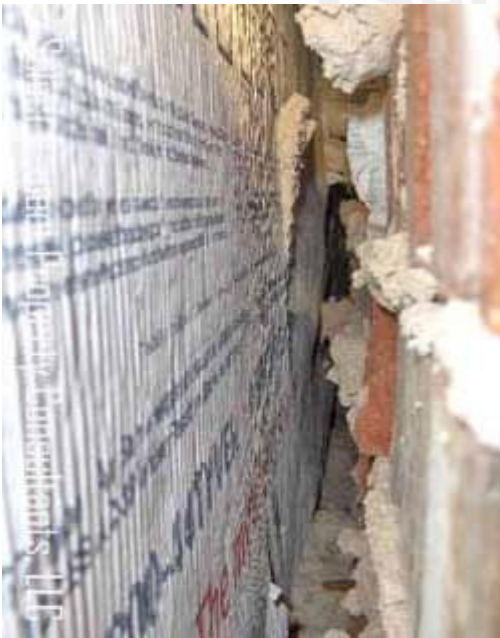
↑ mortar & brick debris in exterior wall void; example
