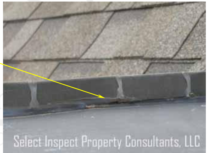
↑ small gap at top of central dormer may contribute to moisture intrusion
