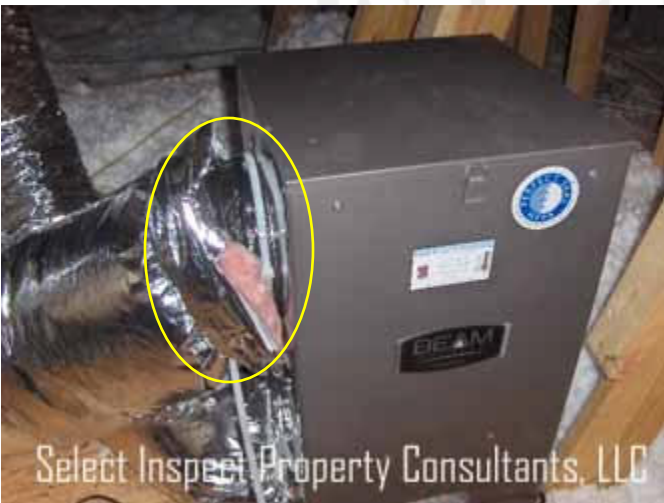
↑ deficient duct connection at south HVAC hepa
