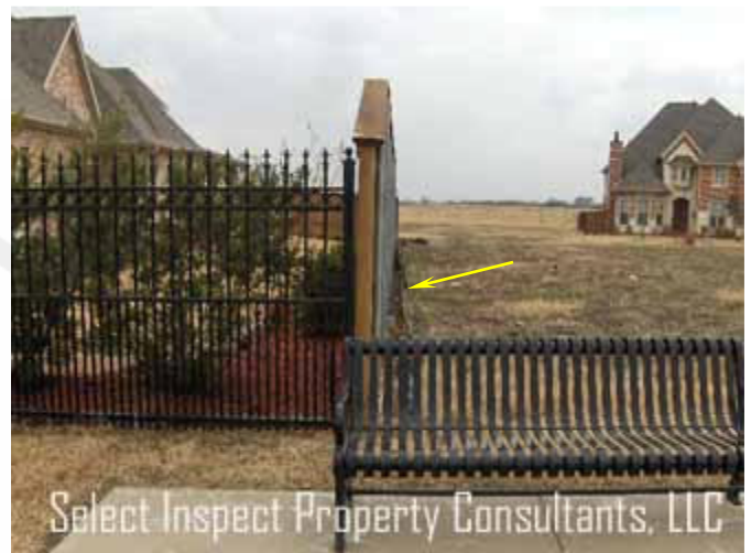
↑ monitor slope from neighboring property; Significant issues were not discovered during the inspection; monitor and maintain
