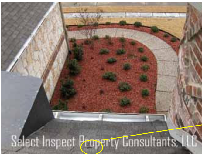
↑ damaged shingle above front entry
