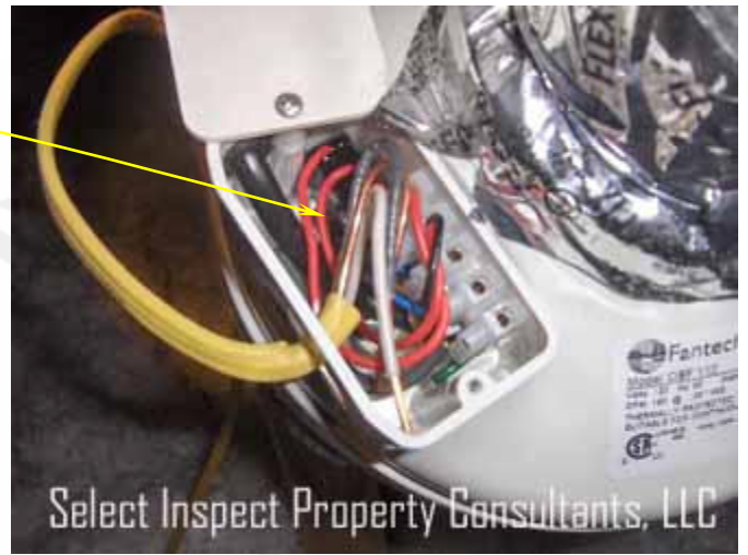
↑ unworkmanlike; incomplete wiring of dryer vent blower
