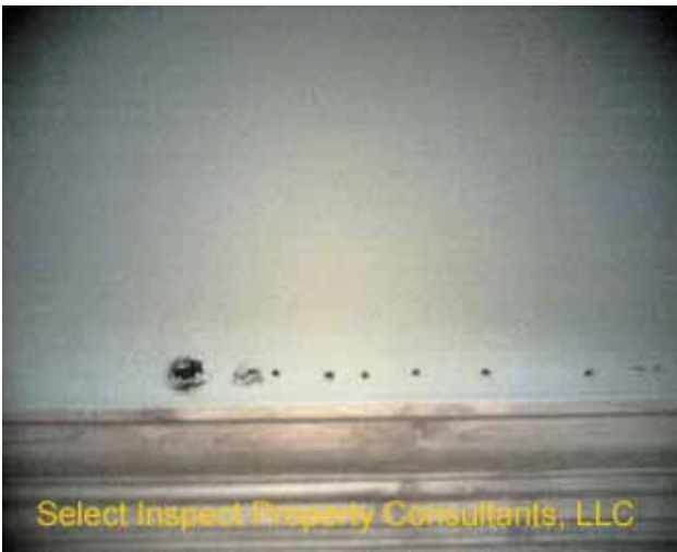
↑ openings in the drywall at the butler pantry; above cabinets; both sides
