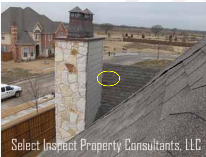
↑ missing shingle tabs at roof adjacent the chimney
