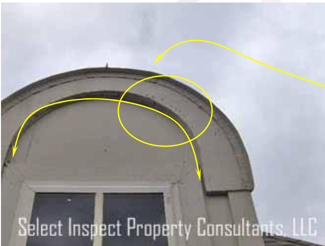
↑ retracting nails & lacking sealant in seams at the central dormer
