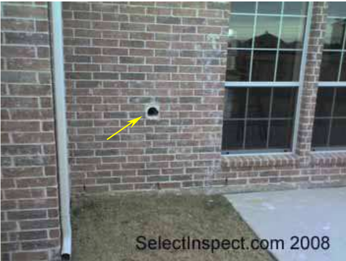
↑ missing cover at fireplace air intake vent
