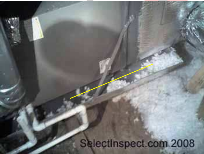
↑ insulation debris in auxiliary pan- air-conditioner
