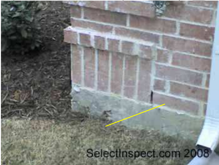
↑ corner crack at north - Repair needs were not discovered at the time of inspection
