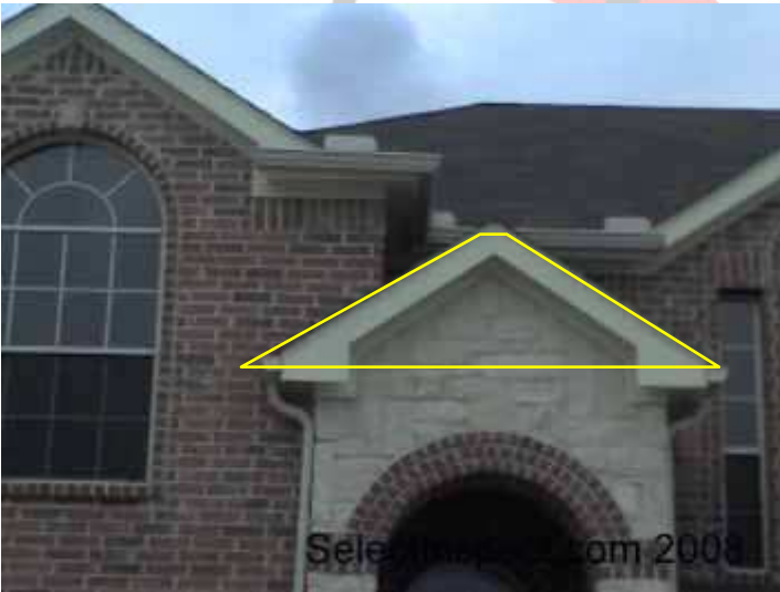
↑ unvented entry ceiling/attic
