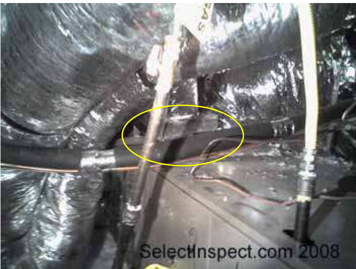
↑ auxiliary filter location- unit #2
