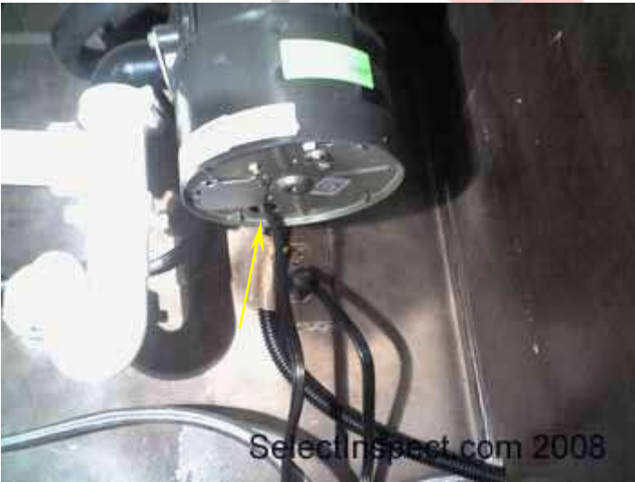
↑ missing electrical clamp at disposal base
