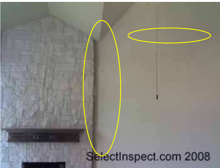
↑ moisture intrusion evidence at family room/fireplace
