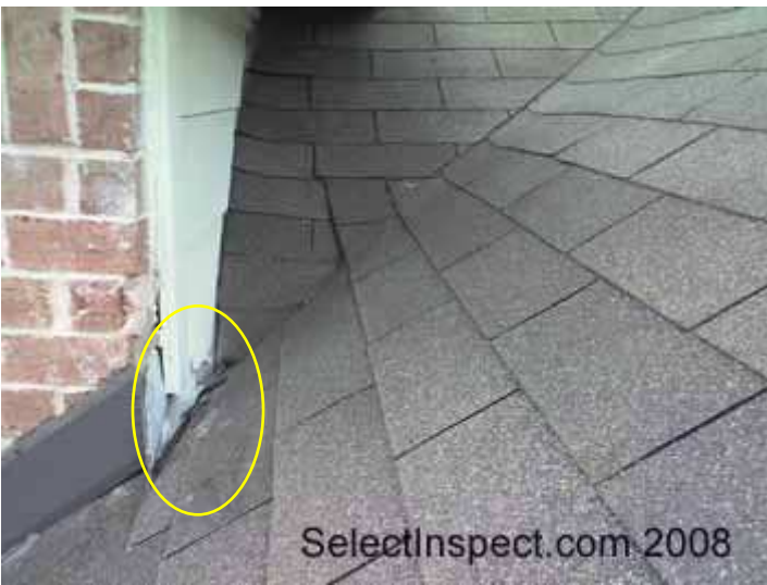
↑ low slope at small valley above patio door
