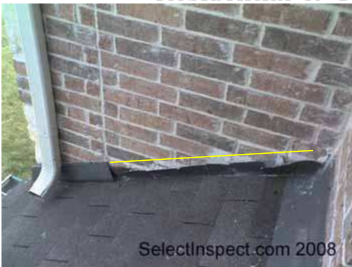
↑ amiss / deficient counter flashing at porch roof - moisture intrusion concern
