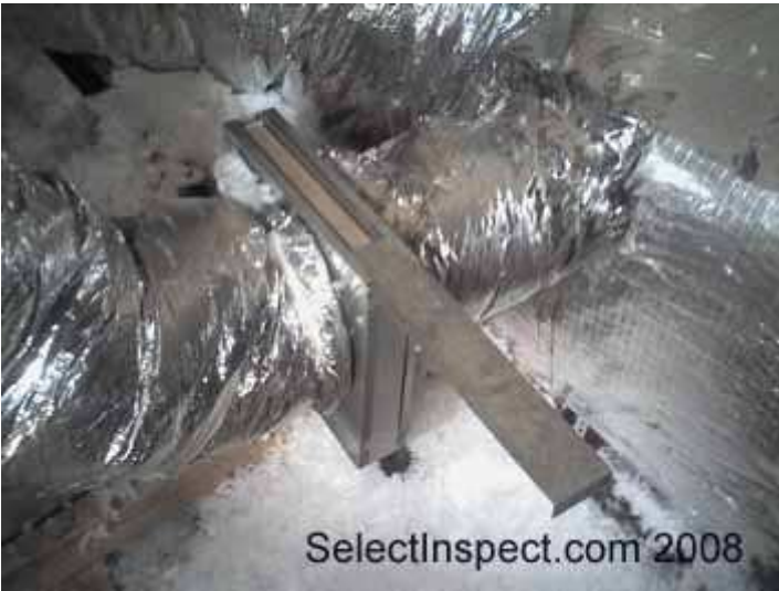
↑ auxiliary filter location- unit #1
