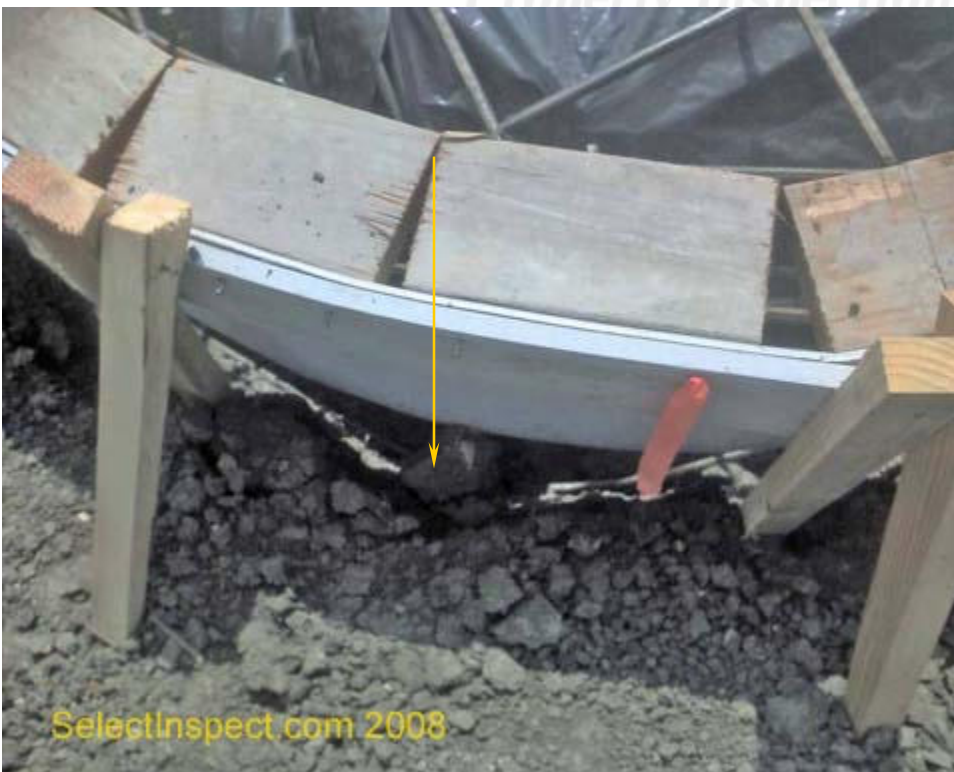
↑ dirt chunks in trench, and less than 3" separation of reinforcing steel & soil
