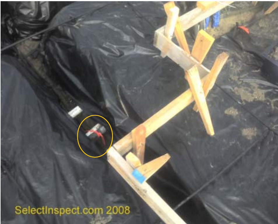
↑ unprotected plumbing supply pipe that will be routed through the concrete. Insulation was open and deficient.
