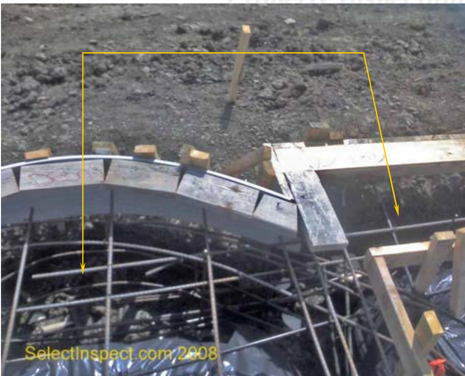
↑ debris in trenches
