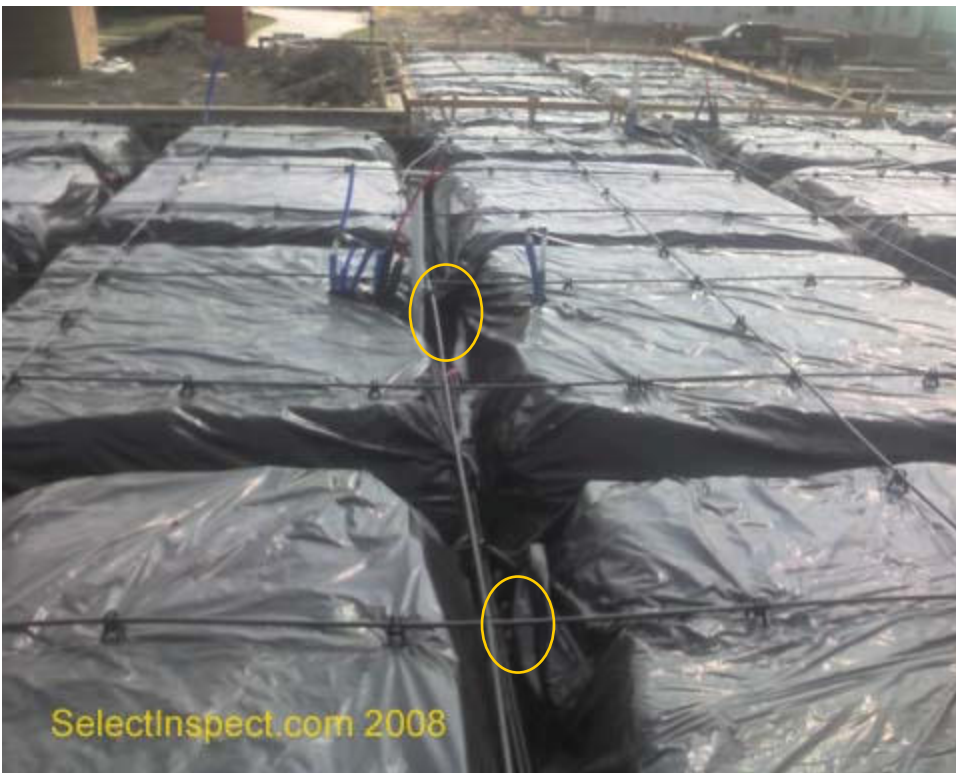
↑ unprotected plumbing supply pipe that will be routed through the concrete.
