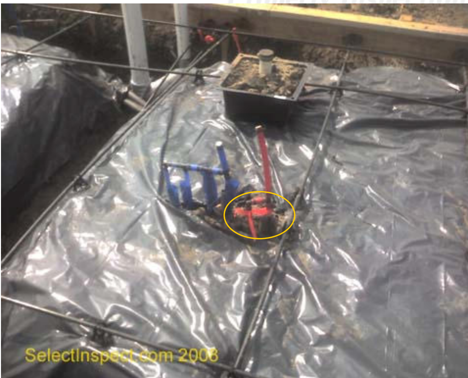
↑ unprotected plumbing supply pipe that will be routed through the concrete. South
