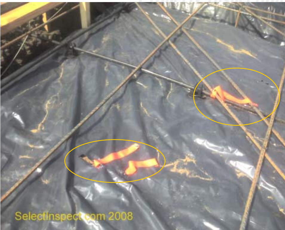
↑ chair needed to raise the reinforcing steel off the vapor barrier/pad & openings in the vapor barrier; reinforcing steel shall be supported on chairs, not by post tension cables; example
