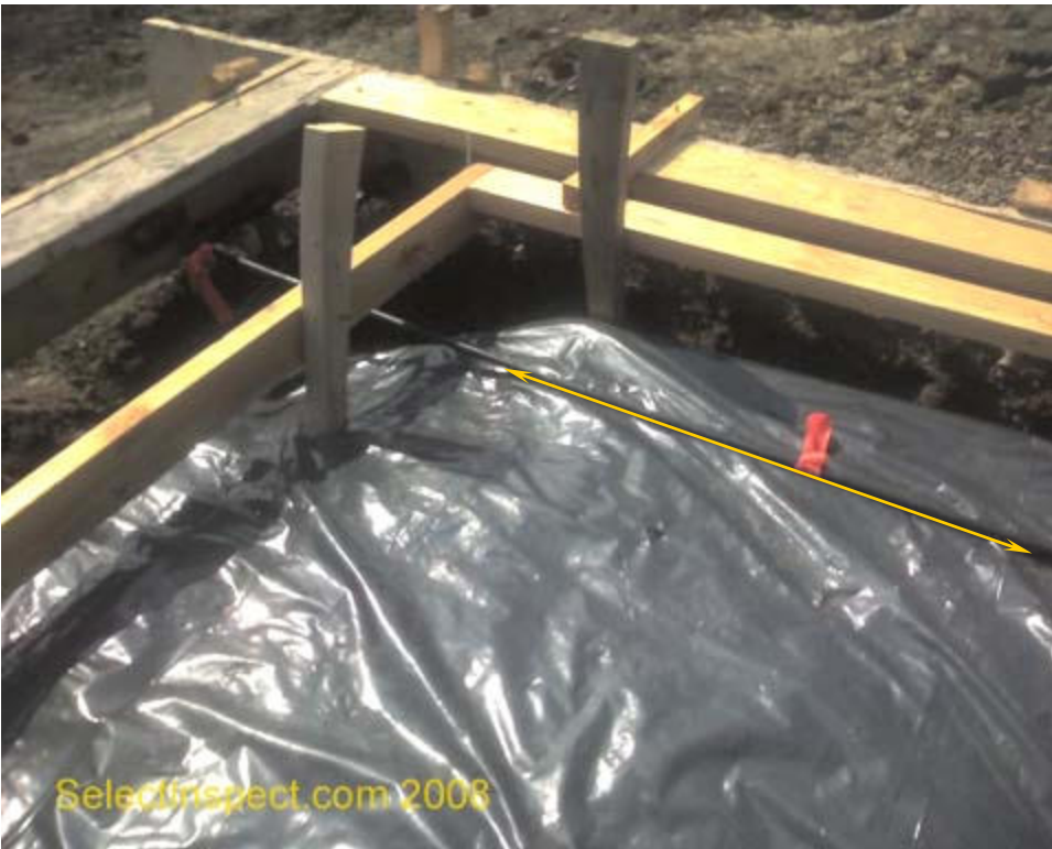
↑ chair needed to raise the post tension cable off the vapor barrier/pad; example
