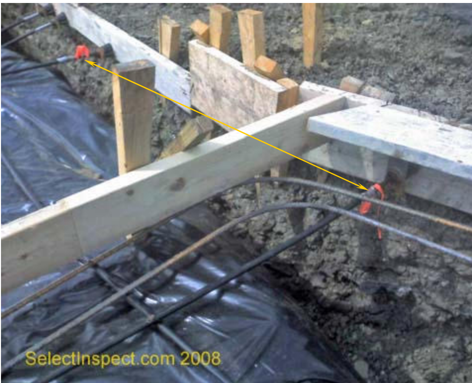
↑ post tension cable sleeve ends need better tape to protect the steel from the corrosive ingredients of concrete; example
