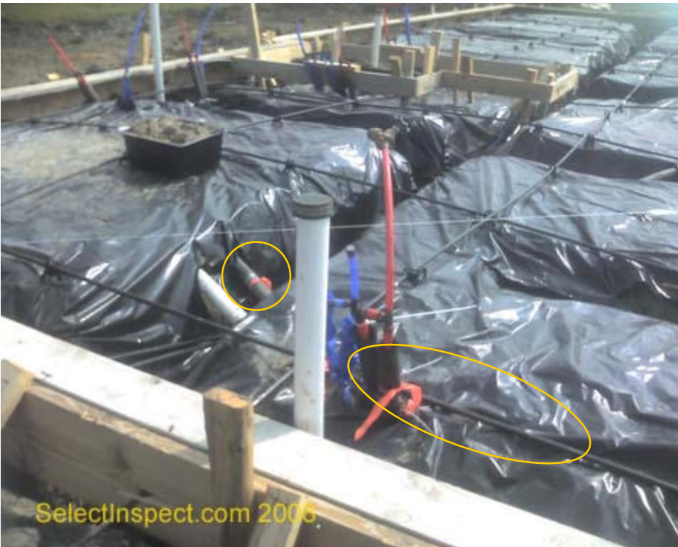
↑ chair needed to raise the post tension cable off the vapor barrier/pad; example and deficient insulation/protection of plumbing supply at northwest
