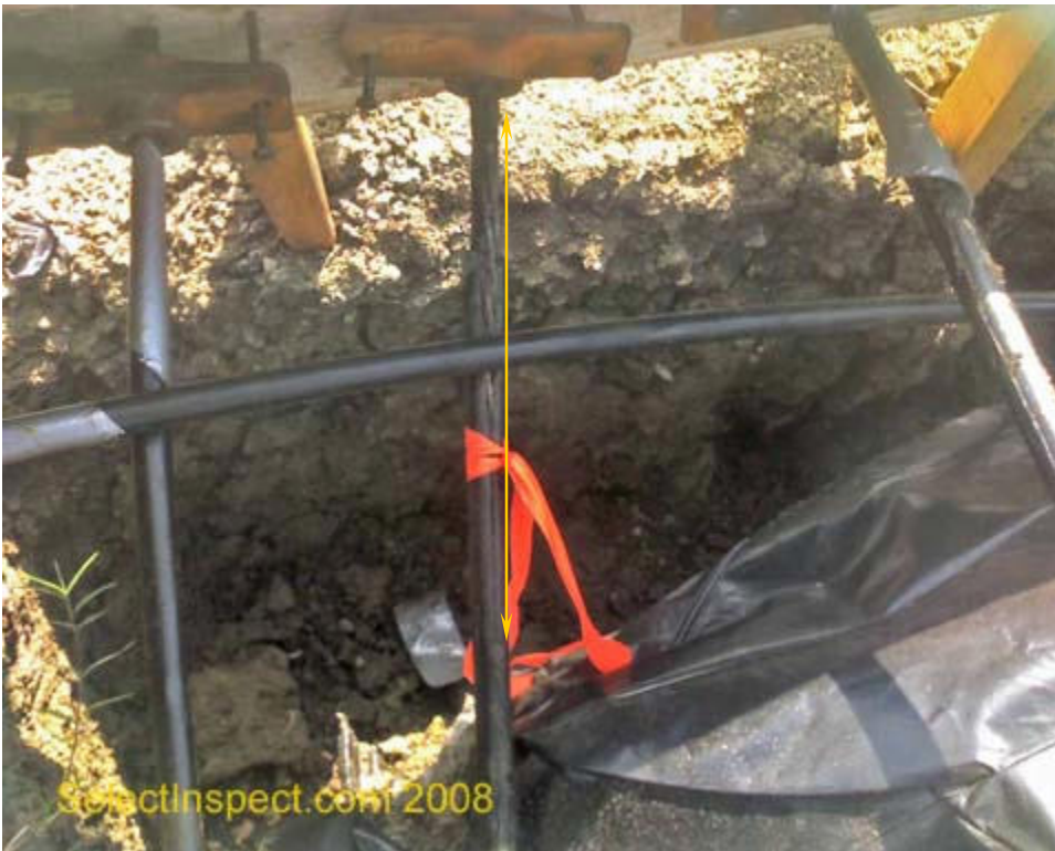
↑ close view of prior image post tension cable sleeve ends need better tape to protect the steel from the corrosive ingredients of concrete.
