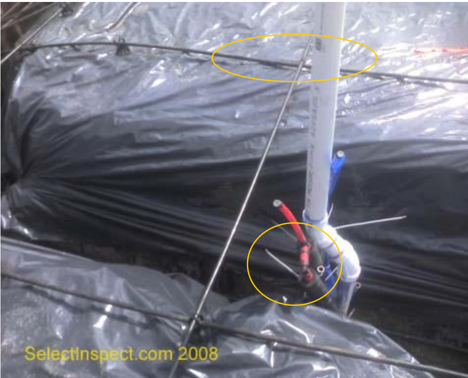
↑ upper- chair needed to raise the post tension cable off the vapor barrier/pad; example lower- unprotected plumbing supply pipe that will be routed through the concrete.
