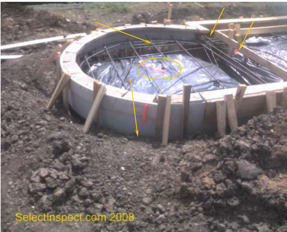
↑ debris in trenches, torn vapor barrier, and less than 3" separation of reinforcing steel to soil
