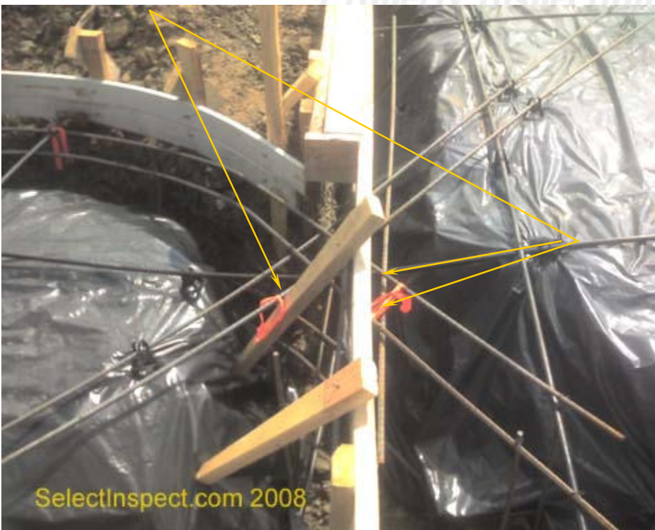
↑ close view of prior image; reinforcing steel is touching the forms at the front rounded feature. Recommended an offset of at least \frac{3}{4} " for concrete to pass on all sides.
