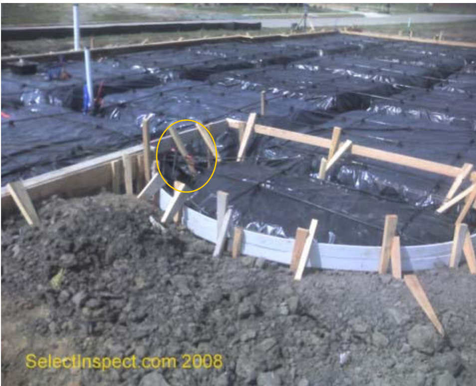
↑ reinforcing steel is touching the forms at the front rounded feature.
