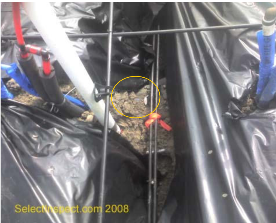
↑ unprotected plumbing supply pipe that will be routed through the concrete. Upper area of top image on prior page
