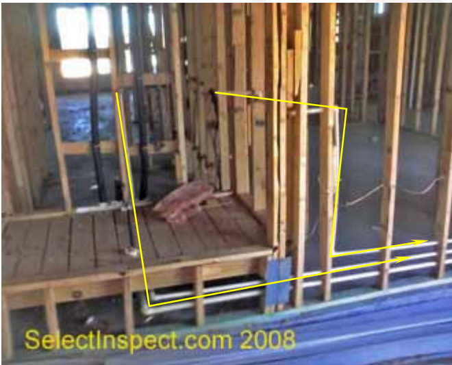
↑ deficient piping size at water heater temperature-pressure-relief lines
