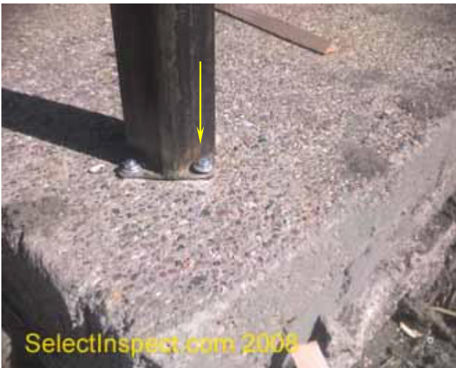
↑ unsecured bolt nut at southwest porch column/post
