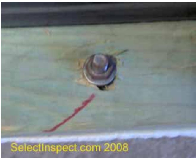
↑ excessive drill hole at anchor; example
