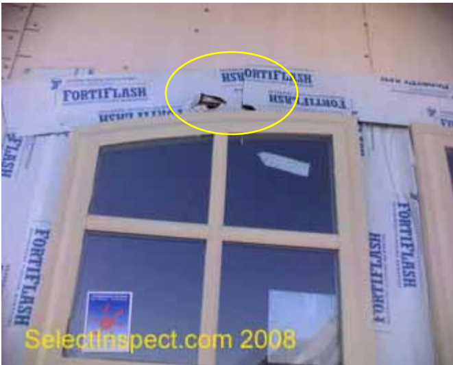
↑ damaged flashing and opening at thermoply sheathing; garage
