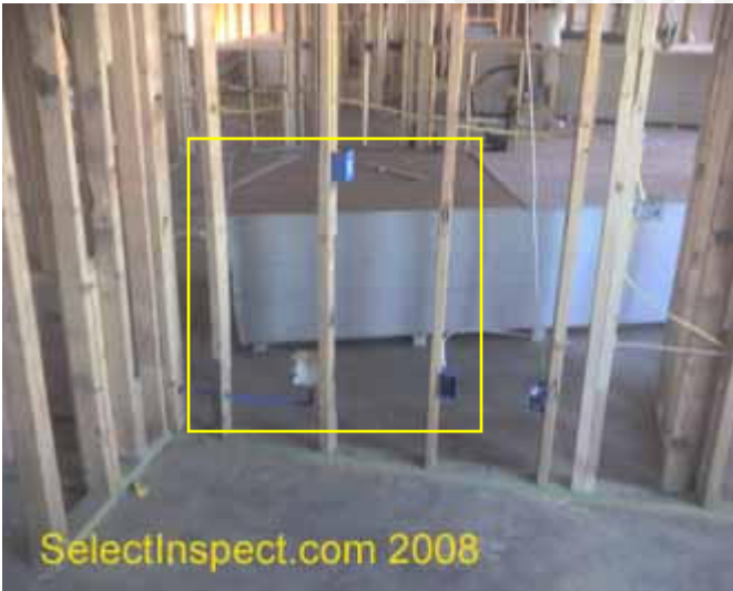
↑ compromised vertical framing at kitchen
