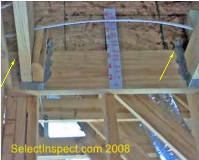
↑ deficient fasteners at southeast bathroom joist hangers
