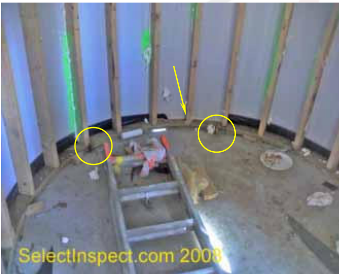
↑ misplaced anchors and deficient vapor barrier at rotunda
