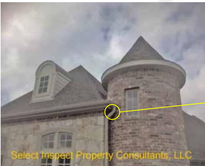
↑ unworkmanlike eave/brick joint; open to eave
