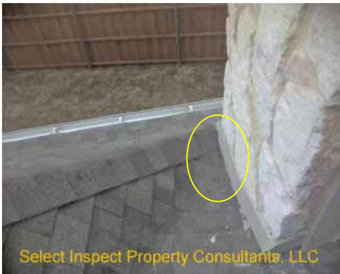
↑ marginal slope at the converging valley adjacent the chimney; prone to ice damming, debris accumulation, & moisture intrusion.
