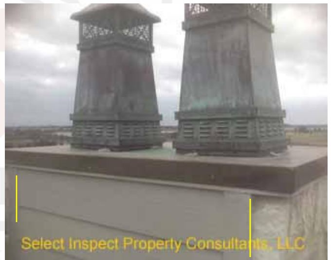
↑ chimney cap is concave rather than convex & trim/stone joints should be sealed / caulked
