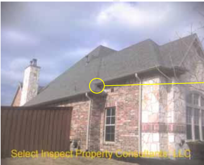
↑ unworkmanlike flashing/trim; opening to attic
