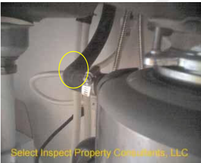
↑ dishwasher drain has a "kink" that will be prone to congestion, backup, and failure of the drain
