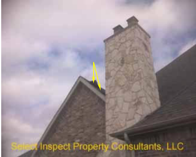
↑ wind damaged shingles adjacent the chimney
