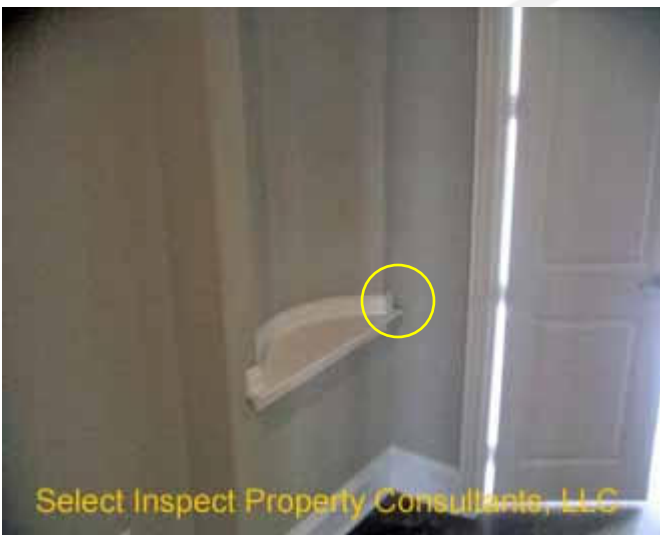
↑ various cosmetic details incomplete; example at master hallway
