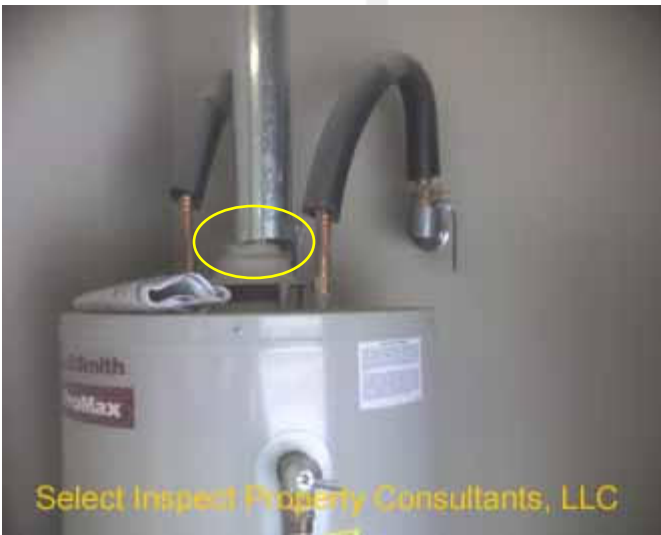
↑ disconnected water heater flue; should be seated & secured.
