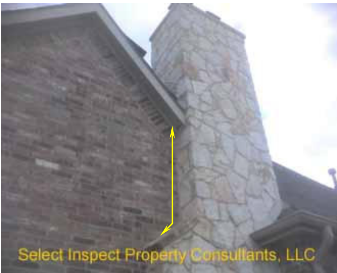
↑ thin mortar crack discovered at joint of stone & brick veneers; Significant issues were not observed concerning this
