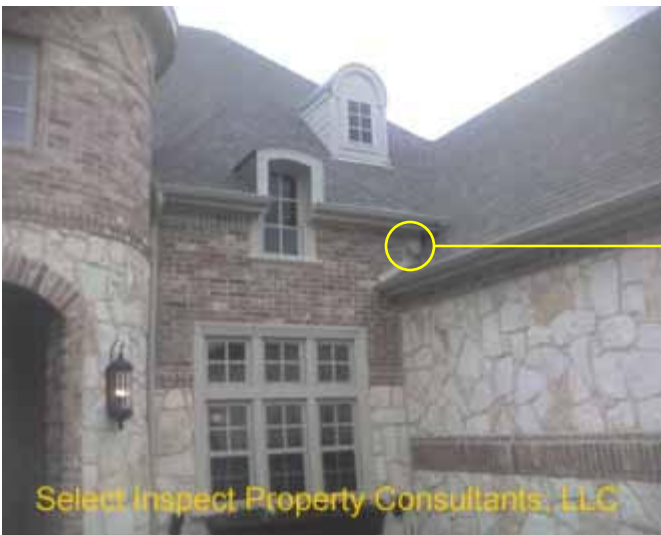
↑ unworkmanlike flashing/trim; exposed decking
