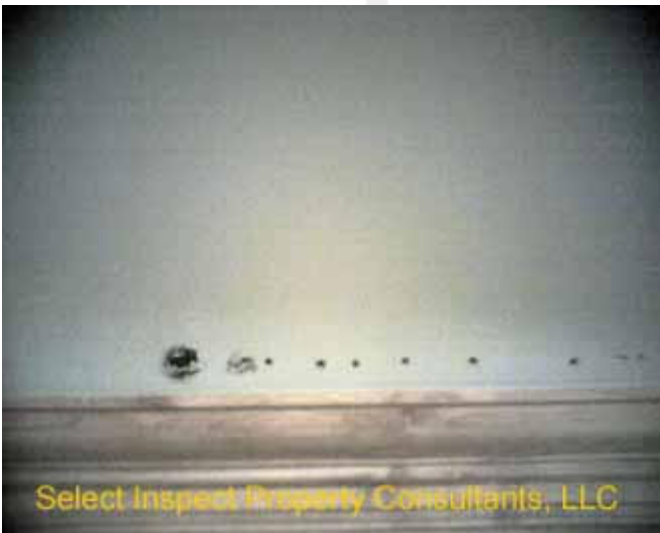
↑ openings in the drywall at the butler pantry; above cabinets; both sides
