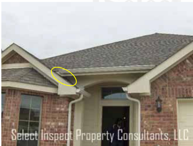
↑ short flashing remains; openings may allow moisture intrusion in driving rains
