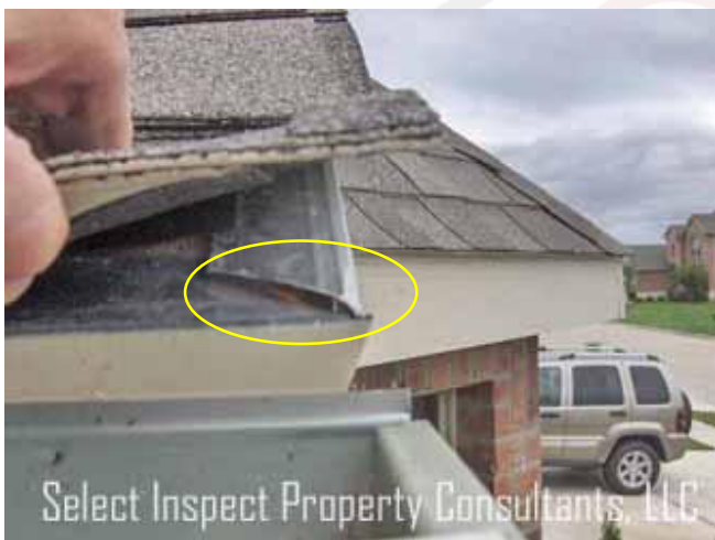
↑ unworkmanlike drip edge flashing & felt remains at southwest; poor/excess cut & opening
