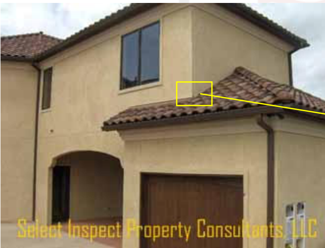
↑ seal flashing joint and stucco touch-up needed
