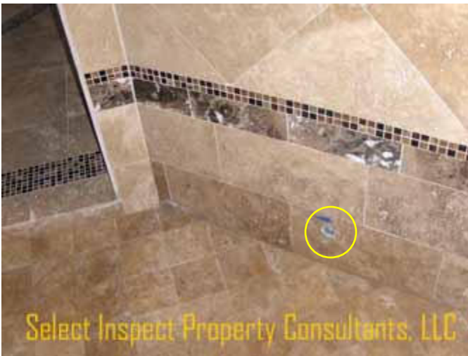
↑ opening at master shower tile
