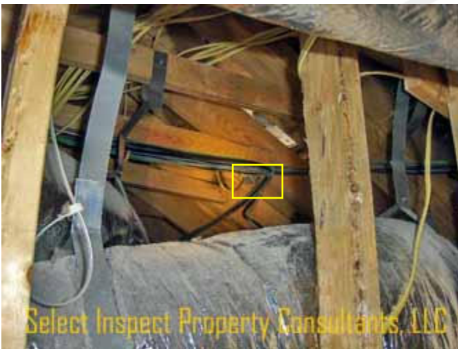
↑ some electrical attic fan thermostat(s) were not readily accessible and these devices were not tested; example at the master attic
