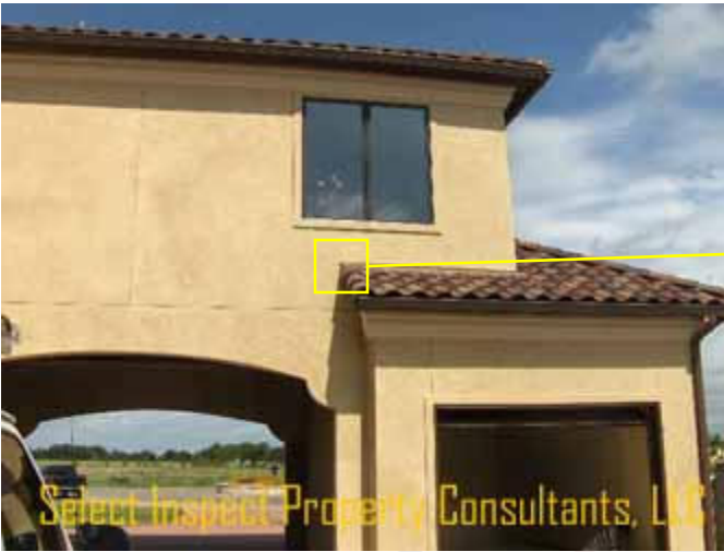
↑ seal flashing joint and stucco touch-up needed
