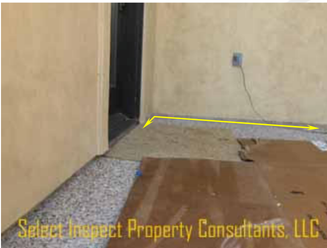
↑ stucco was low/hidden foundation edge; example
