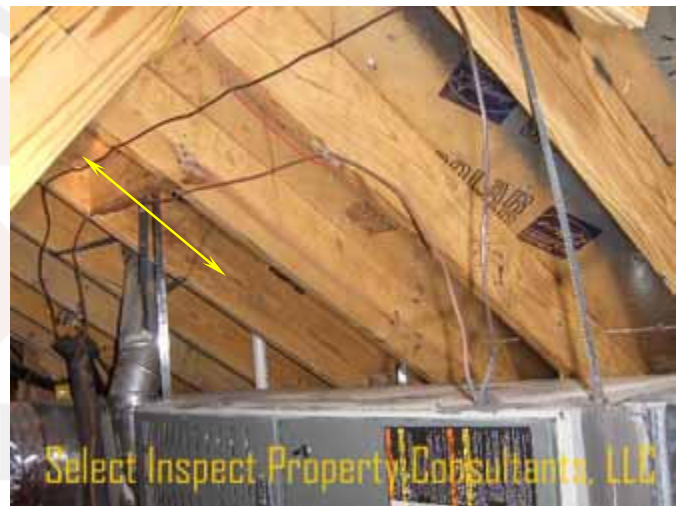
↑ cracked rafter discovered above HVAC #3; north attic
