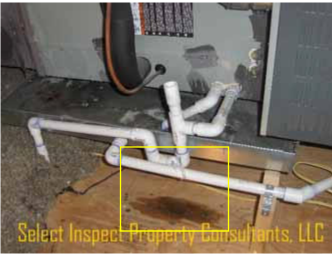
↑ example; primary condensate drain non-insulated; condensate staining/dripping below the traps @ master, east, & 2 north attic HVAC.
