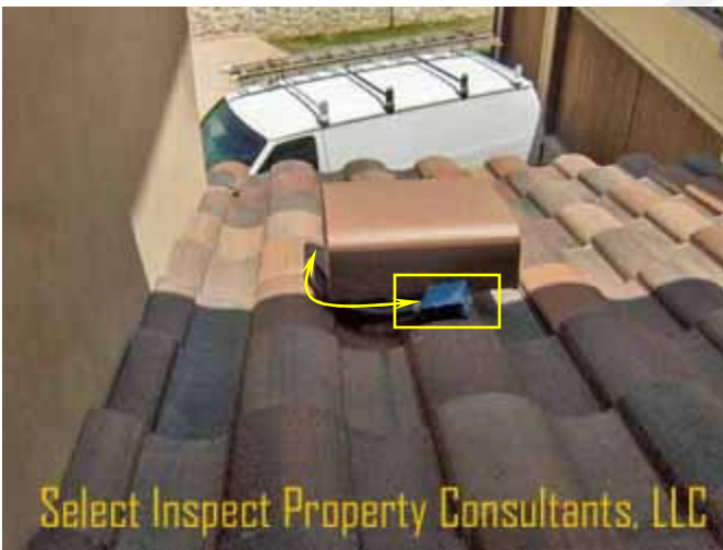
↑ junction box and conduit at the northeast roof looks out of place.
