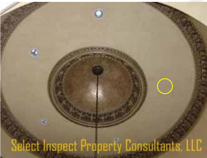
↑ it appeared that a recessed light was missing (visually unusual; empty space) above the stairway
