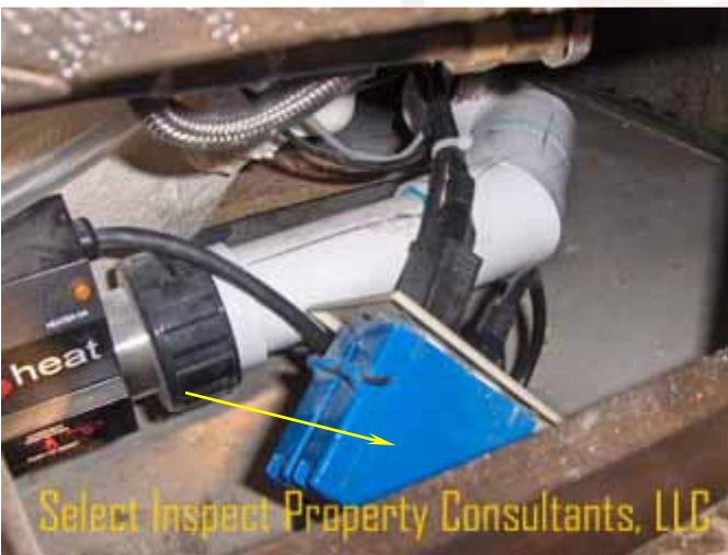
↑ unsecured electrical box below the jetted tub
