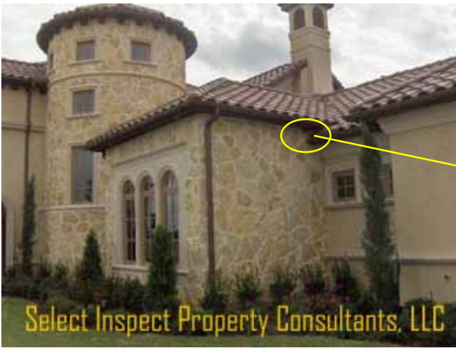
↑ stone was incomplete/missing at the southwest office/study
