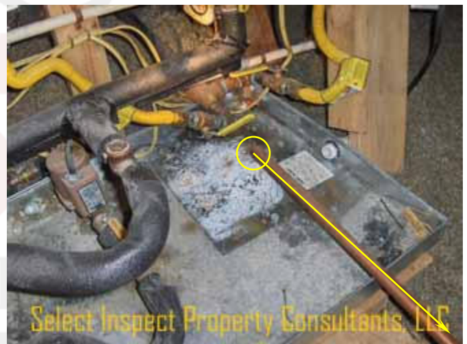
↑ this copper pipe in the master attic had undetermined purpose & undetermined termination; discovered at the water heater auxiliary pan
