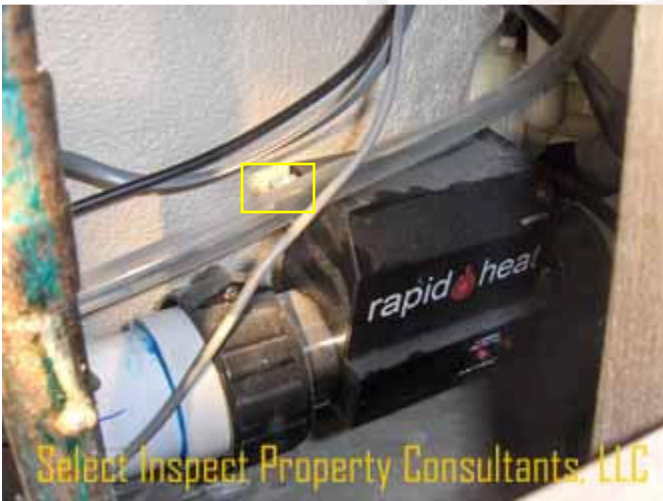
↑ jetted tub heater was bonded through the electrical cord, though the bonding / grounding terminal was unused.
