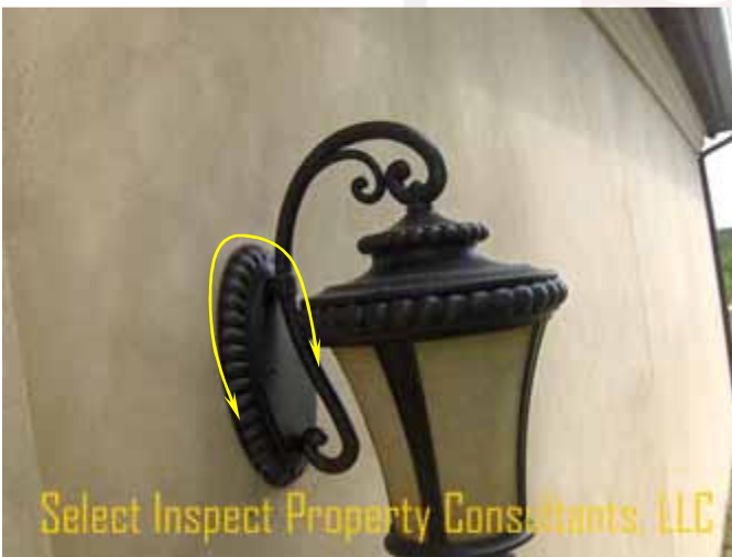
↑ caulking/sealant needed atop exterior lights; example
