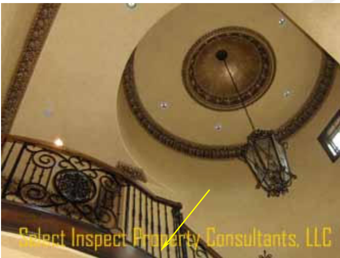
↑ various trim joints were not flush; example at main stair loft
