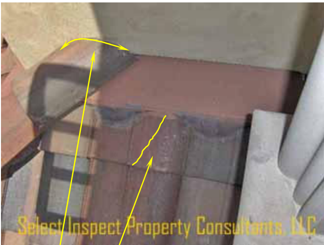
↑ slipped tile; cracked tile; close view of image above
