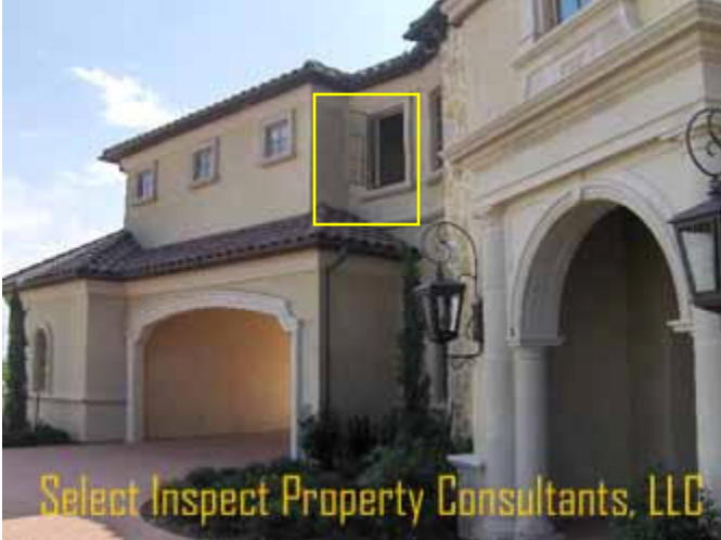
↑ cracked tile; missing mud seal/gaps; window not functioning as intended
