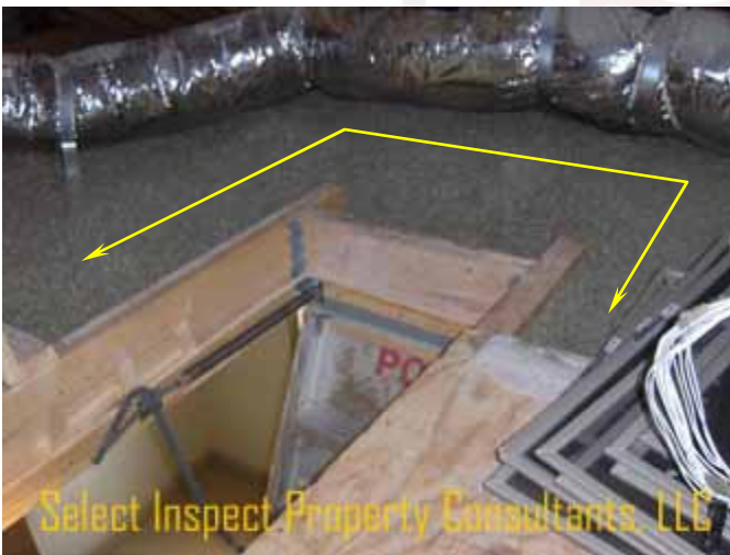
↑ lack of decking at top of north hall attic stair
