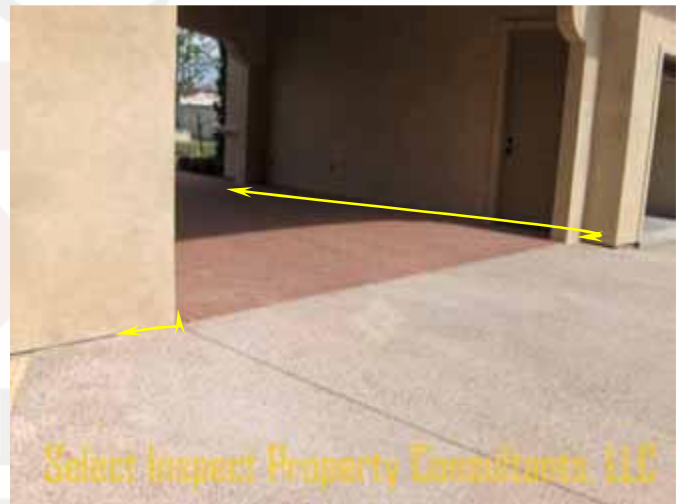
↑ stucco was low/hidden foundation edge; example
