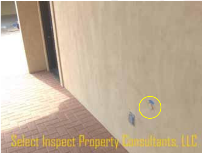
↑ stucco obstructs this plumbing clean-out at the porte-cochere
