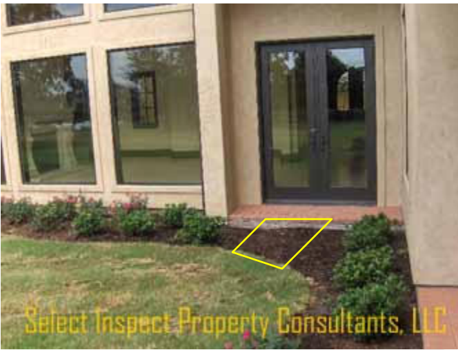
↑ this area seemed empty without some type of paver/stone leading from the patio to the grass
