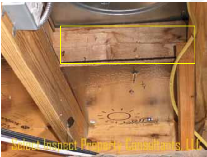
↑ moisture staining at the electrical fan above HVAC #2; north attic
