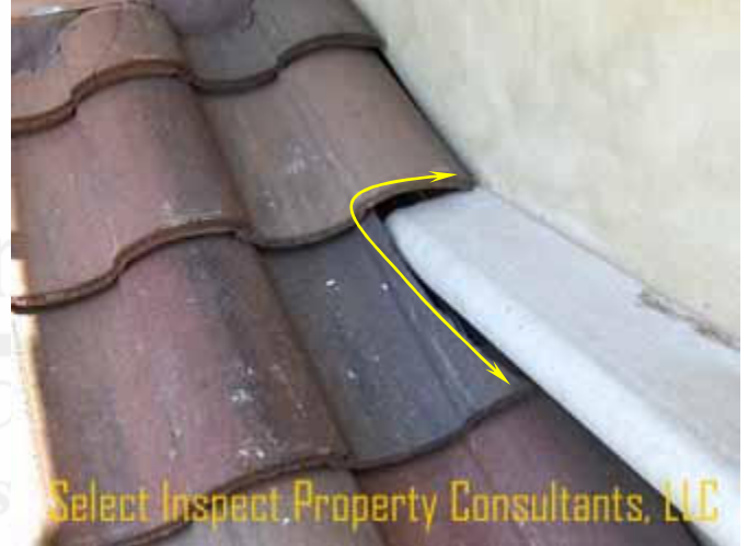
↑ close view of image at left; mud/flashing missing; slats visible
