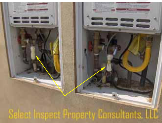
↑ temperature/pressure relief piping was smaller than required by most device manufacturers
