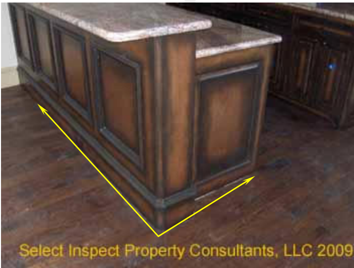
↑ gaps remain at game room bar area
