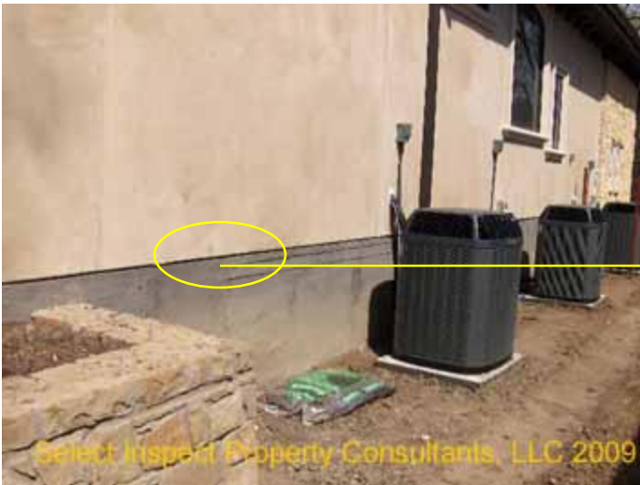
↑ damaged stucco at south
