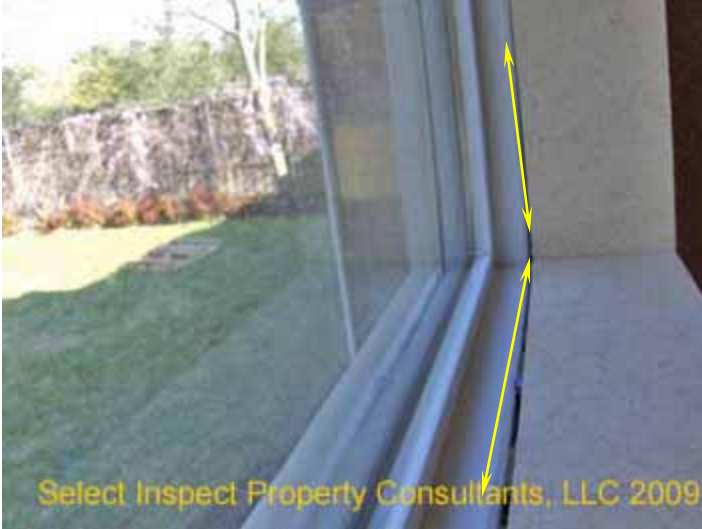
↑ sealant / grout needed at the guest bathroom window
