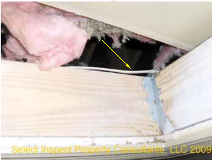
↑ Unprotected electrical wires within 6 feet of scuttle; game room attic scuttle
