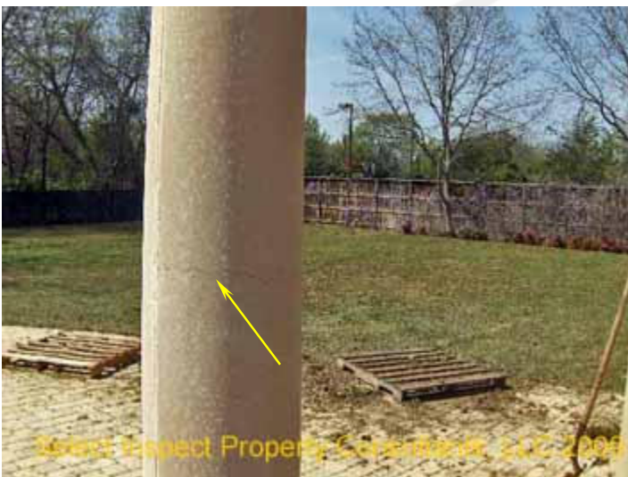
↑ close view example cracked column
