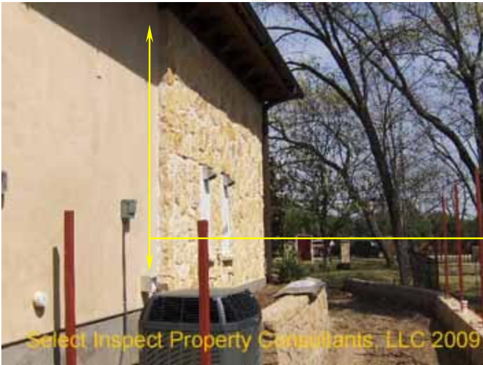
↑ unfinished stucco; exposed house wrap
