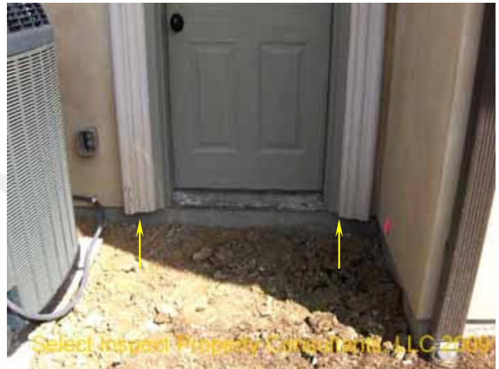
↑ recommend paint/sealant at the exposed underside trim at doorway
