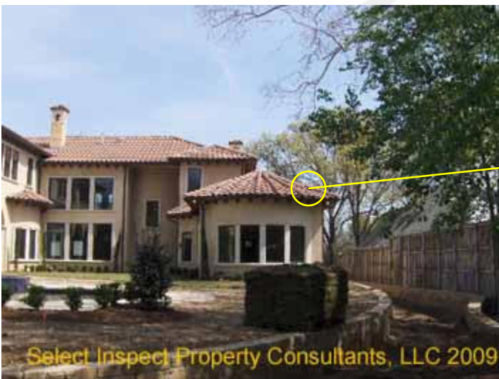
↑ askew roof tile at master bedroom
