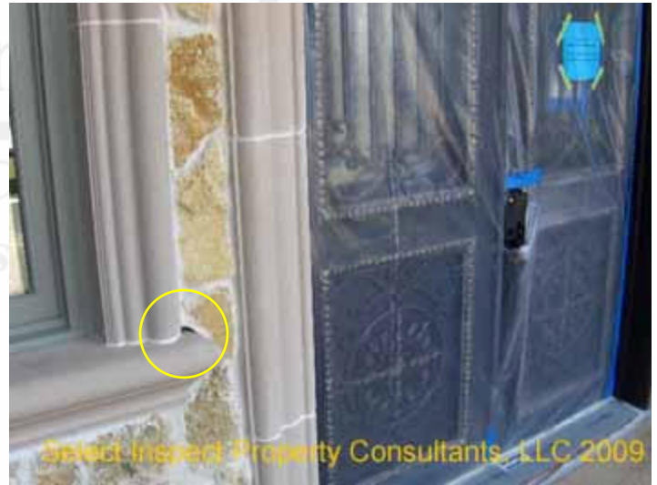
↑ mortar tuck pointing needed
