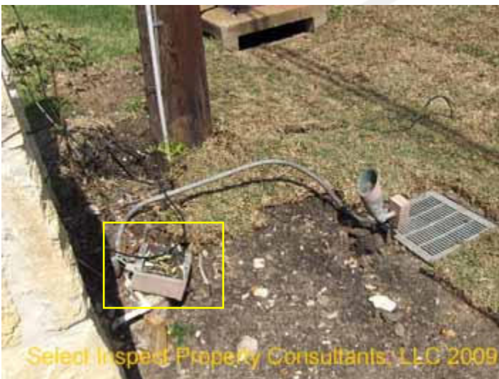
↑ exposed electrical at northeast near the street may be a hazard.
