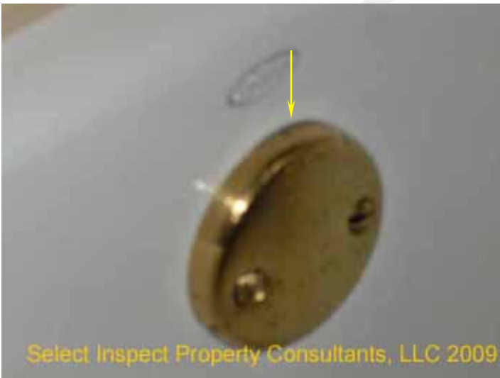
↑ askew overflow cap & opening
