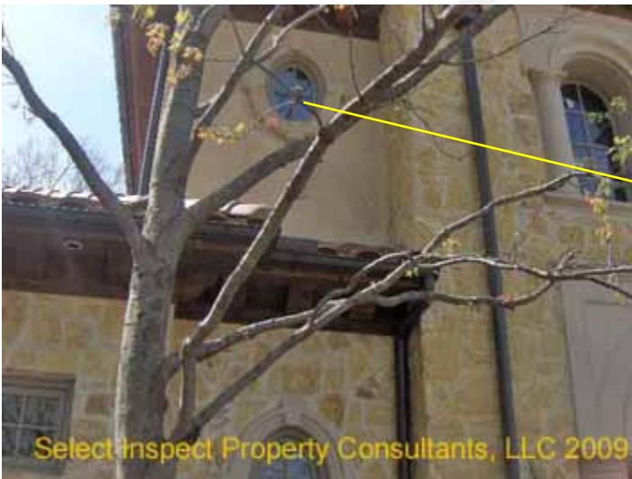
↑ mortar tuck pointing needed
