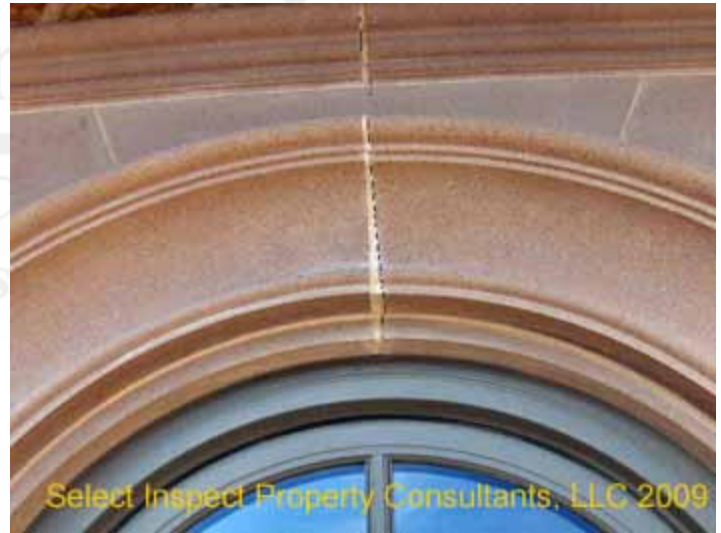
↑ mortar tuck pointing needed
