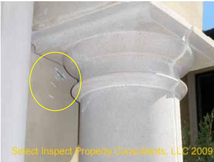
↑ scratched stucco at family room patio
