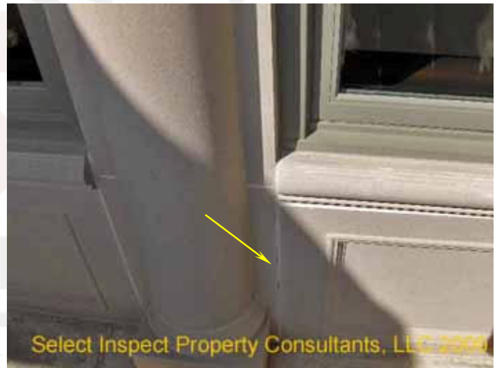
↑ mortar tuck pointing needed
