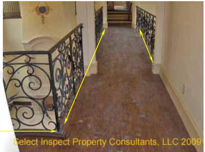
↑ gaps remain at rail mountings/wood floor
