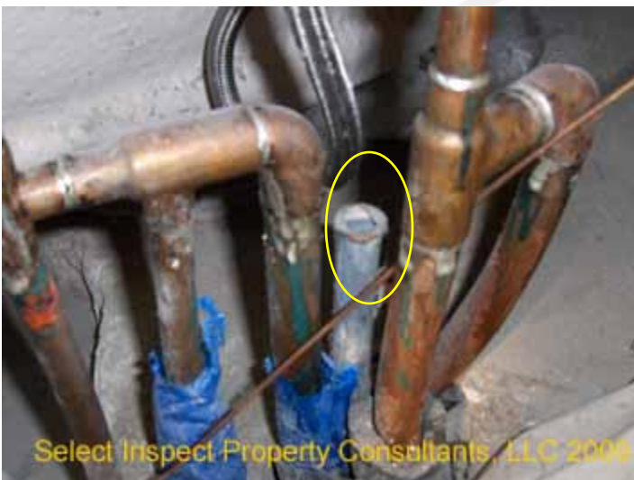
↑ hollow plumbing support stake may be a future entry point for wood destroying insects
