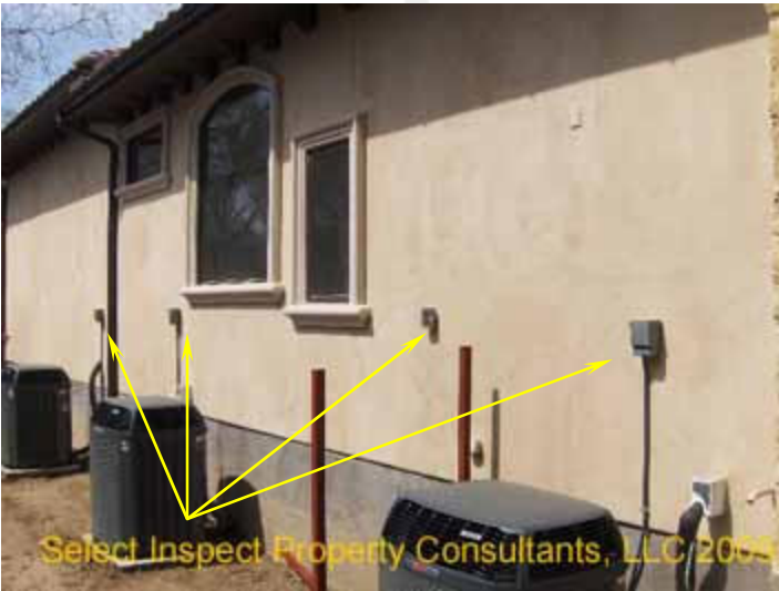
↑ sealant needed at Air-conditioner service disconnects; example at south
