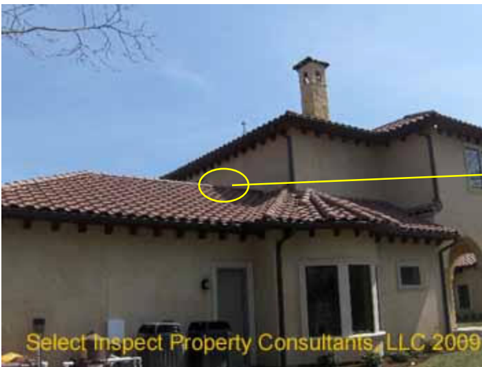
↑ damaged tile & suspected damaged ridge support/vent
