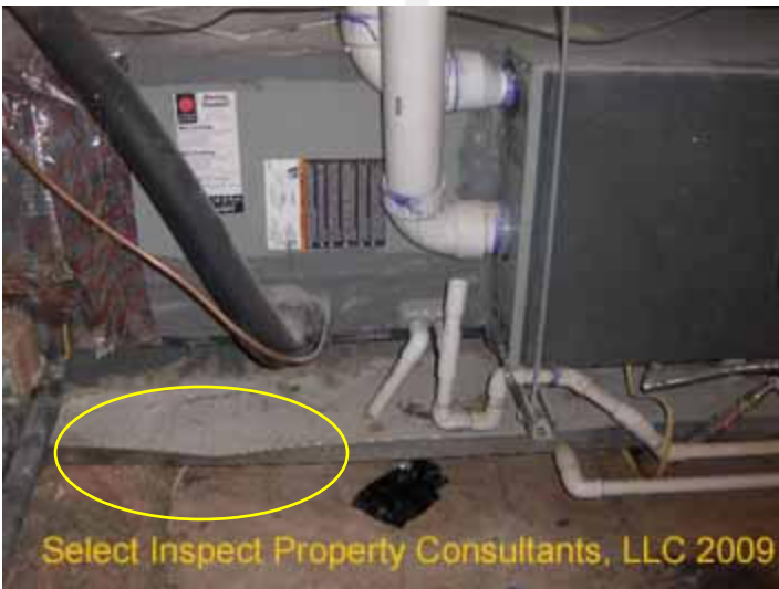
↑ deficient auxiliary pan at master bedroom HVAC
