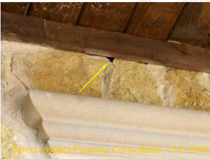
↑ mortar tuck pointing needed
