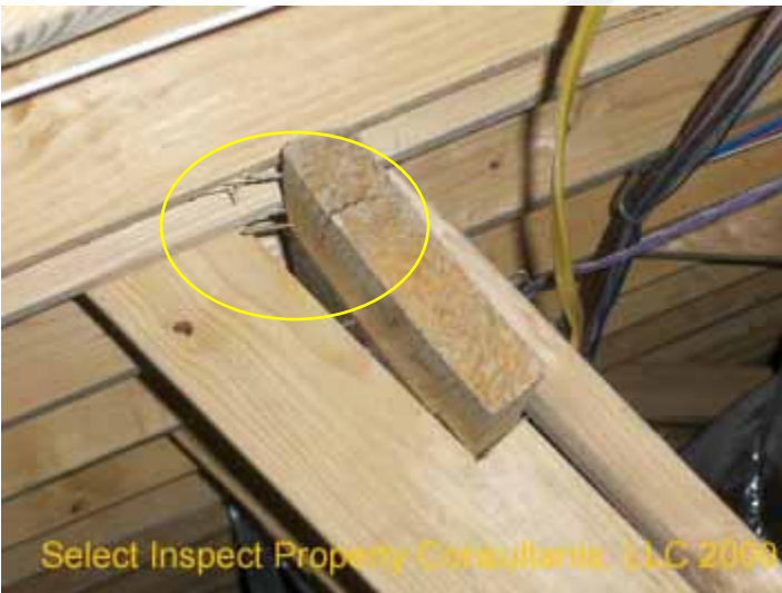
↑ marginal angles & nailing; example at struts
