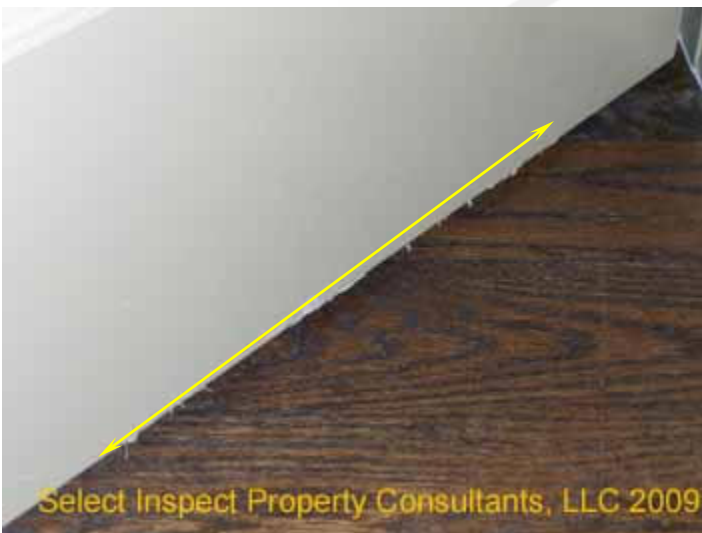
↑ unworkmanlike paint finish at game room bathroom door
