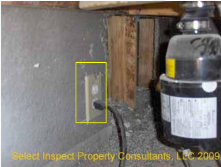
↑ damaged receptacle(s) cover below master bathtub
