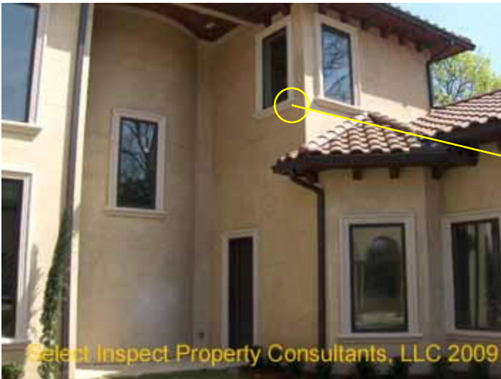
↑ discoloration (moisture or cosmetic ?)
