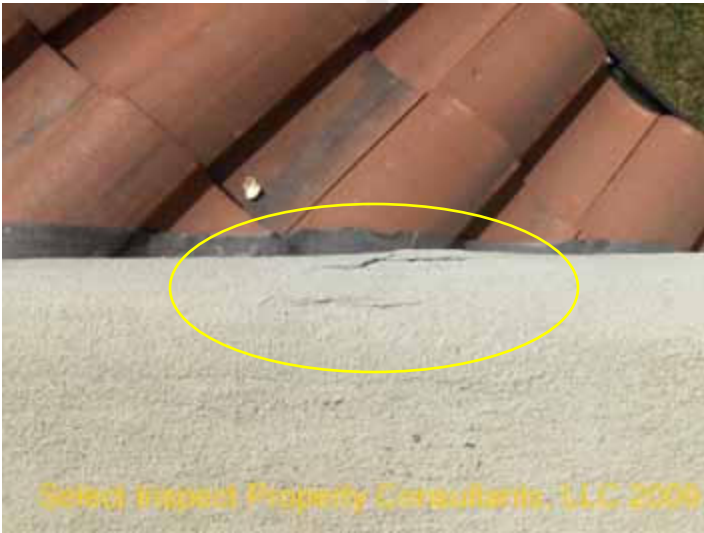
↑ damaged stucco/EIFS at game room window
