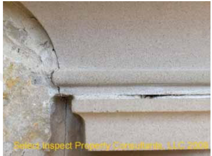
↑ mortar tuck pointing needed
