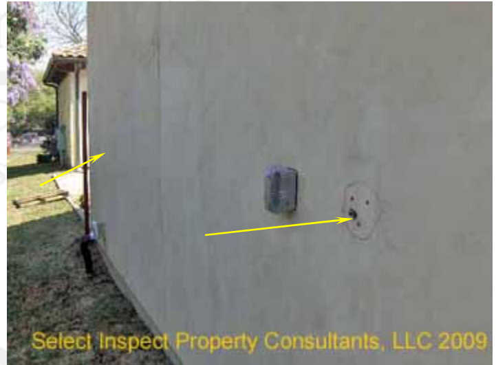
↑ abandoned electrical & openings at north garage
