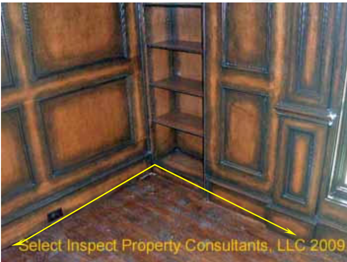
↑ close view of image above
