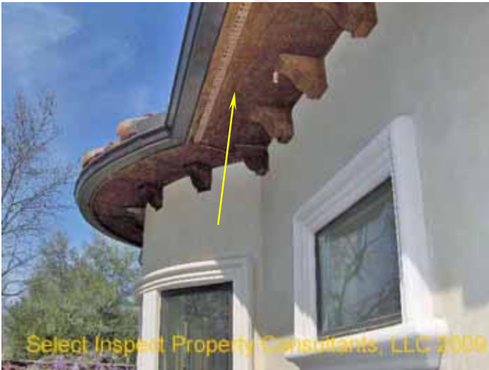
↑ slight discoloration; peeled soffit; very minor
