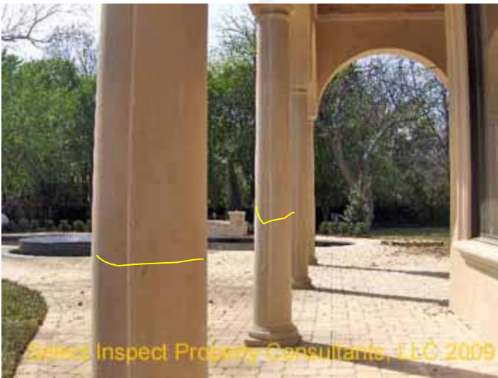
↑ 5 of 8 columns were cracked at the patio
