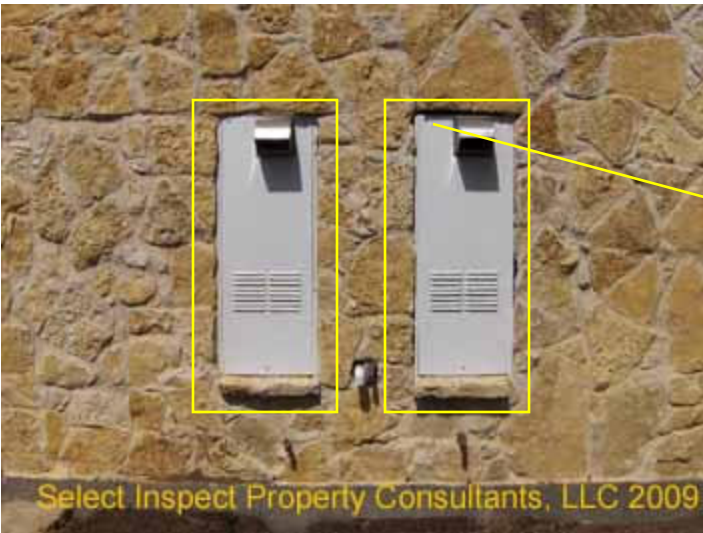
↑ openings at hot water equipment
