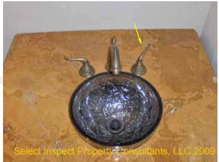
↑ askew water control
