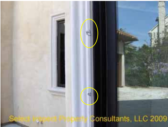
↑ damaged stucco at driveway door
