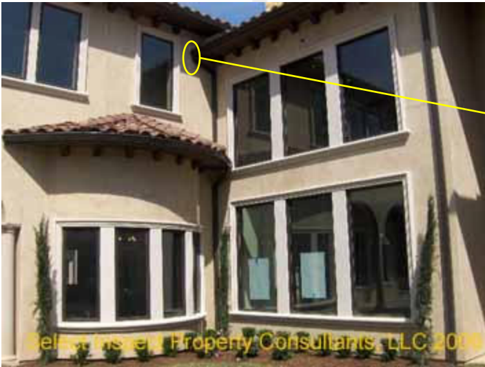
↑ discoloration; undetermined cause
