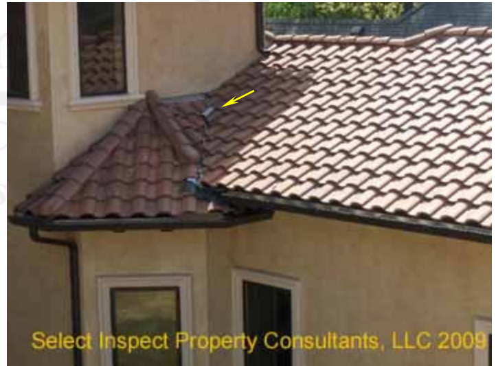
↑ debris at master bedroom roof
