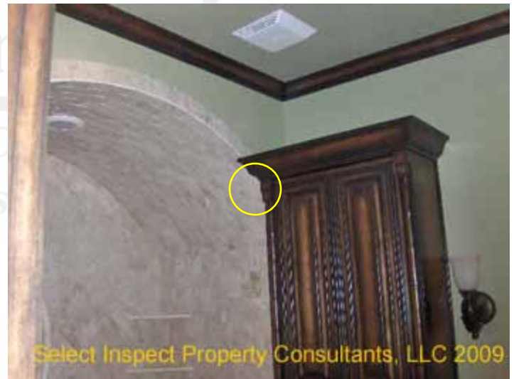
↑ unfinished detail; upstairs southern bedroom cabinet
