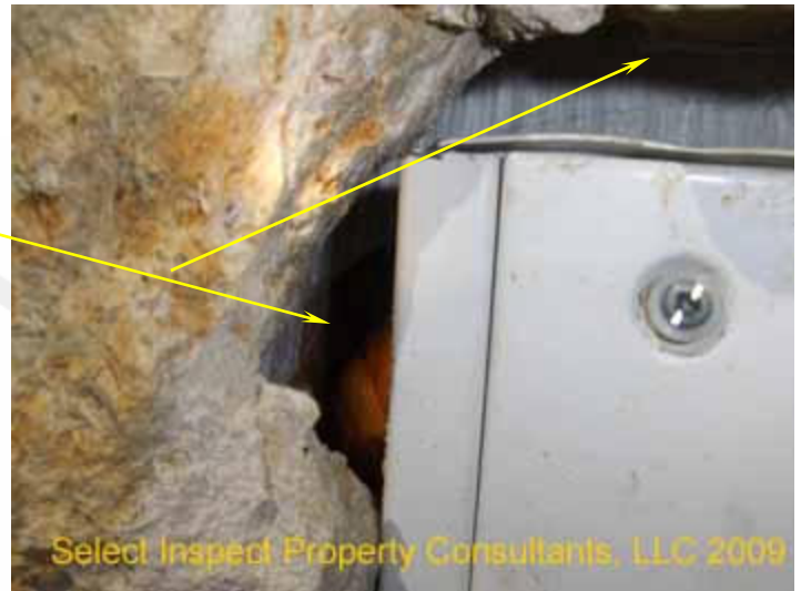
↑ exposed substrate; openings at moisture barrier
