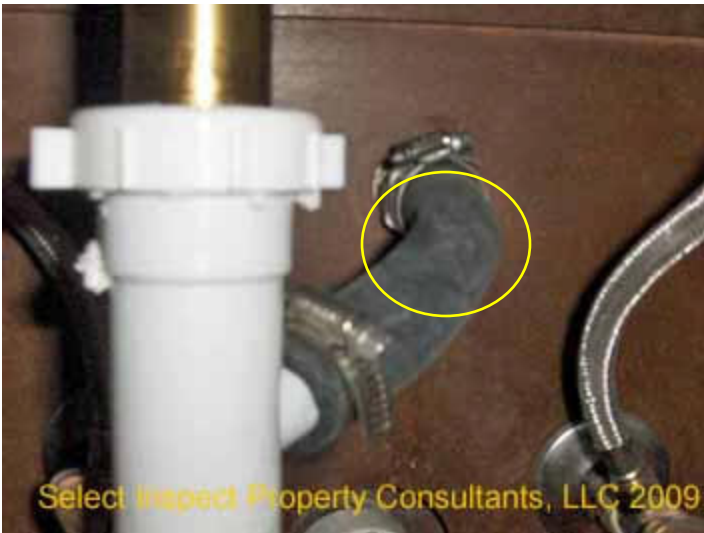
↑ crimped air-conditioner primary condensate line is prone to failure
