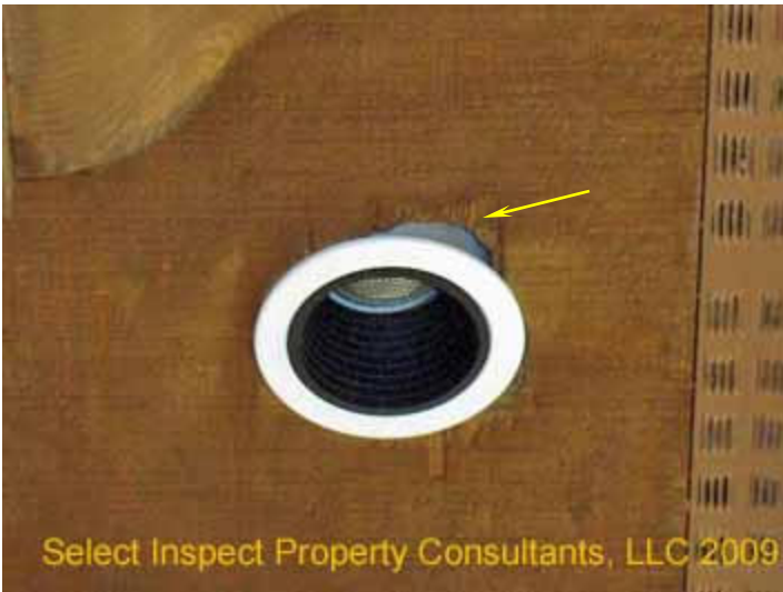
↑ damaged soffit & reveal at southeast eave light
