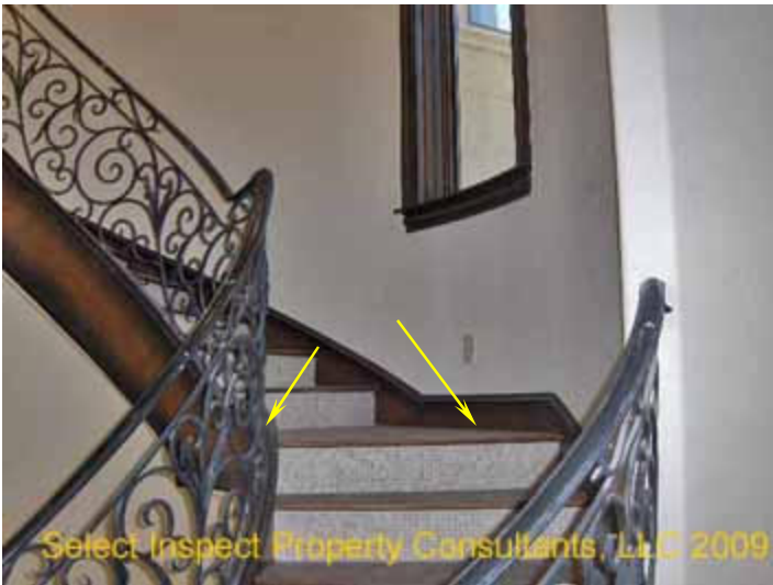
↑ gaps remain at landing
