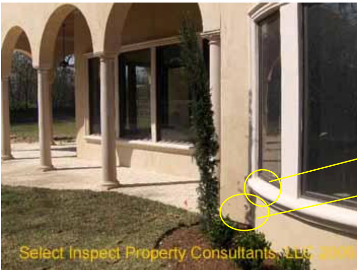
↑ damaged stucco & undetermined open pipe (cleanout?)
