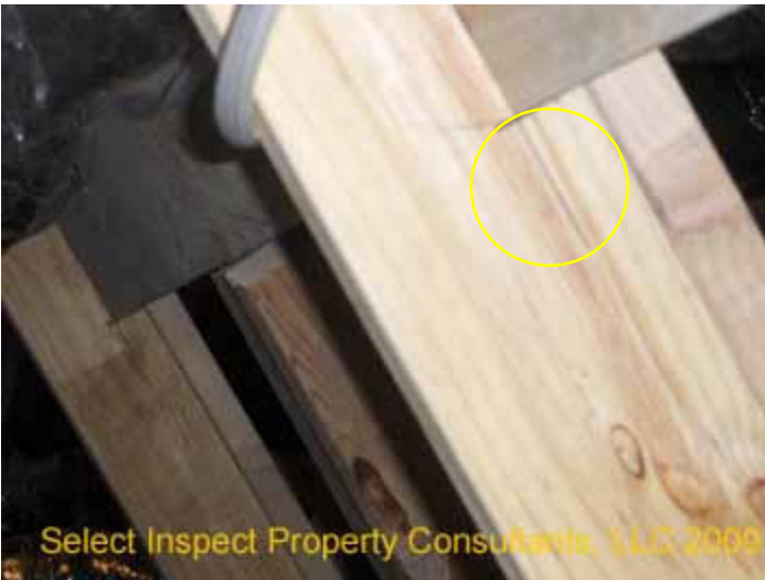
↑ over cut strut; Significant issues were not found or observed concerning this item at the time of inspection
