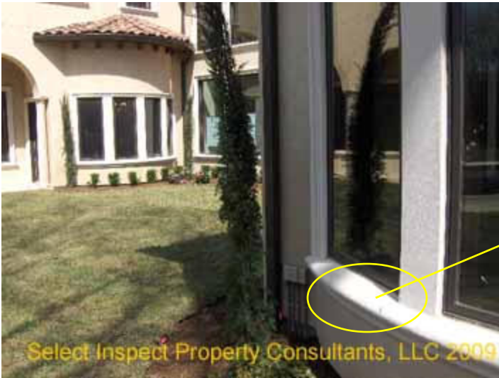
↑ damaged stucco at master bedroom window
