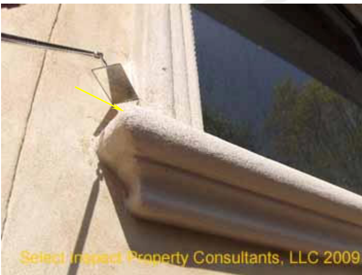
↑ sealant needed; master bathroom
