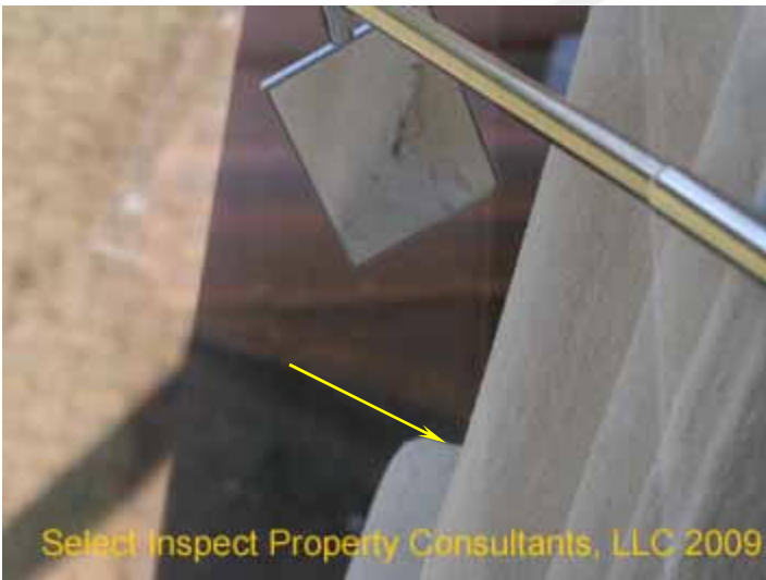
↑ sealant needed; game room window
