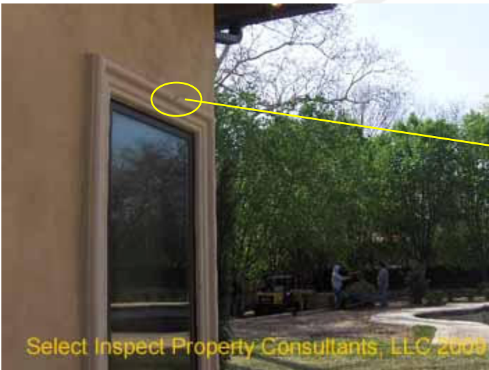
↑ damaged stucco at master bedroom window
