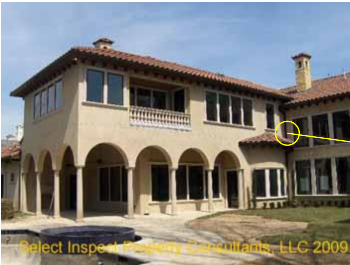
↑ questionable stucco; could not directly access here
