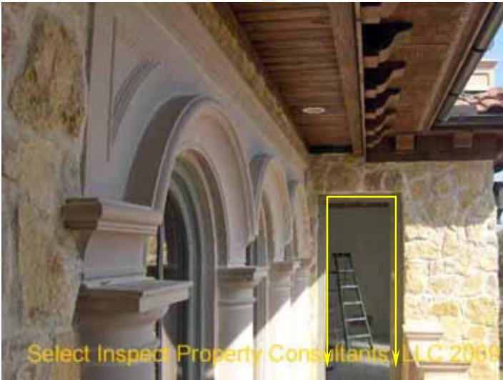
↑ mortar tuck pointing needed & unsealed exterior doorway
