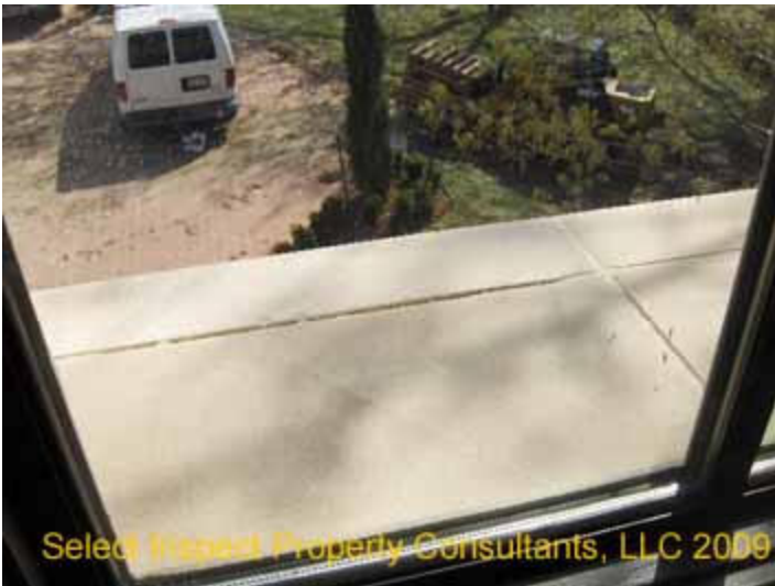
↑ mortar tuck pointing needed
