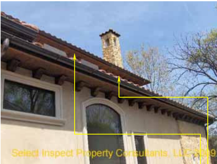
↑ bent soffit vent & unfinished trim/fascia at south
