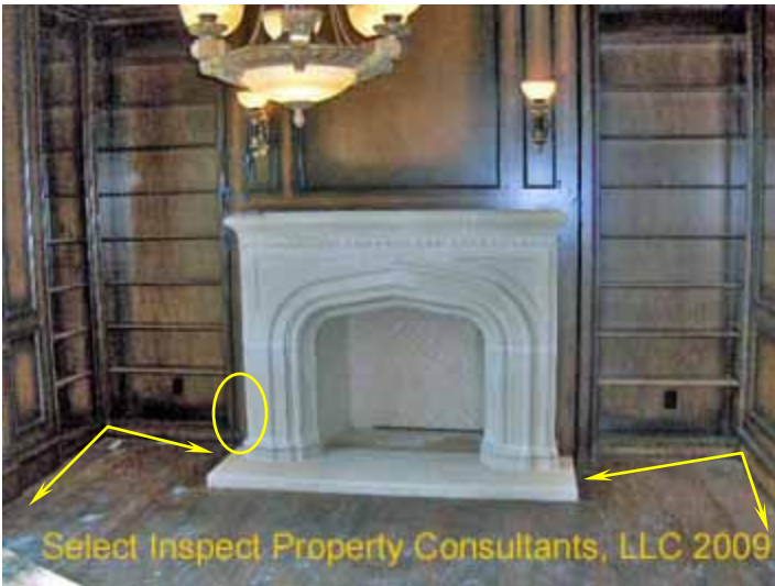
↑ gaps remain at perimeter; peeling veneer at the left
