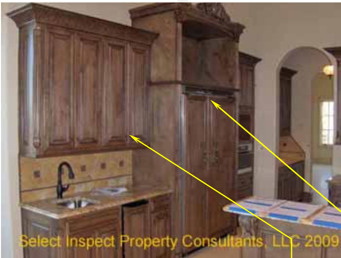
↑ askew cabinet hardware & refrigerator panels
