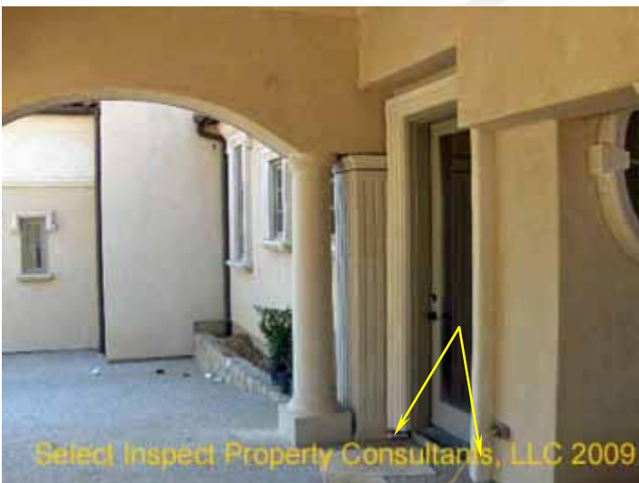
↑ exposed framing/substrate below eastern exterior door
