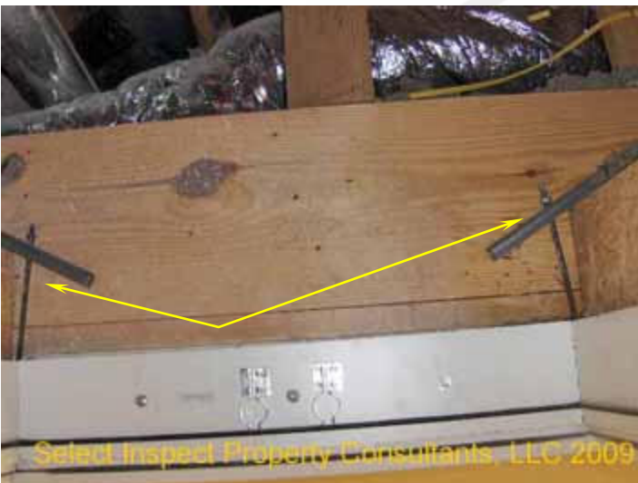
↑ deficient installation of scissor ladder
