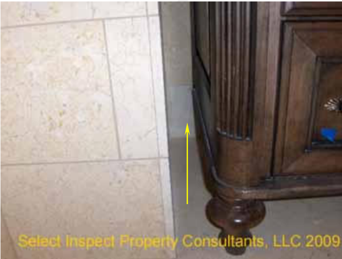
↑ unfinished "hard-board" material at the downstairs 1/2 bathroom.
