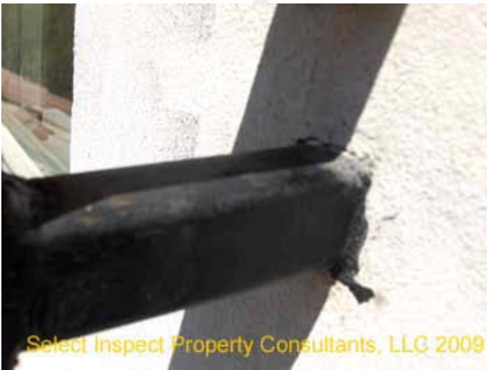
↑ balcony rail mountings should be sealed at stucco wall
