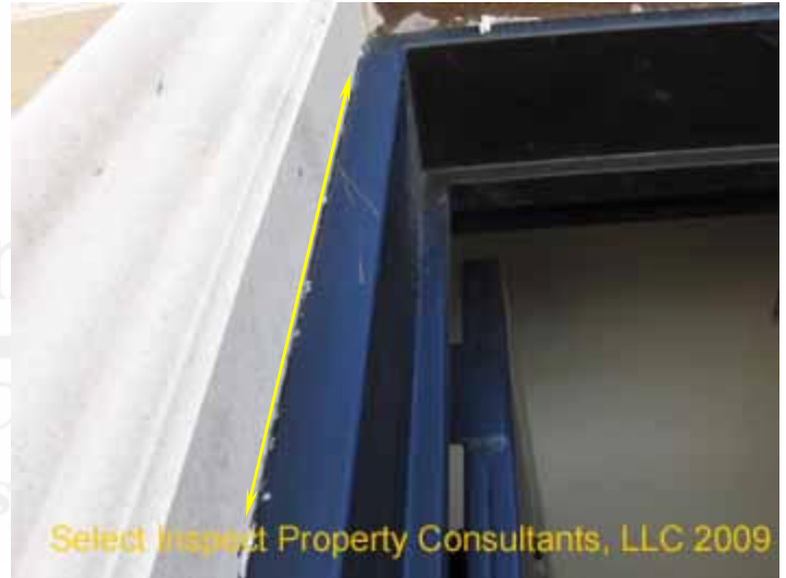
↑ unsealed exterior perimeter
