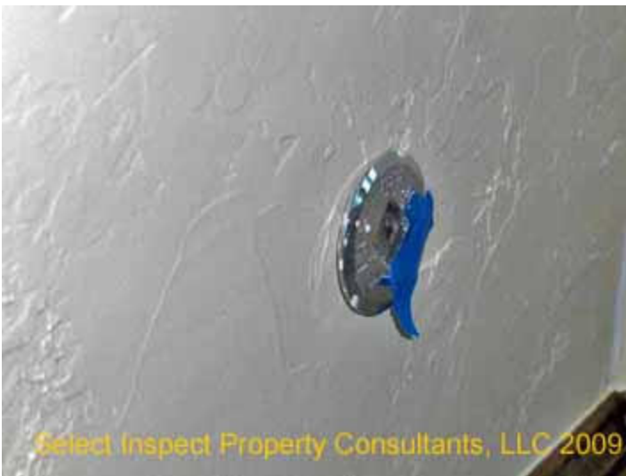
↑ reveal at gas shut-off valve
