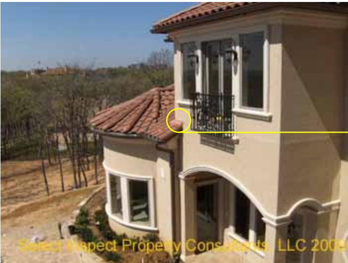
↑ opening exists at flashing
