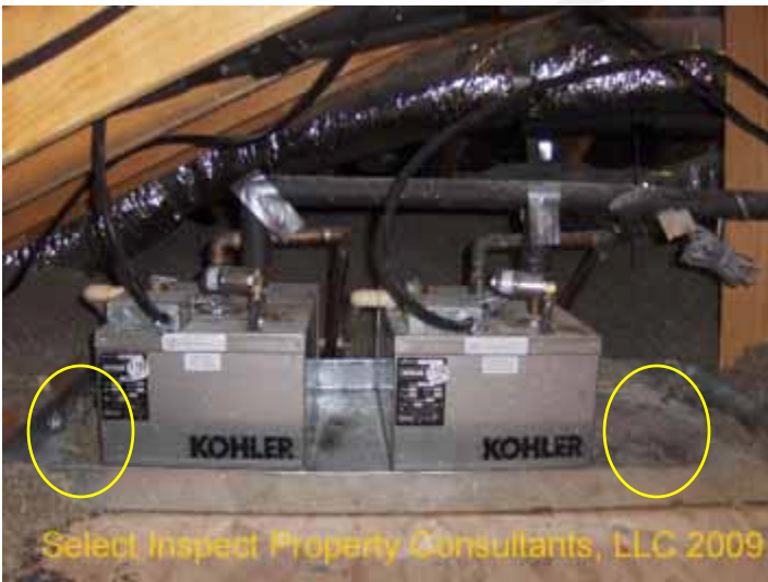
↑ debris should be cleared from the auxiliary pan of the steam equipment
