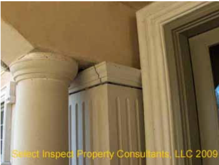
↑ incomplete mortar at the porte-cochere columns; example
