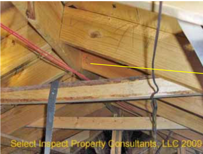
↑ cracked rafter at right of HVAC #5
