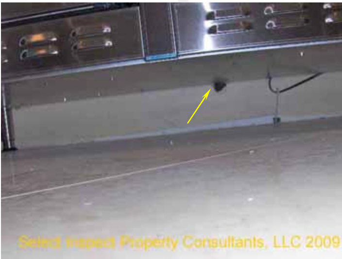
↑ not readily accessible gas shut-off valve at stove/oven
