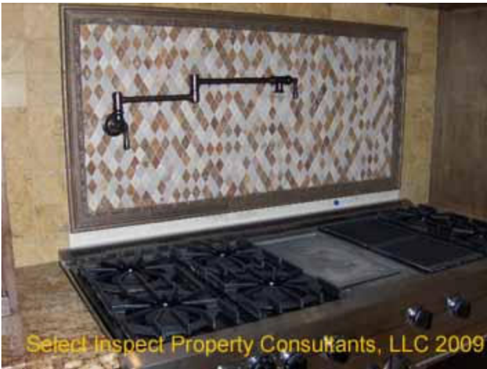
↑ missing tile at stove backsplash
