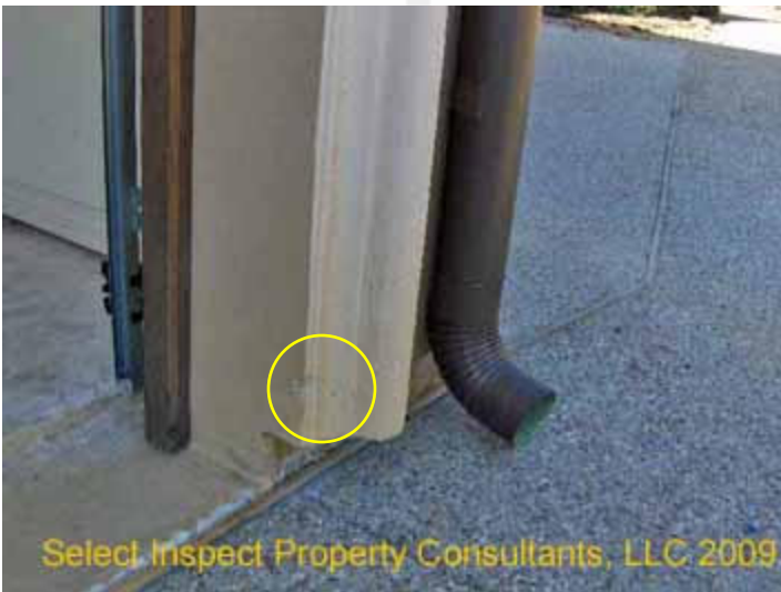
↑ damaged Artificial Stucco / EIFS at the garage trim
