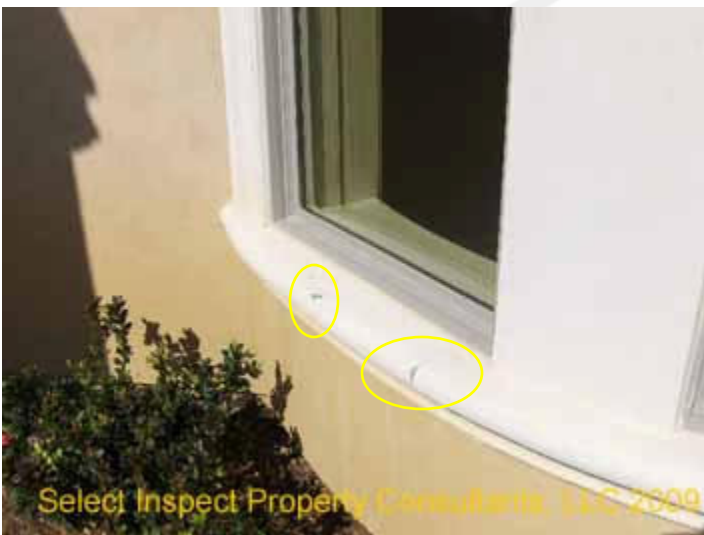
↑ damage/openings at the dining room window sill
