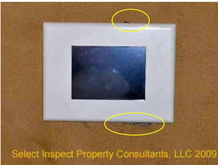
↑ openings at the patio smart system control
