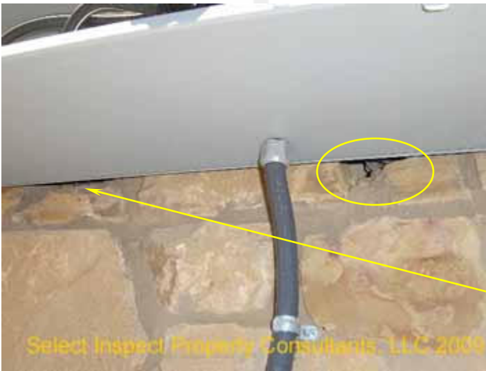
↑ unworkmanlike conduit (lack of securing nut) and openings below raceway
