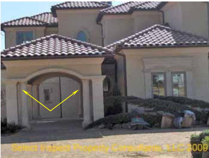
↑ incomplete mortar at porte-cochere columns
