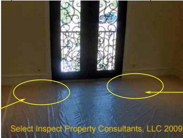
↑ moisture discovered at the northern bedroom balcony area; interior flooring
