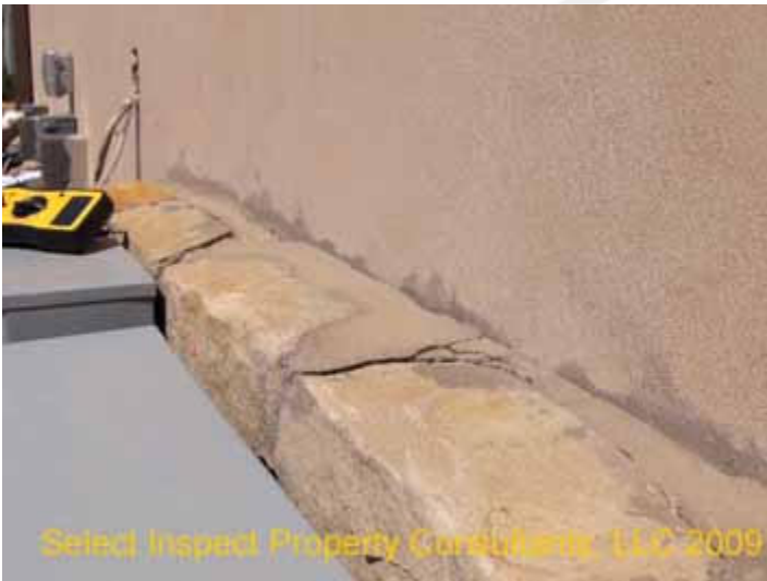
↑ cracked stone mortar at the electrical service
