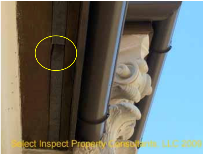
↑ deficient soffit vent near north balcony
