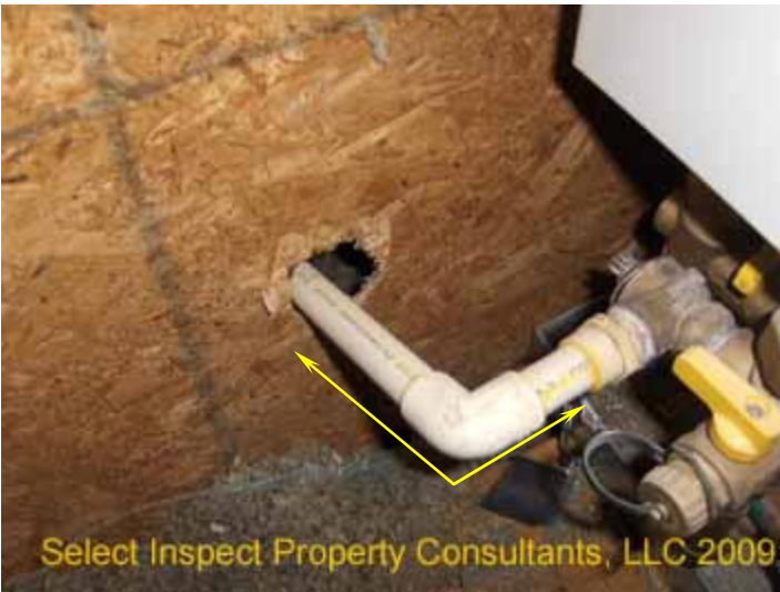
↑ drain piping is +- .035" less inside diameter than required by the temperature-pressure-relief manufacturers.
