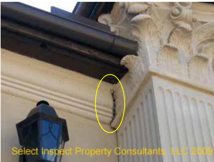
↑ unfinished stucco edge at the upper front column
