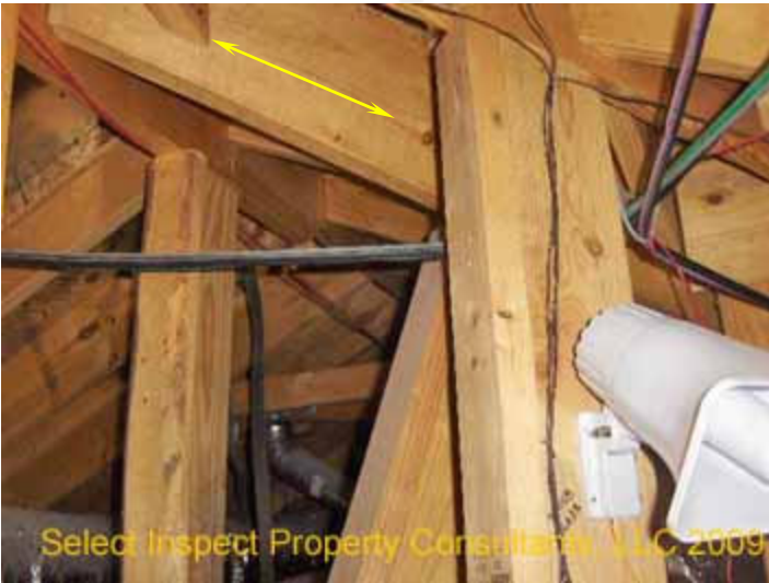
↑ cracked rafter at left of HVAC #5
