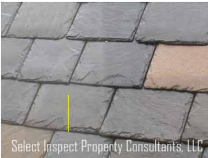
↑ cracked slate north of bedroom 2 front window; minor
