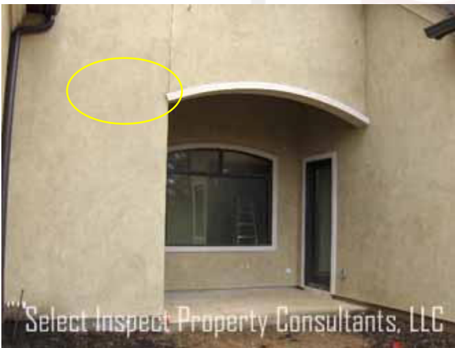
↑ stress crack at master north patio
