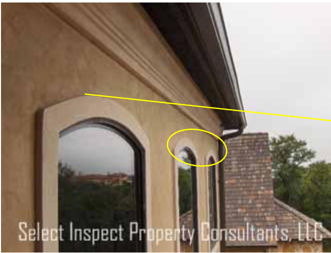
↑ damaged artificial stucco at top of living room windows
