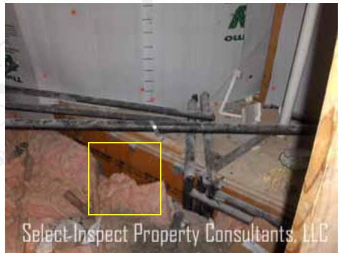
↑ deficient insulation above laundry room
