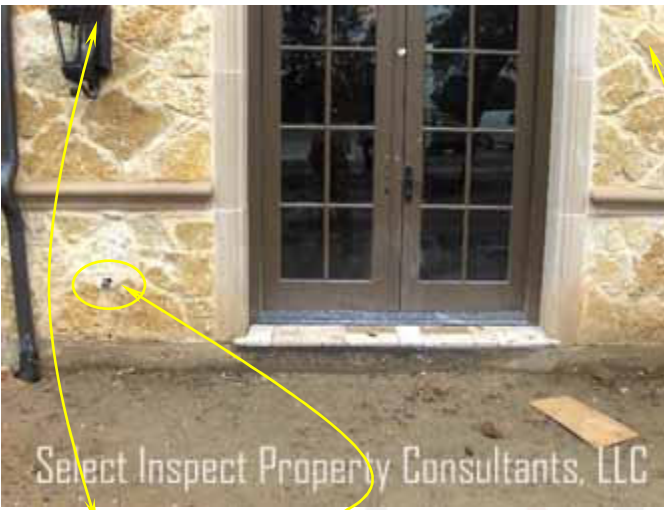
↑ openings & unsealed wall at gas valve component(s); right lamp was missing
