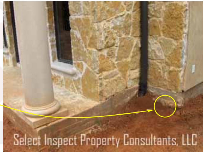
↑ form stake at the master patio should be removed
