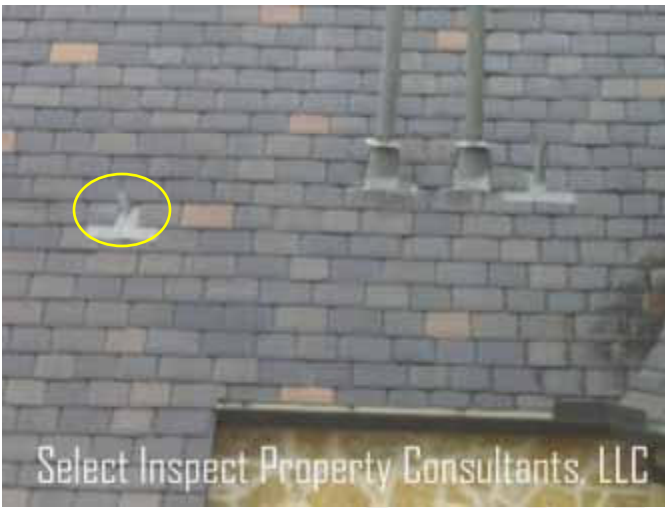
↑ plumbing vent less than 6" above roof; drive side of porte-cochere
