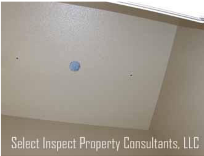
↑ openings & missing light; guest bath closet
