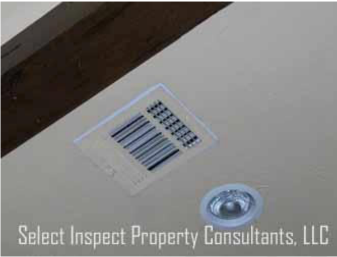
↑ paint needed at office/study air registers; supply & return
