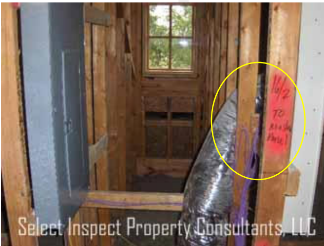
↑ crimped air ducting; example; south walk-in attic
