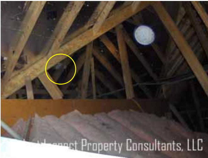
↑ some attic fans & all fan thermostat(s) were not readily accessible
