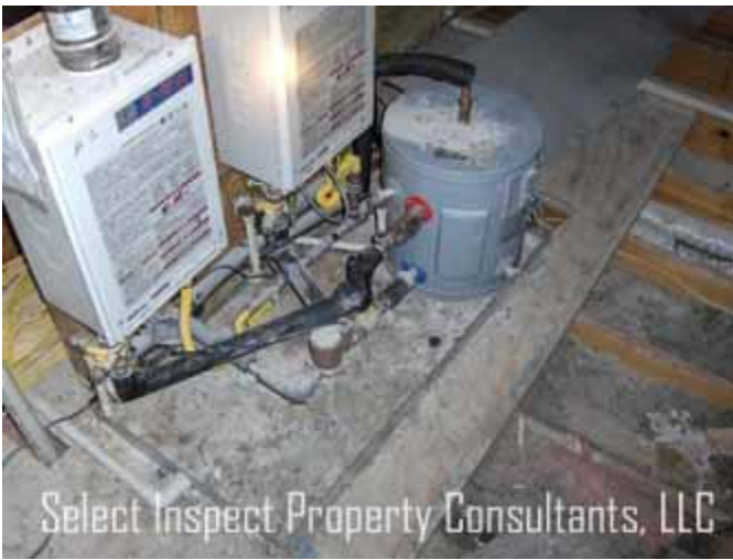
↑ debris in water heater pans should be cleared
