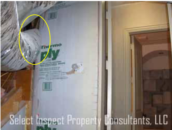
↑ crimped air ducting; example at south walk-in attic
