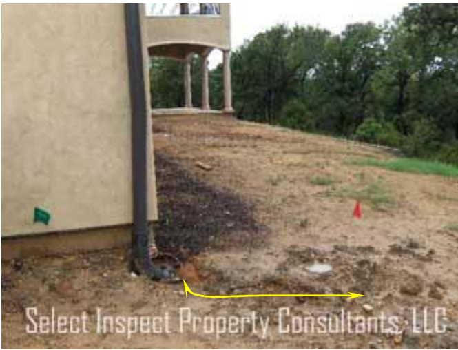
↑ incomplete area drain at north corner of three-car garage
