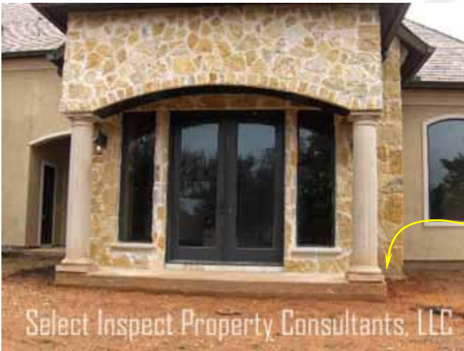
↑ uncaulked windows & door perimeter at master
