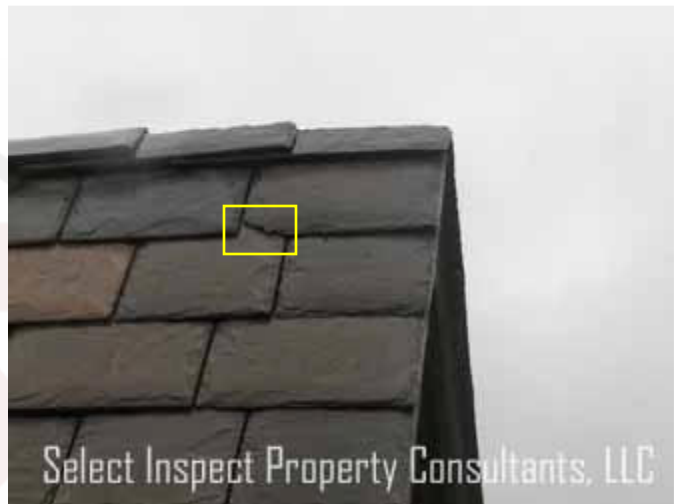
↑ chipped slate corner at peak above media room
