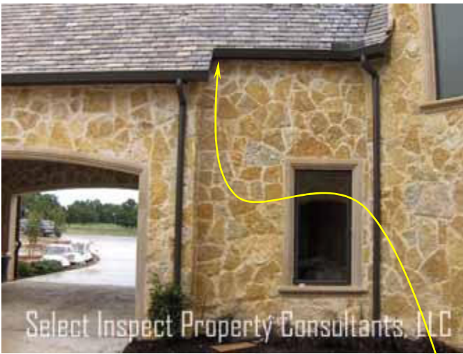
↑ deficient termination of exhaust fan(s)
