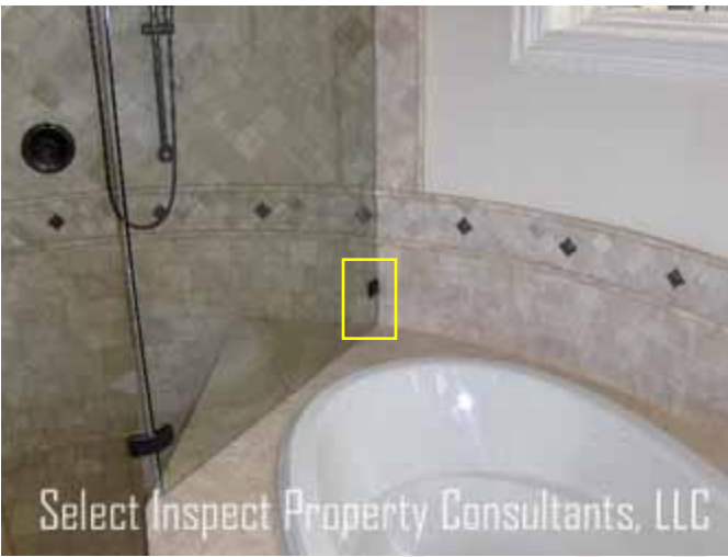
↑ glass wall leaks at bathroom #2 mounting component(s)
