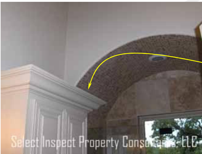
↑ incomplete finish at guest bath tile/cabinet
