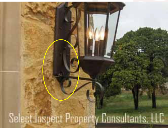
↑ damaged coach at east corner of three-car garage
