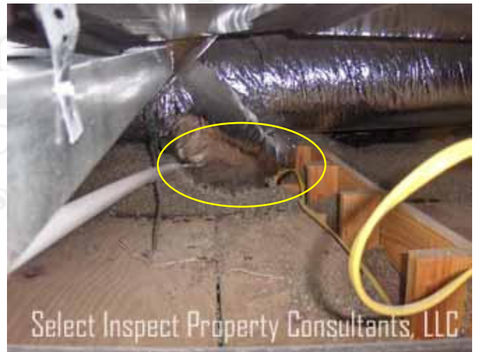
↑ crimped air ducting; example HVAC #2; north attic
