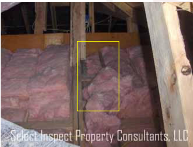
↑ deficient insulation above the family room
