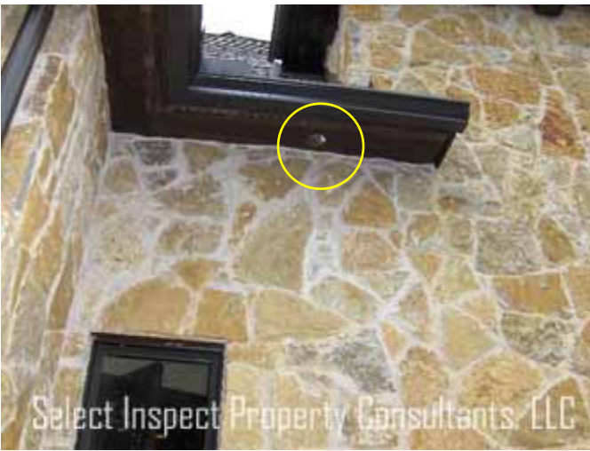
↑ deficient exhaust fan(s) termination at master bathroom
