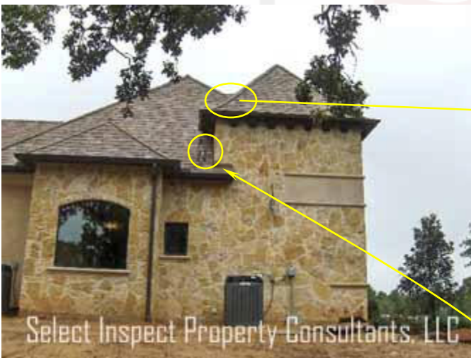
↑ slipped shingle & questionable plumbing vent flashing at south above master bathroom
