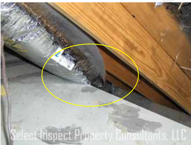
↑ crimped air ducting; example HVAC #2; north attic
