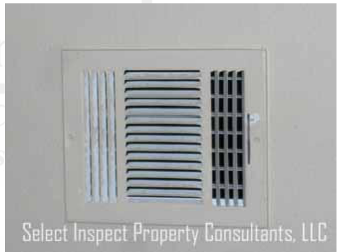
↑ unworkmanlike paint at guest bedroom air register
