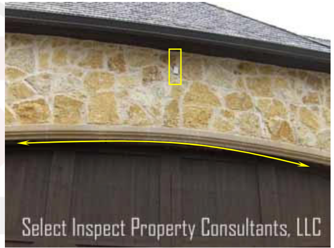
↑ recommend sealant at detached garage junction box & header was incomplete
