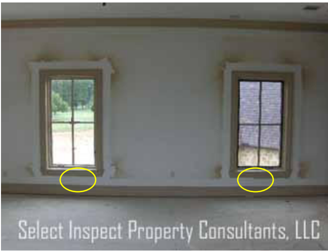
↑ stress cracks at gameroom #2
