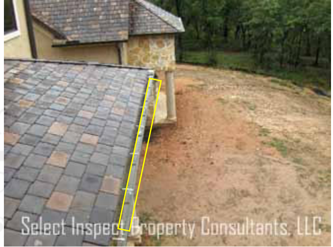
↑ negative gutter slope at rear porch
