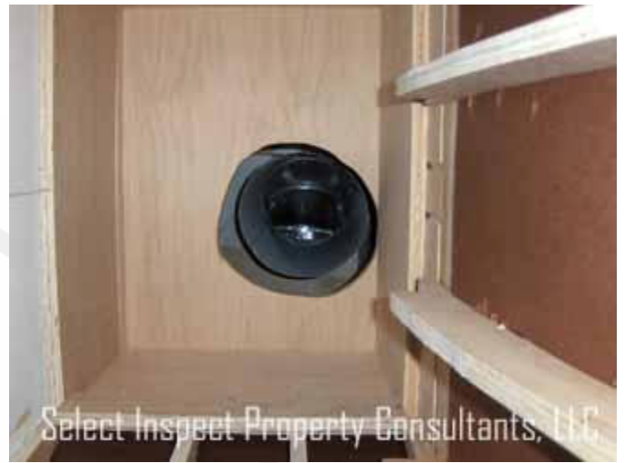
↑ may be difficult connecting kitchen vent to not readily accessible vent duct
