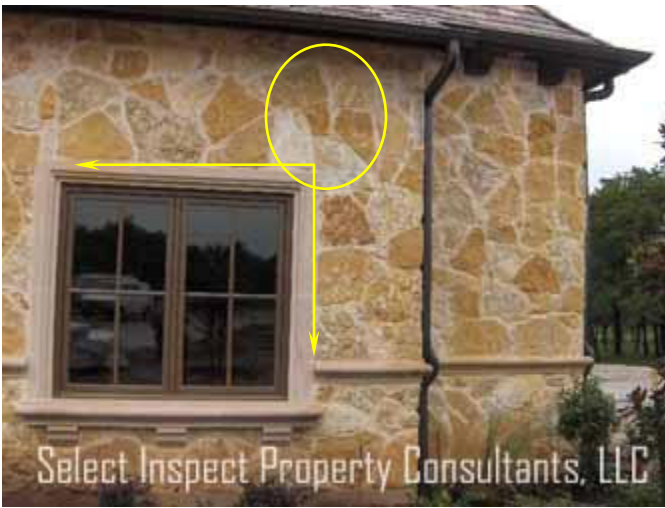
↑ nails & stress crack at detached garage window
