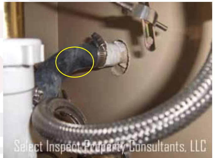
↑ crimped condensate drain may be prone to failure; condition minor during the inspection; bathroom #4
