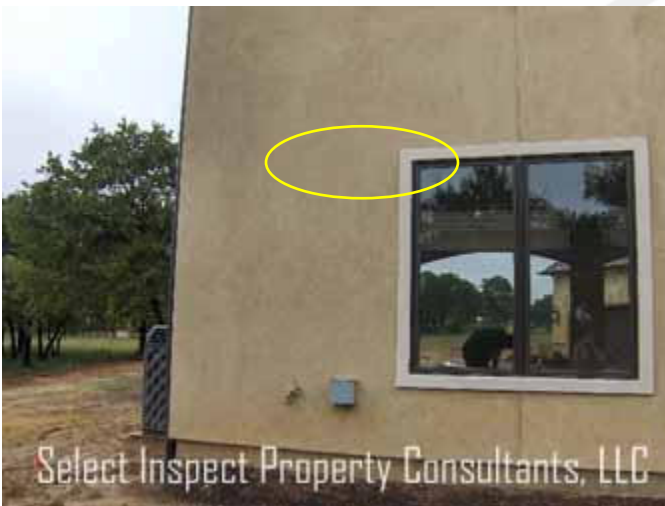
↑ stress crack at north
