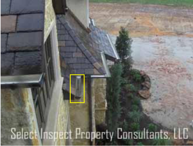
↑ negative gutter slope at porte-cochere
