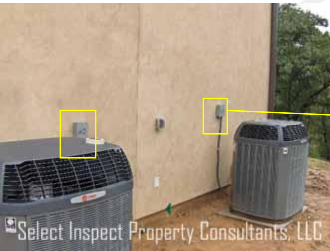
↑ sealant needed at condenser(s) service disconnects
