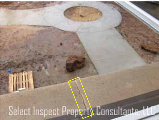
↑ example stone sill mortar needing tuck-pointing
