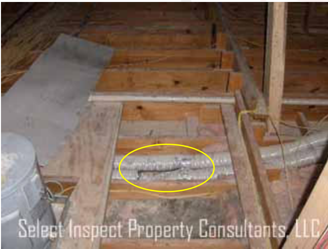
↑ damaged exhaust fan(s) duct in east walk-in attic
