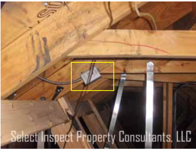
↑ deficient thermostat(s) control at upper north attic; from bedroom #5; control was recessed into the junction box
