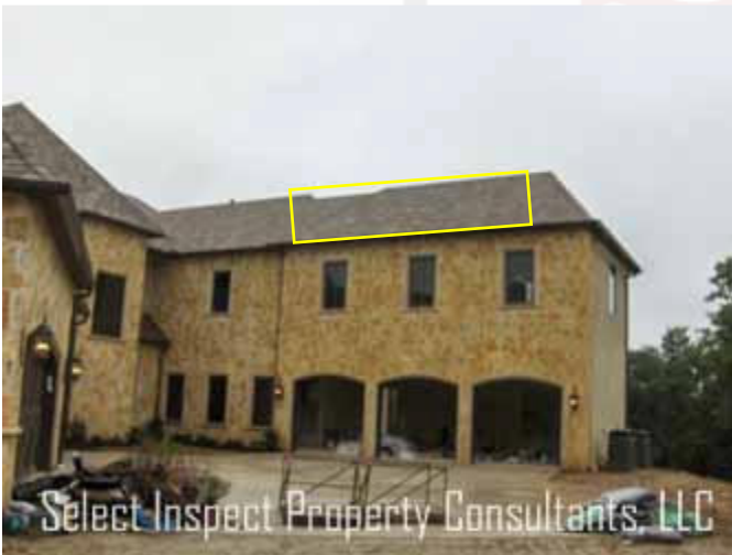
↑ example uneven slate at roof
