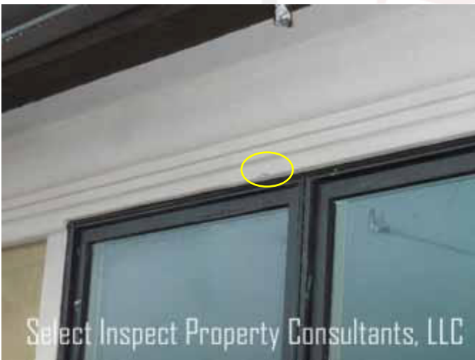
↑ damaged artificial stucco at top of bedroom #5 window
