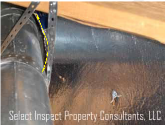
↑ #3 flue did not meet clearance requirements to combustibles; upper central attic
