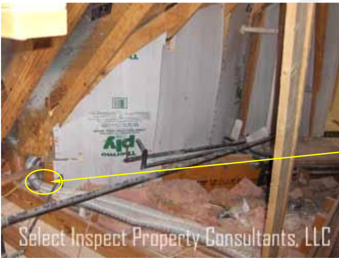
↑ damaged/disconnected exhaust fan(s) duct in east walk-in attic
