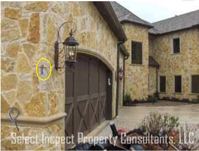
↑ caulking/sealant needed atop exterior lights; example & mortar deficient at detached garage
