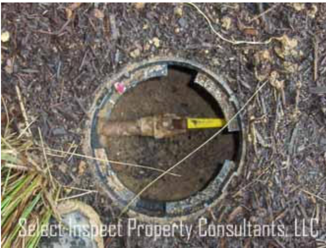
↑ Shut-off-valves require 3" clearance from soil; handle is corroded; right of front entry
