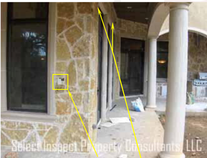
↑ deficient junction box cover & junction box seal at rear porch
