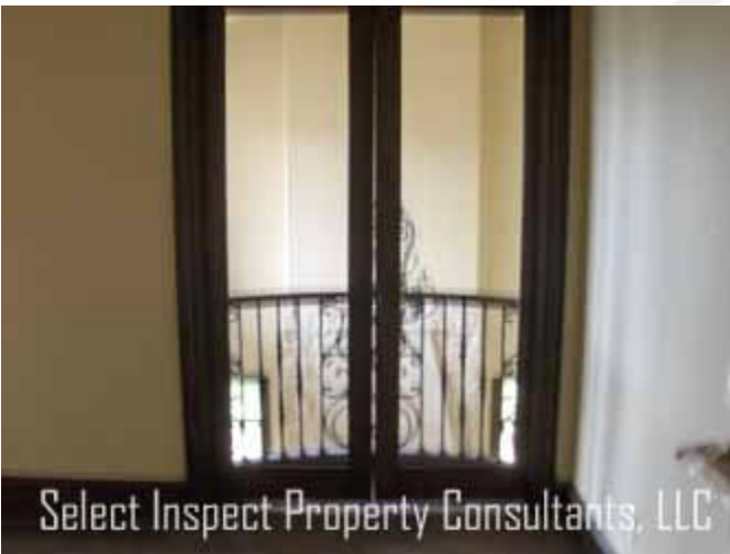
↑ gameroom loft doors were unsquare & not functioning as intended
