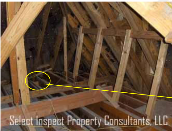
↑ marginal boring; metal reinforcement plate not seen at gas penetration through top plate at detached garage attic
