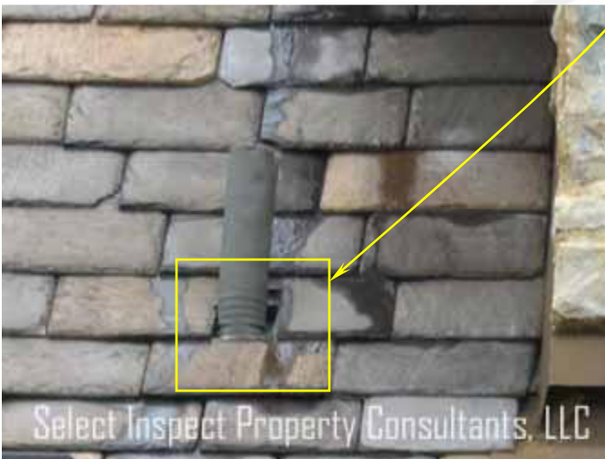
↑ close view of image above; apparent opening & this was inconsistent with other plumbing vents
