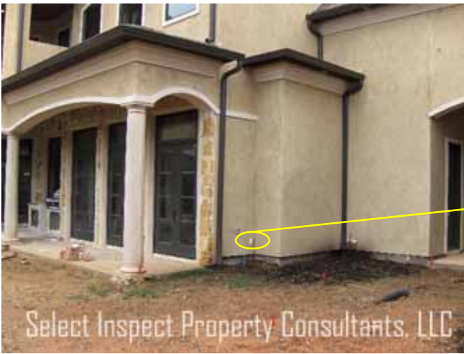
↑ deficient stucco at living room west
