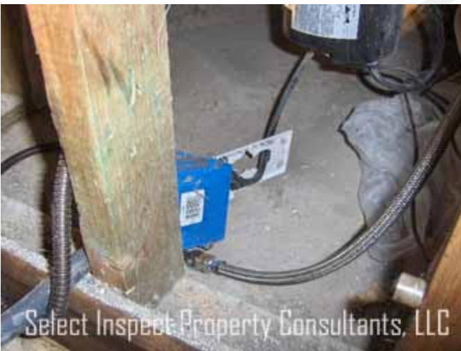
↑ deficient cover & unsecured receptacle below jetted tub
