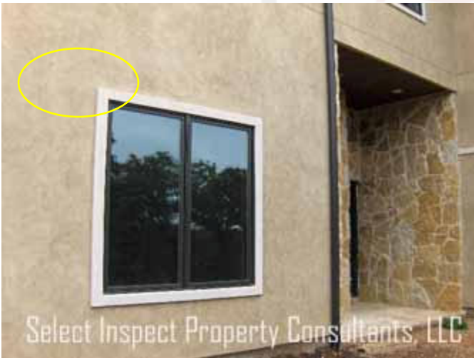
↑ stress crack at guest bedroom window
