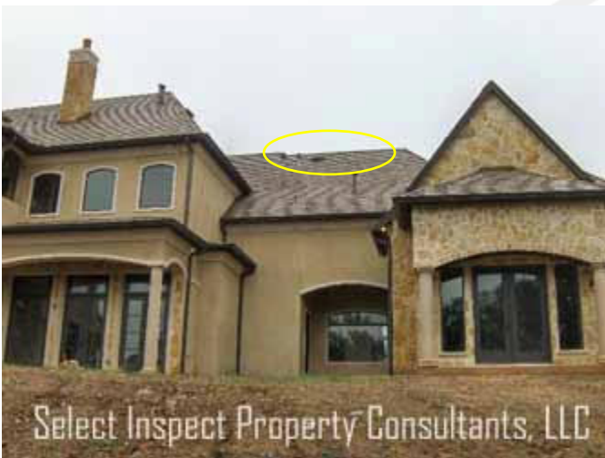
↑ missing shingles at west roof ridge
