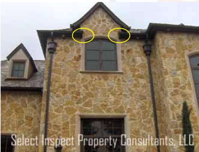
↑ recommend sealant at eave/wall
