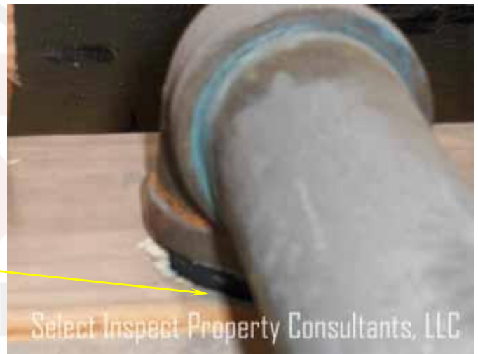
↑ close view of image at left; ideally the opening should be minimum 5/8" from plate edge
