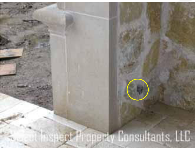
↑ seal needed at front porch gas valve
