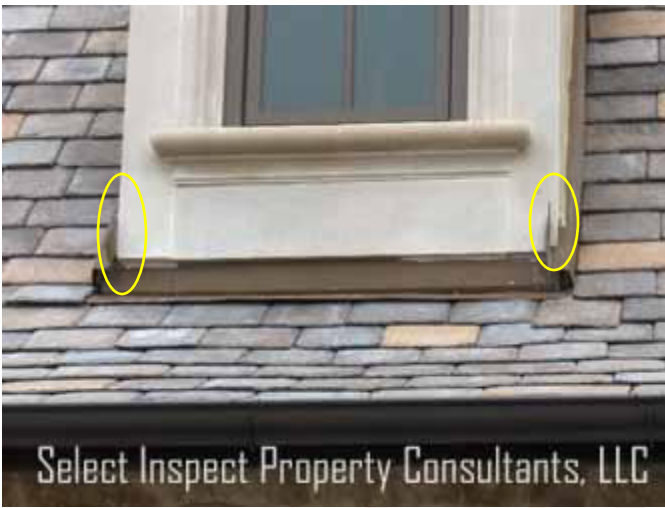
↑ recommend sealant at flashing details; detached garage dormer
