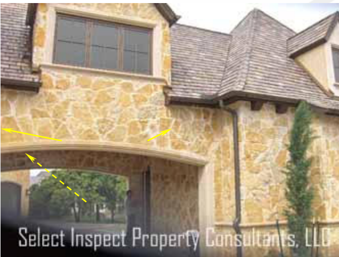
↑ same as above & cracks discovered
