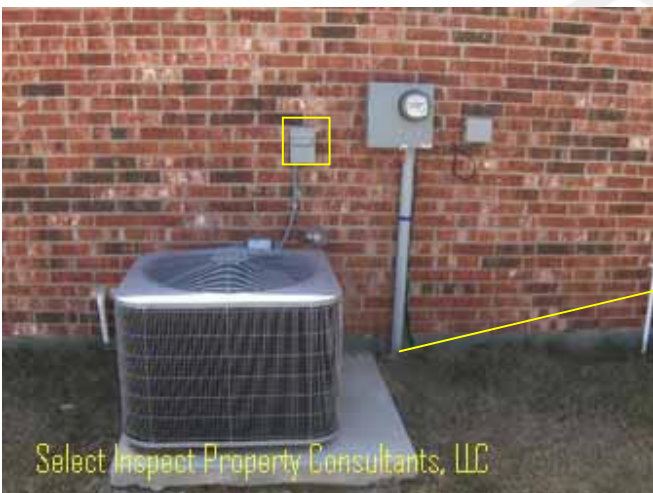
↑ incorrect location of air conditioning condenser(s) service disconnect; inadequate clearance of electrical panel for service personnel
