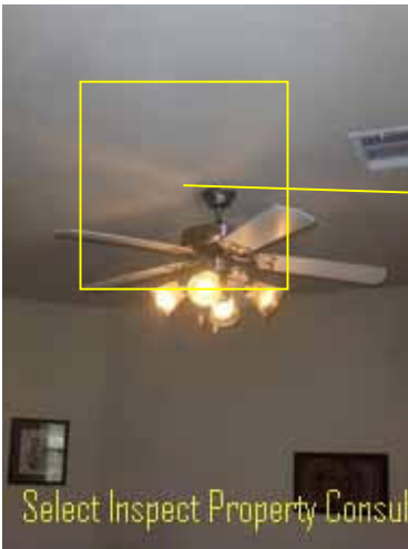
↑ Thermal imaging indicated slightly warmer area at master ceiling
