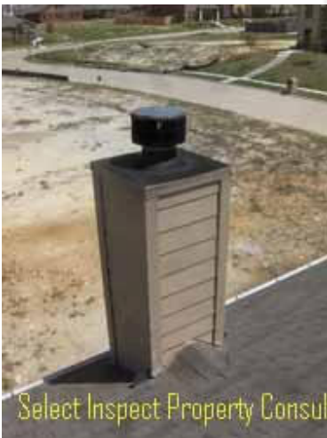
↑ soot staining at chimney cap
