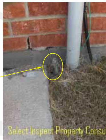
↑ grounding electrode protrudes grade; deficient
