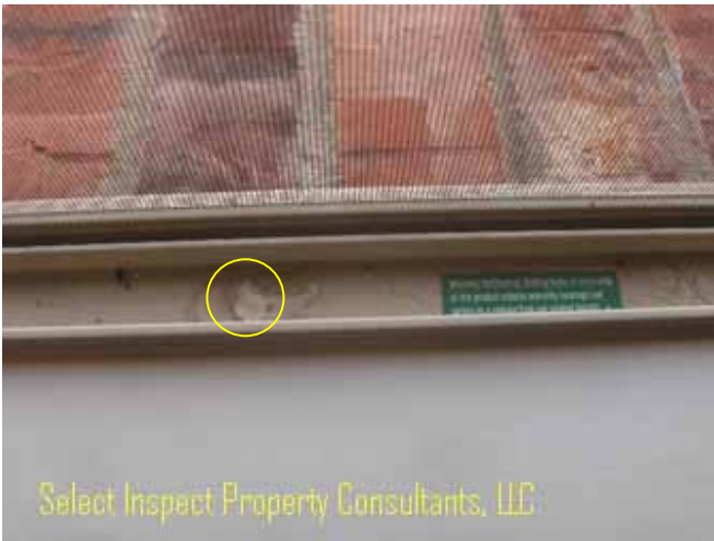
↑ Alarm holes at the lower portion of the window voids the manufacturer warranty
