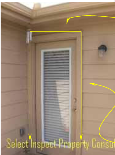
↑ sealant needed at door perimeter & trim / siding joints
