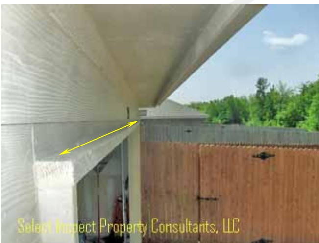
↑ inadequate paint (exposed wood) at overhead door header
