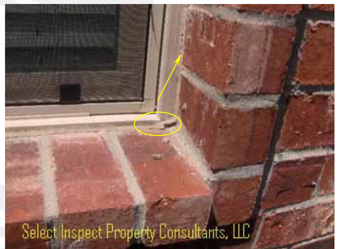
↑ sealant touch-up needed at windows; example
