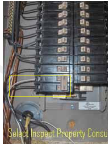
↑ inadequately sized electrical conductors at pool equipment 30amp overcurrent-protection-device; unworkmanlike.
