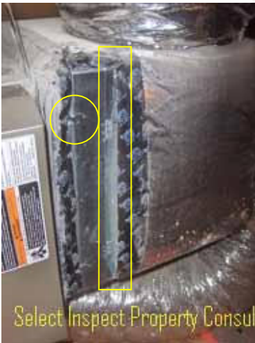
↑ inadequate seal & deficient filter door latch- HVAC #3 in attic
