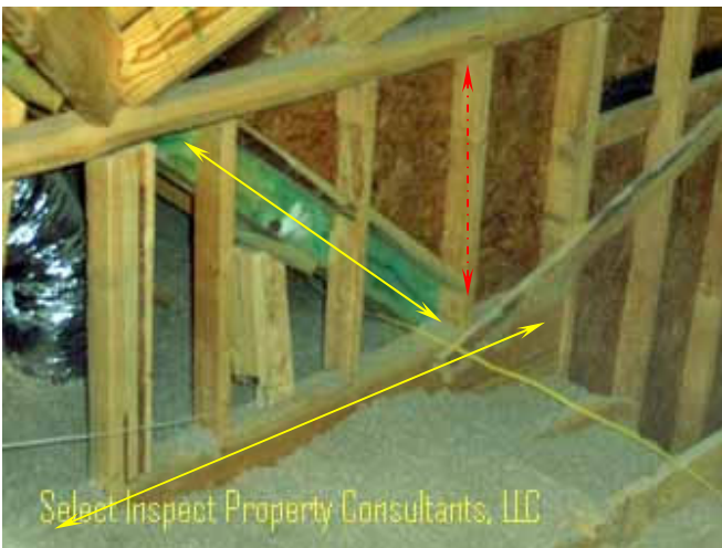
↑ attic adjacent the images above- red line is approximately location of exterior mortar crack
