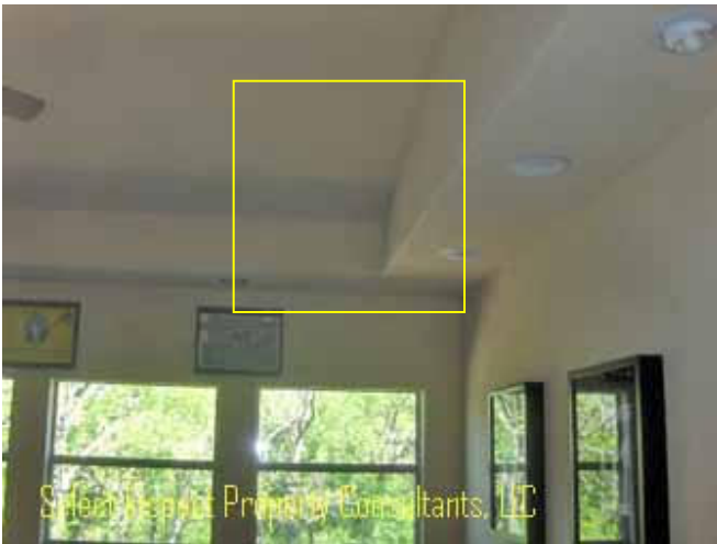
↑ Thermal imaging implies energy loss at gameroom northeast
