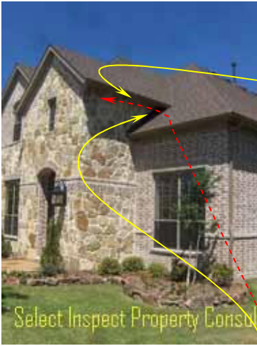
↑ structural stress evidence at the southeast
