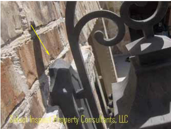
↑ caulking/sealant needed atop exterior lights; example
