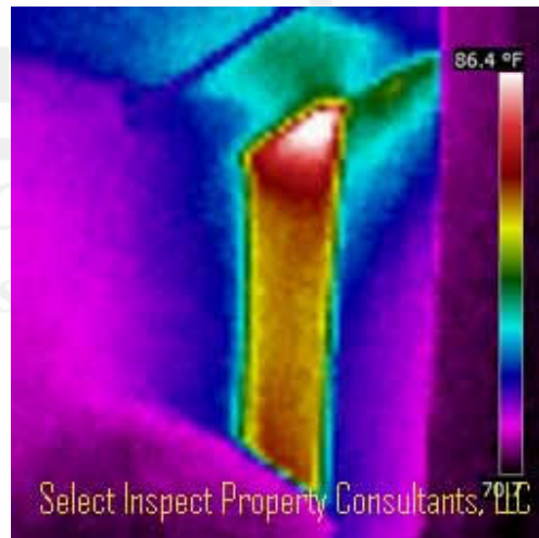
↑ the dryer vent during operation is naturally warmer than the wall, though there may be lacking insulation in the wall void at this chase
