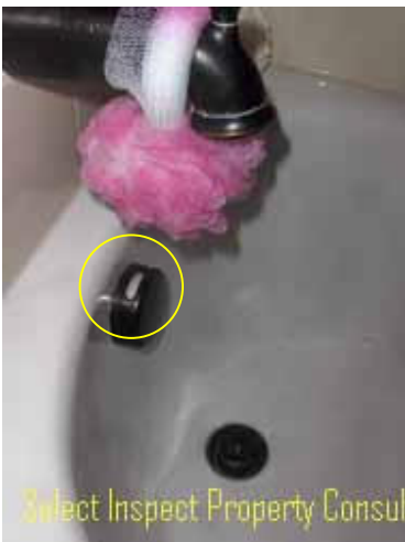
↑ inverted overflow at upstairs bathroom east
