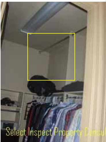
↑ Thermal imaging implies energy loss at master closet adjacent the dryer vent
