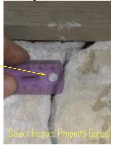
↑ + 1/8" during the inspection
