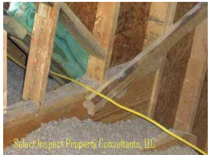
↑ close view of image at left; obvious stress not discovered, though suspect down load stress toward the south of the diagonal beams (green/treated)
