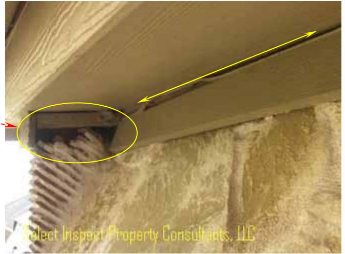
↑ missing trim & sealant stress separation at frieze-board/soffit
