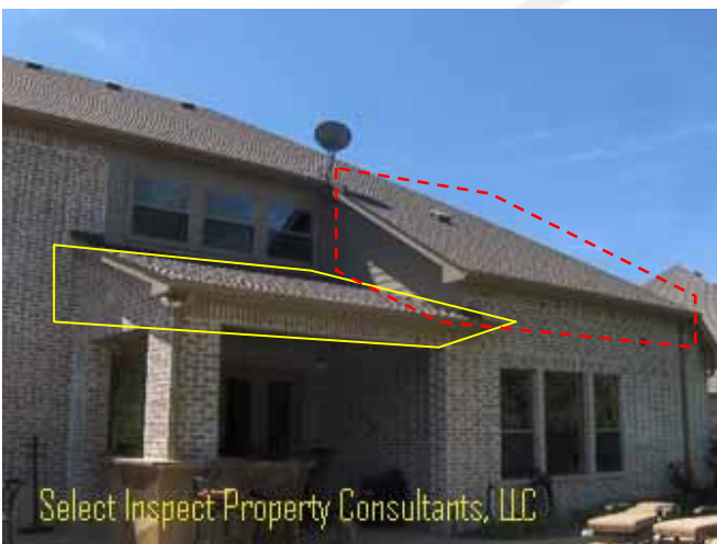
↑ missing upper venting at rear porch attic-inaccessible; missing access to attic above the master bedroom
