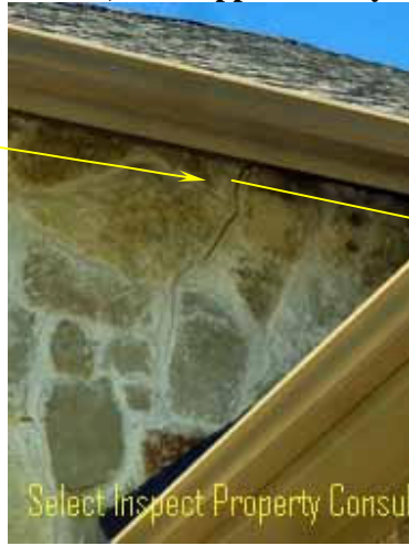
↑ close view of image at left; mortar crack
