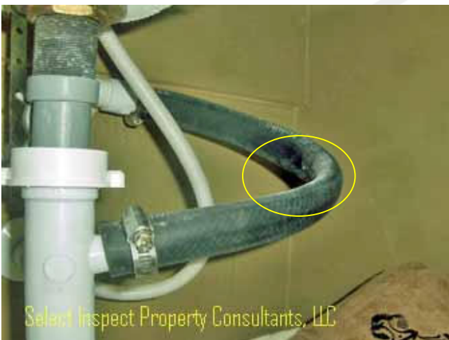
↑ crimped condensate drain is prone to failure
