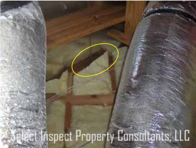
↑ amiss insulation at gameroom northwest corner
