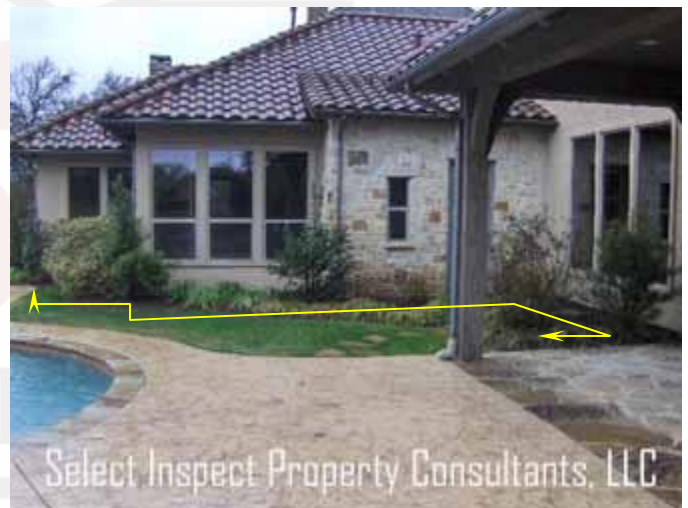
↑ poor drainage at rear; multiple locations & pooling water
