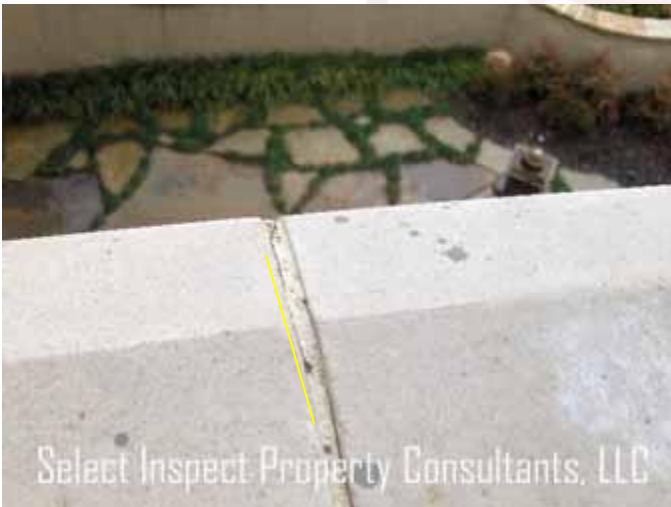
↑ cracks at cast stone mortar; example
