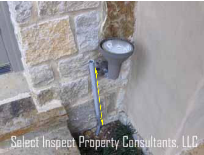
↑ undetermined conduit & wiring at front porch
