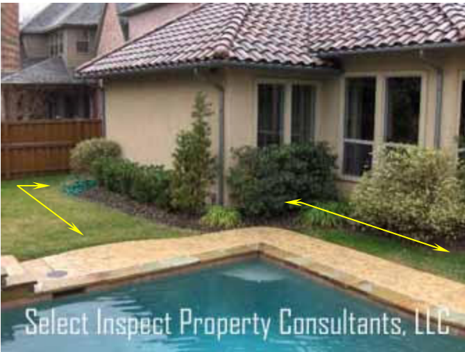
↑ poor drainage at the southeast
