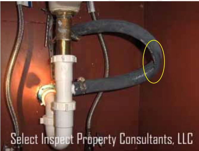
↑ crimped condensate drain is prone to failure; split bath
