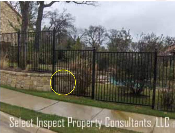
↑ loosely secured stone & example location of retaining wall cracks
