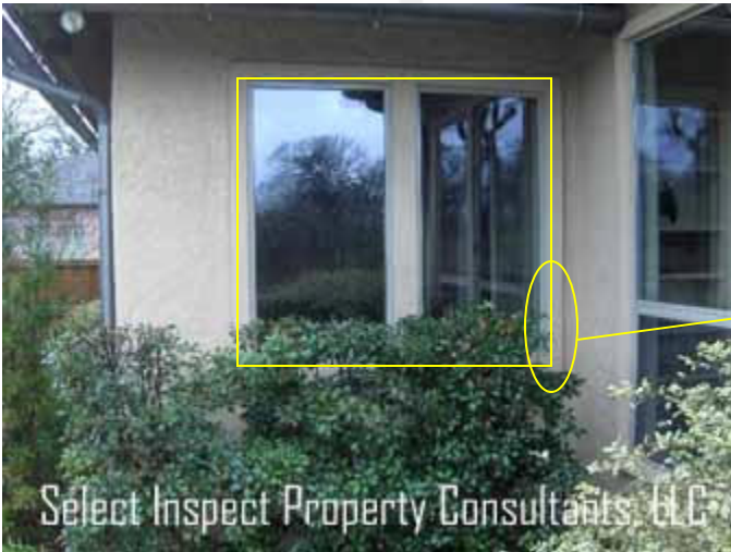
↑ damaged stucco/artificial stucco & sealant needed
