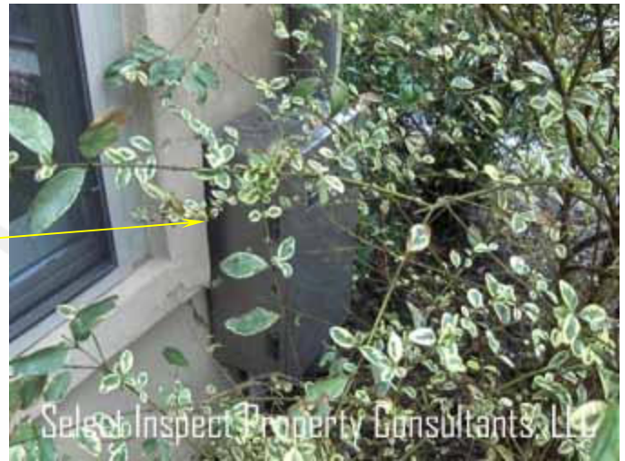
↑ close view of image at left; electrical box was also inadequately secured
