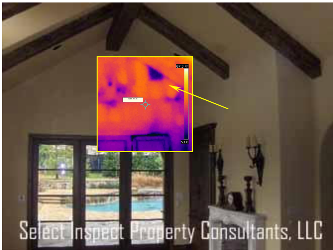
↑ darker thermal areas imply apparent missing insulation at breakfast nook vault wall & slight air infiltration at the doorway (common)
