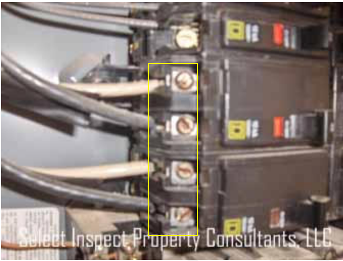
↑ moisture evidence/corrosion at electrical component(s); right panel
