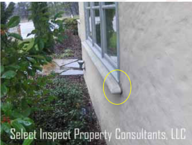
↑ sealant needed; example
