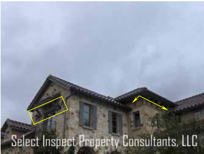
↑ sealant needed at beam penetrations
