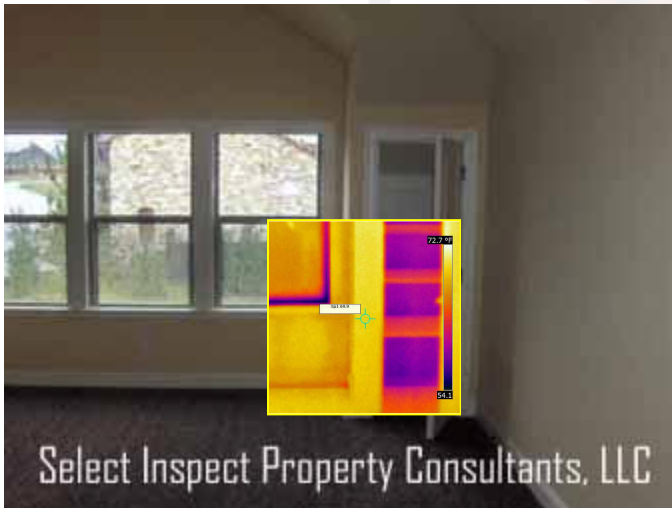
↑ darker thermal areas imply gameroom closets to have lacking insulation at exterior wall; example at right side closet
