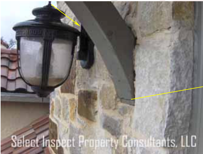
↑ sealant needed; example at lights & beam
