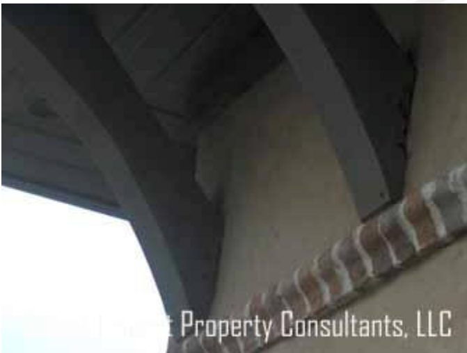
↑ sealant needed; close view of image above
