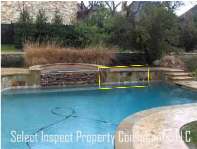
↑ thin cracks & efflorescent noted at pool wall; Significant issues were not discovered; monitor & maintain.
