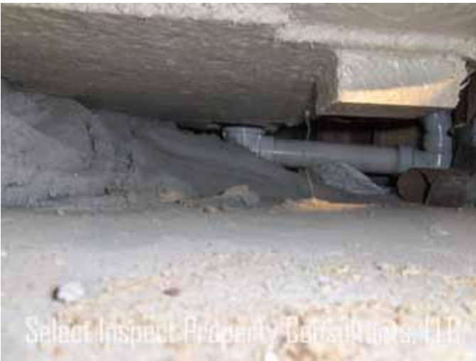
↑ incomplete mortar bed support below master bathtub
