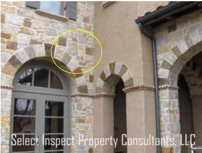
↑ crack at mortar
