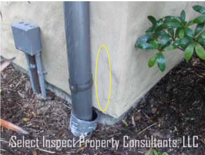
↑ crack at stucco; & sealant needed at penetrations; master east
