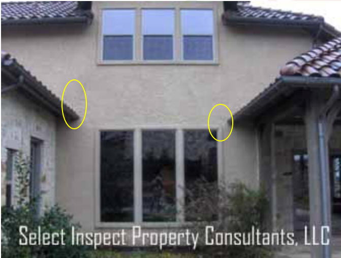
↑ cracks at stucco
