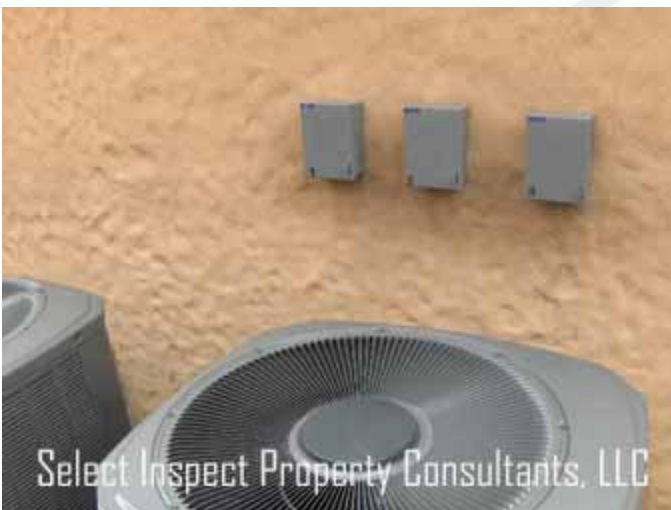
↑ incorrect location of air conditioning condenser(s) service disconnect
