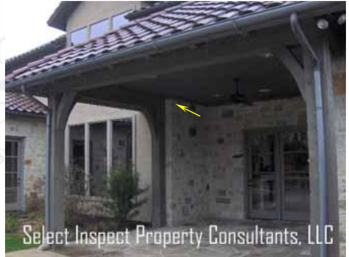
↑ crack at mortar
