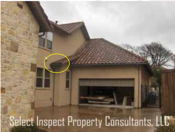
↑ amiss gutter slope; not draining
