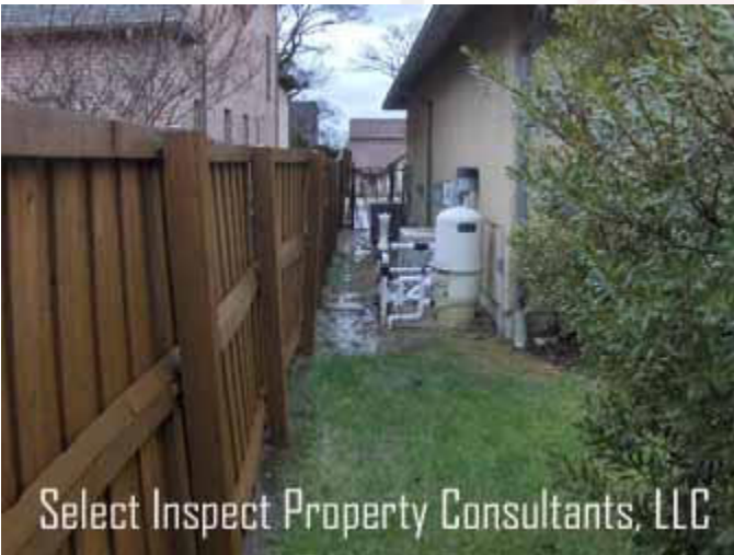
↑ poor drainage at the south
