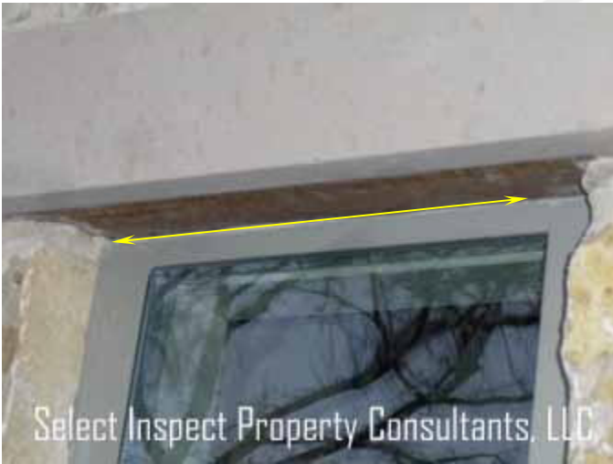
↑ undetermined flashing & sealant recommended at window lintels; example
