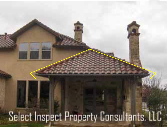
↑ rear porch attic did not have an access; Conditions in not readily accessible/inaccessible locations remain undetermined
