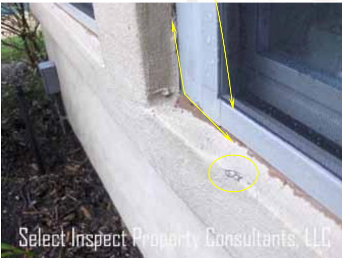
↑ damaged stucco/artificial stucco trim & sealant needed
