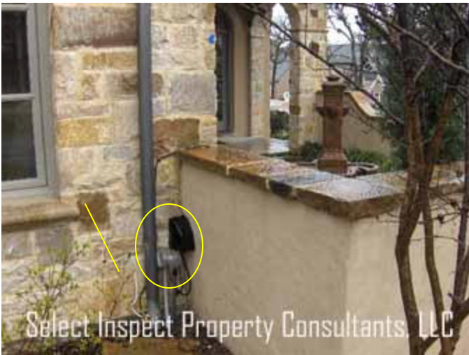
↑ crack at mortar & deficient electrical weatherproofing
