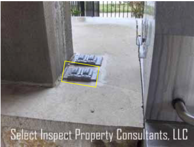
↑ receptacle at grill prone to moisture intrusion; front receptacle was not ground-fault circuit interrupt (GFCI) protected
