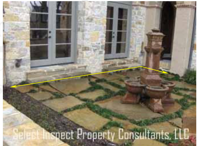
↑ high soil example & weep openings not discovered at front porch
