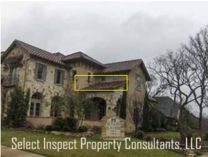
↑ cracked tile had been patched; chipped tile noted
