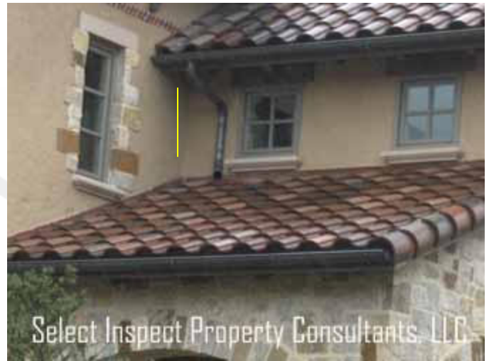
↑ crack at stucco
