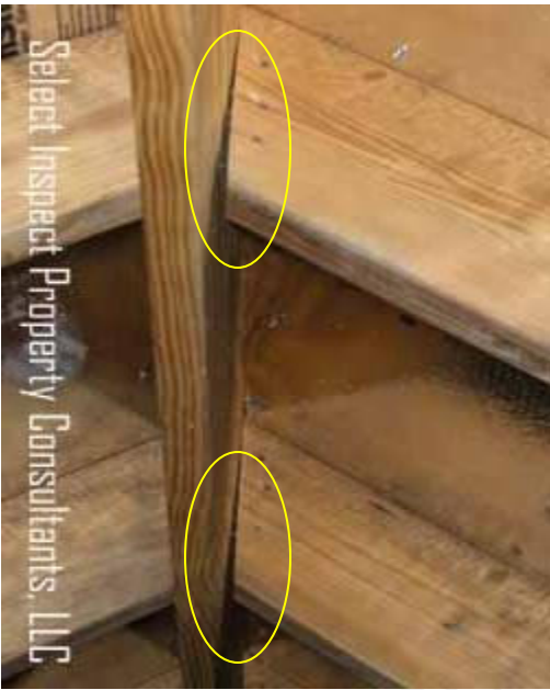
↑ slight separation at rafter in single garage attic
