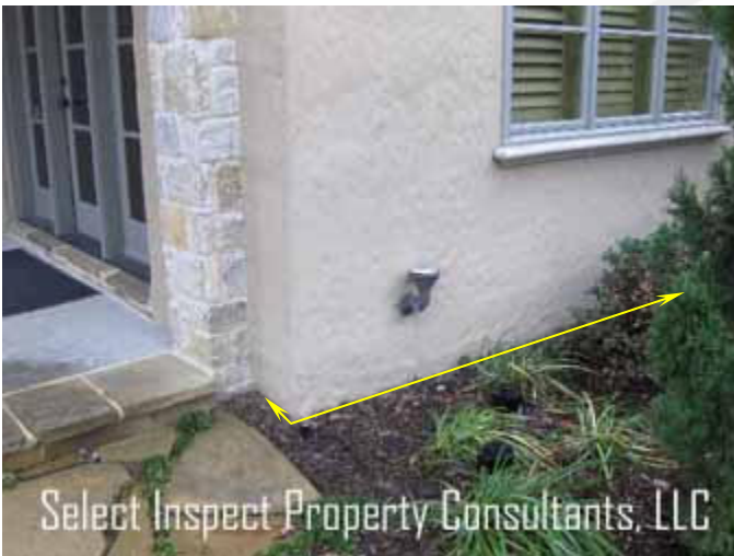
↑ high soil at stucco; obstructed stucco weep screed/drainage; library
