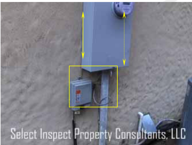
↑ sealant needed at equipment boxes/penetrations
