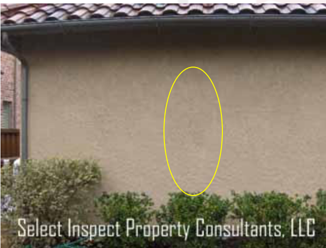
↑ cracks at stucco; master east
