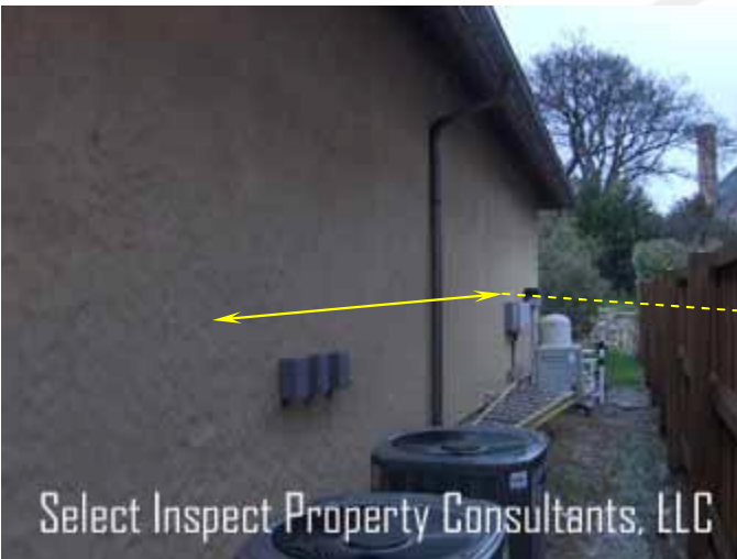
↑ cracks at south stucco
