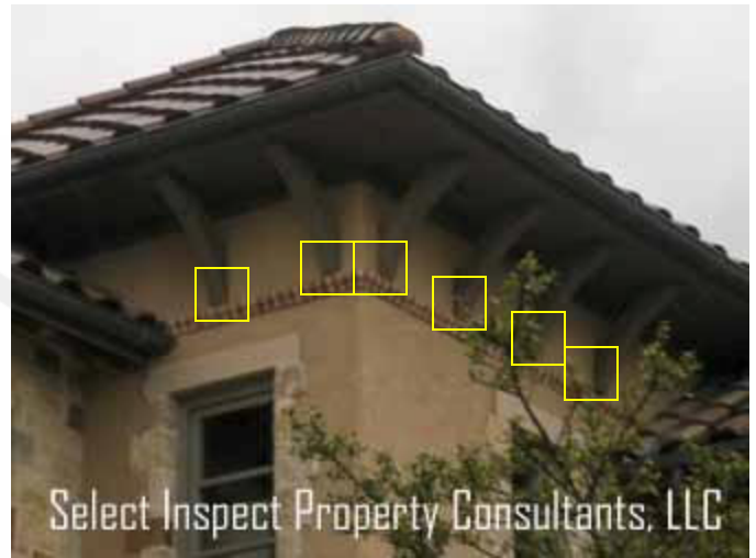
↑ sealant needed; example; close view of image at left
