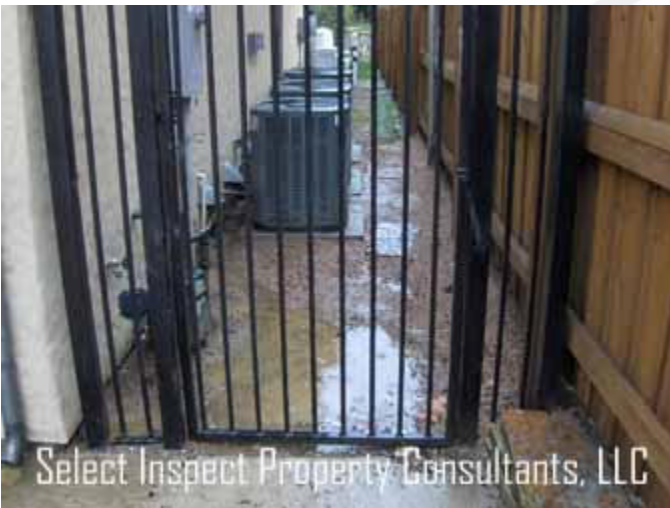
↑ poor drainage at the south; driveway is higher than grade; pooling water
