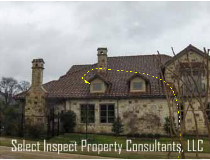
↑ moisture staining at interior of dormer
