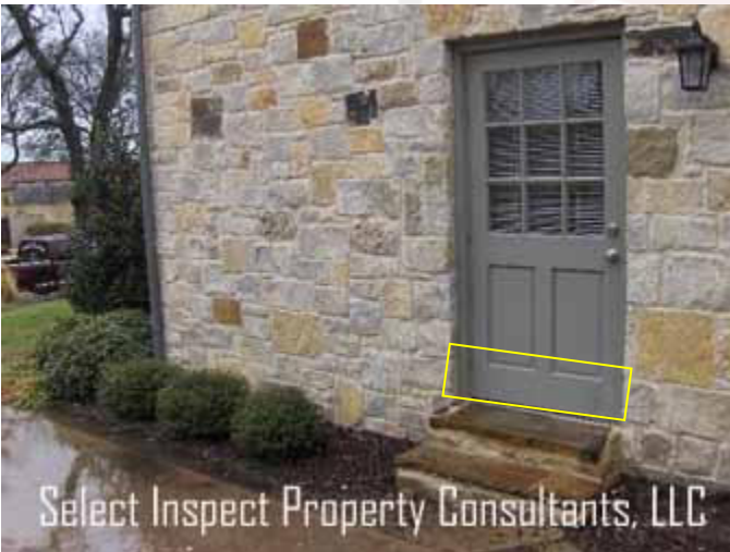
↑ exterior door damage
