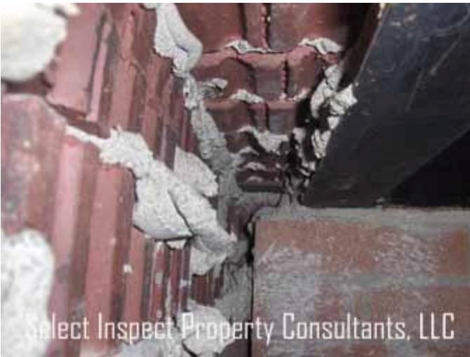
↑ inadequate seal at fireplace lintel/smoke shelf
