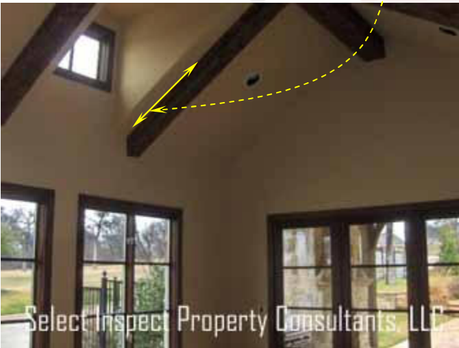
↑ moisture staining at interior drywall
