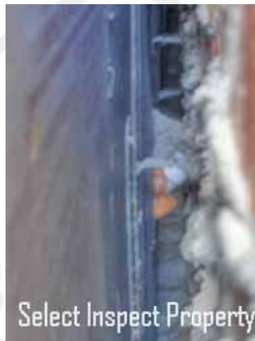
↑ debris in wall void
