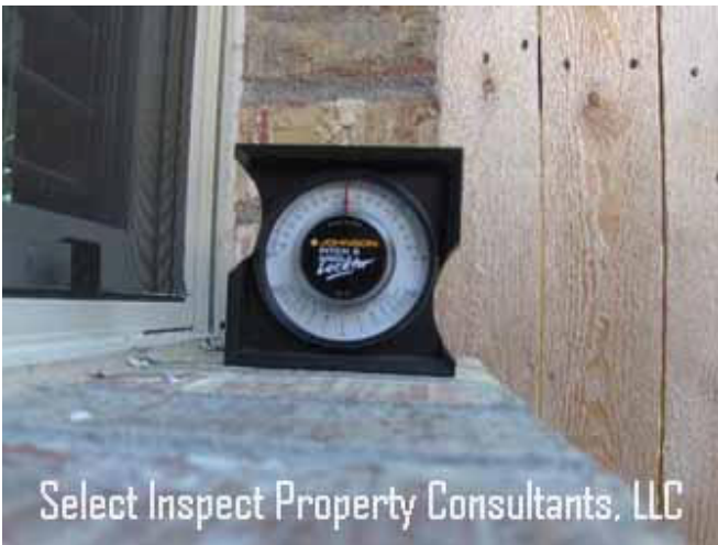
↑ brick ledge(s) had inadequate slope; example
