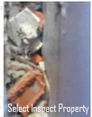
↑ debris in wall void
