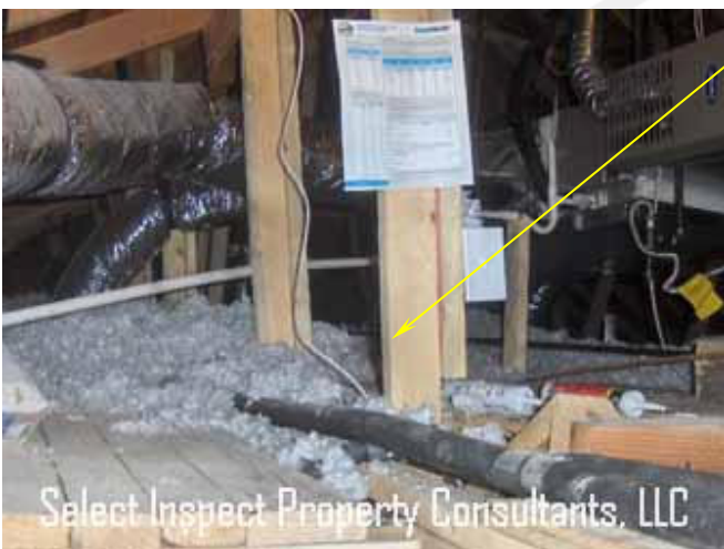
↑ there should be a minimum 24" pathway to the HVAC from the top of the access, with no gaps or obstructions
