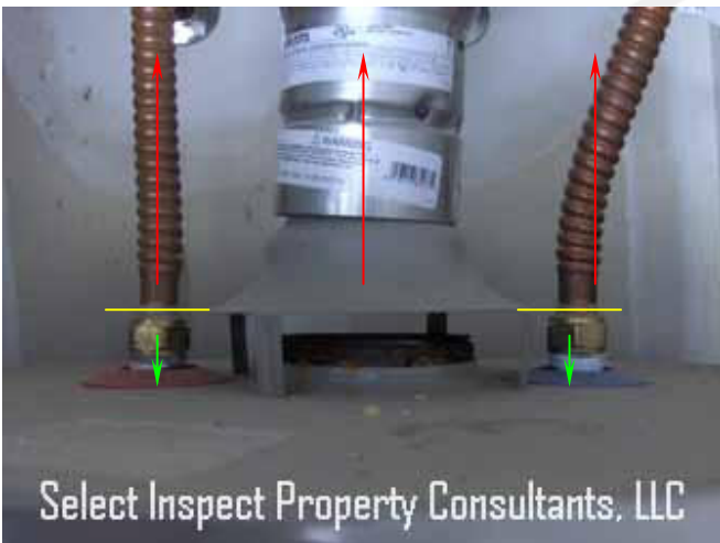
↑ electrical bond was not continuous above plastic compression fittings or at flue; water heater
