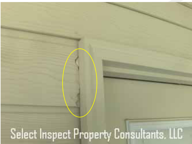
↑ damaged siding at rear porch door area
