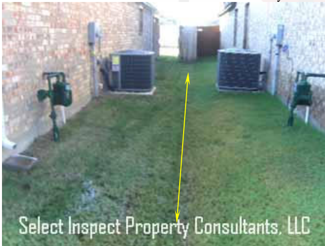
↑ pooling water at west swale; Monitor; should drain within 48 hours of rain
