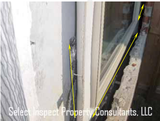
↑ deficient window tape seal needs replacement
