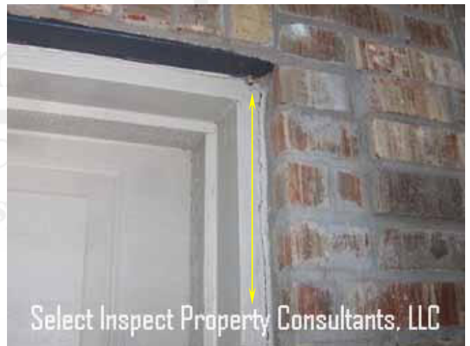
↑ garage overhead door frame separation at right
