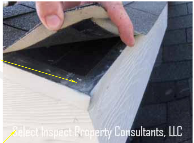
↑ unworkmanlike drip edge flashing at front gable
