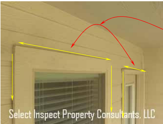
↑ missing z-flashing; example locations & unsealed trim/siding joints
