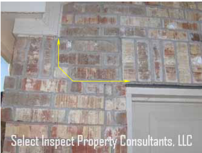
↑ mortar cracks at garage left
