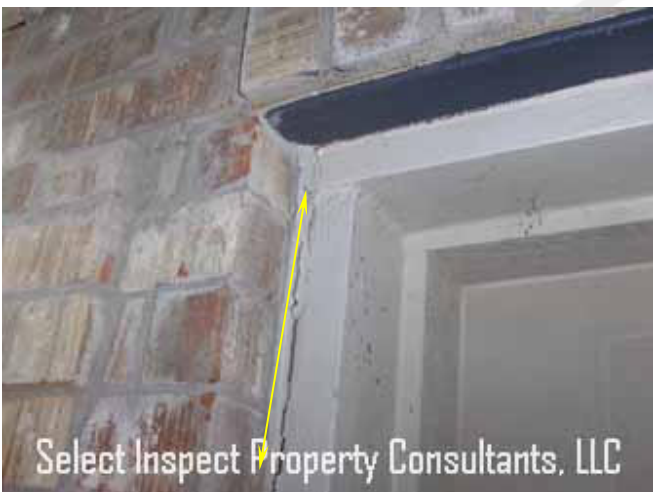
↑ garage overhead door frame separation at left
