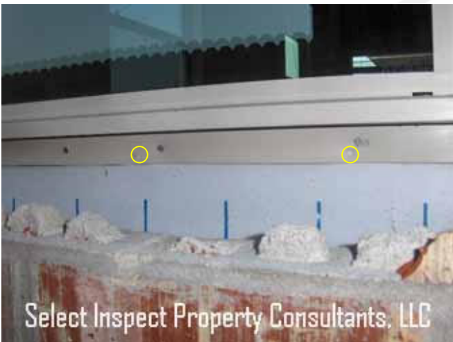
↑ unworkmanlike nailing of windows; example; suspected most/all other windows also incorrect.
