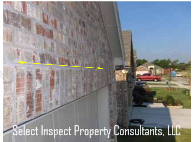
↑ sag/mortar cracks at garage overhead door
