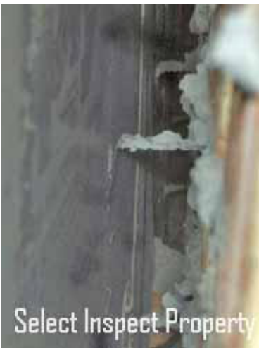
↑ debris in wall void
