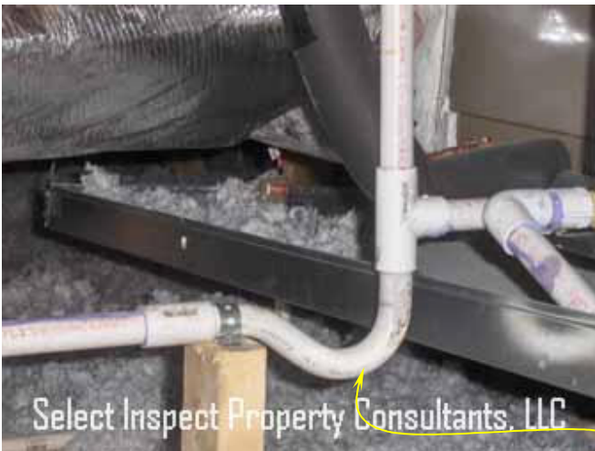
↑ debris in air conditioning auxiliary pan & non-insulated primary condensate drain
