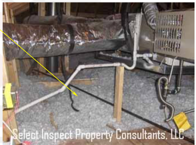
↑ 30" unobstructed service area was amiss at the HVAC
