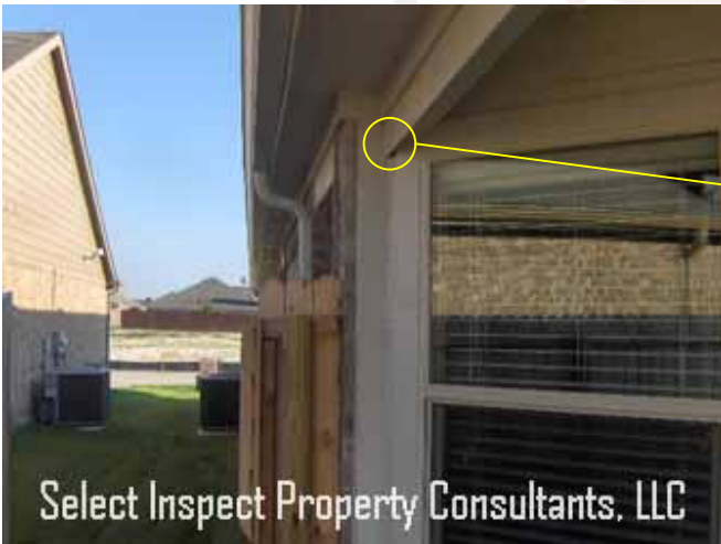
↑ opening exists at rear porch
