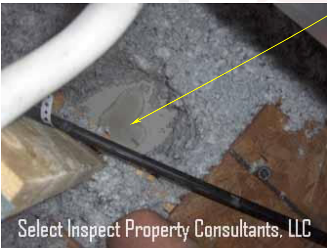
↑ active condensate dripping & moisture damage at ceiling drywall below the primary condensate drain trap
