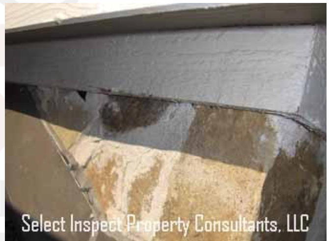
↑ openings & mortar cracks; front porch under left eave
