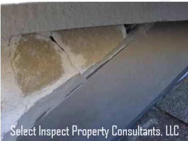
↑ openings & mortar cracks; front porch under right eave
