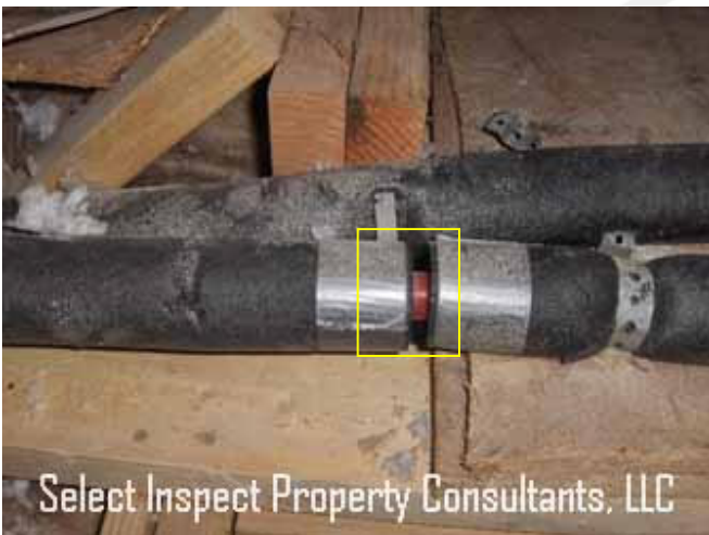
↑ inadequate insulation at hot water piping, adjacent the attic access
