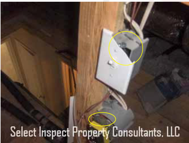
↑ damaged switch cover & excess reveal at junction box; attic
