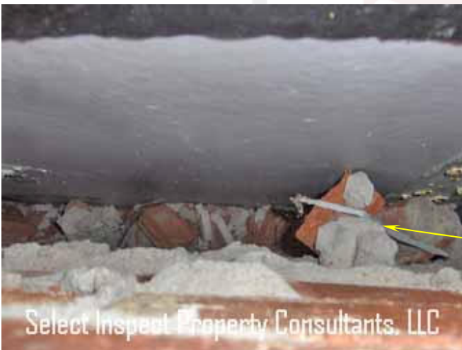
↑ debris in wall void
