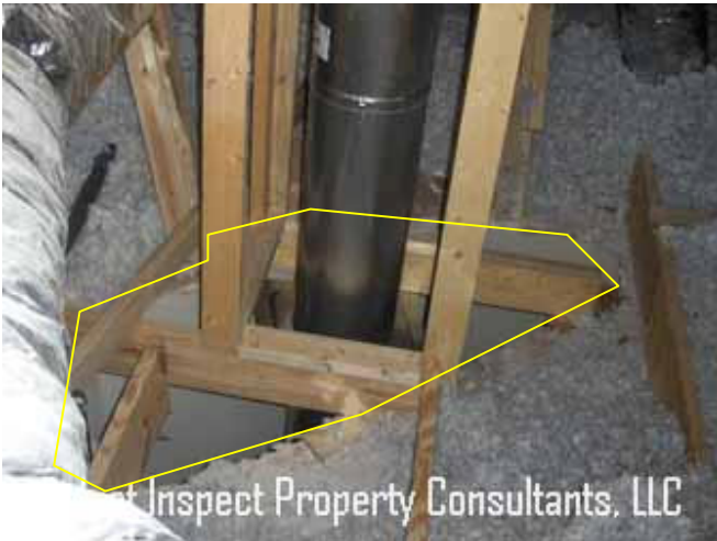
↑ fire-blocking was amiss/deficient at the fireplace flue/chase
