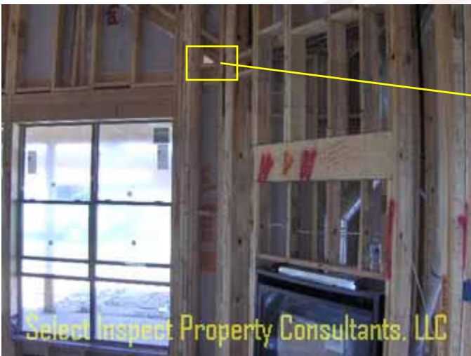
↑ sealant needed; example; at family room
