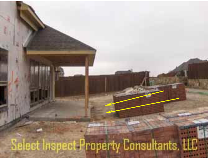
↑ inadequate / negative drainage at west; consider area drains
