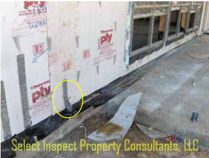
↑ unworkmanlike hold-down strap modification; west
