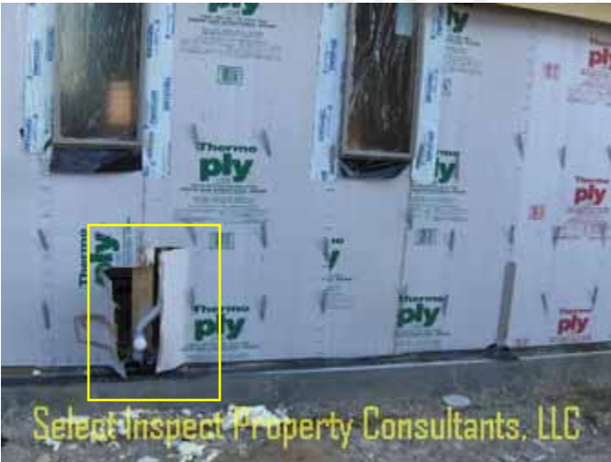
↑ tape flash & sealant improvement recommended
