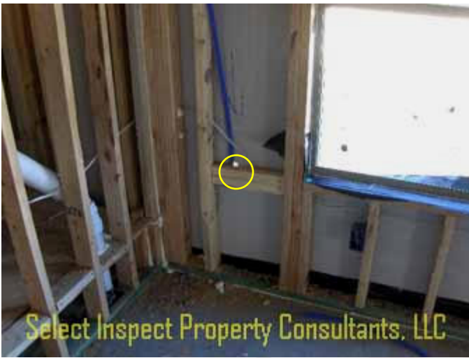
↑ sealant needed; example; at master bedroom southwest
