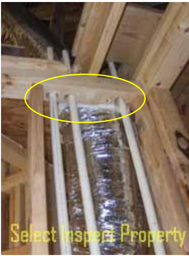
↑ sealant needed; example; northeast closet/chase
