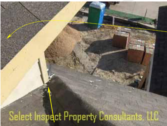
↑ debris should be cleaned from roof; example at front converging valley
