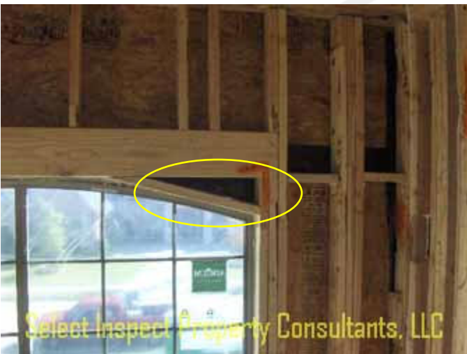
↑ sealant needed; example; east
