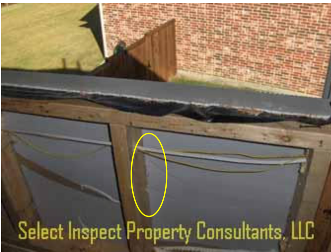
↑ sealant needed; example; north bedroom
