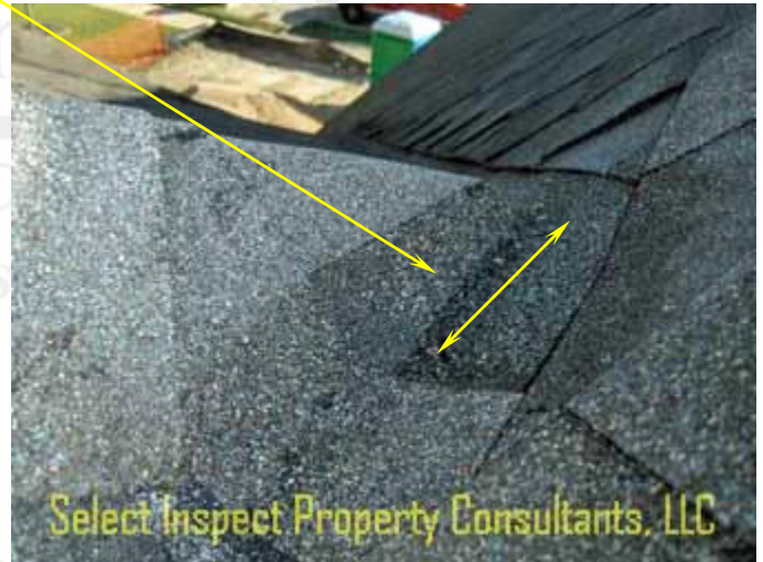
↑ moisture remains at this flat/negative section
