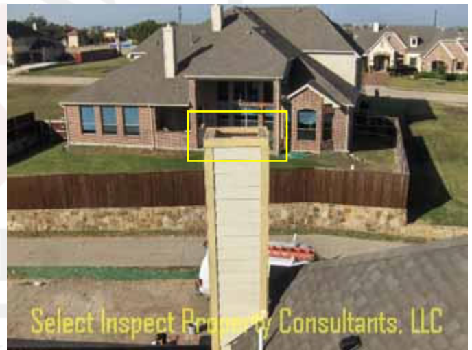
↑ chimney cap not present during the inspection
