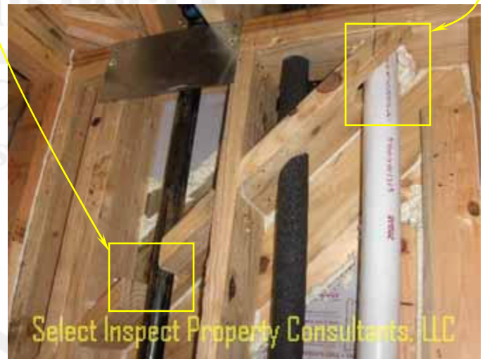
↑ Thursday ; sealant needed; & excess notching; west bathroom; related image below ↓
