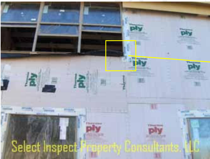
↑ tape flash & sealant improvement recommended
