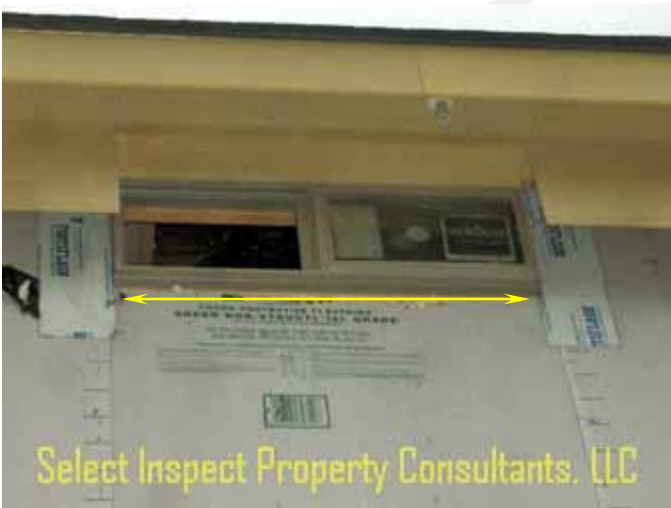
↑ window moisture barrier/flashing missing at the upstairs bathroom north window; window would need to be removed to install properly; or check with manufacturer for approved alternatives
