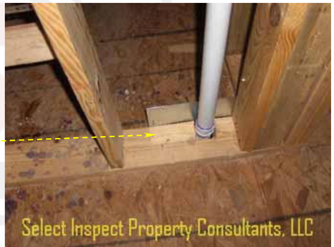
↑ sealant still needed; pipe & steel plate had been added as of Friday morning
