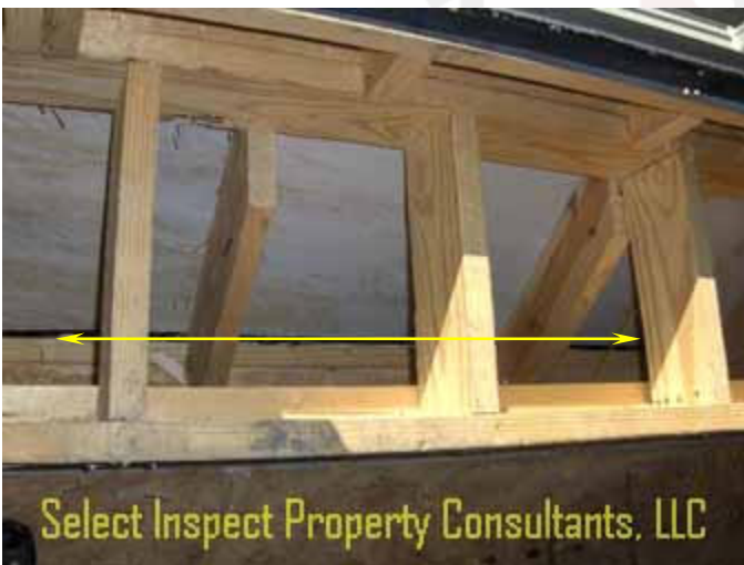
↑ sealant needed; example; at south bedroom bench
