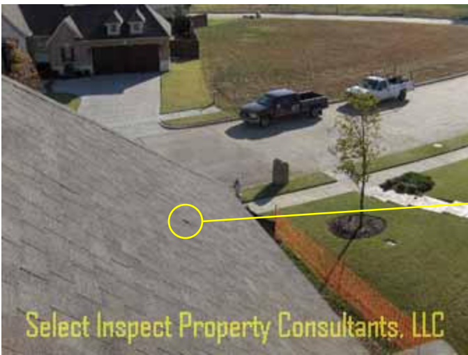
↑ undetermined damage at south-southeast roof
