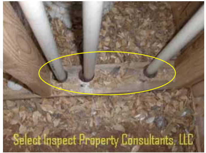
↑ sealant needed; example; bottom of pic at left
