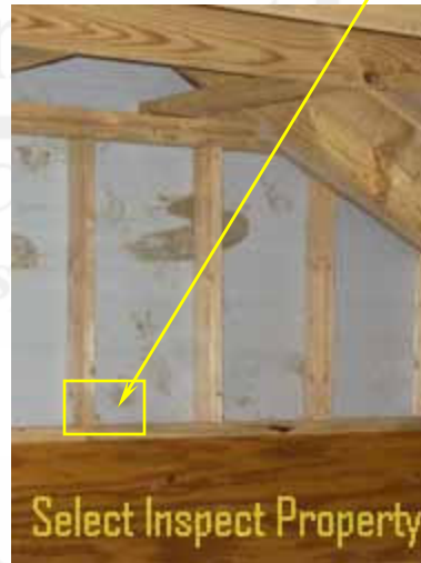
↑ close view of image above
