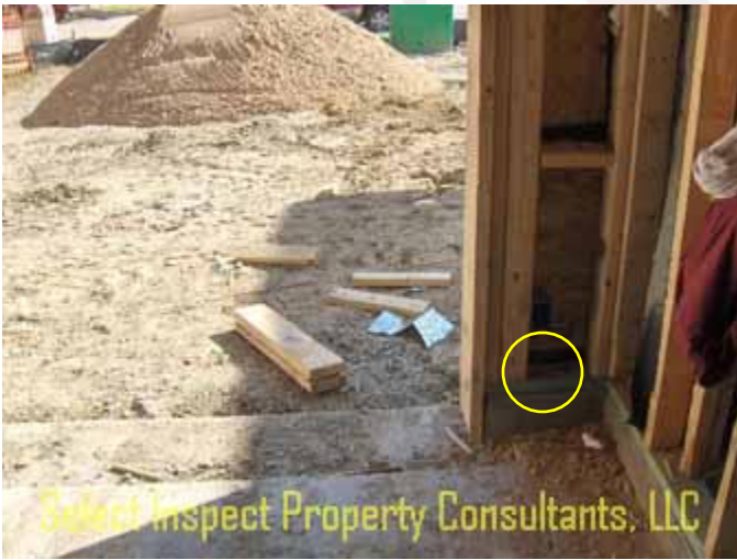
↑ missing anchor bolt nut single garage
