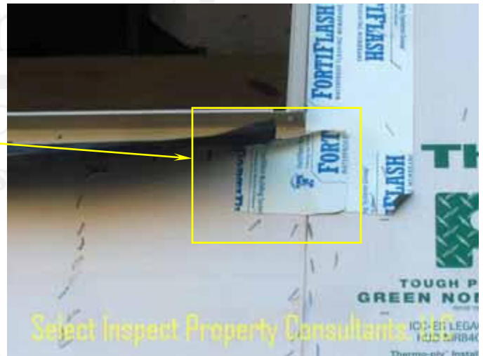
↑ tape flash is below, rather than above the moisture barrier flashing
