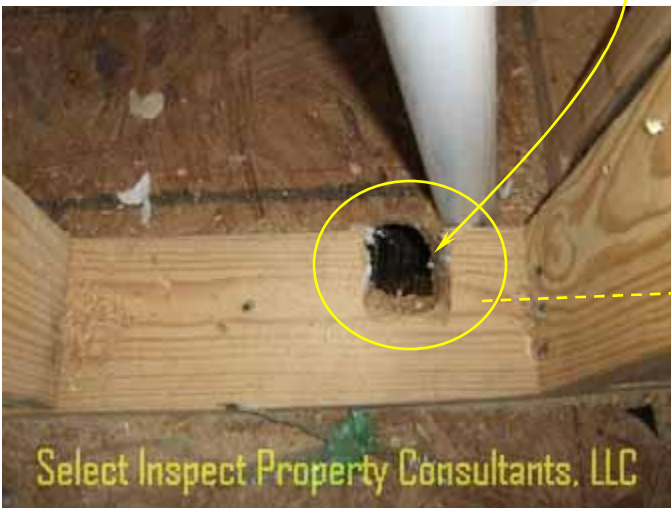
↑ sealant & bracing needed; close view of image above; Thursday
