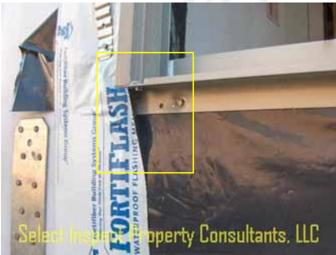
↑ tape flash & sealant improvement recommended; & example unworkmanlike window nailing
