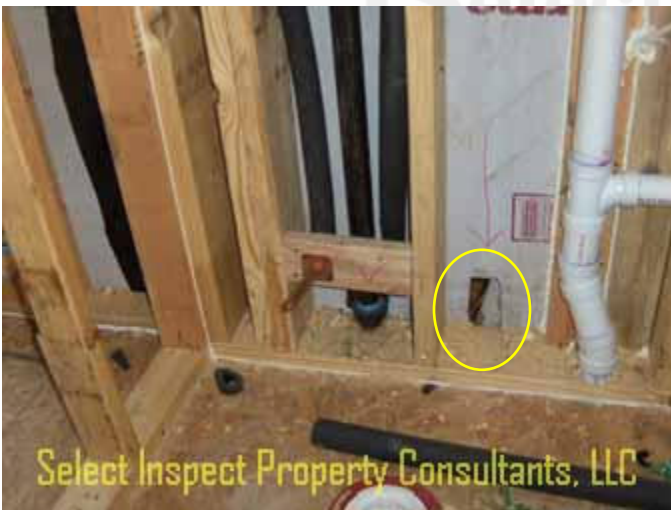
↑ sealant needed; example; at east bathroom
