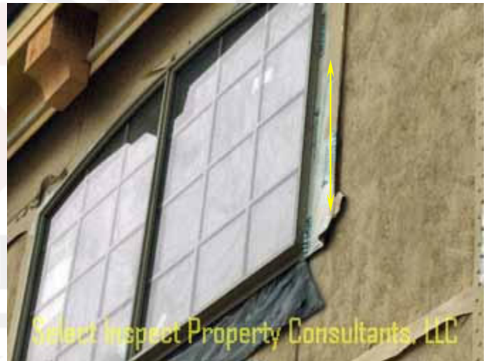
↑ tape flash & sealant improvement recommended; east-northeast bedroom upstairs (over single garage); poor adhesion
