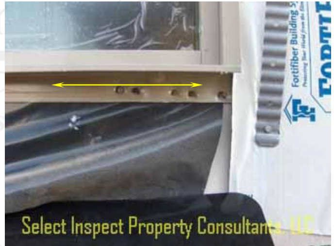
↑ unworkmanlike nailing of windows; example
