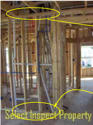
↑ sealant needed; example; north bathroom
