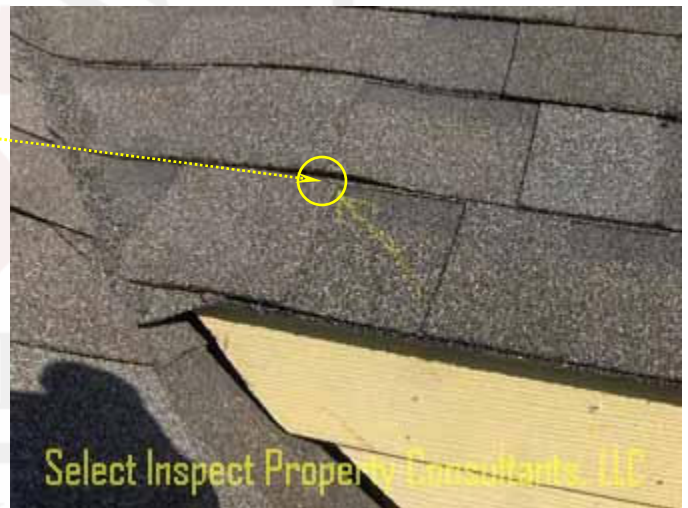
↑ uncaulked, exposed fasteners upper front
