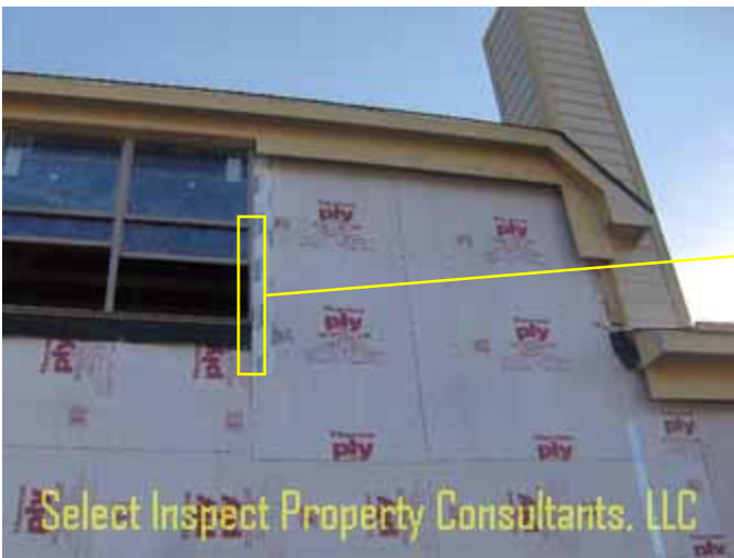
↑ tape flash & sealant improvement recommended
