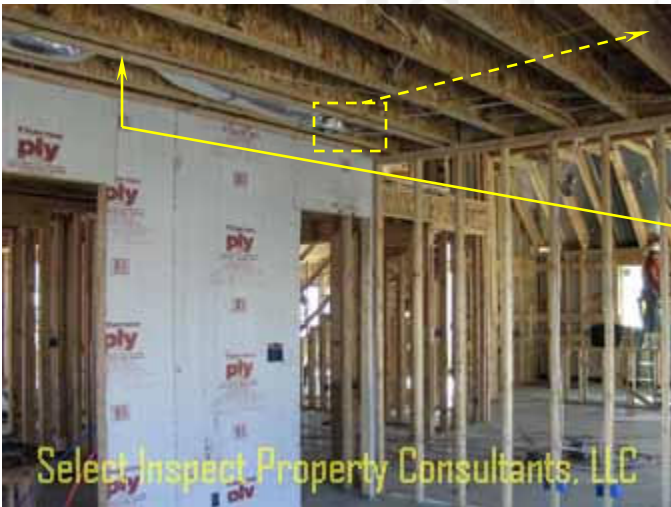
↑ crimped air ducting & less than ideal air register location; master bedroom
