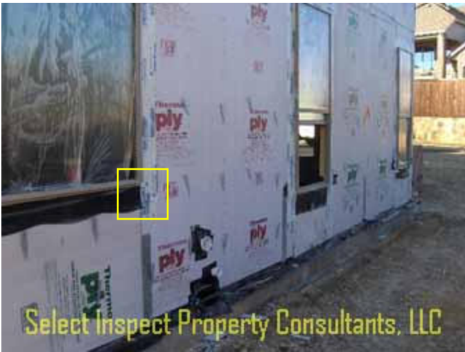
↑ tape flash & sealant improvement recommended
