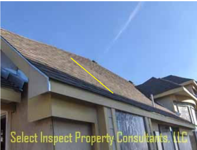
↑ slight sag noted at breakfast nook roof; issues not discovered at interior/framing
