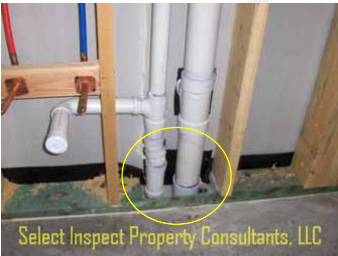
↑ sealant needed; example; at master bathroom
