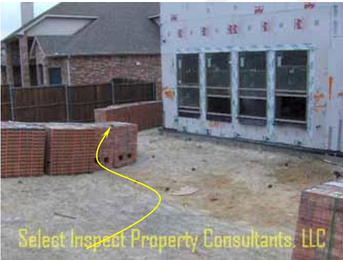
↑ swale at northwest appeared adequate
