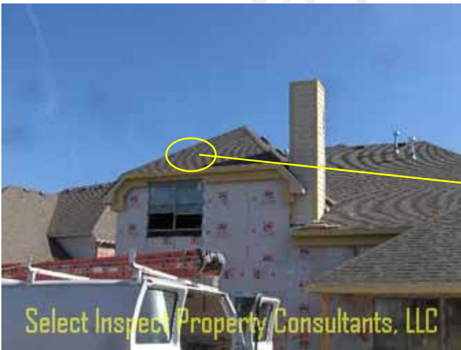
↑ undetermined debris upper west-northwest
