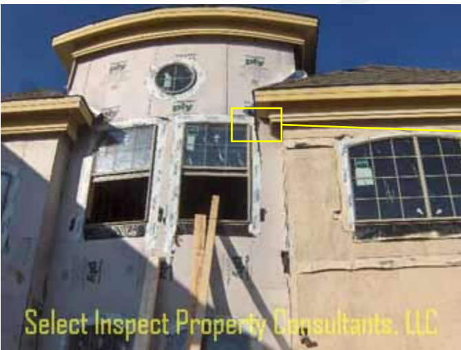
↑ tape flash & sealant improvement recommended
