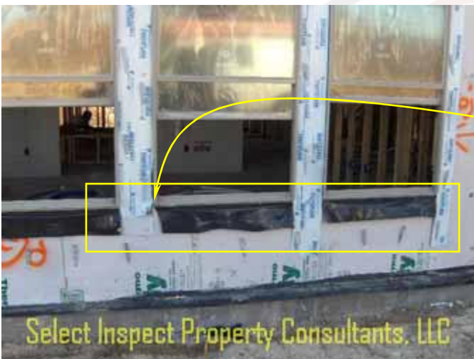
↑ tape flash & sealant improvement recommended
