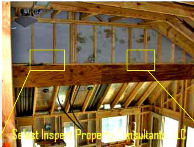
↑ sealant needed; example; at family room
