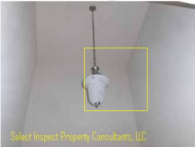
↑ Thermal imaging implies energy loss at foyer; closet window adjacent this at the upstairs
