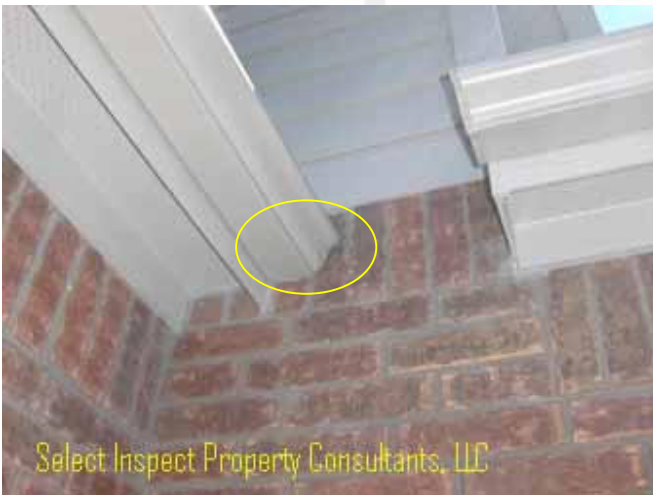
↑ bent gutter end prone to cap leakage; west near the air conditioning condenser(s)
