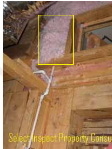
↑ there should be a minimum 24" pathway to the HVAC from the top of the access, with no gaps or obstructions
