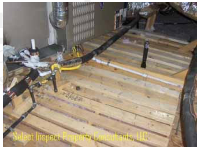
↑ gaps at attic floor service area
