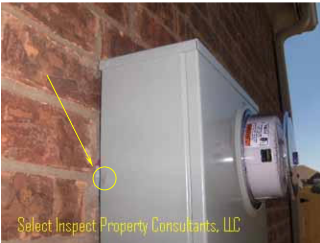
↑ dent & cracked paint; early rust starting; electrical meter; immediate corrective/improvement needs may be subjective.
