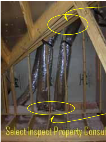
↑ crimped & inadequate support of air ducting; example at garage attic
