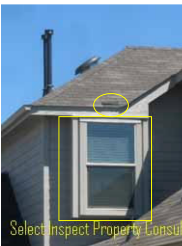
↑ damaged shingle tab & inverted trim
