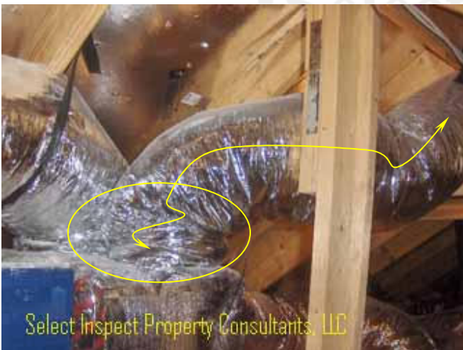
↑ crimped & inadequate support of air ducting; example
