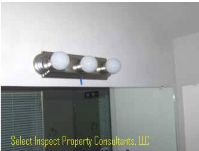
↑ uneven master bathroom lights –spacing over mirrors was inconsistent; east sink
