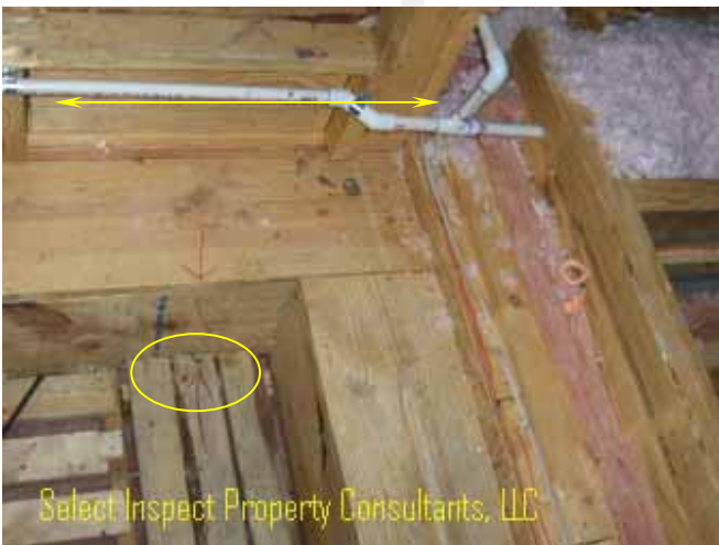
↑ protruding nails near attic access & primary condensate drain is prone to damage in this location
