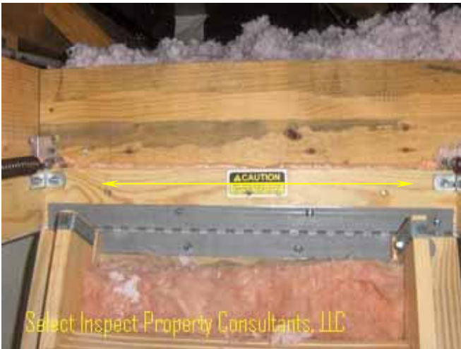
↑ deficient attic stair install; missing proper fasteners
