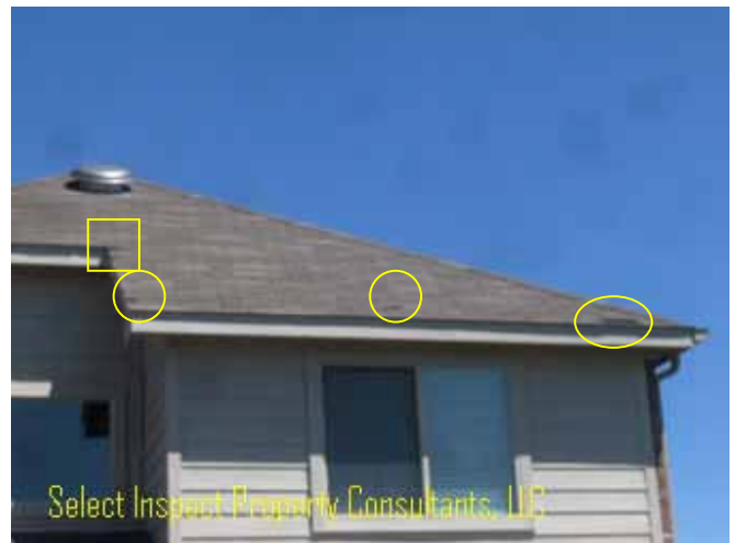
↑ damaged shingle tabs
