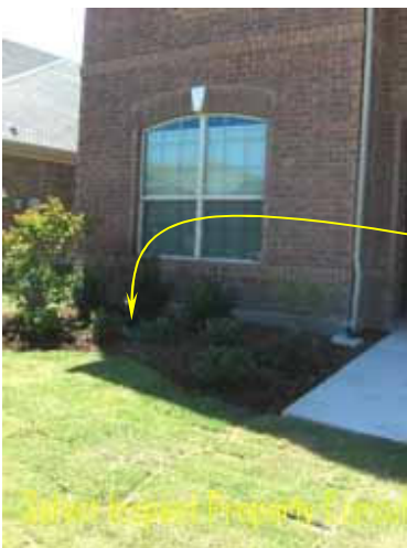
↑ water shut-off-valve location
