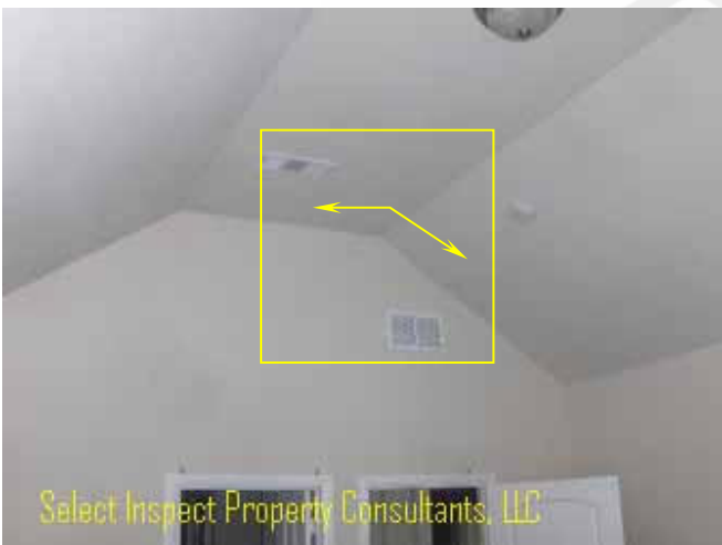
↑ Thermal imaging implies energy loss at master
