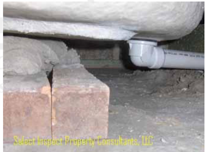
↑ inadequate support of master bathtub
