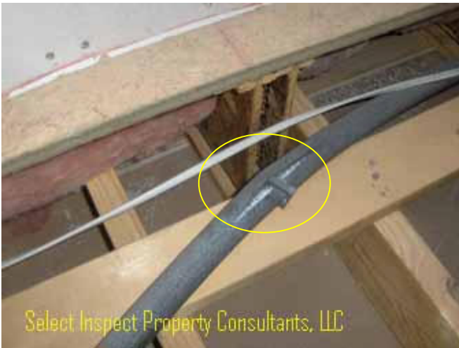
↑ unworkmanlike securing of plumbing pipe; insulation amiss; garage attic
