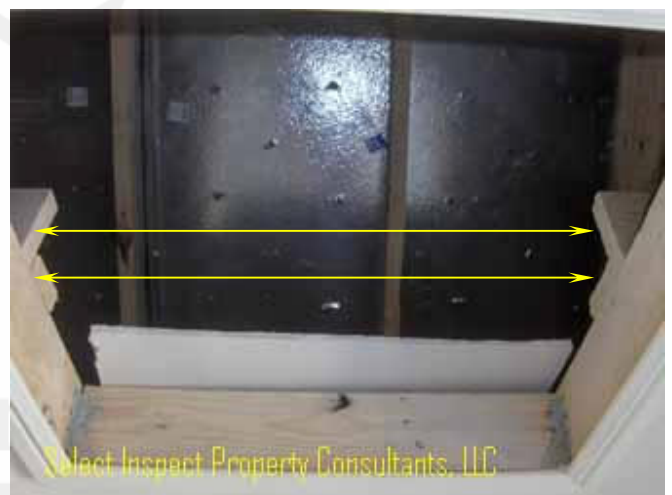
↑ lateral joist bracing cut at garage attic hatch
