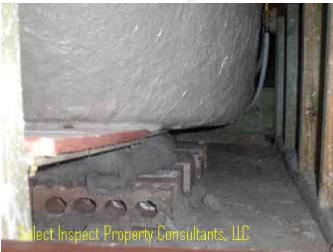
↑ inadequate support of master bathtub
