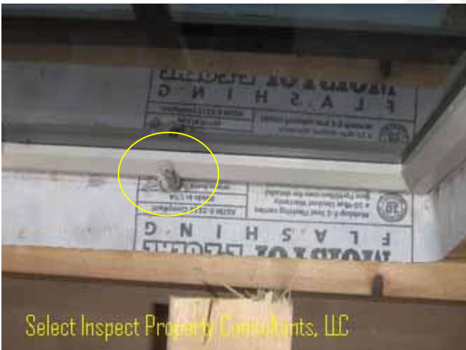
↑ drilled window & flashing; undetermined reason; garage attic
