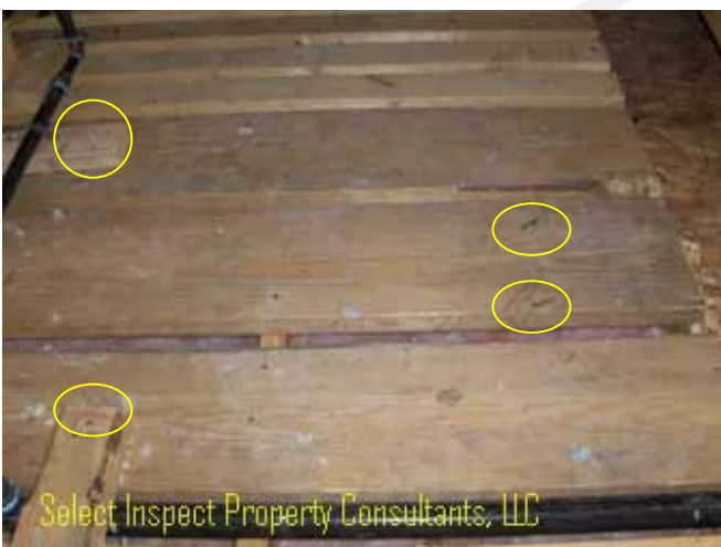
↑ protruding nails, may snag/cut service personnel
