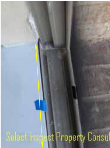
↑ 2 master bedroom window discovered as unsealed at the sills
