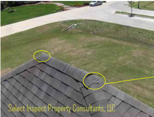
↑ unworkmanlike nailing; example
