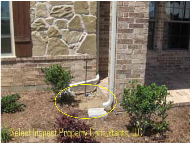
↑ erosion left of front porch & reversed splash blocks; rain not directed to terminate minimum 6 feet from structure
