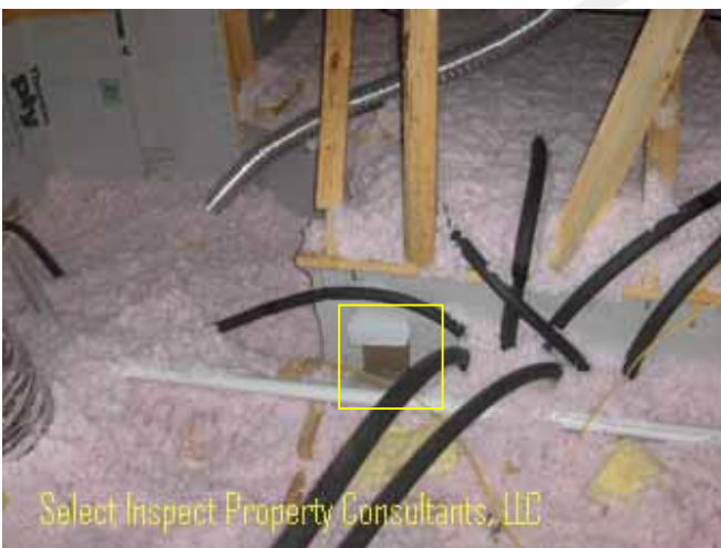
↑ missing insulation section adjacent the master bathroom-northeast
