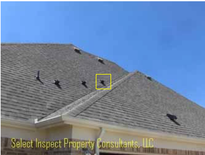
↑ vent/flashing closer than minimum 6" from valley; north
