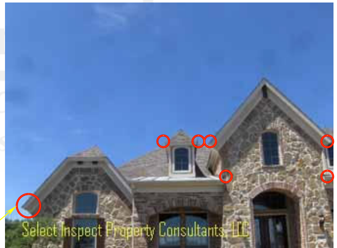
↑ example-unworkmanlike drip edge/felt; corners should have no gaps; rake (diagonal) edge & roof felt should be atop the eave (lower) edge flashing; roof underlayment should be under rake flashing
