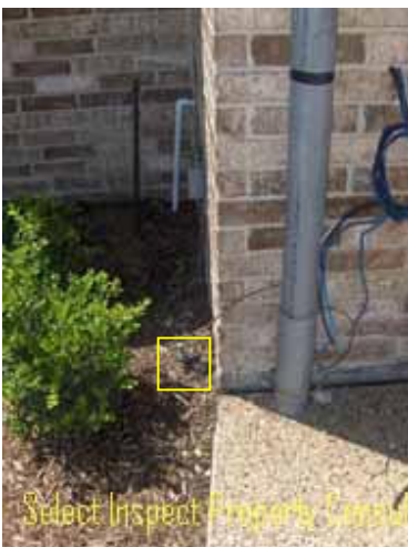
↑ grounding electrode protrudes grade; deficient
