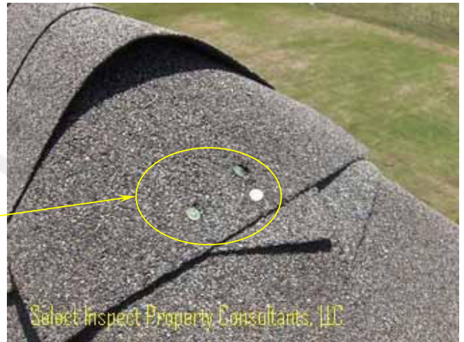
↑ askew/crooked, overdriven, & uncaulked, exposed fasteners
