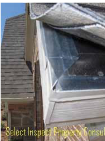
↑ unworkmanlike drip edge flashing & roof underlayment
