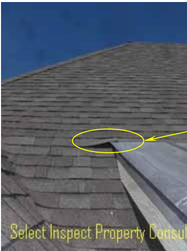
↑ inadequately sealed shingle lap
