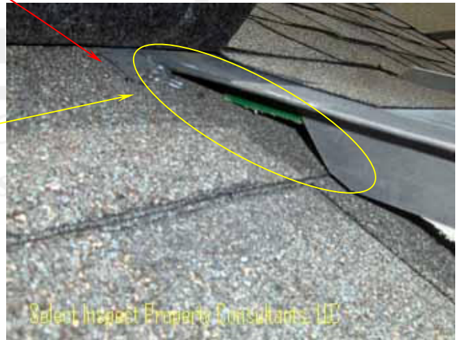
↑ short flashing; openings, visible roof deck; prone to moisture intrusion
