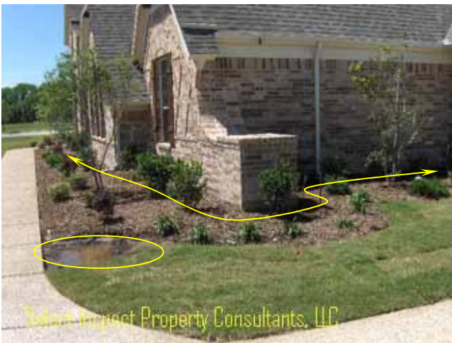
↑ pooling water & marginal grading
