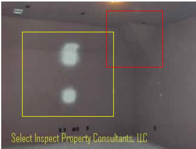
↑ Thermal imaging implies energy loss at the media room; *patches may have missing insulation behind, or may still be cooler from recent drywall work
