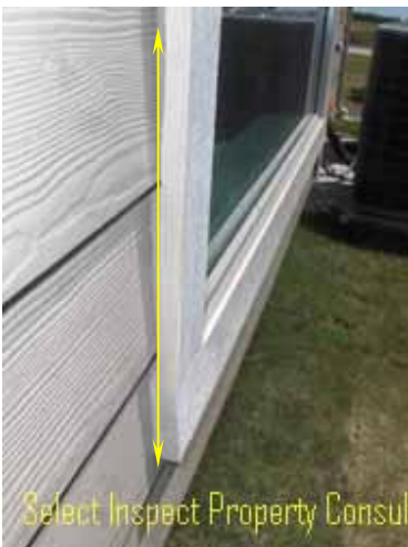
↑ close view of image above
