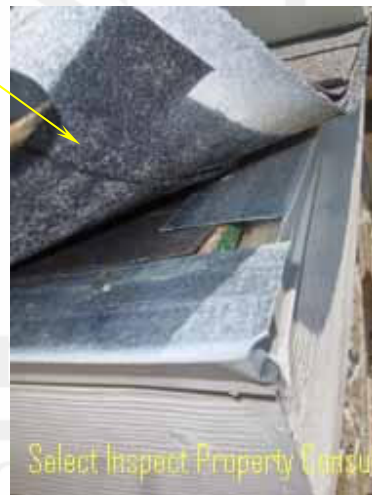
↑ close view of image above; example of multiple similar conditions discovered
