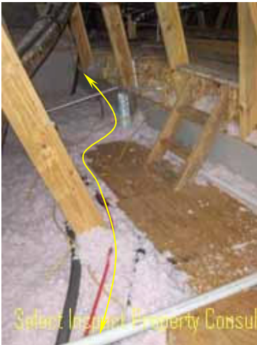
↑ non-insulated plumbing pipe (red implies hot water) near the attic access
