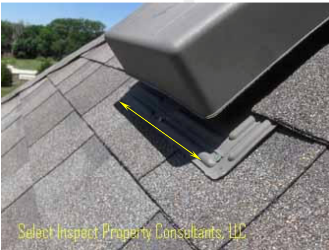
↑ example uncaulked, exposed fasteners at roof vent; center nail under driven
