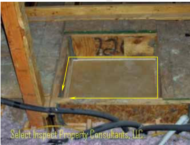
↑ inadequate seal at garage attic hatch
