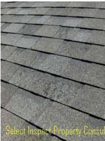
↑ worn shingles discovered at the west & south; example at the west
