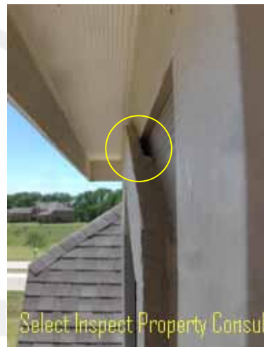
↑ openings discovered above dormer window trim
