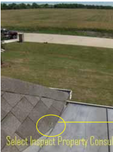
↑ overdriven nail & uncaulked, exposed fasteners, split shingle
