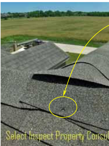
↑ example overdriven nails & uncaulked, exposed fasteners
