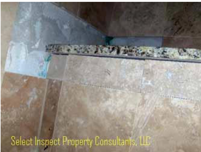
↑ openings, missing tile, damaged cement board joints, & missing grout at master shower; appears to be "in progress"
