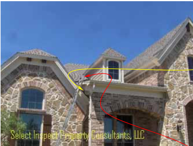
↑ unworkmanlike flashing & converging valley; very prone to moisture intrusion
