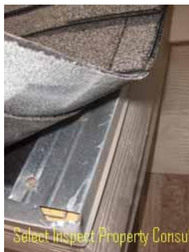
↑ unworkmanlike drip edge flashing & roof underlayment
