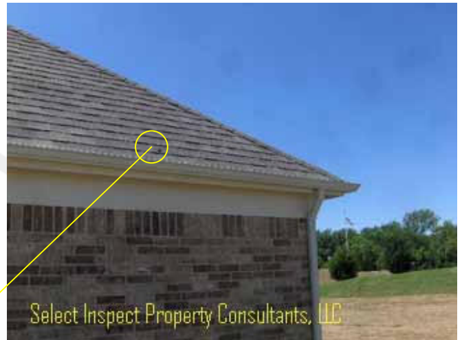
↑ example damaged shingle tab; northwest
