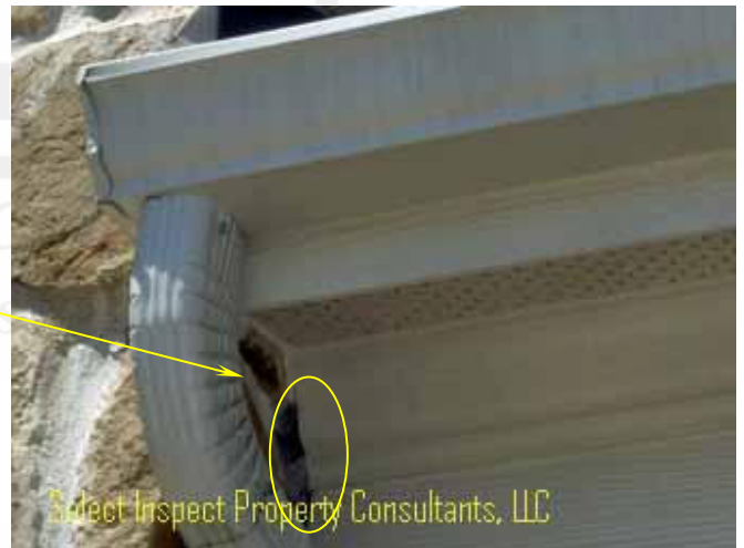
↑ close view of image at left; sealant needed
