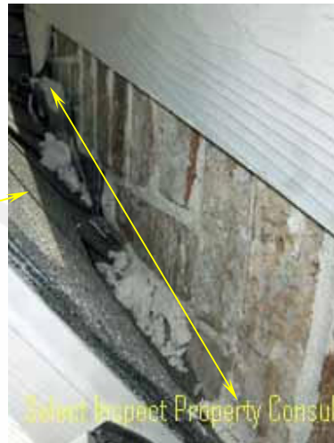
↑ close view of image at left; amiss flashing, debris; openings
