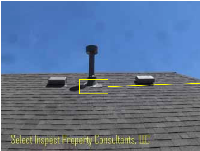
↑ lifted flashing at flue; west-southwest
