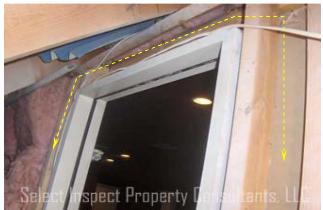
↑ deficient insulation confirmed at walk-in attic door perimeter
