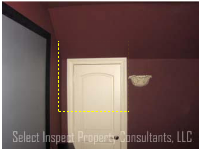
↑ Thermal imaging implies energy loss at media room walk-in attic
