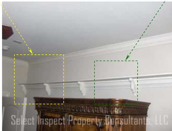
↑ Thermal imaging implies energy loss at the east bedroom
