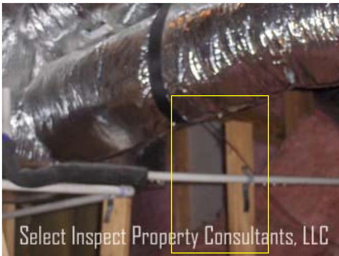
↑ missing insulation adjacent in the attic
