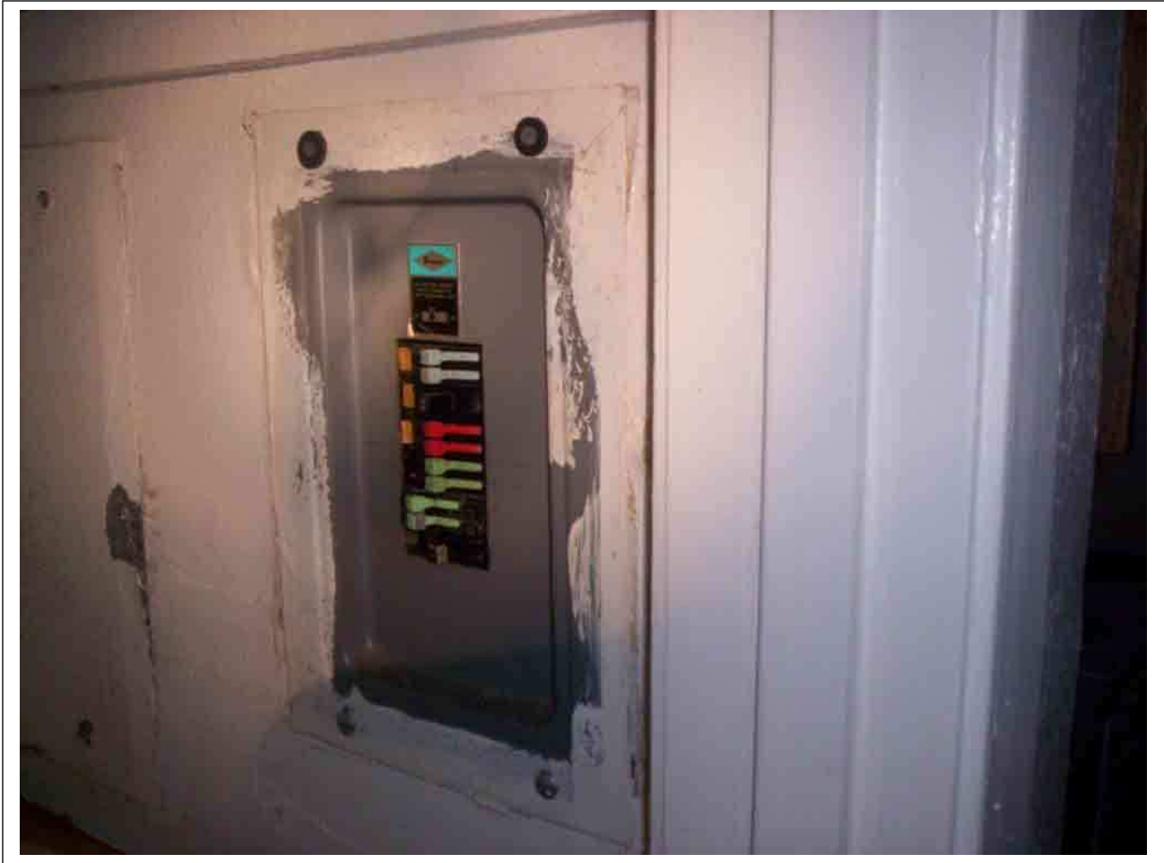
51. Comments: Typical interior electrical panel box
