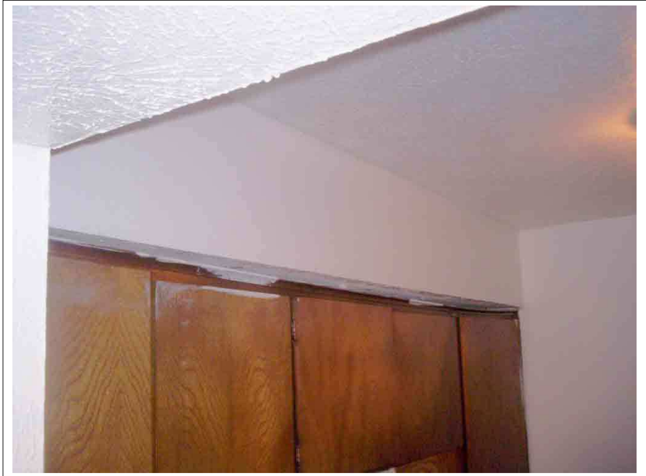
33. Comments: unit 120- marginally secured cabinetry
