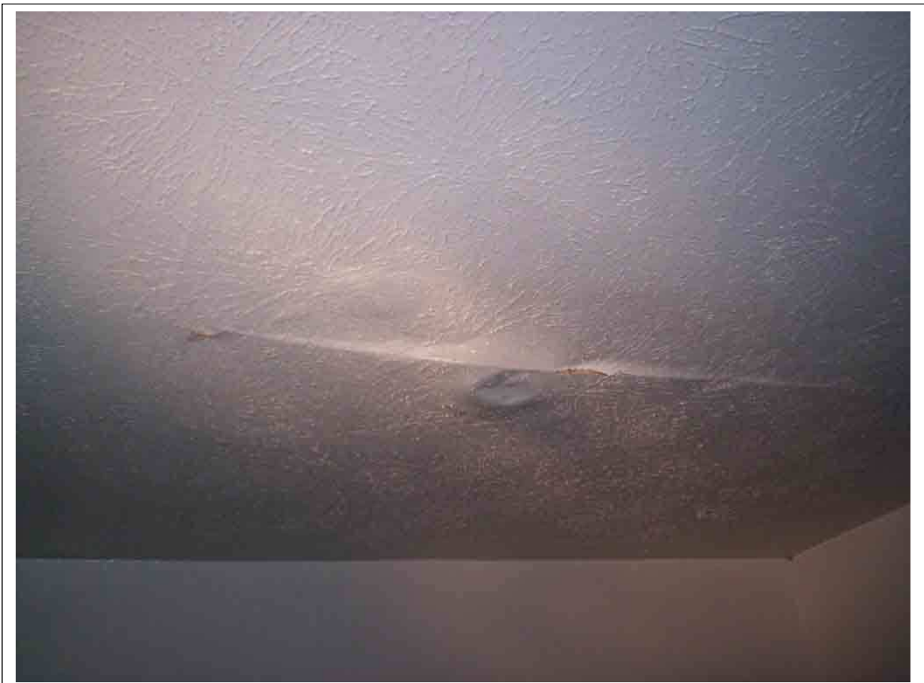
28. Comments: unit 224 – moisture intrusion evidence H&S
