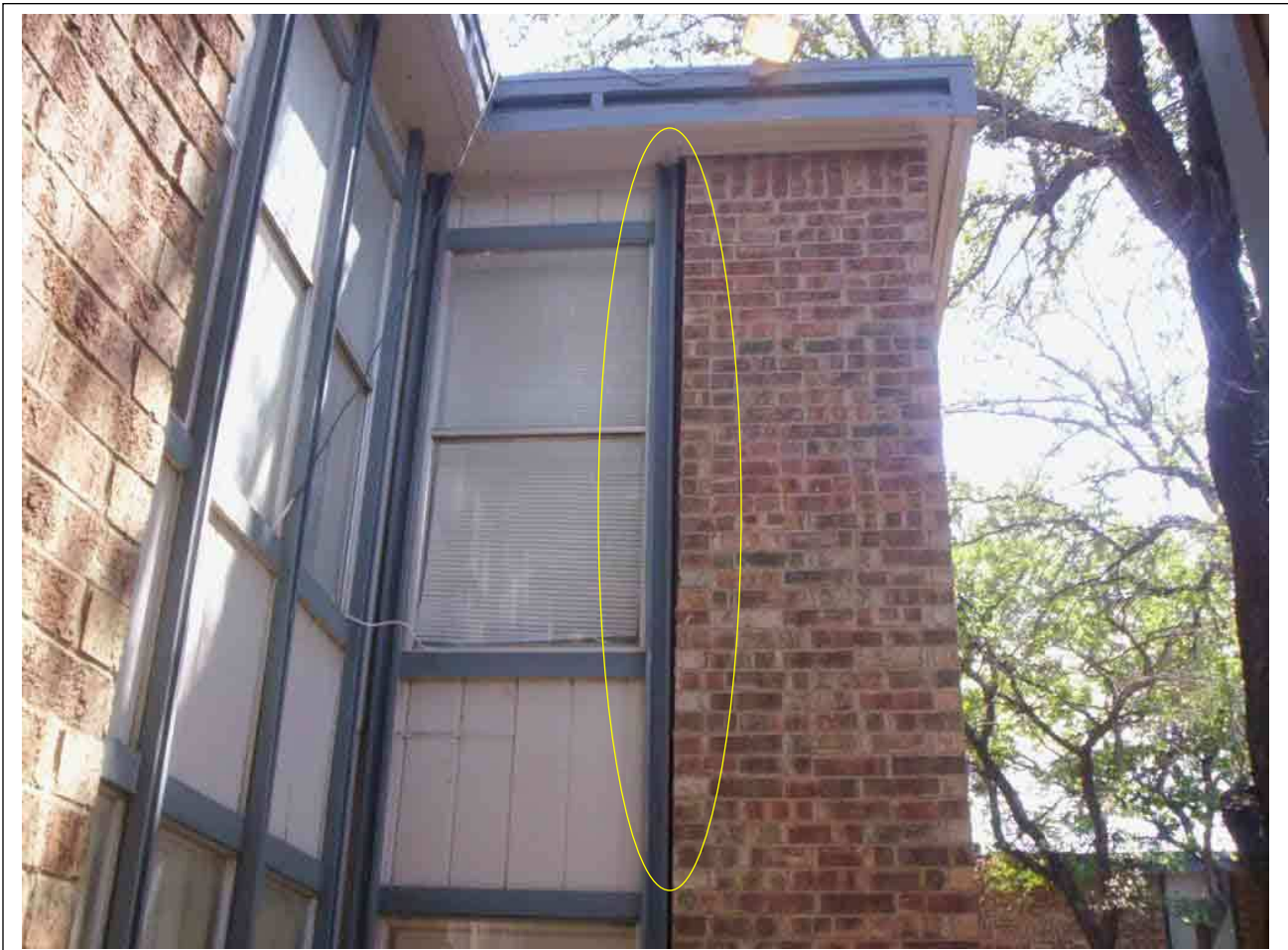
16. Comments: brick / framing separation example at Bldg 5
