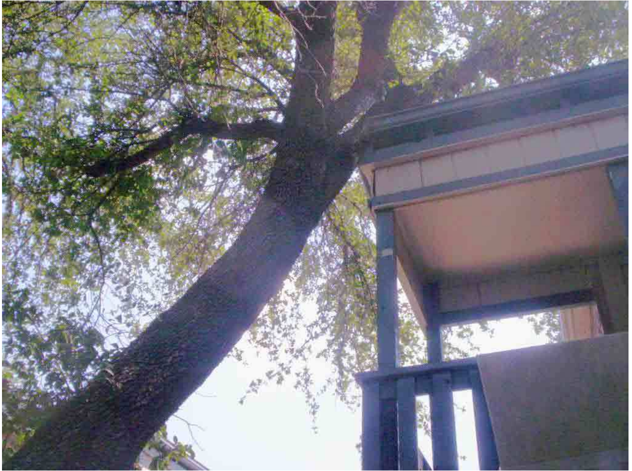
9. Comments: Bldg 2- tree impeding structure
