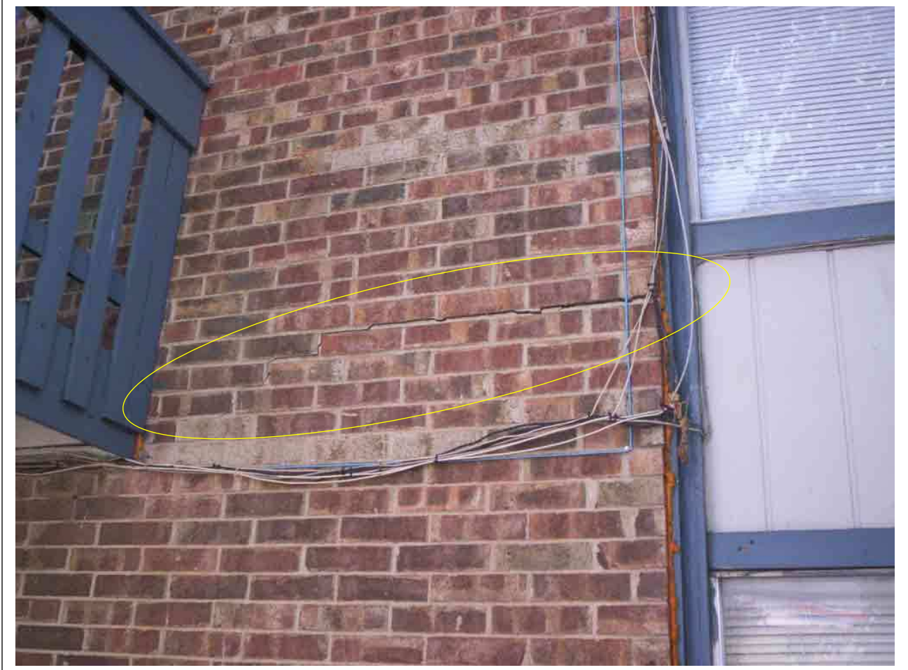
15. Comments: large (+- 3/8") brick / mortar crack at southern side of Bldg 5
