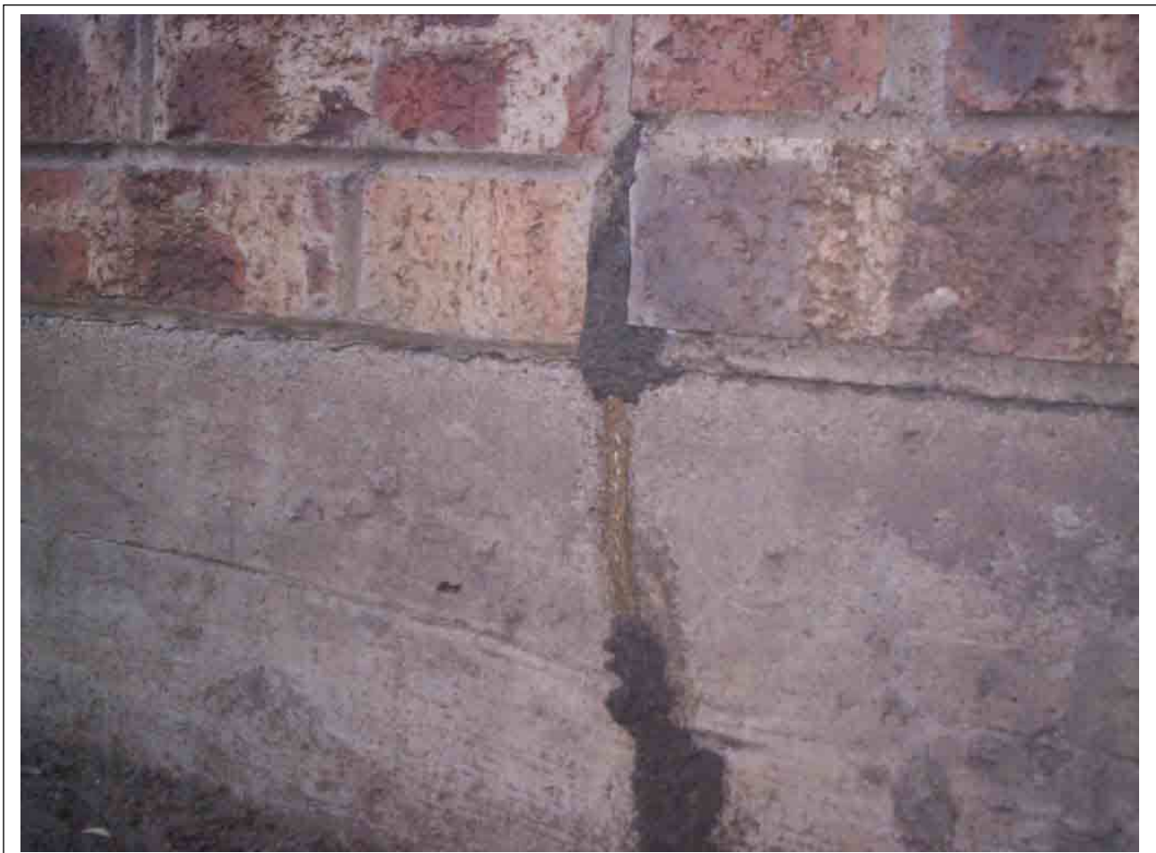
22. Comments: active termites- example Bldg 2
