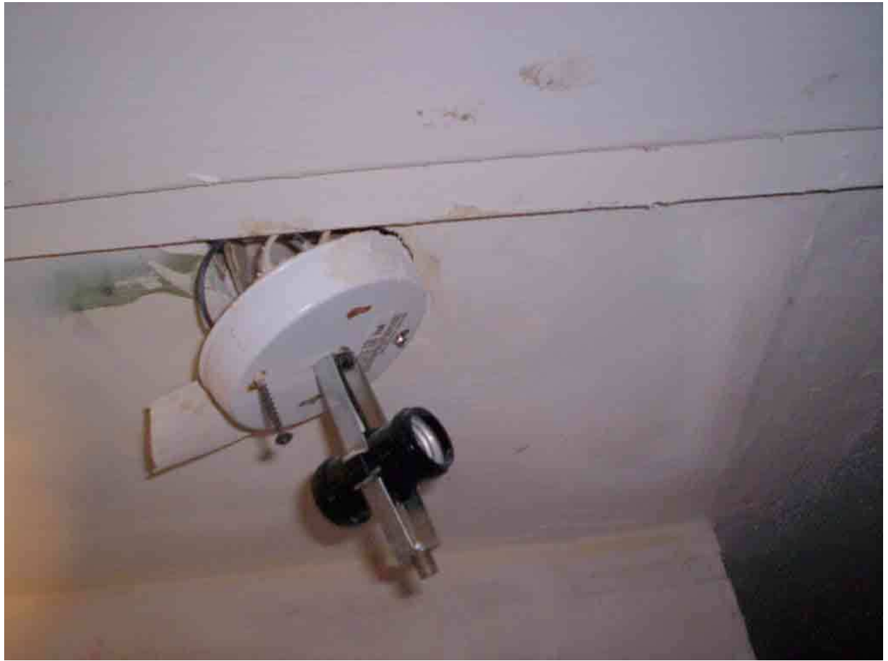
37. Comments: unit 135- amiss / deficient electrical fixture H&S
