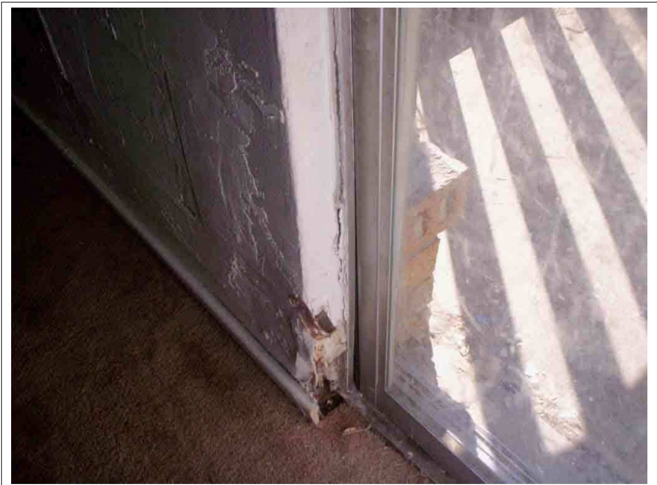
32. Comments: unit 119- rot/moisture damage at patio interior H&S
