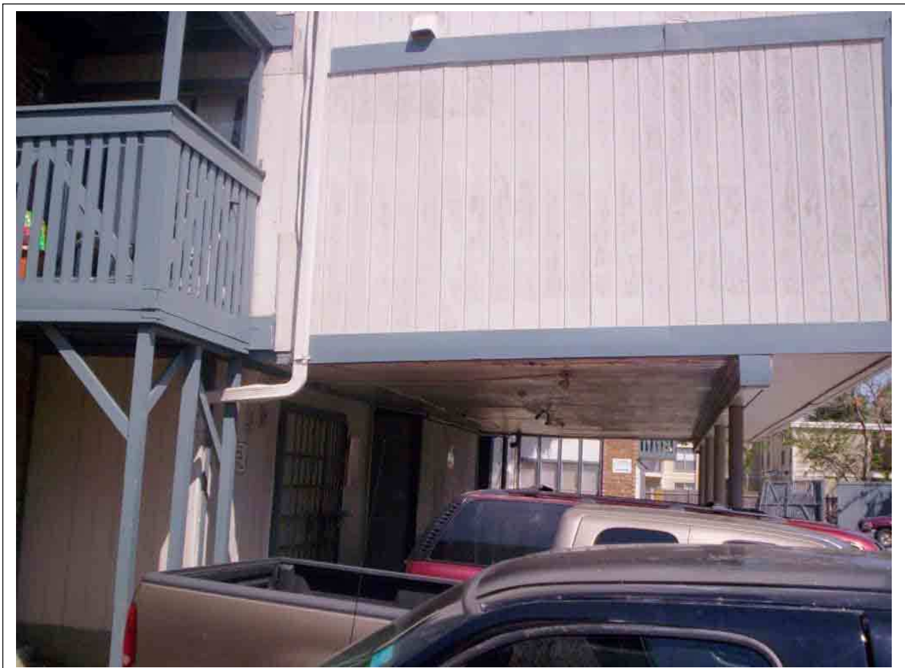
18. Comments: questionable integrity of cantilevered structure- north side of Bldg 2
