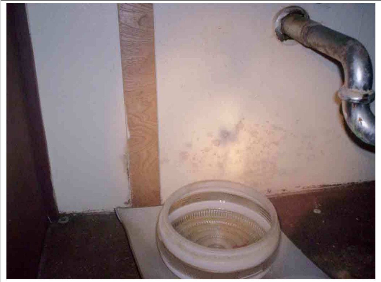
41. Comments: unit 221- moisture intrusion / fungus below bar sink H&S
