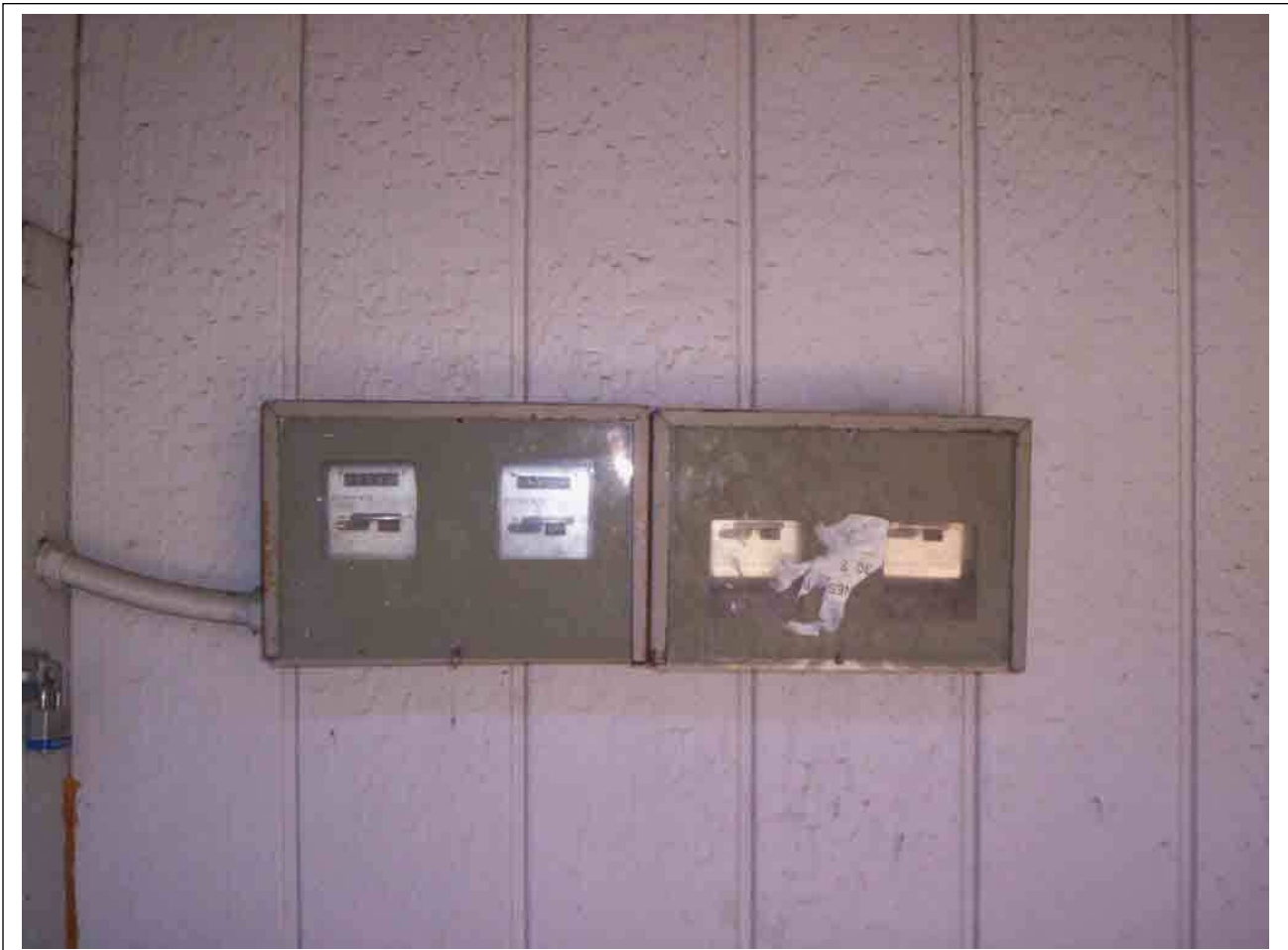
50. Comments: Typical electric meter- discovered services were 90 amp
