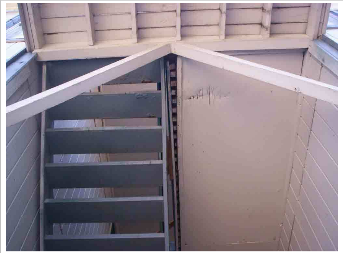
3. Comments: Bldg 2- decay at under stair components.
