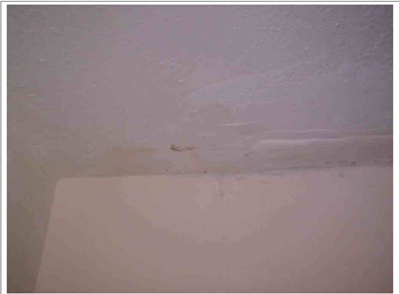
42. Comments: unit 225- moisture intrusion evidence H&S
