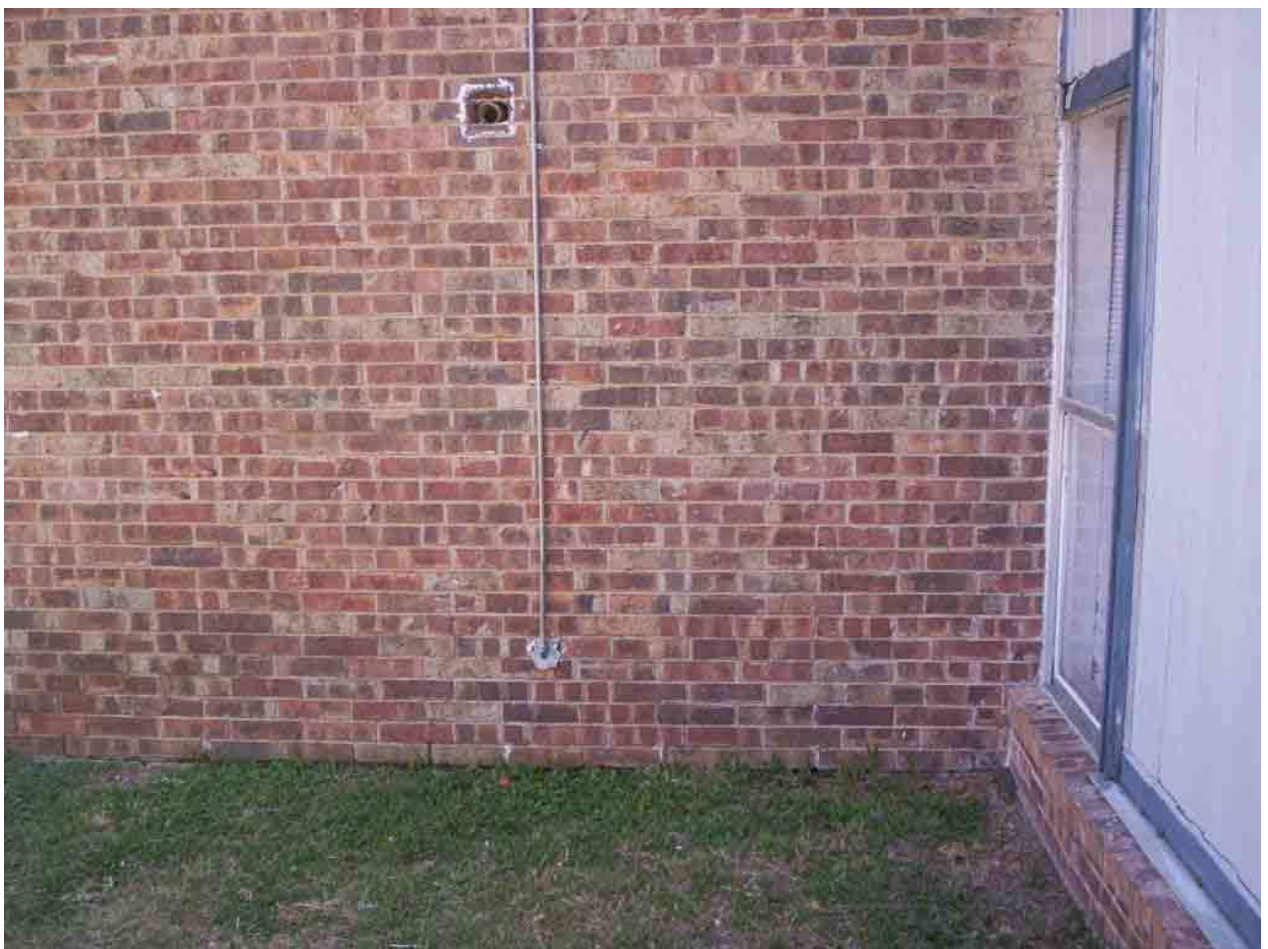
10. Comments: Bldg 2- moisture seepage from within- lower amiss vent cover- upper
