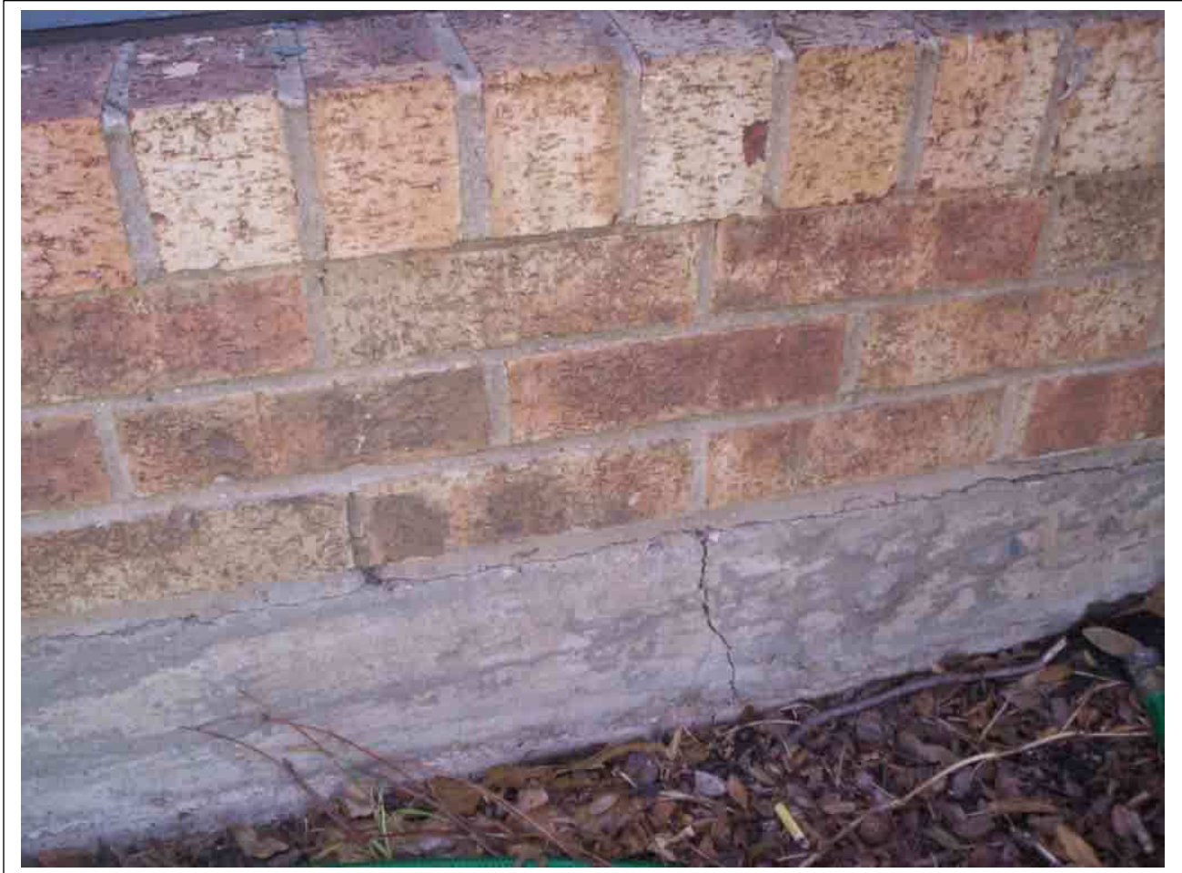
17. Comments: foundation slab crack- example
