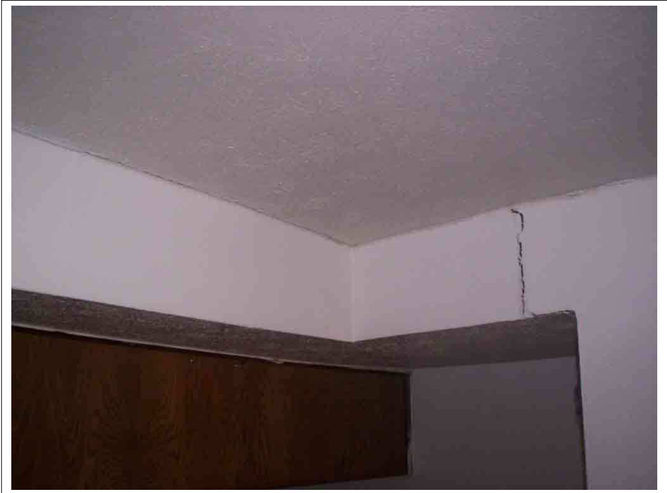
39. Comments: unit 204 foundation stress indication
