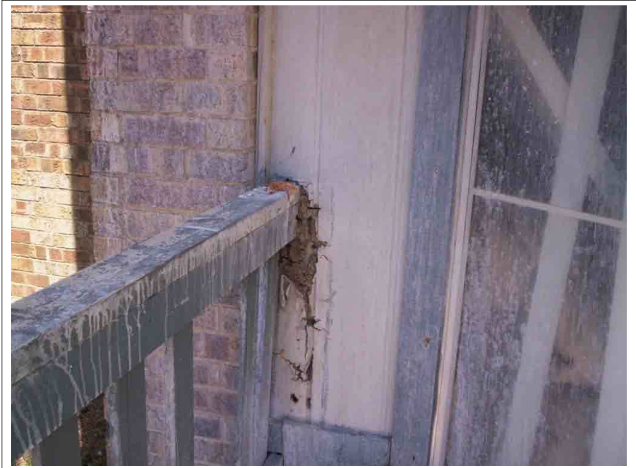
5. Comments: Bldg 3 -wood destroying insect and rot/moisture damage
