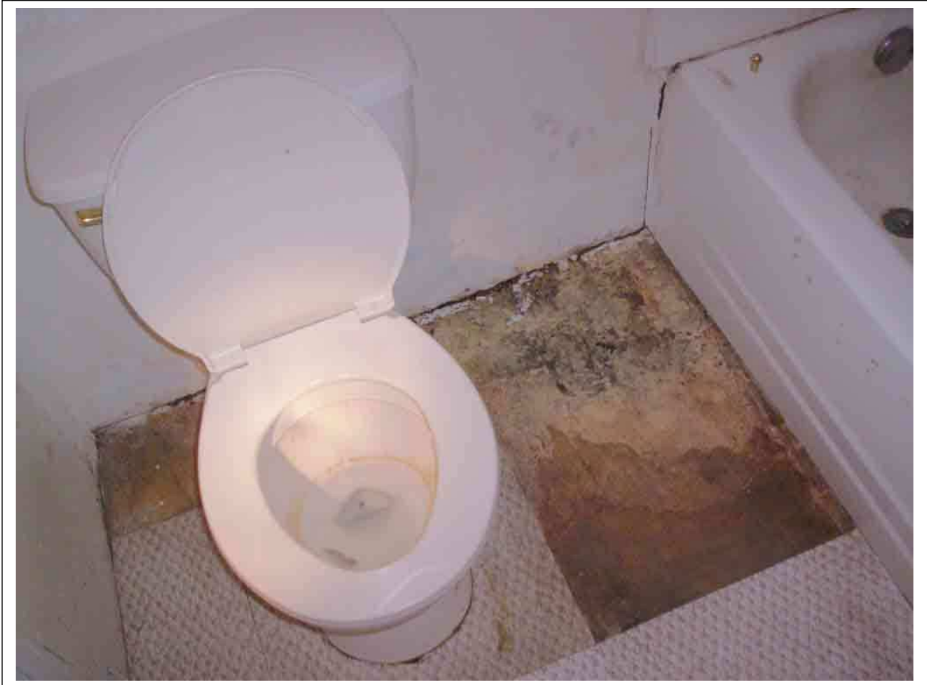
35. Comments: unit 135 leakage ongoing, moisture intrusion / fungus.
