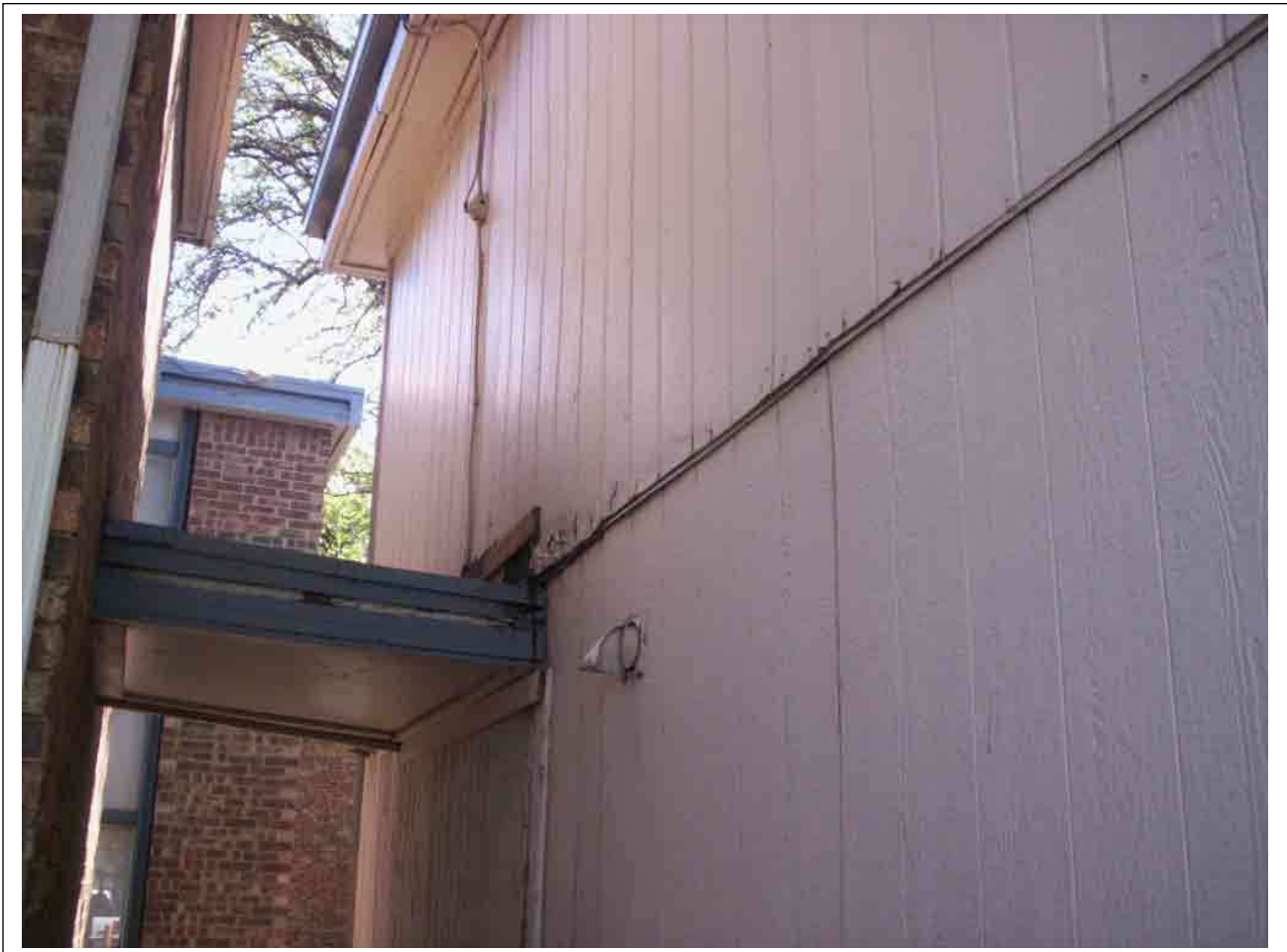
8. Comments: Bldg 6- rot/moisture damage at cladding
