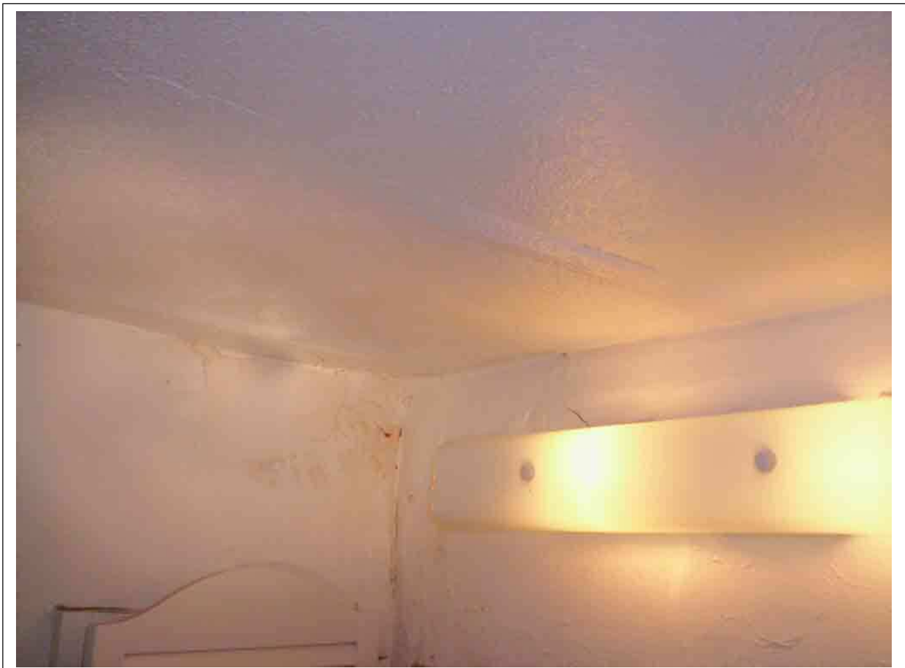
44. Comments: unit 233 – moisture intrusion evidence H&S
