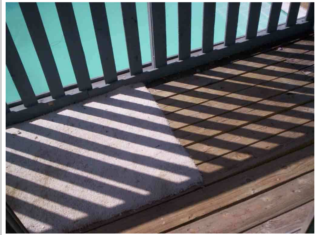
43. Comments: unit 232- unsteady balcony floor structure H&S
