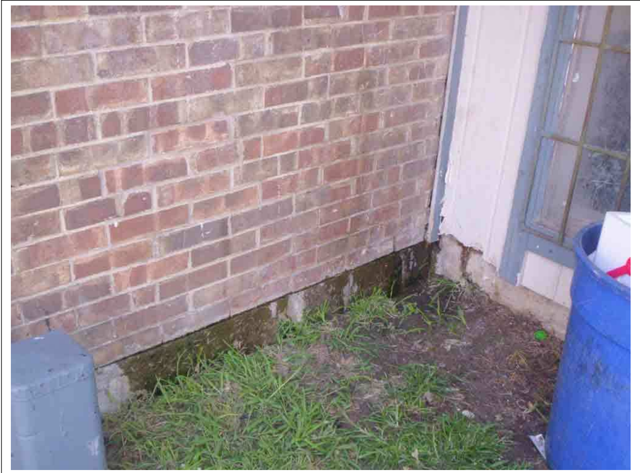
11. Comments: moisture seepage from within building- example 2
