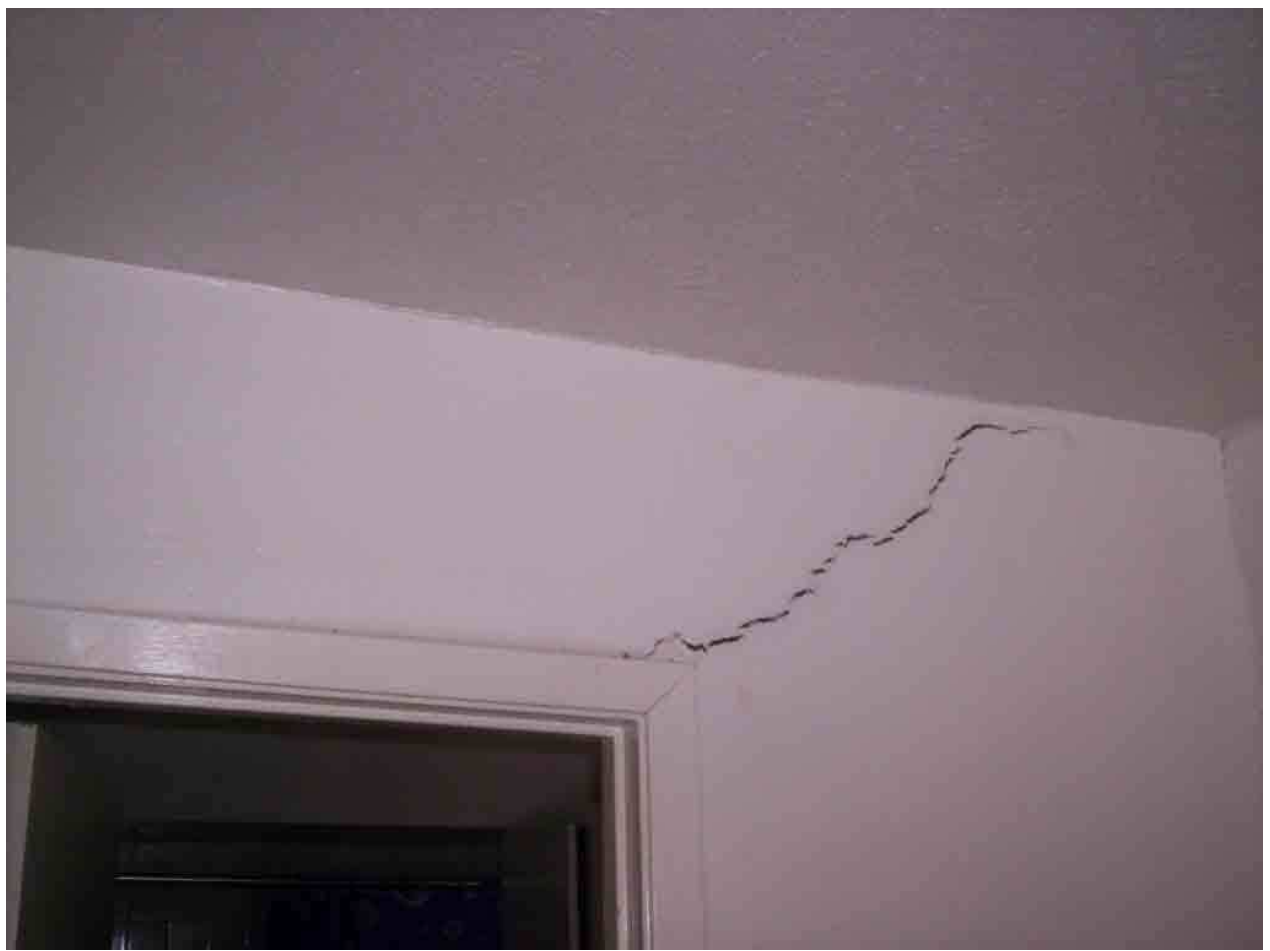
38. Comments: unit 204 – foundation stress indication
