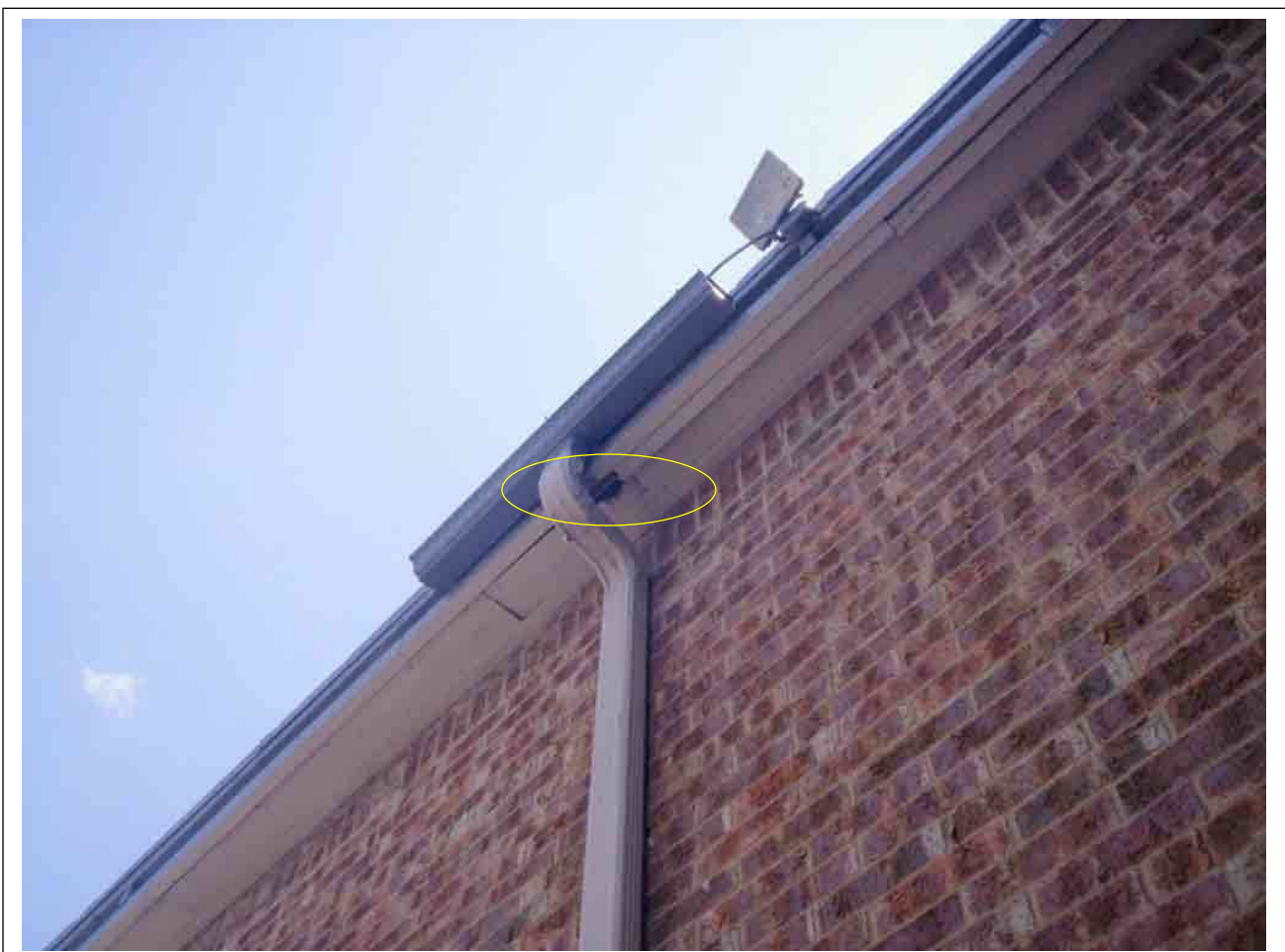
20. Comments: eave rot/moisture damage south Bldg 5. Suspect amiss gutter.
