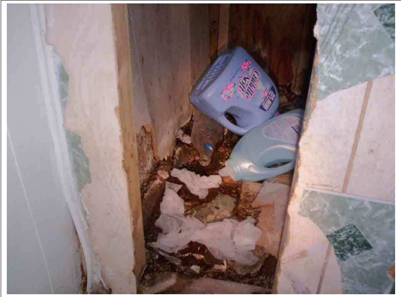
47. Comments: ongoing leakage, rot/moisture damage, fungus under shelf unit southwest corner of laundry room
