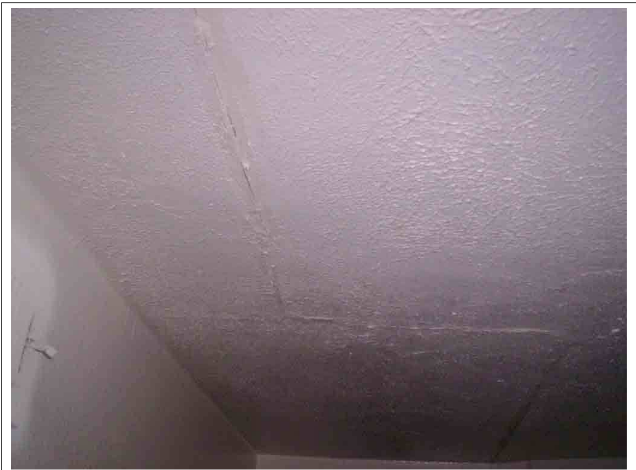
40. Comments: unit 216 foundation stress indication
