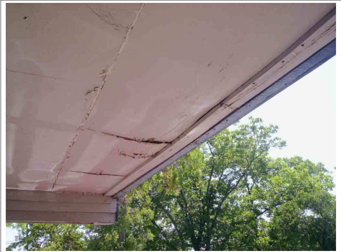
19. Comments: moisture leakage and rot/moisture damage at underside of cantilevered structure
