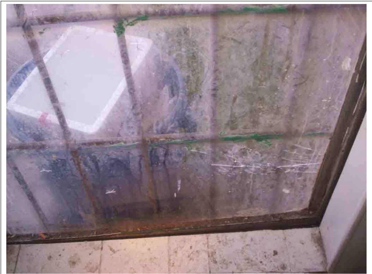
48. Comments: damaged window at laundry room
