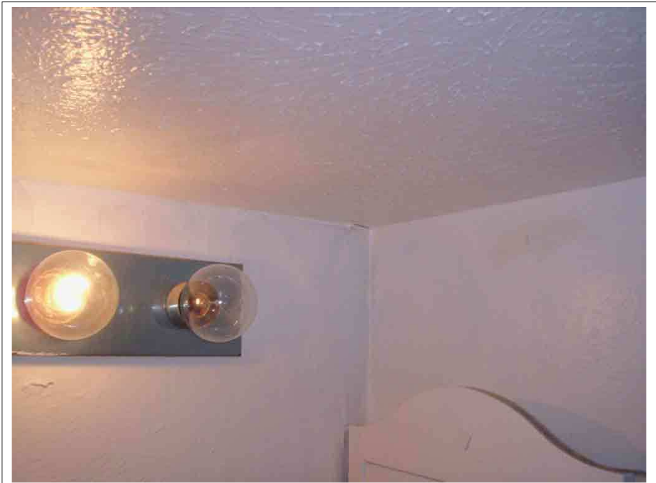
30. Comments: unit 109- moisture intrusion evidence H&S
