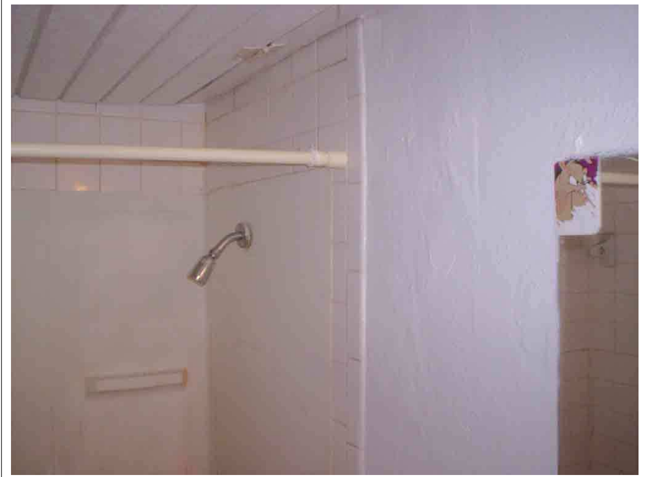
25. Comments: unit 106 moisture intrusion wall and ceiling H&S
