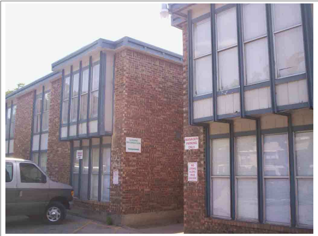
7. Comments: Bldg 3 & 4- rot/moisture damage at siding/trim (upper overhanging window features)
