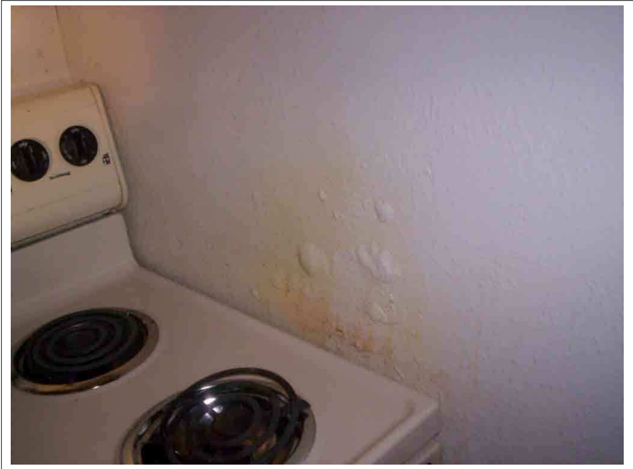
31. Comments: unit 119- heat damaged wall adjacent stove- H&S
