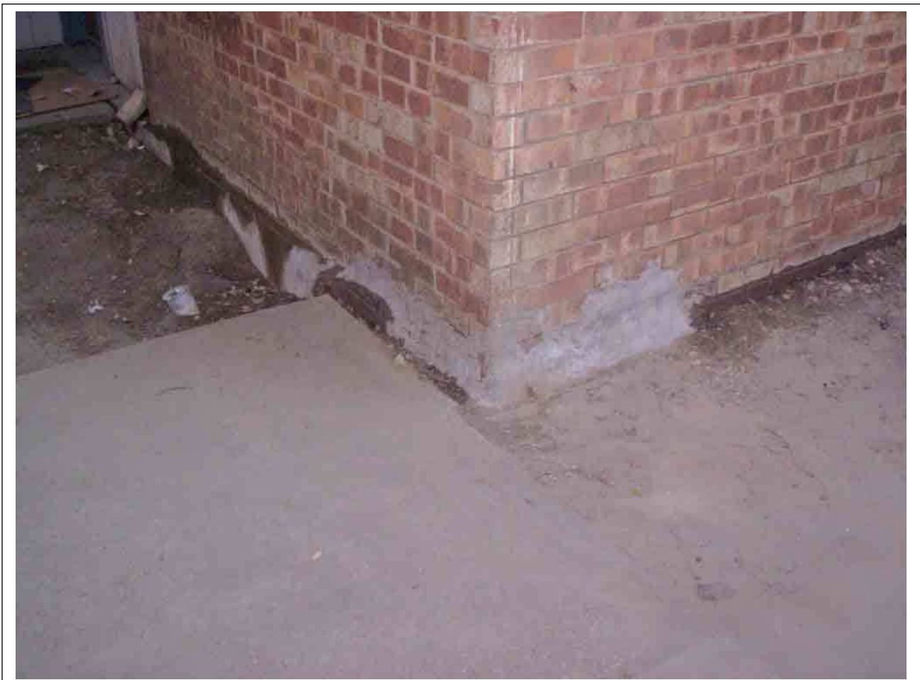
12. Comments: moisture seepage from within building- example 3
