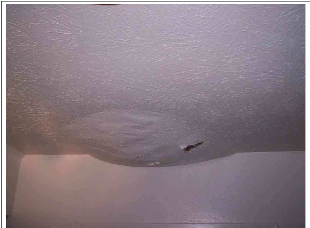
34. Comments: unit 123- moisture intrusion evidence
