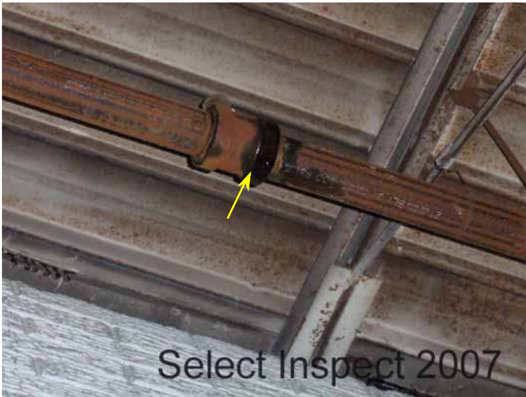
↑ suspected leakage evidence at fire sprinkler piping at the warehouse.
