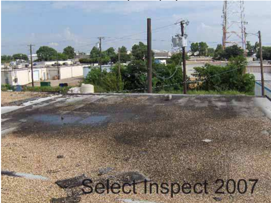
↑ northeast roof- pooling water and poor drainage conditions
