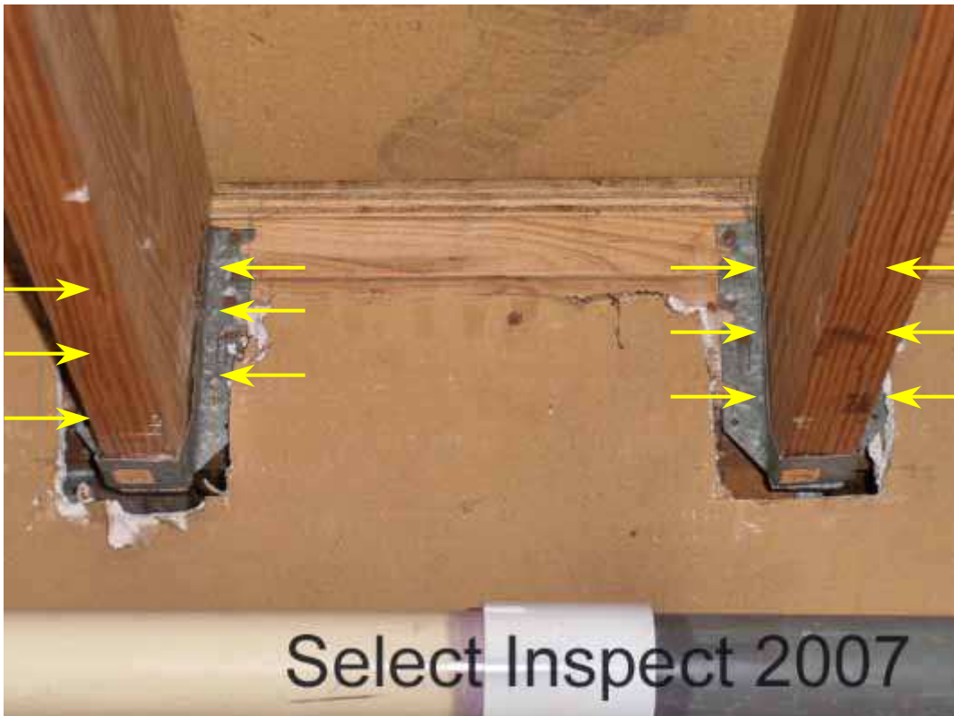
↑ Joist hangers were incorrectly fastened at the downstairs mechanical closet Hangars should be fit to the related framing; and all nail openings should be filled with appropriate fasteners.- fasteners were missing at joist connections
