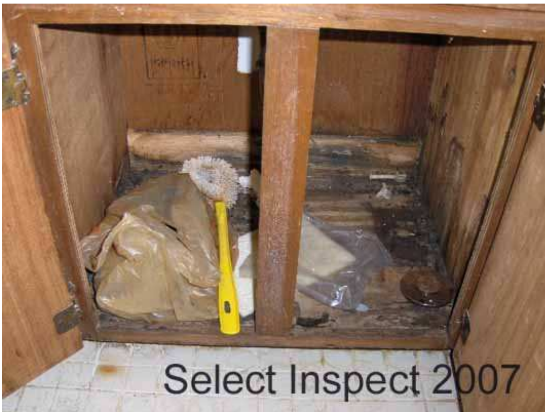
↑ moisture intrusion, fungus, and decay (rot) below men's bathroom sink
