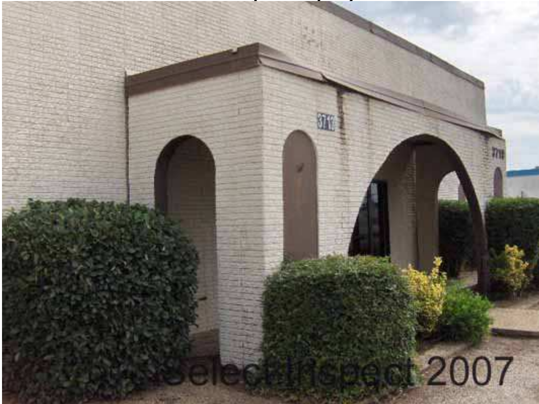
↑ porch feature at unit xxxx leaning from structure, amiss / deficient roofing and flashing.
