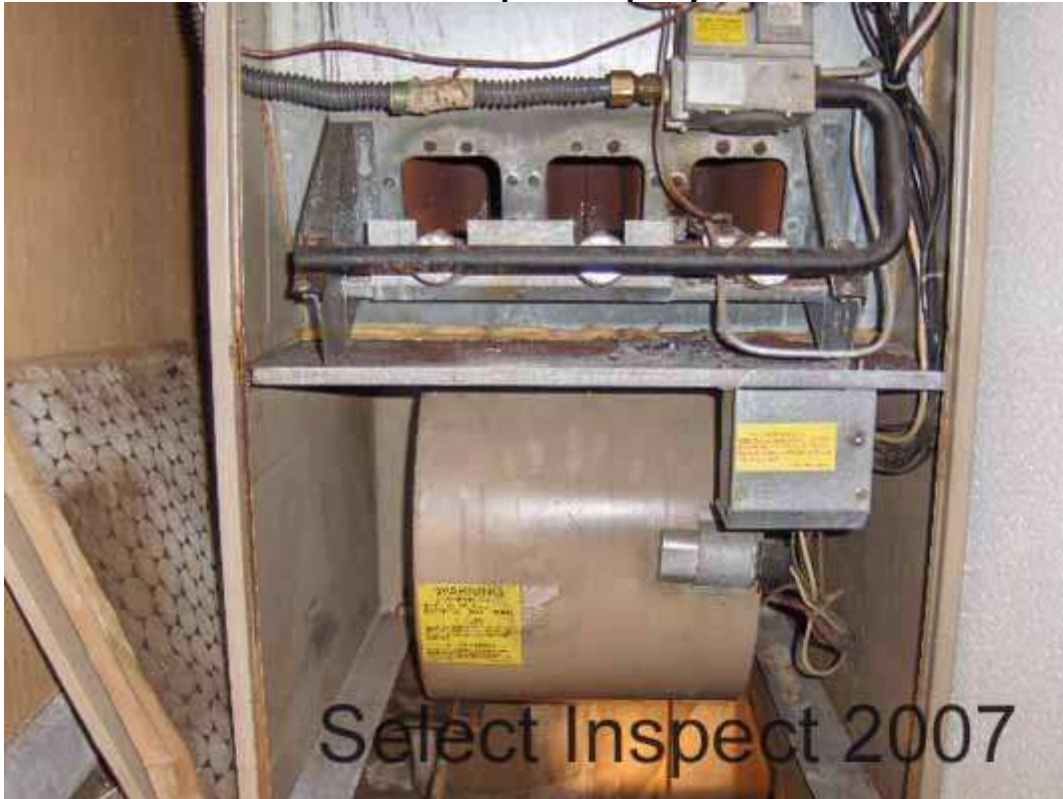
↑ HVAC interior system- typical corrosion and aged components- Reinstall heat shield (was next to the unit at the time of inspection) and monitor this item periodically; maintain as needed
