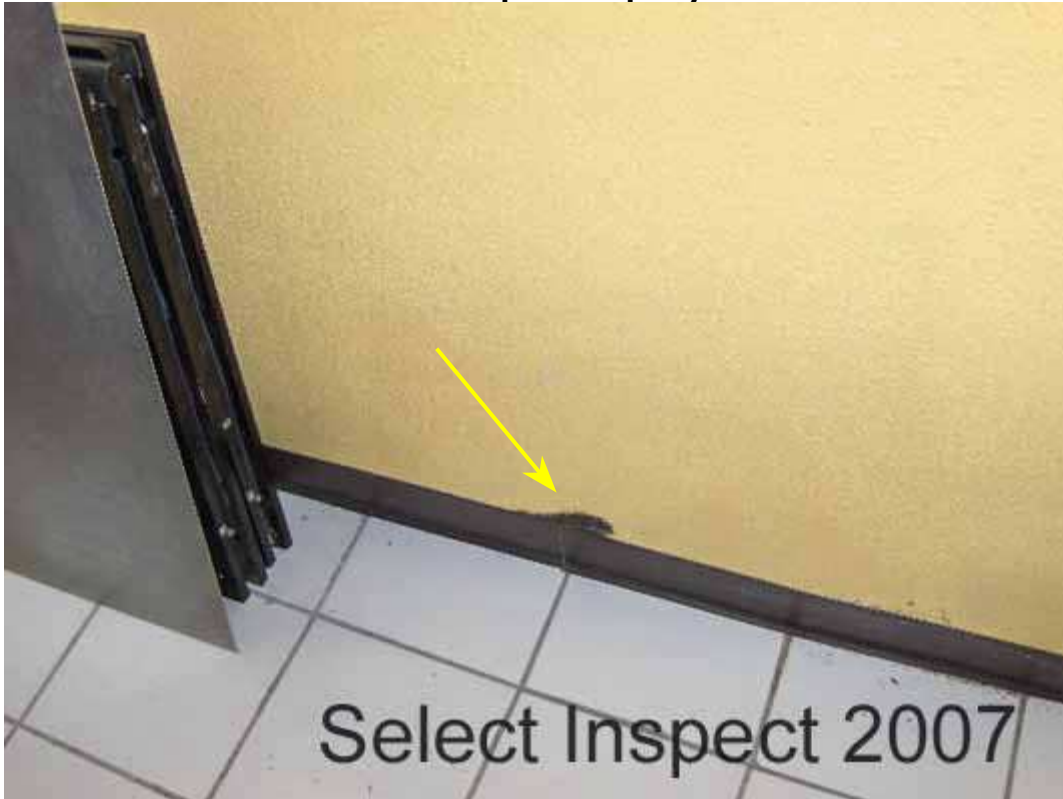
↑ moisture intrusion / fungus discovered at central right clean room- north wall and adjacent wall in the room to the north of this location
