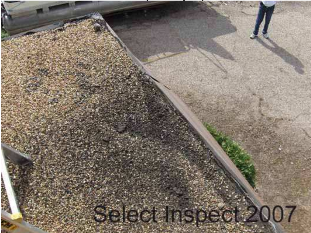
↑ southeast corner of xxxx porch – sunken and amiss flashing, deflection, suspected rot of supporting framing
