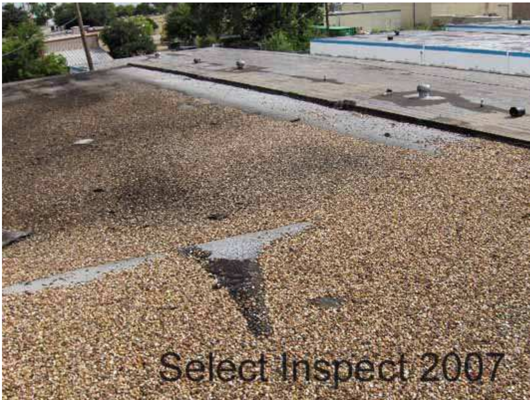
↑ example roof surface- bulges, and exposed fiberglass mat
