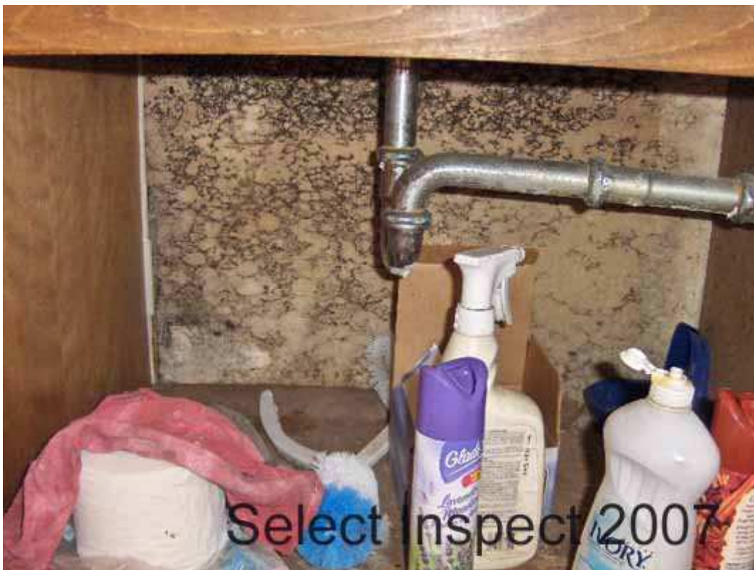
↑ moisture intrusion / fungus at men's sink right side bathroom unit xxx
