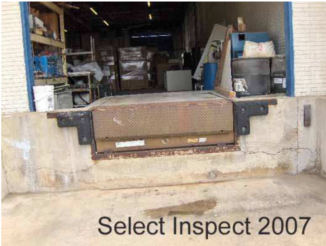
↑ foundation stress at loading dock- Monitor this item periodically and maintain as needed.
