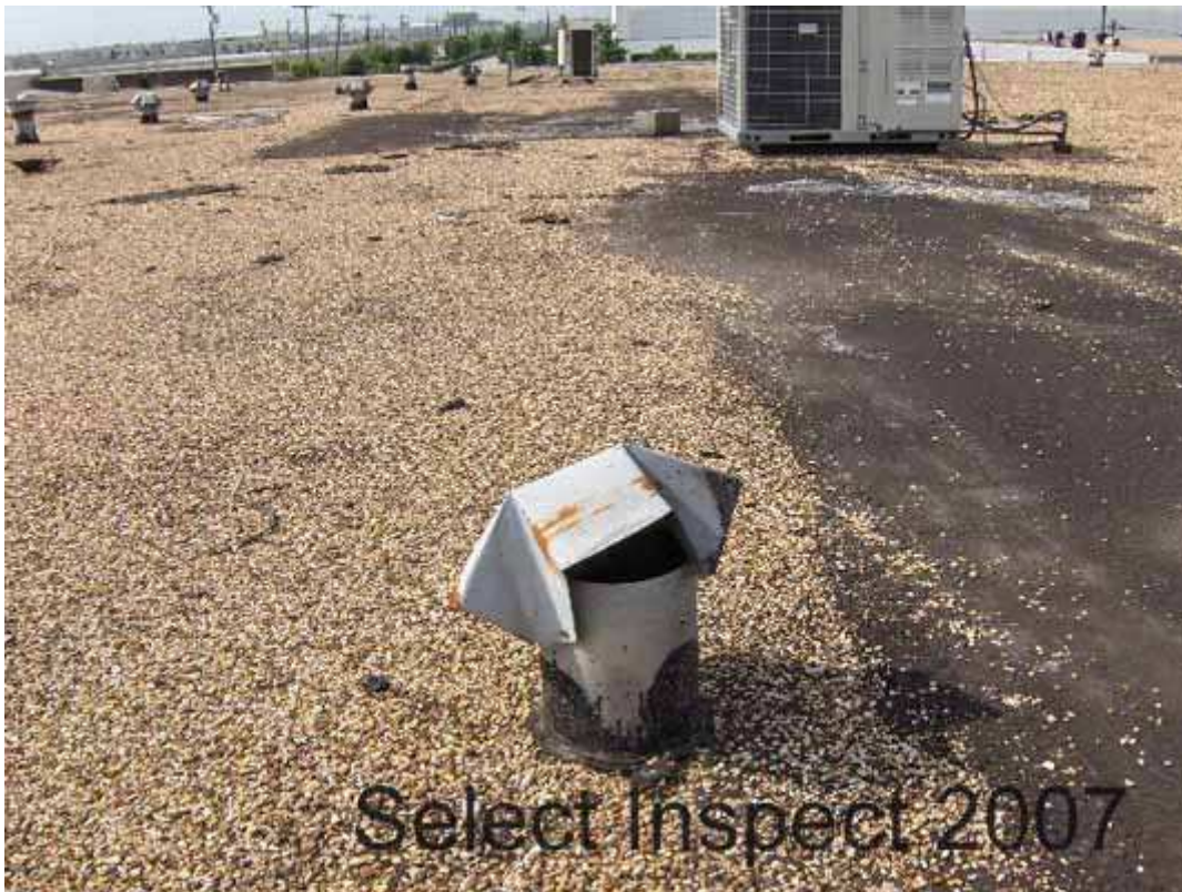
↑ amiss / deficient roof vent cap- may allow moisture intrusion
