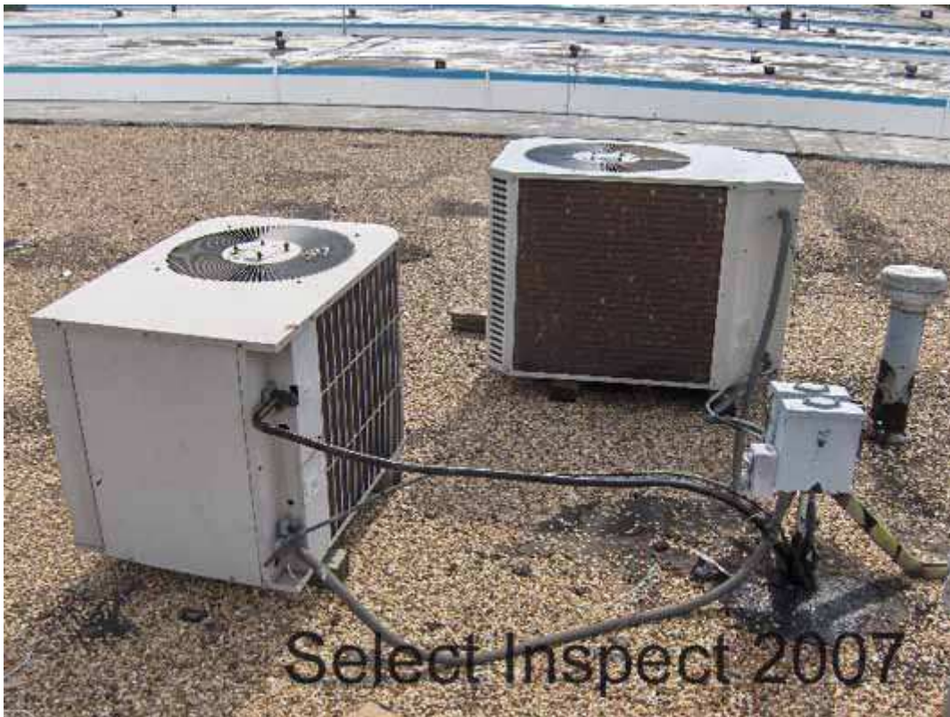
↑ example- air-conditioner condensers and related equipment
