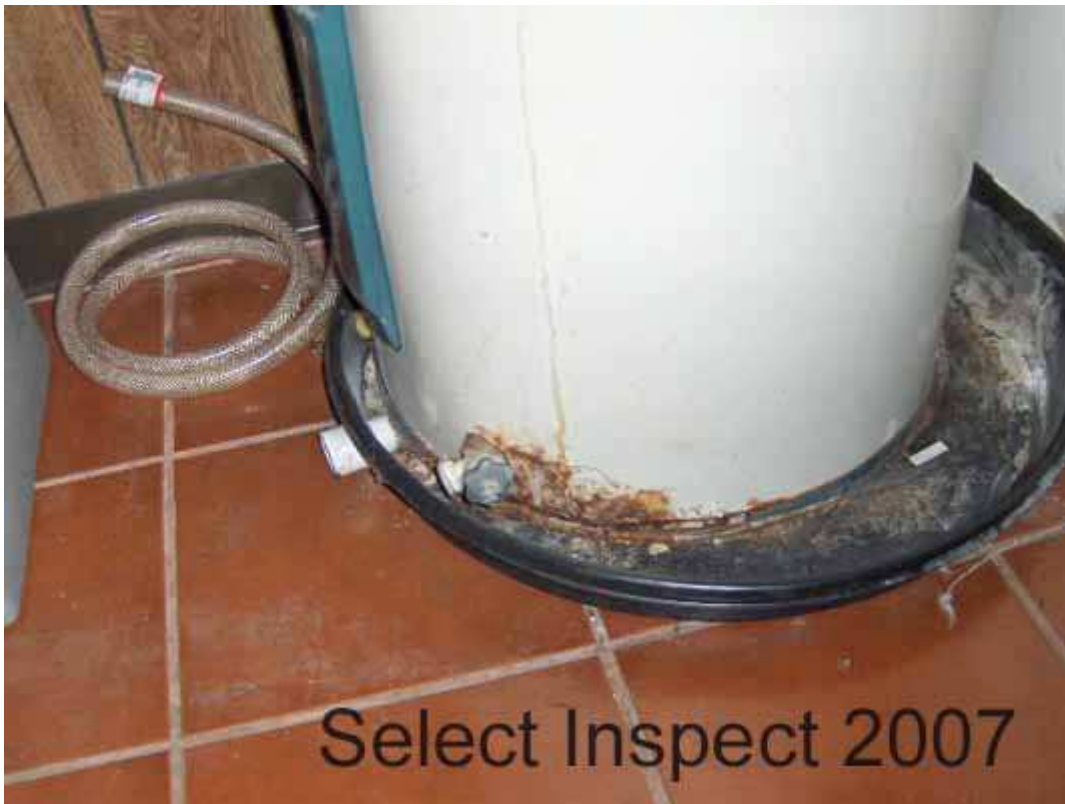
↑ excess corrosion at water heater
