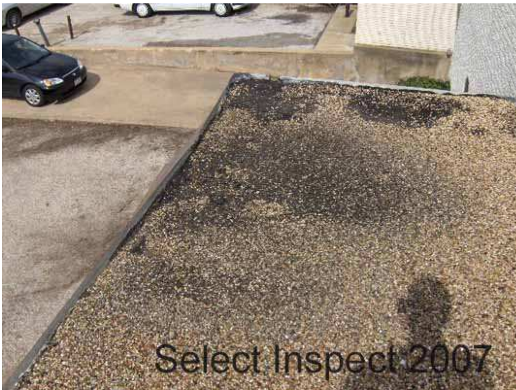
↑ southwest corner of xxx porch – sunken and amiss flashing, deflection, suspected rot of supporting framing
