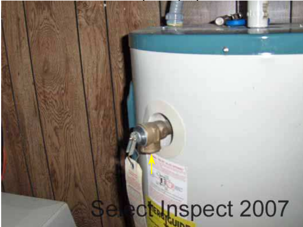
↑ temperature-pressure-relief missing a drain pipe extension to an appropriate exterior termination point
