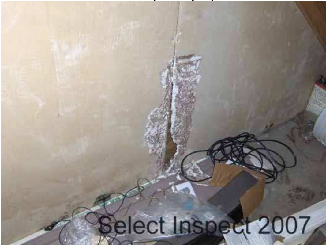
↑ evidence of Prior subterranean termite activity under stairway
