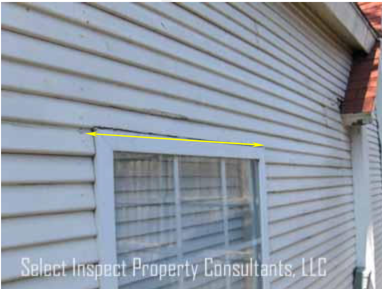
↑ missing flashing above windows & doors; example at window
