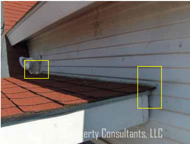
↑ missing flashing; kick-out-flashing; at ramp entry roof
