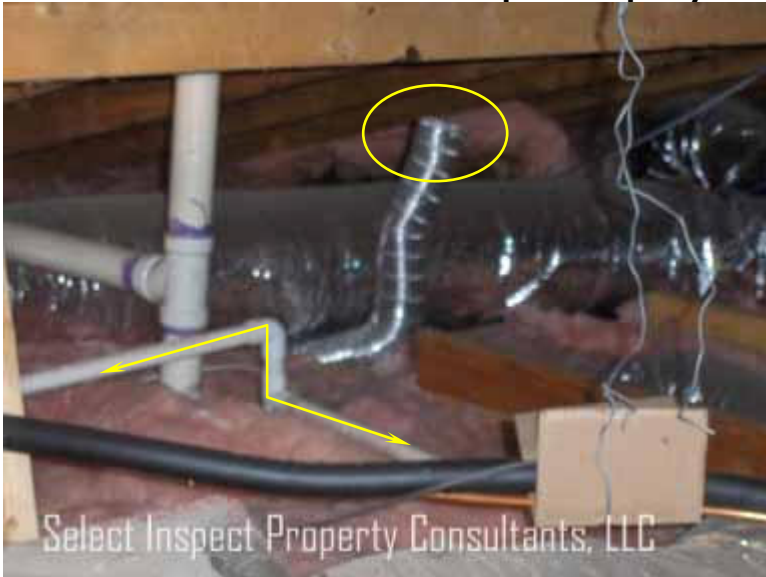
↑ exhaust fan(s) improperly terminate in the attic, rather than exterior & unworkmanlike routing of air conditioning condensate drains
