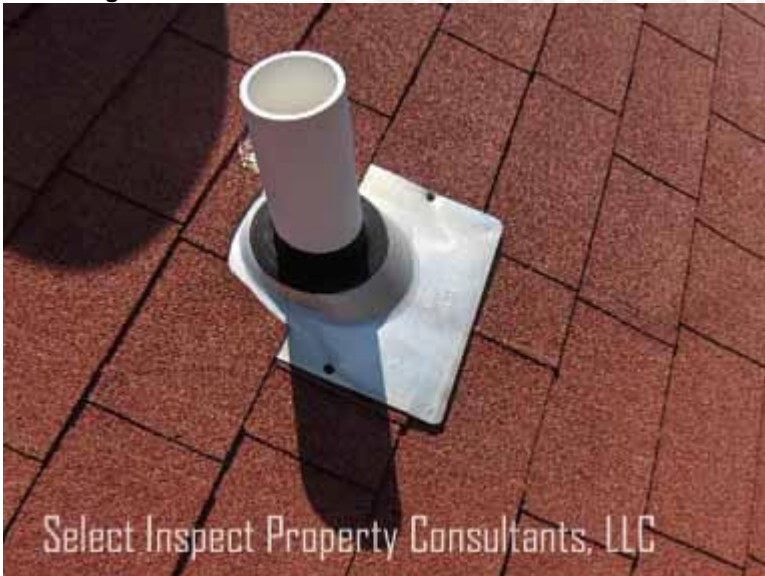
↑ uncaulked, exposed fasteners & unpainted vent stack; example
