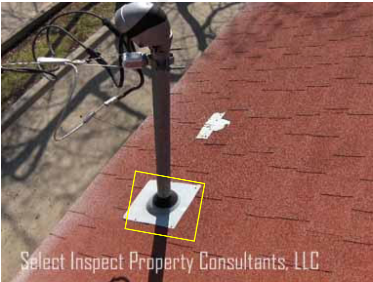
↑ unworkmanlike electrical mast penetration & flashing boot
