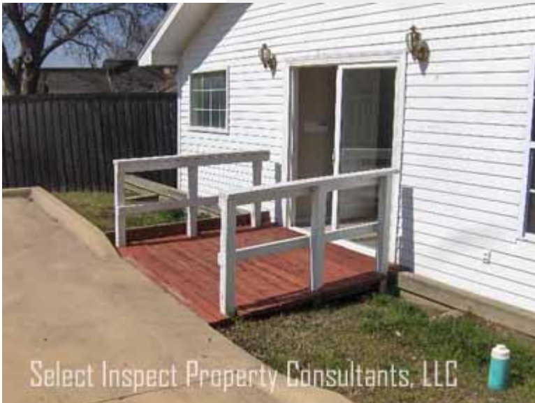
↑ handicapped door was not wide enough
