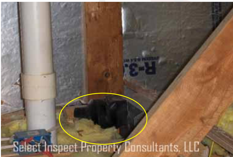
↑ exhaust fan(s) improperly terminate in the attic, rather than exterior ; example
