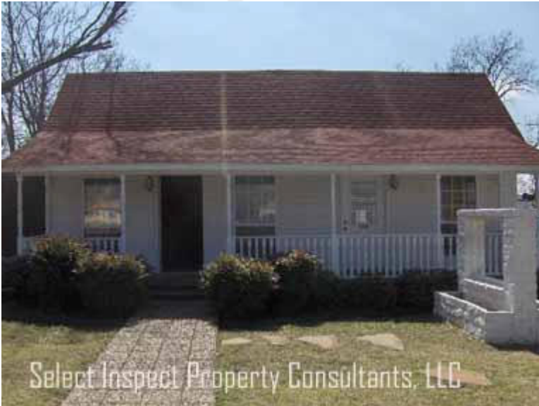
↑ deflection at front porch roofline
