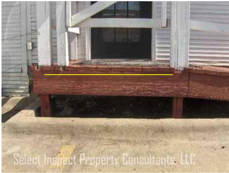
↑ ramp platform was not level
