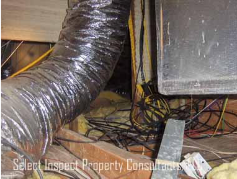
↑ multiple deficiencies at HVAC; example
