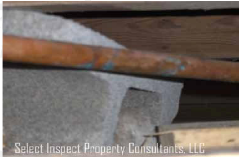
↑ unworkmanlike broken block support under beams
