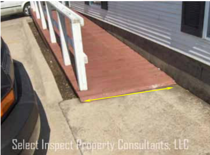
↑ lip at ramp is too high/steep
