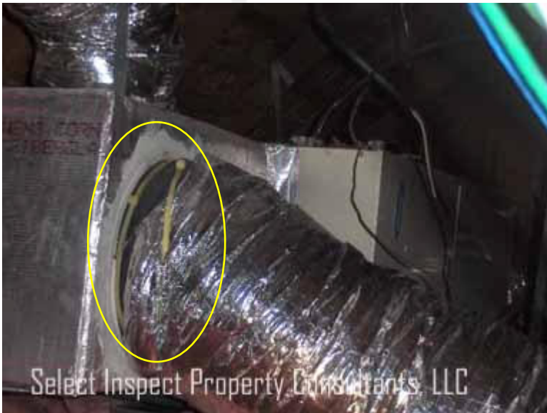
↑ amiss air duct connection to plenum; example
