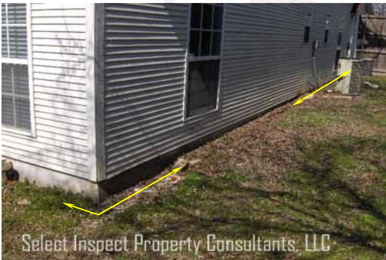
↑ deficient grading; example
