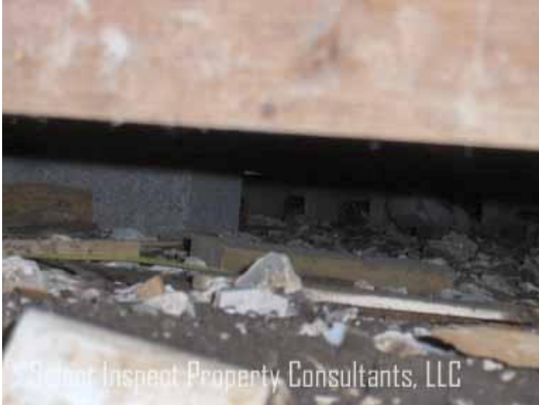
↑ low clearance in crawl space; wood-to-ground debris; inaccessible
