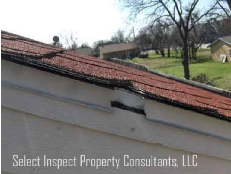
↑ minor damage at rake shingles & missing drip edge flashing; 7043
