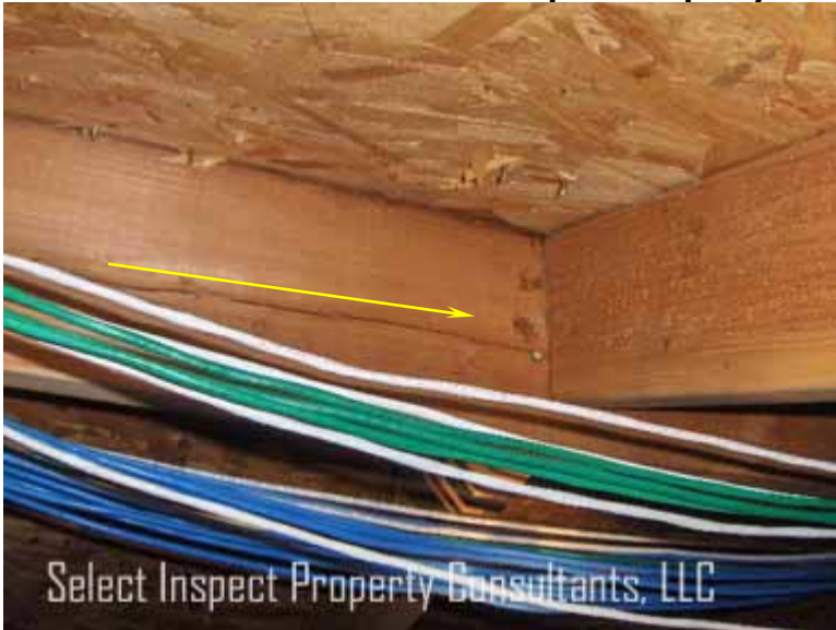
↑ example cracked framing in attic
