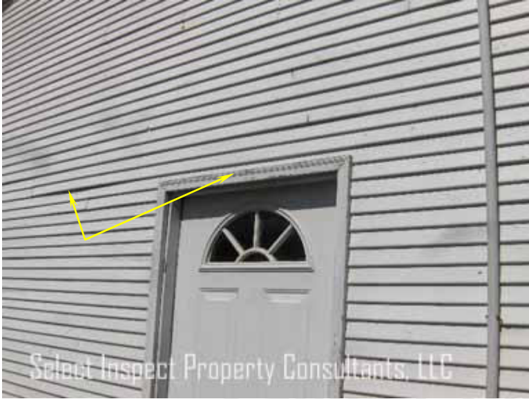
↑ wavy siding & missing flashing above door
