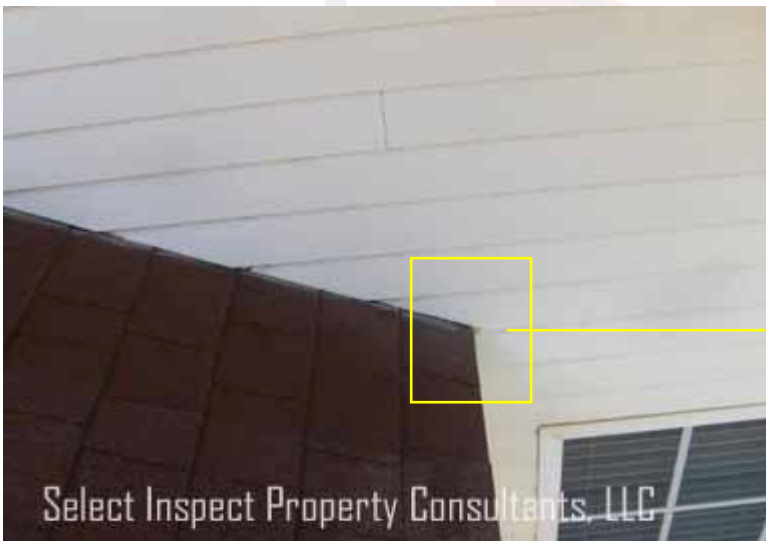
↑ missing kick-out-flashing; example
