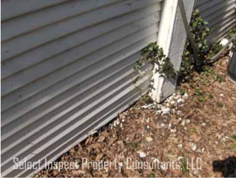
↑ high soil; low siding; prone to wood destroying insects & decay
