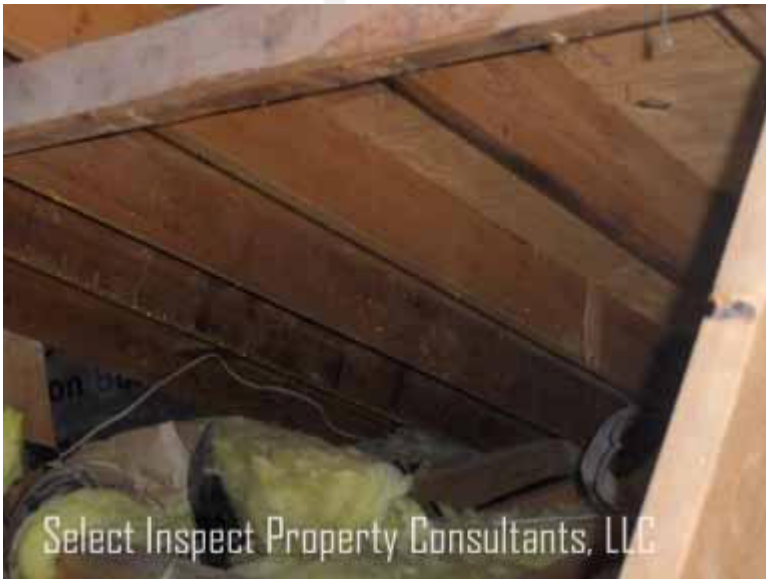
↑ deficient insulation; example
