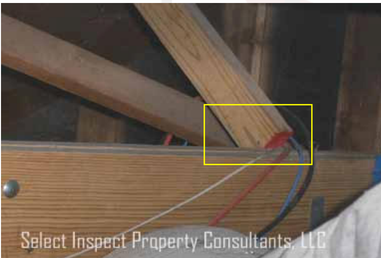
↑ unworkmanlike strut connection to attic beam; example
