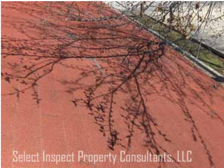
↑ tree damaged shingles
