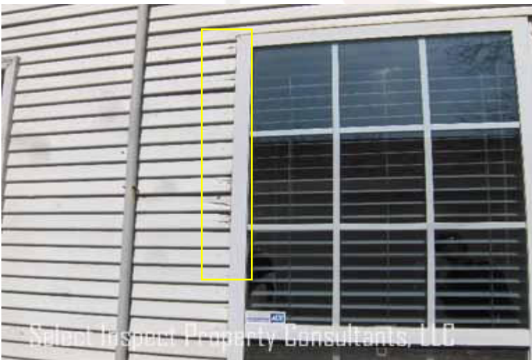
↑ moisture damage at siding adjacent window; example
