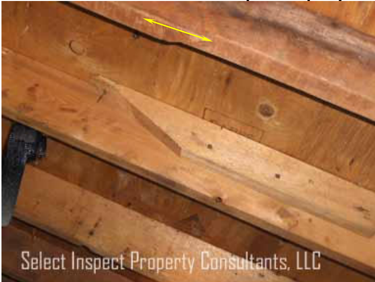
↑ cracked attic framing; example
