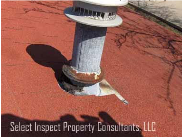
↑ corroded flue component(s); flues had been abandoned & could be removed
