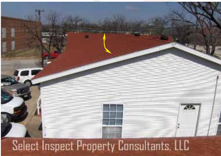
↑ deflection noted at roof
