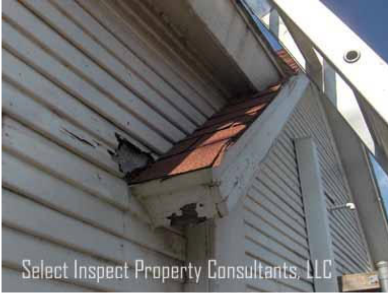
↑ amiss flashing & moisture damage; east wall
