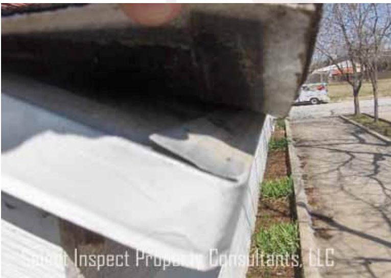
↑ deficient drip edge flashing corner; example
