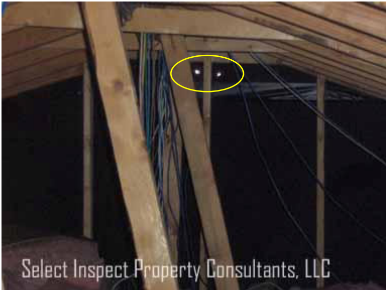
↑ daylight seen from attic; small holes at gable wall; 7075 south
