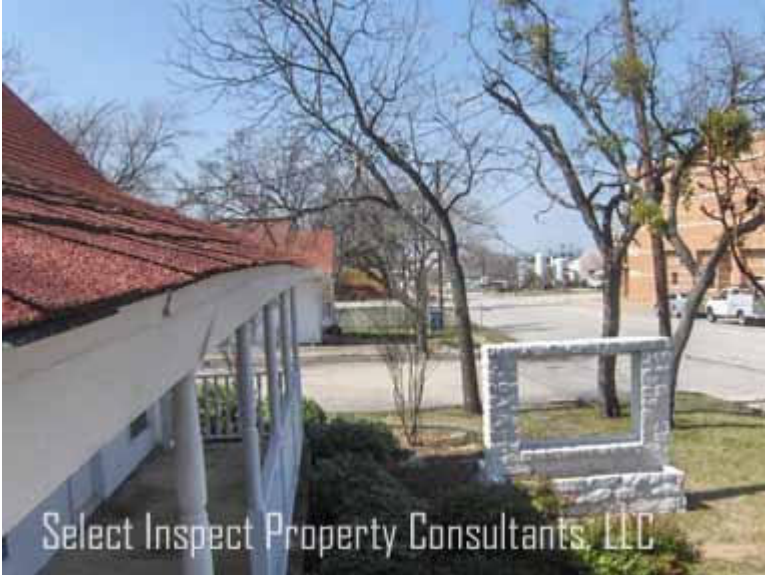
↑ deflection at front porch roofline
