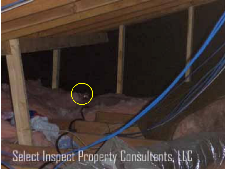
↑ daylight seen from attic; small hole at gable wall; 7075 south
