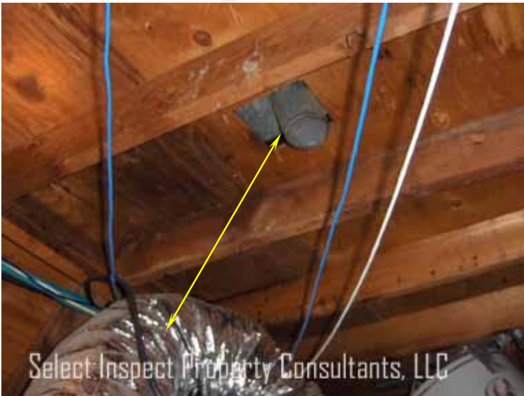
↑ crimped air ducting; example & abandoned furnace flue
