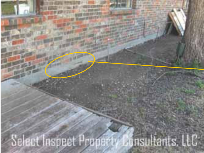
↑ spalling concrete & exposed corroding reinforcement steel at the west.
