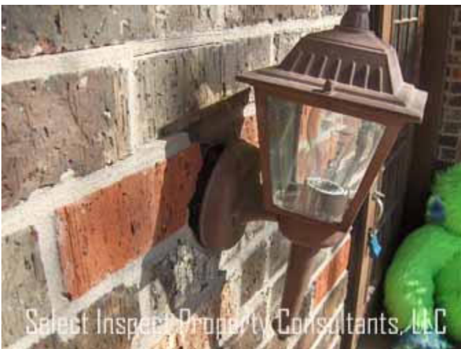
↑ inadequately secured electrical at exterior; example
