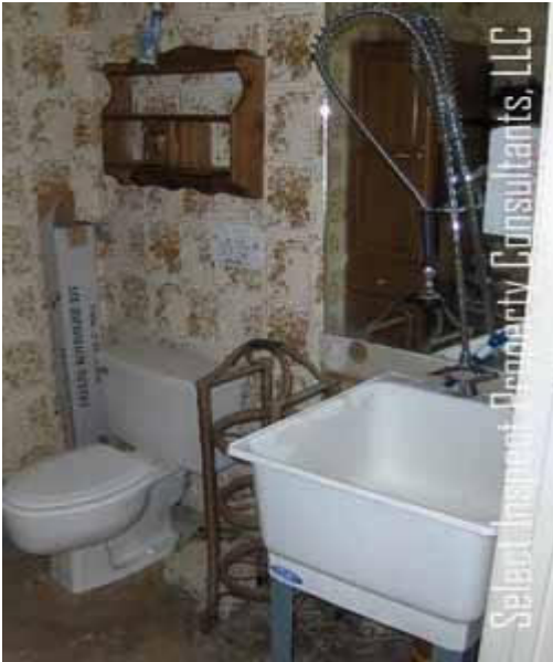
↑ moisture damage & fungus below west bathroom sink & along the wall; may be from adjacent leaking toilet
