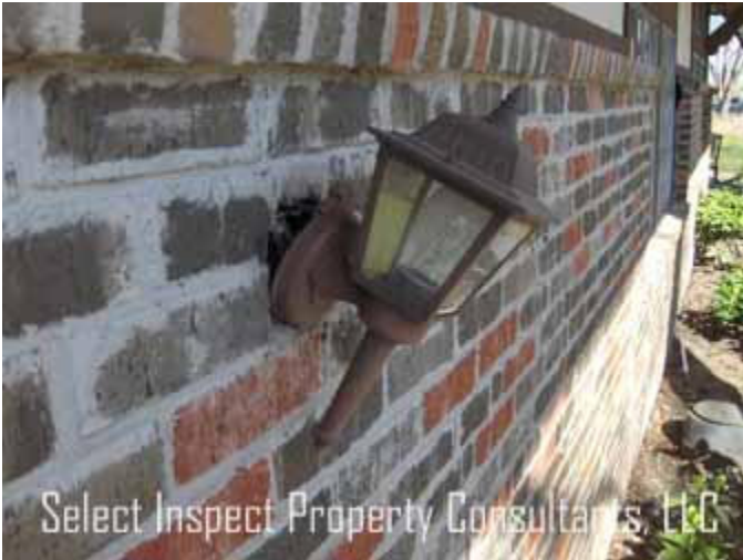
↑ inadequately secured electrical at exterior; example
