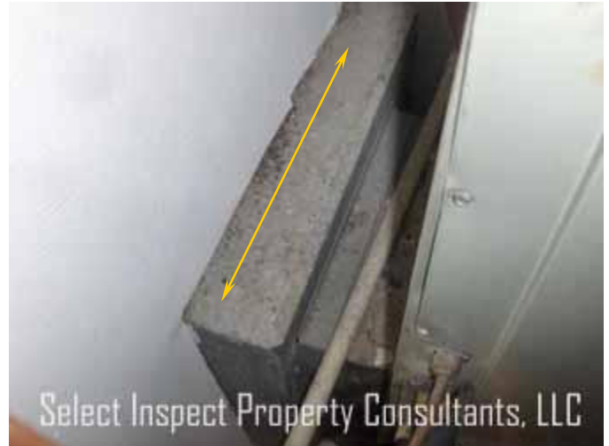
↑ rodent/pest droppings present at the HVAC equipment; unsanitary
