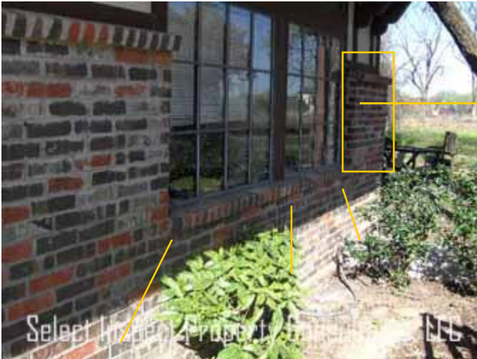
↑ brick & or mortar cracks & stress separation at the east-northeast
