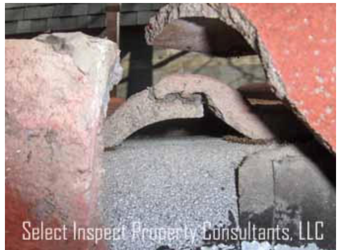
↑ damaged roof tiles; openings will allow moisture intrusion
