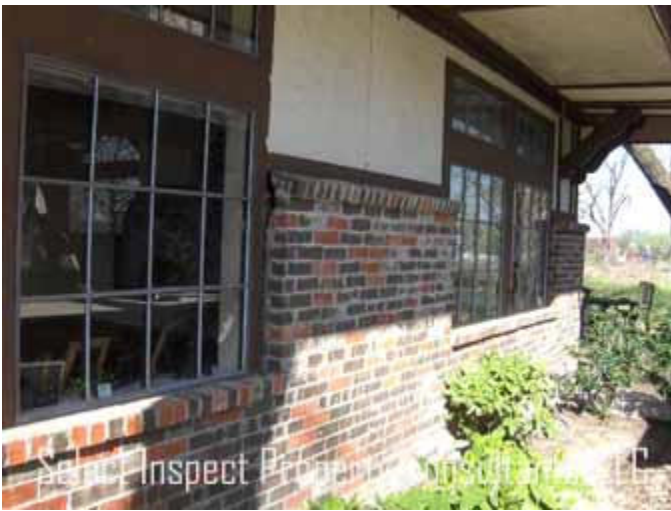
↑ excess stress & rodent opening at the east
