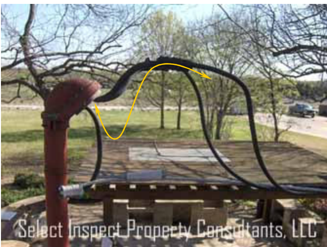
↑ inadequate drip loop at electrical service; to prevent rain dripping into the electrical mast head & conductors
