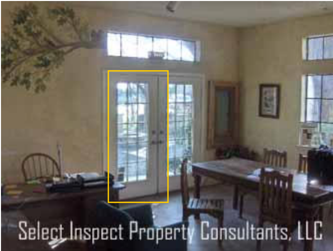
↑ left door was not functioning as intended; various stress cracks noted throughout the interior
