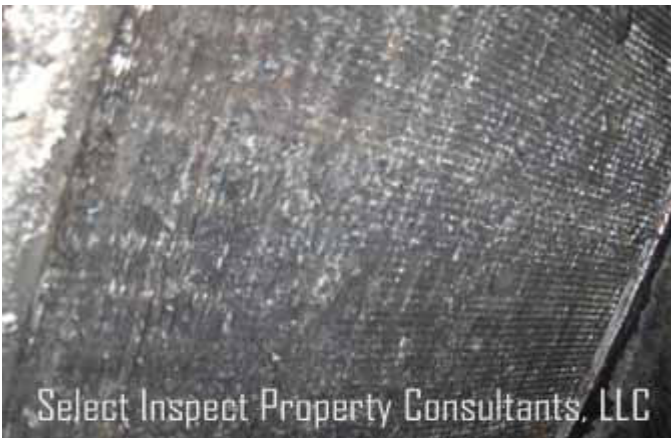
↑ evaporator(s) coils were filthy; congested
