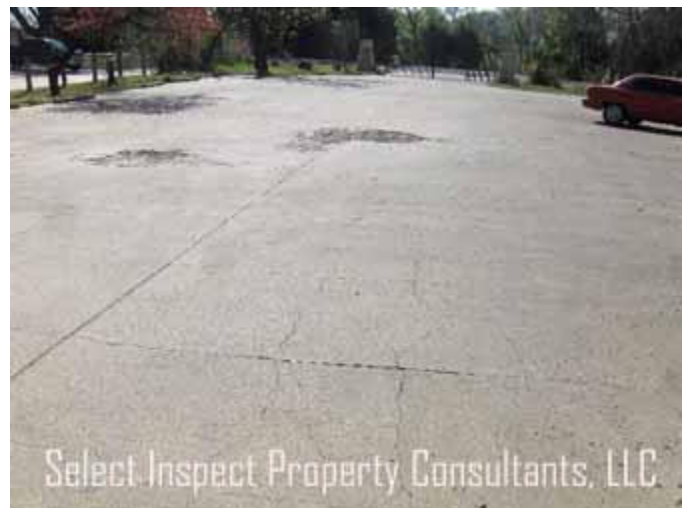
↑ potholes at entry drive
