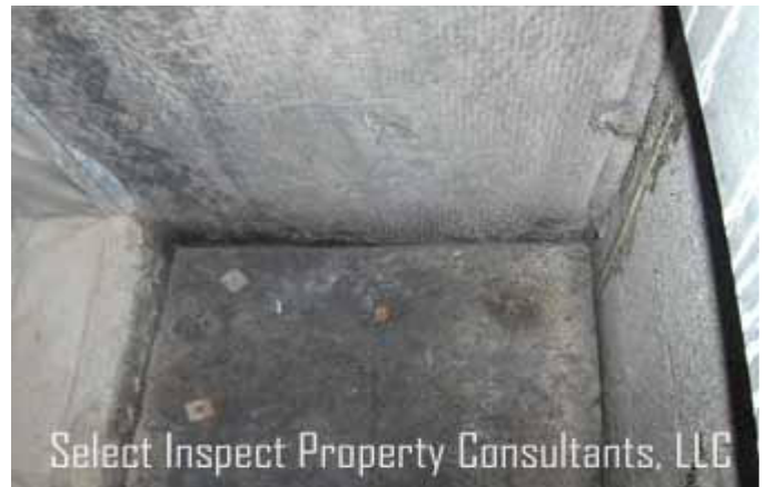
↑ HVAC plenum was dirty
