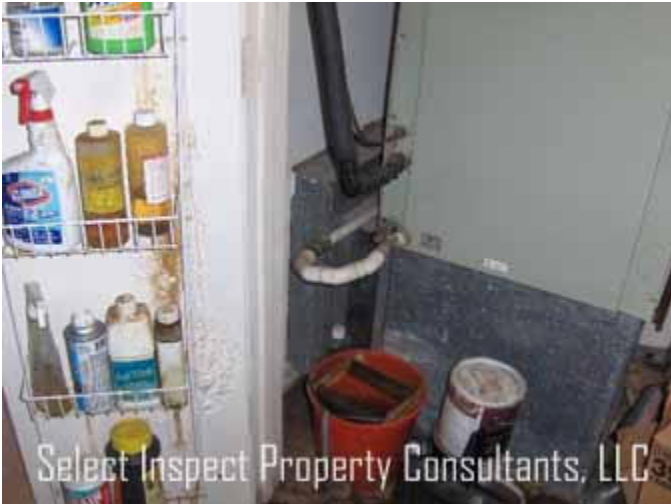
↑ do not store chemicals in the HVAC plenum/mechanical closet area
