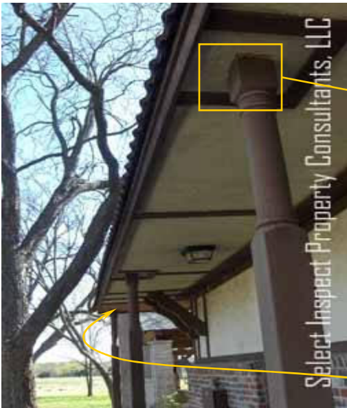
↑ separation & differential movement at rear porch columns
