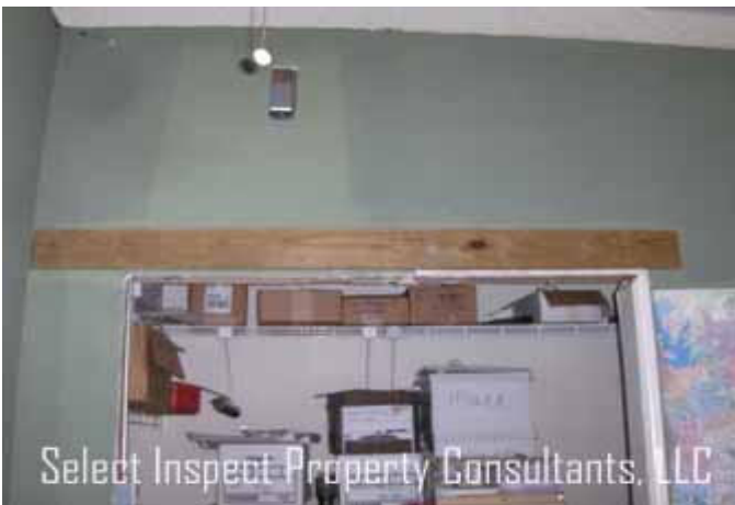
↑ unworkmanlike modification of wall structure at east office/study
