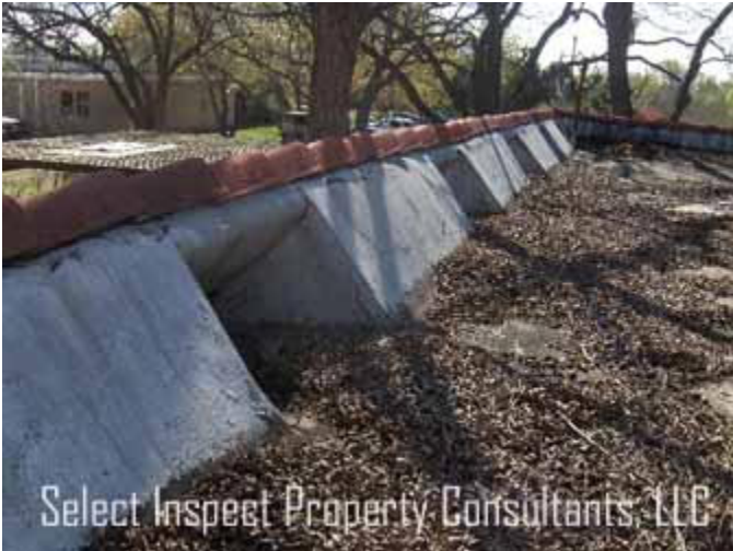
↑ roof scuppers were not functioning as intended, congested & deficient; excess debris
