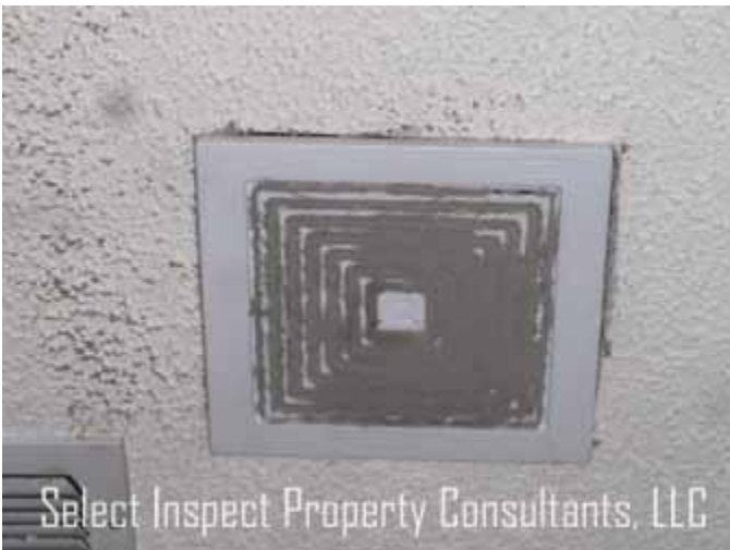
↑ congested exhaust fan(s) is a potential fire hazard if the motor overheats
