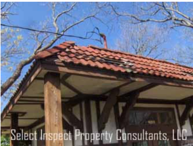
↑ aged roof tiles; many missing & damaged
