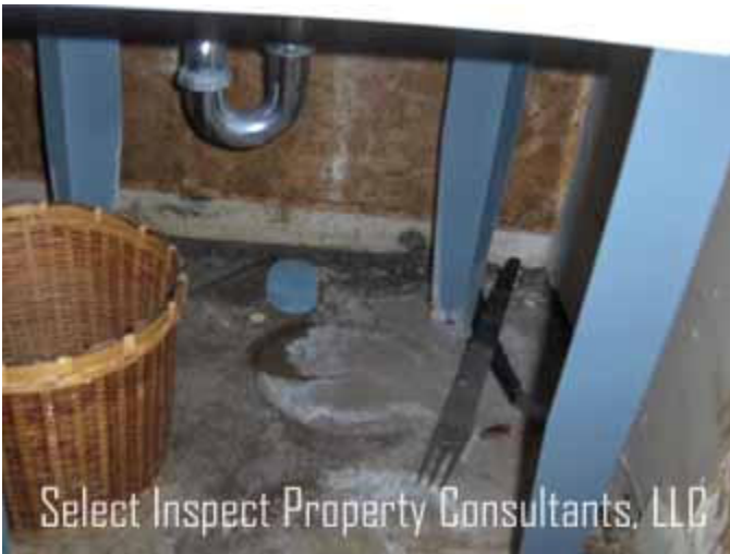
↑ moisture damage & fungus below west bathroom sink
