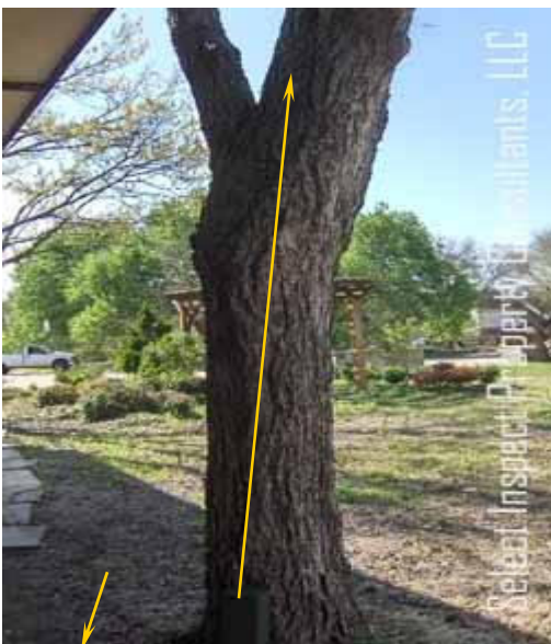
↑ tree light electrical should be secured & in conduit for at least 8 feet from grade; & the conduit on the soil was unprotected from foot traffic/damage
