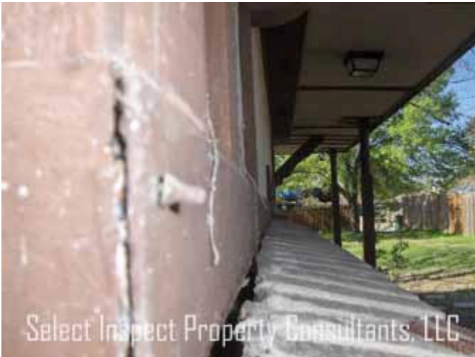
↑ excess stress separation at the northeast.
