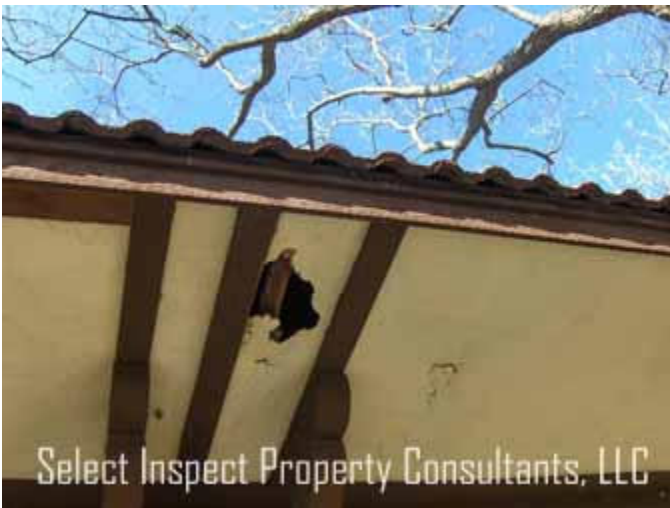
↑ rot & or rodent opening at east eave
