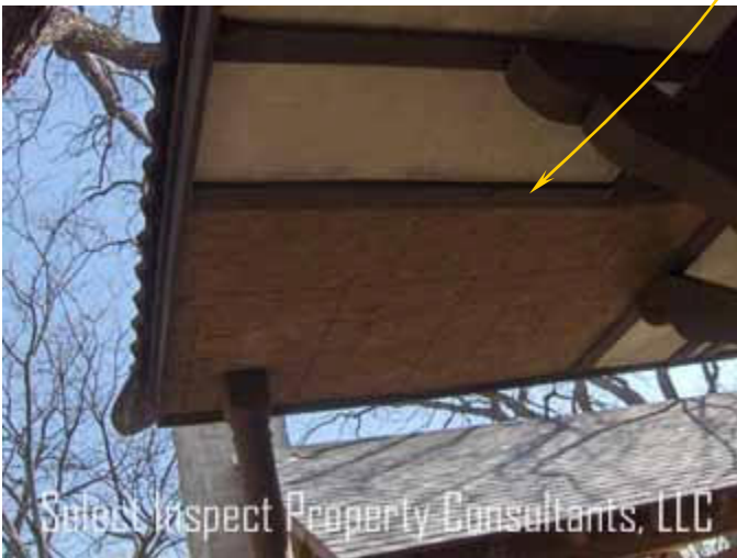
↑ repair of eave; likely rot history
