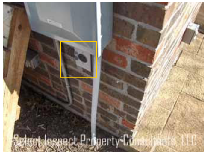
↑ missing exterior electrical receptacle cover example
