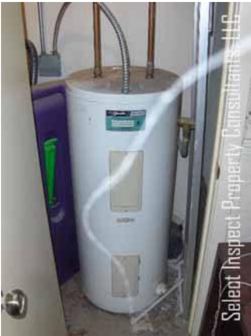
↑ antiquated water heater; no auxiliary pan & drain.
