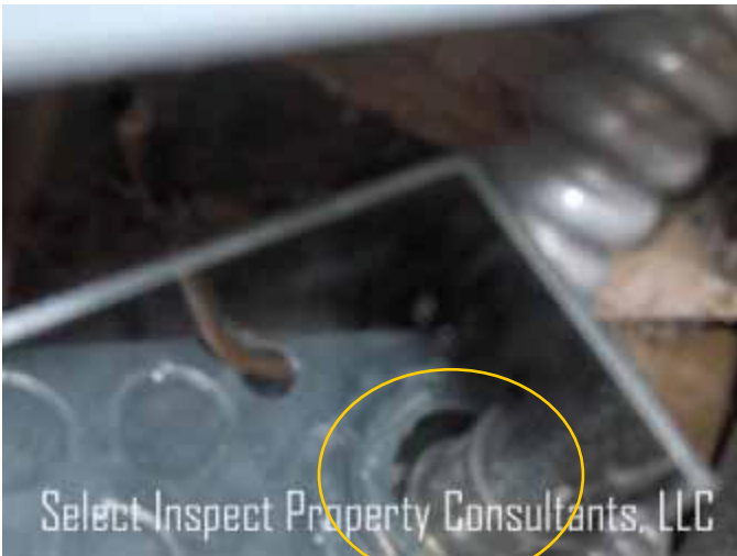
↑ unworkmanlike electrical in interior service panel; deficient conduit connection
