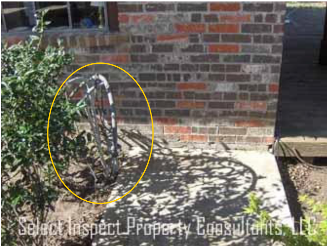
↑ abandoned electrical at the northeast; these were not energized during the inspection.
