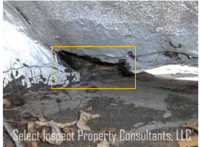
↑ opening at scupper flashing will allow moisture intrusion; example
