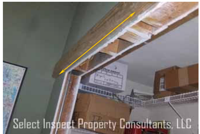
↑ cut framing with unworkmanlike "intended header"; close view of image at left
