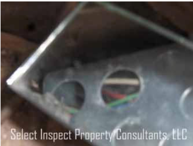
↑ unworkmanlike electrical at interior service panel; missing bushings at knock-outs.
