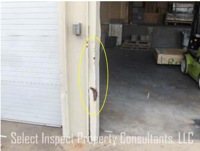
↑ exposed steel/metal at exterior should be cleaned of loose paint & rust then painted to resist corrosion; example at the west shop doorway
