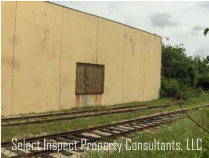
↑ stress cracks & deteriorating concrete & steel
