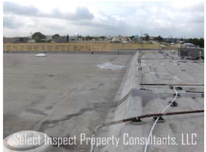
↑ air conditioning condensate should drain off, rather than be allowed to pool on the roof.
