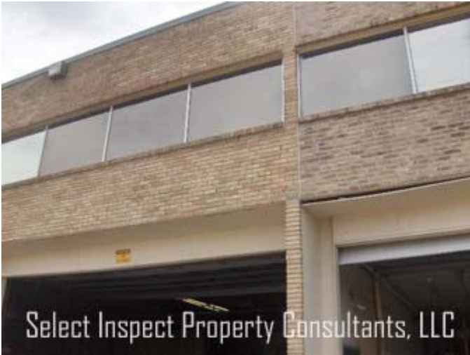
↑ cracked windows discovered at the gallery
