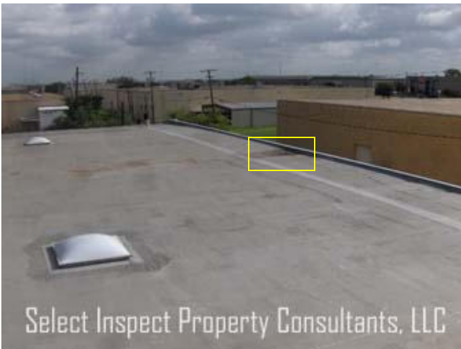
↑ rear (east) warehouse scupper is not at obvious low point to receive rain water for disposal
