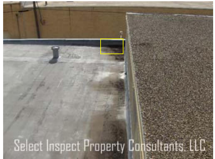
↑ water runs to the east & does not immediately run off; consider adding a scupper at this location.
