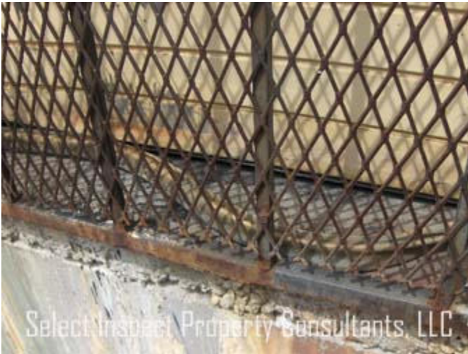
↑ deficient weatherstrip at east dock door
