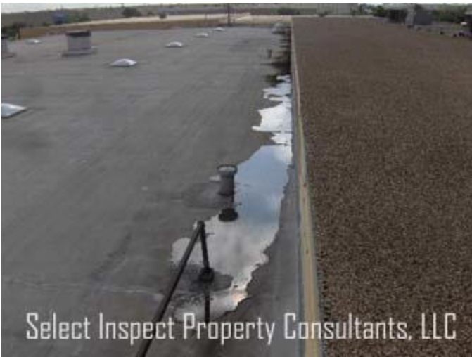
↑ inadequate slope at junction of warehouse & conditioned warehouse roofs
