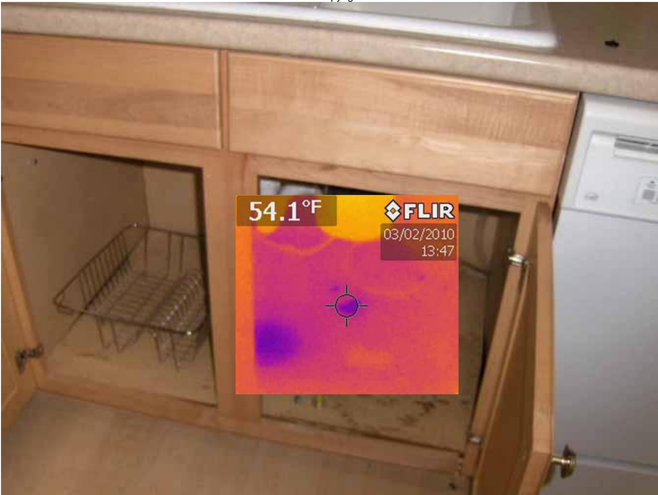
↑ moisture staining evidence & leakage history below the kitchen sink at 7043
